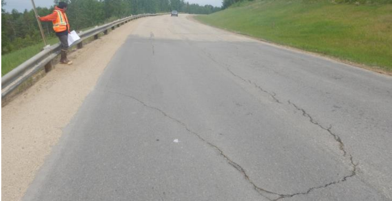
Photo No. 7 – Reflective Diagonal Crack at the north end of the Mid-Hill Slope Section
