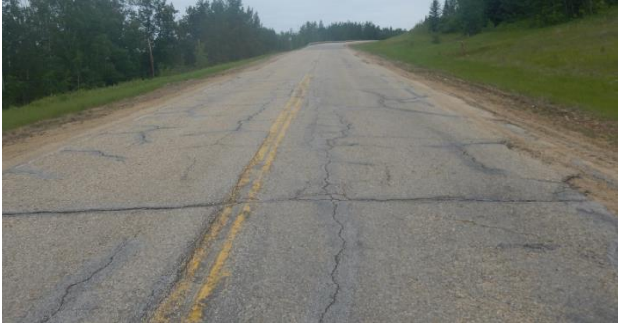
Photo No. 3 – Looking north at multiple open longitudinal cracks in the highway surface between the MH#1 location and the Mid-Hill slope section
