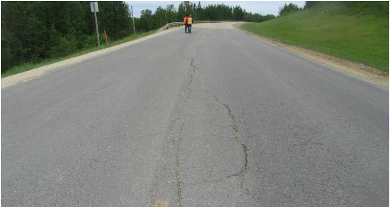
Photo No. 6 – Reflective Longitudinal Cracks at the Mid-Hill Slope Section (looking north)
