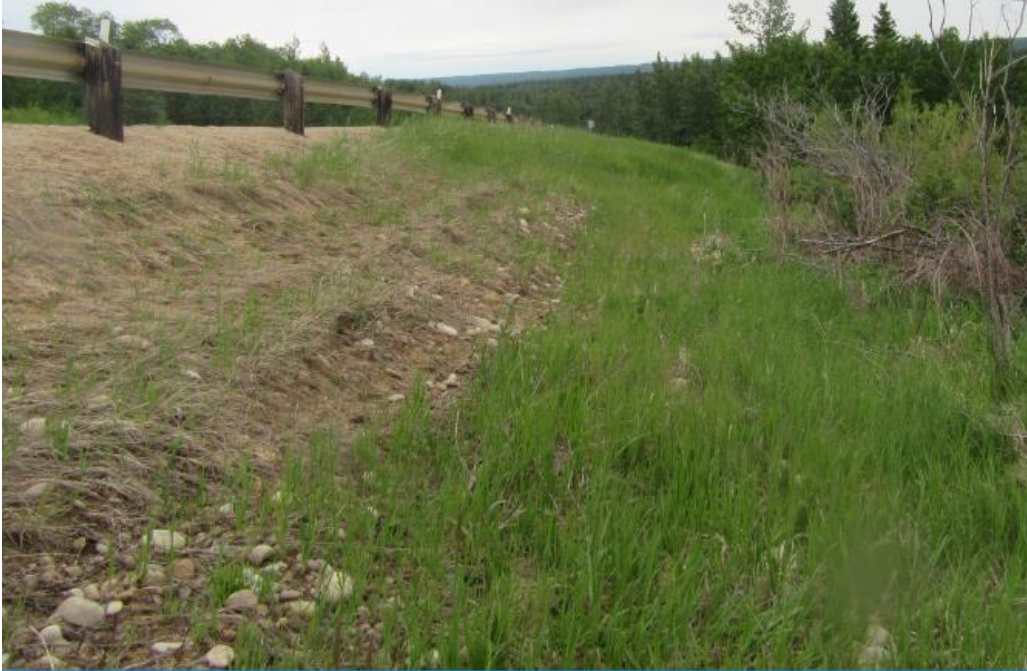
Photo No. 9 – Looking south at graben back scarp
