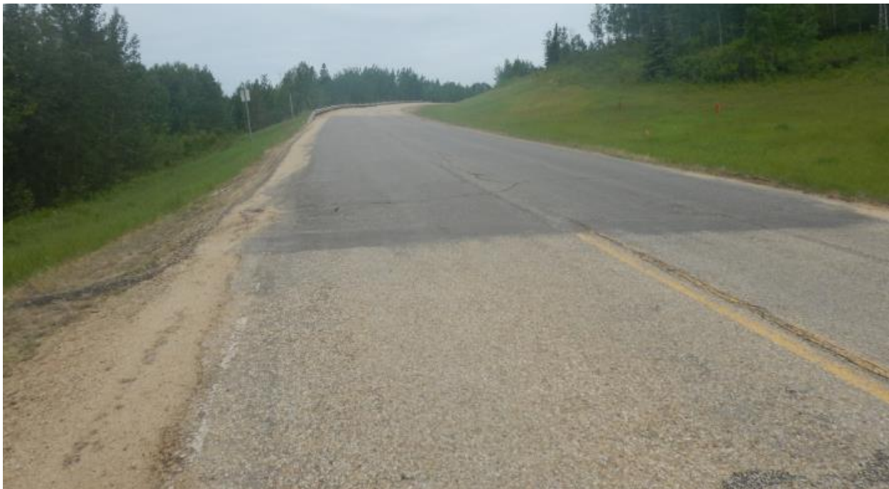
Photo No. 4 - Looking North at 2017 ACP Patch placed over the Mid-Hill Slope Section
