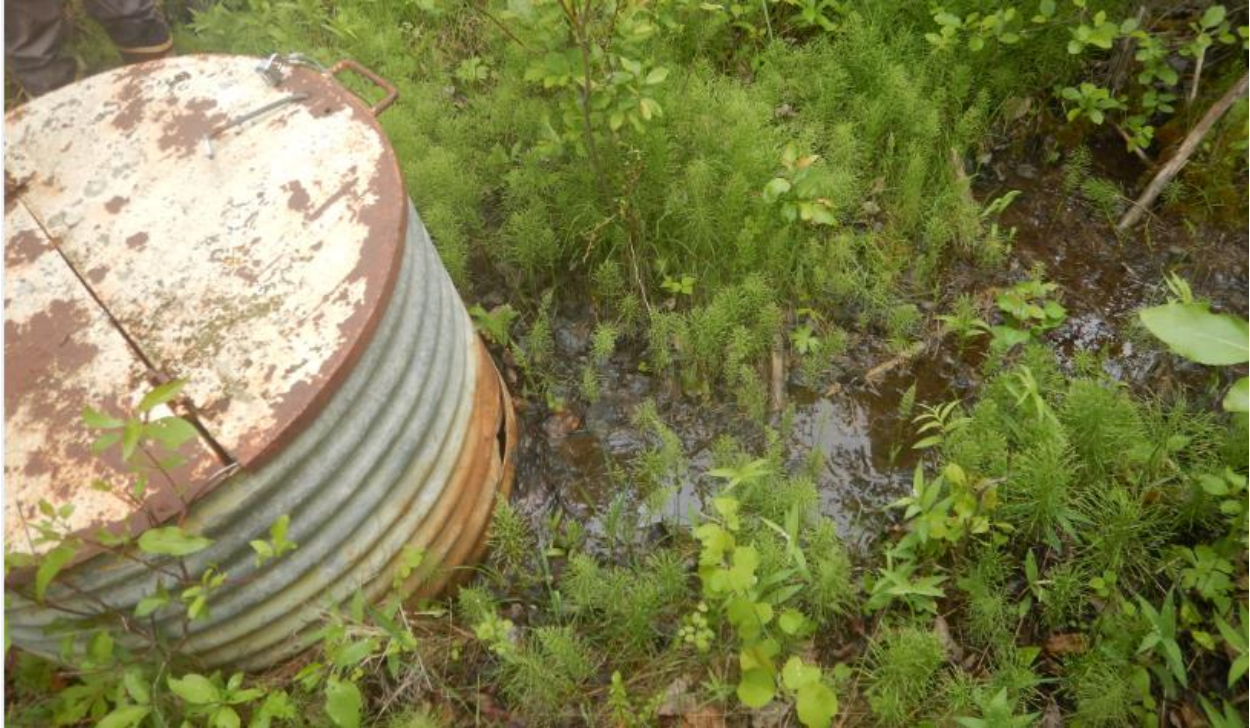
Photo No. 1 – Seepage and standing water near MH#1
