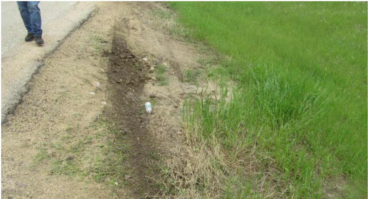
Photo No. 2 – Looking at the slight drop/settlement development near the edge of the road
