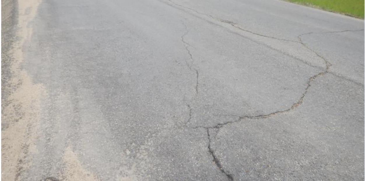
Photo No. 5 – Reflective diagonal crack at the southern limit of Mid-Hill Slope Section (looking northeast)
