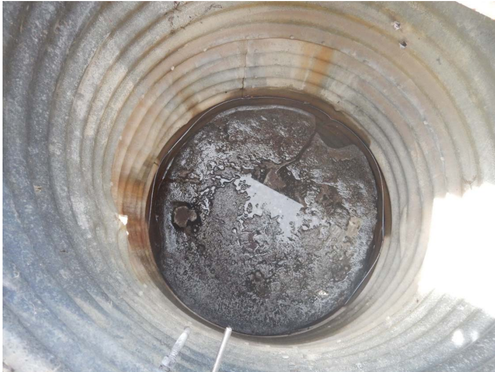
Photo No. 1 – Standing water and ice inside MH#1
