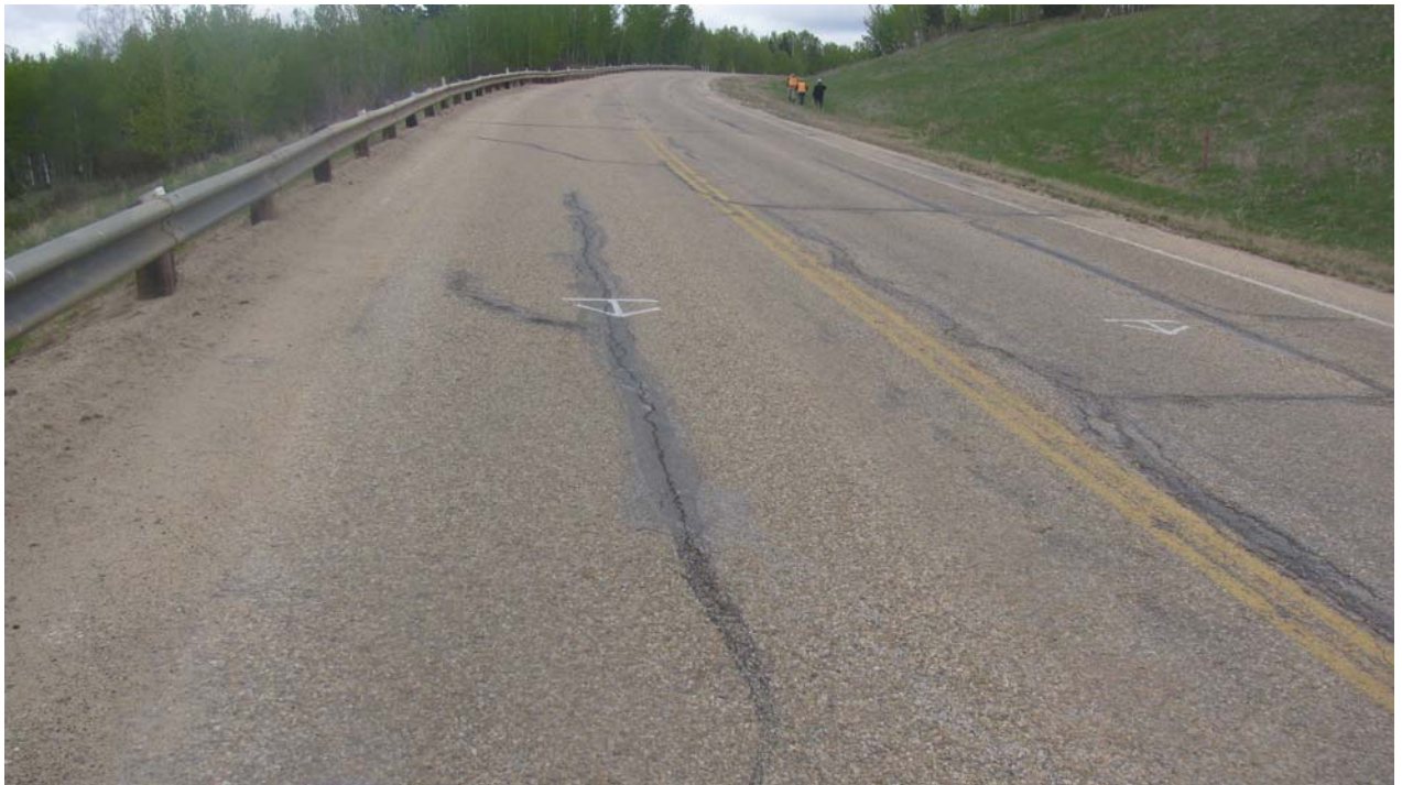
Photo #8 Looking northwest at a longitudinal crack - Mid-Hill slope section
