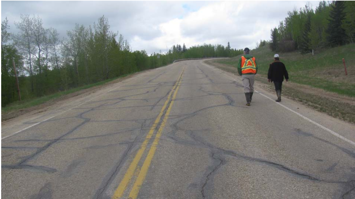
Photo #3 Looking north at multiple open longitudinal cracks in the highway surface between the southern limit of the Mid-Hill slope section and MH#1 location.
