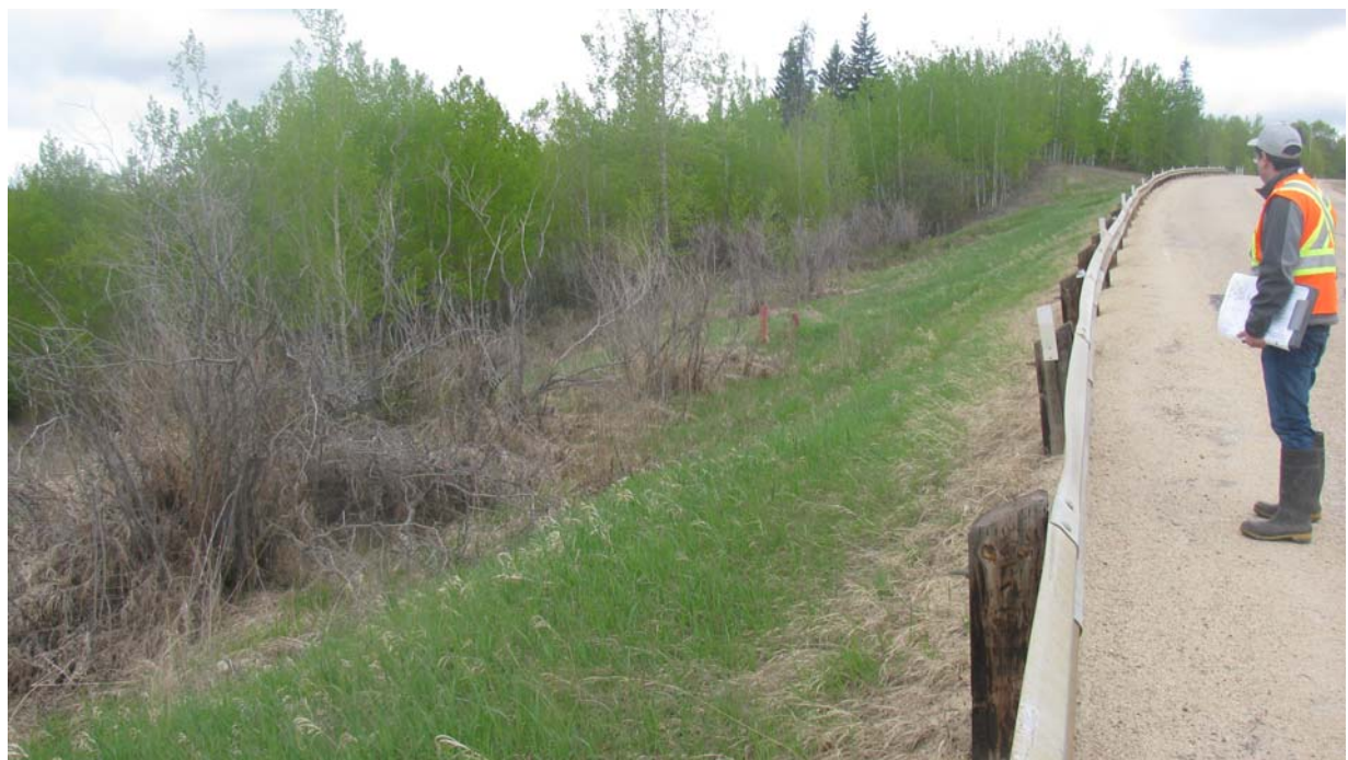
Photo #9a Looking northwest at an old graben feature of a dormant landslide location downslope of the highway to the north of the Mid-Hill slope section
