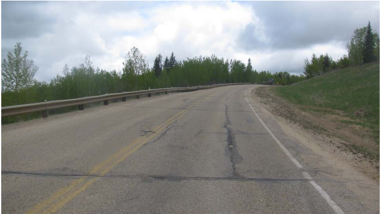
Photo #10 Looking northwest at multiple open cracks to the north of the Mid-Hill slope section; A sag in the guardrail and a dip in the highway SBL were noted above the dormant landslide located to the north of the Mid-Hill slope section
