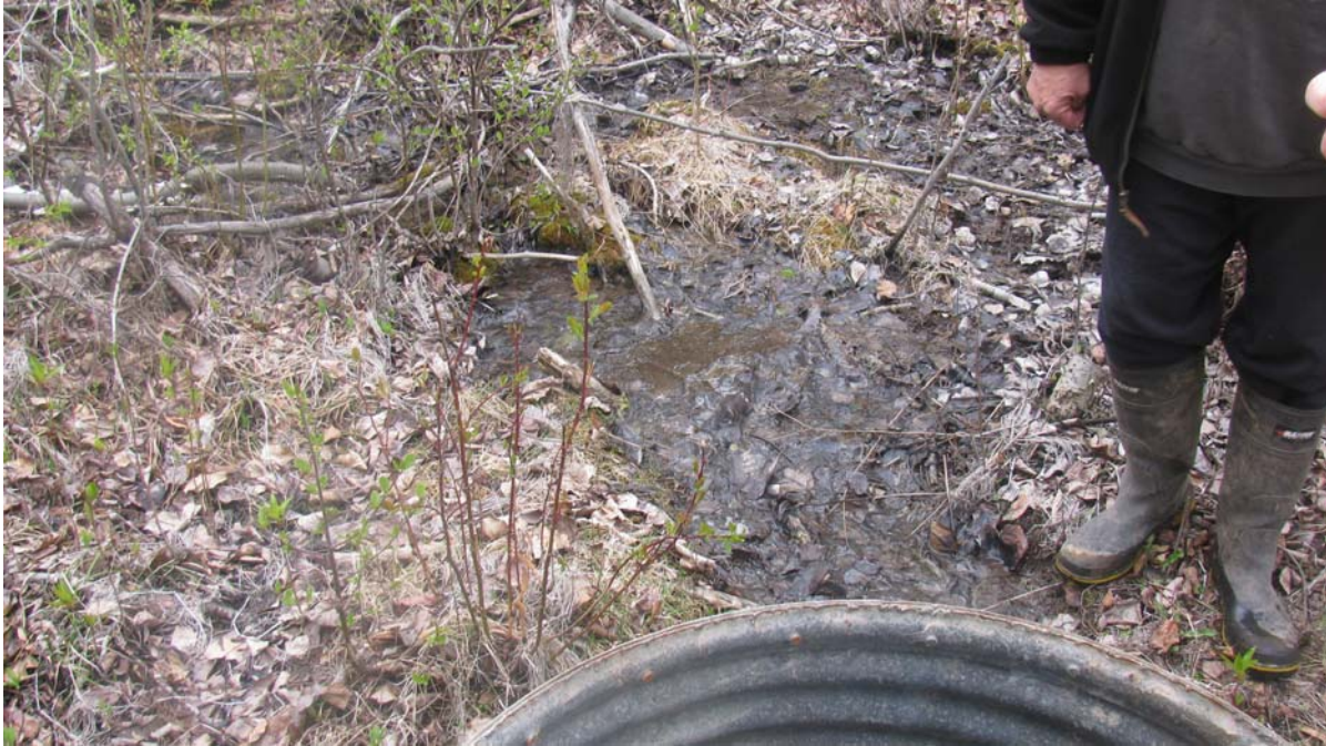
Photo #1 Looking at the area located upslope of drainage collection manhole #1. Note the presence of seepage from the hill side
