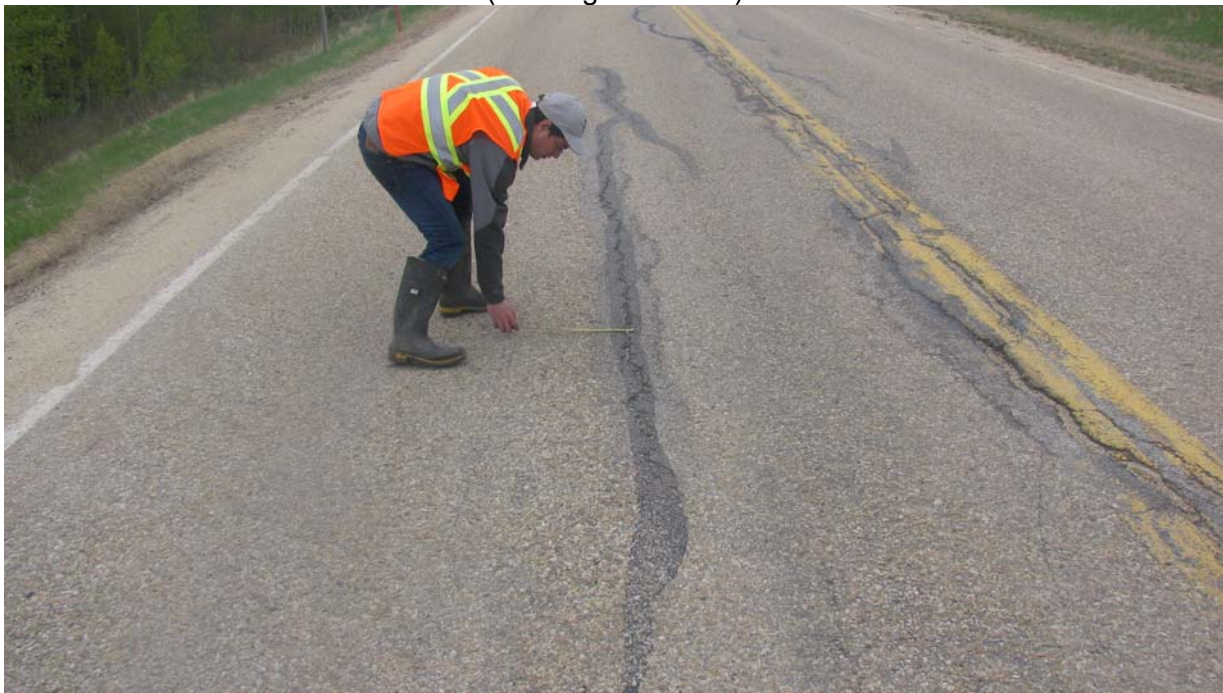
Photo #6 Open longitudinal crack within the Mid-Hill slope section (Looking Northwest)
