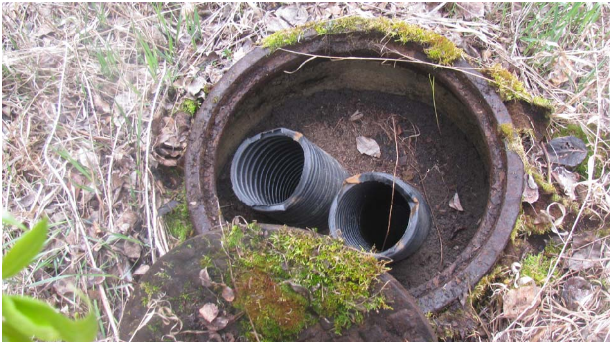
Photo # 11 Subdrain Manhole MH5. Two 150 mm diameter HDPE pipes
