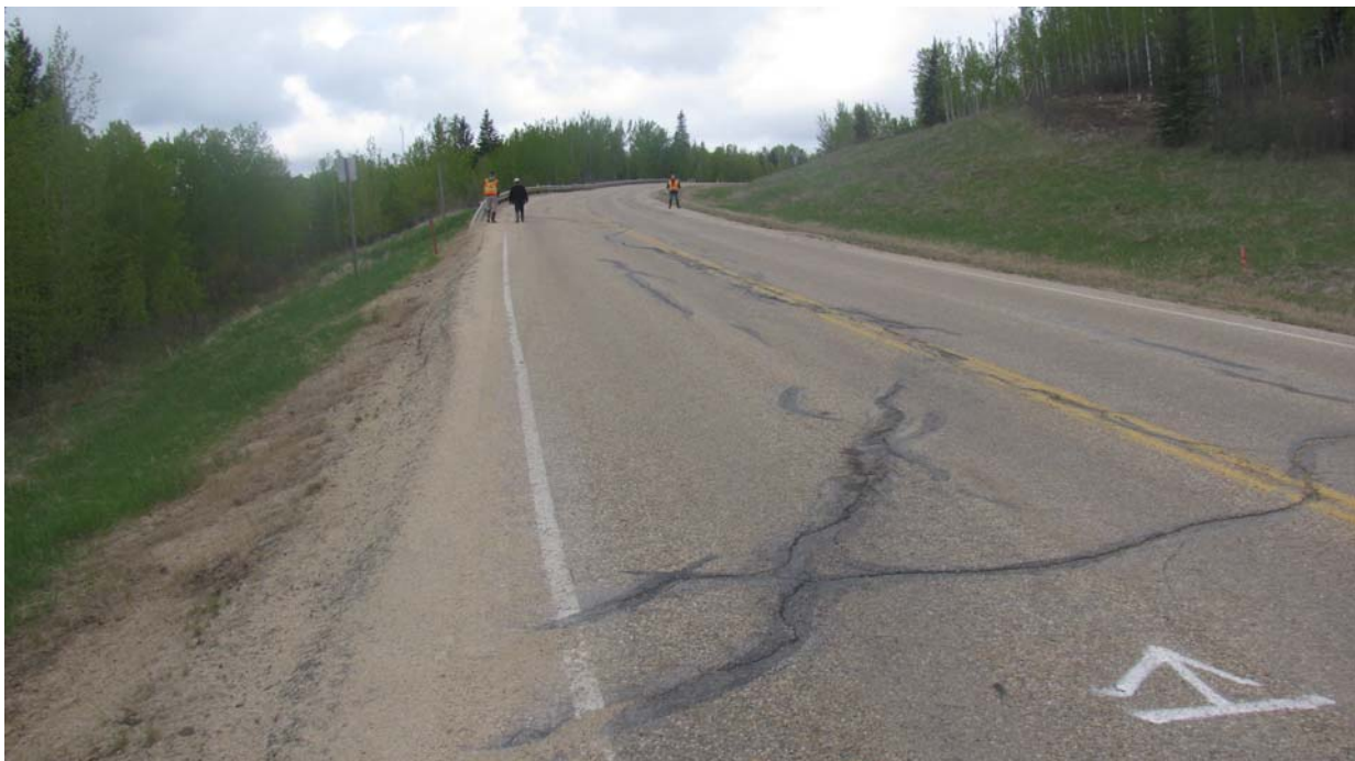
Photo #4 Open diagonal crack at the southern limit of Mid-Hill slope section (Looking northwest)
