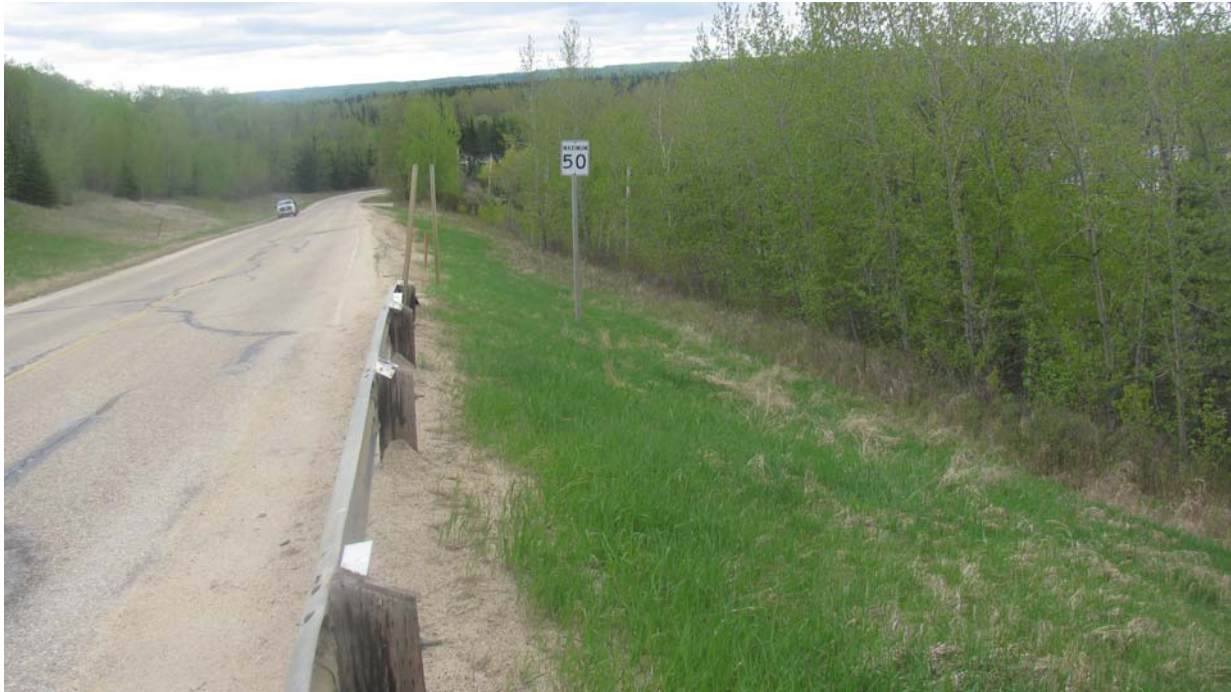
Photo #9 Looking southeast at the dip developed within the Mid-Hill slope section; the southern limit of the Mid-Hill slope section is near the 50 km/h sign
