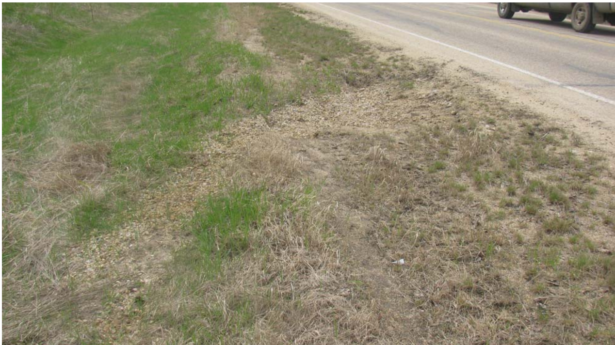
Photo #13 Looking at the slight drop/settlement development near the edge of the road.
