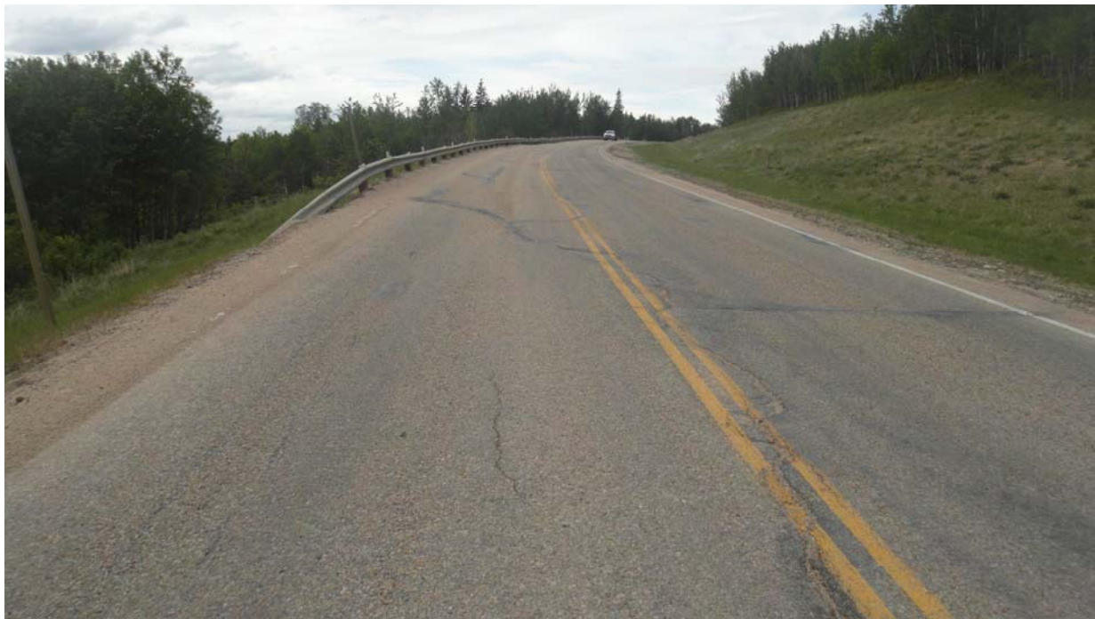
Photo #8 Open arc-shaped crack at the northern limit of Mid-Hill slope section (Looking northwest)
