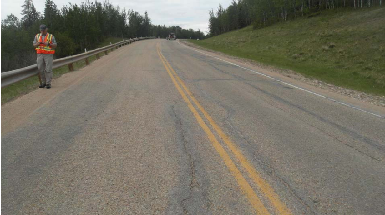
Photo #11 Looking northwest at multiple open cracks to the north of the Mid-Hill slope section
