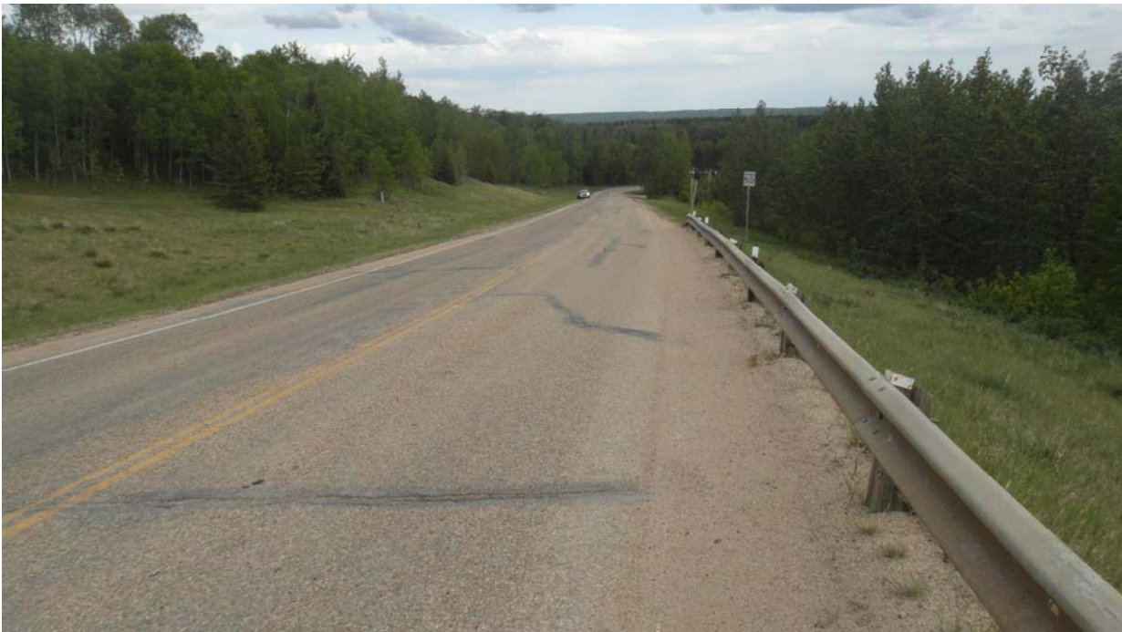
Photo #10 Looking southeast at the dip developed within the Mid-Hill slope section; the southern limit of the Mid-Hill slope section is near the 50 km/h sign
