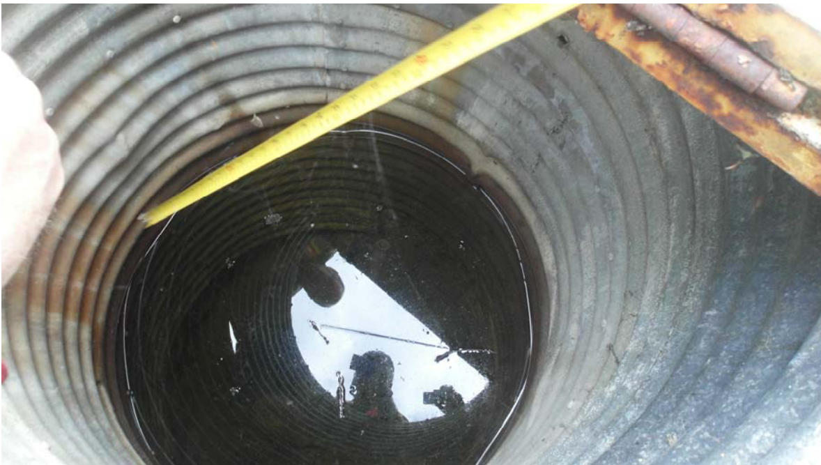
Photo #2 Standing clear water inside MH#1
