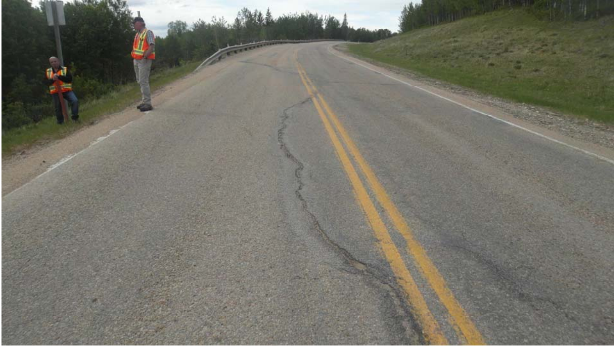
Photo #7 Open semi-longitudinal crack with the middle of the of Mid-Hill slope section (Looking northwest)
