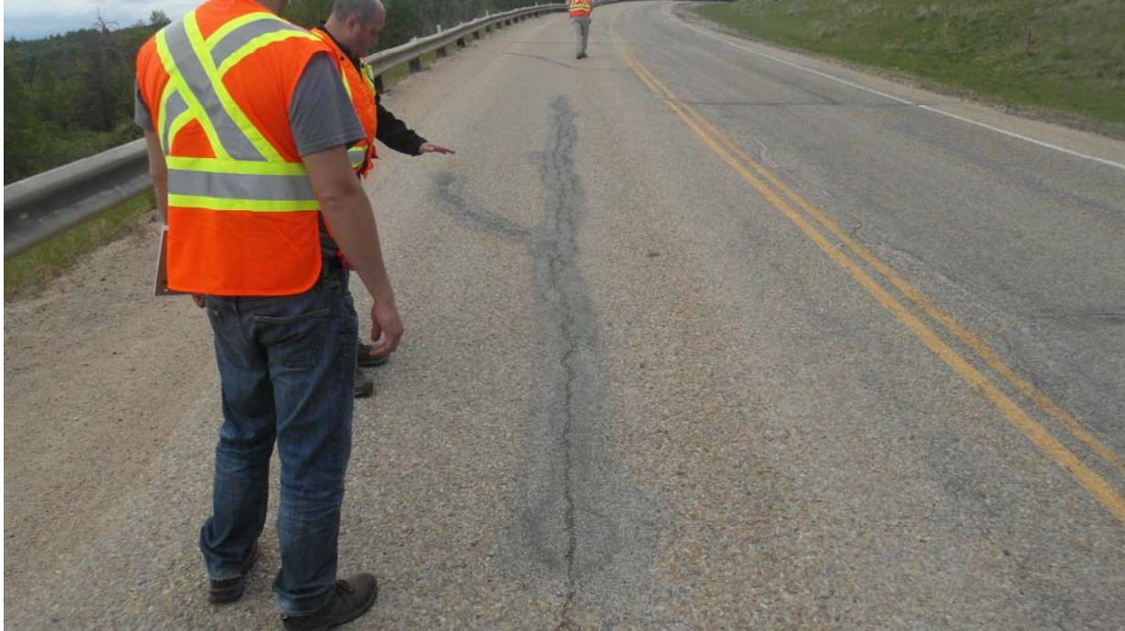
Photo #9 Looking northwest at a longitudinal crack - Mid-Hill slope section
