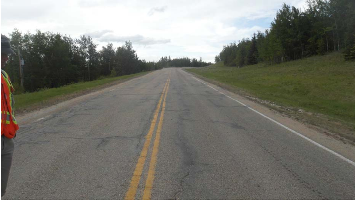
Photo #3 Looking north at multiple open longitudinal cracks in the highway surface between the southern limit of the Mid-Hill slope section and MH#1 location.
