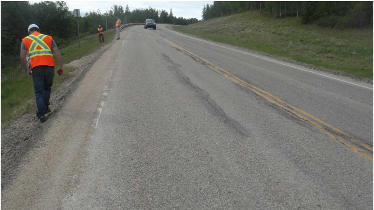
Photo #6 Open longitudinal crack within the Mid-Hill slope section (Looking northeast)
