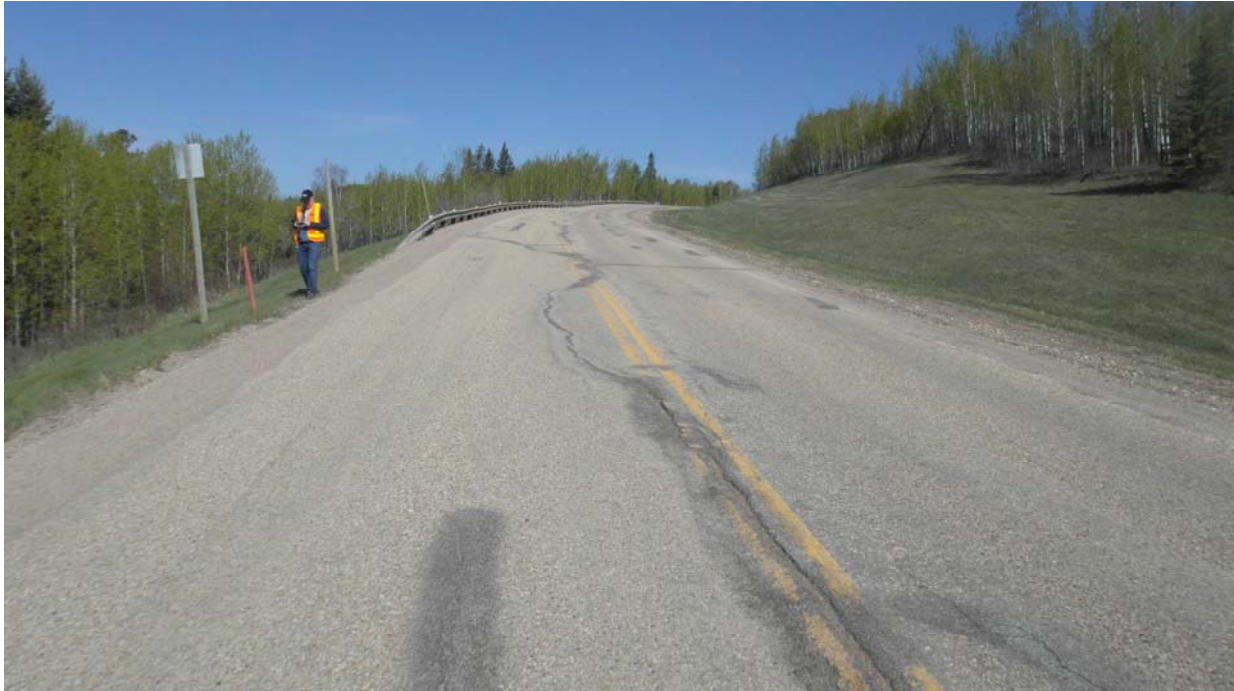
Photo #7 Open arc-shaped crack at the northern limit of Mid-Hill slope section (Looking northwest)
