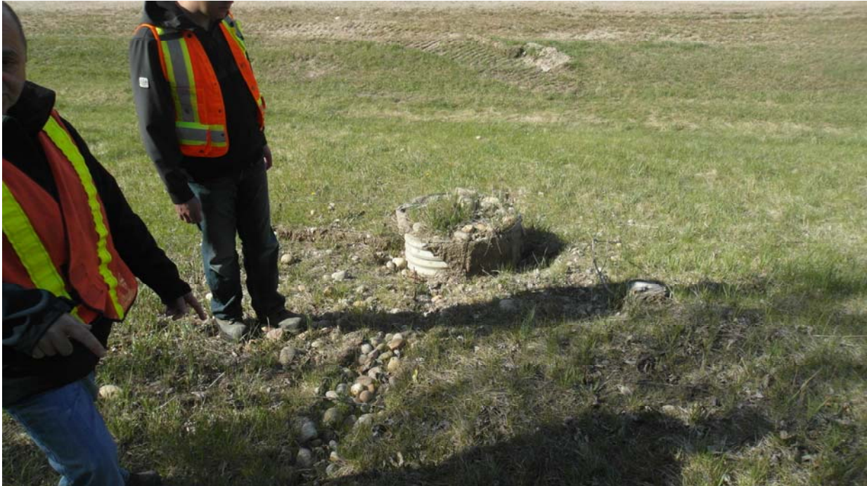
Photo #3 Looking at the manhole filled with cobbles located downslope of MH#1; note the rock filled trench by the manhole.
