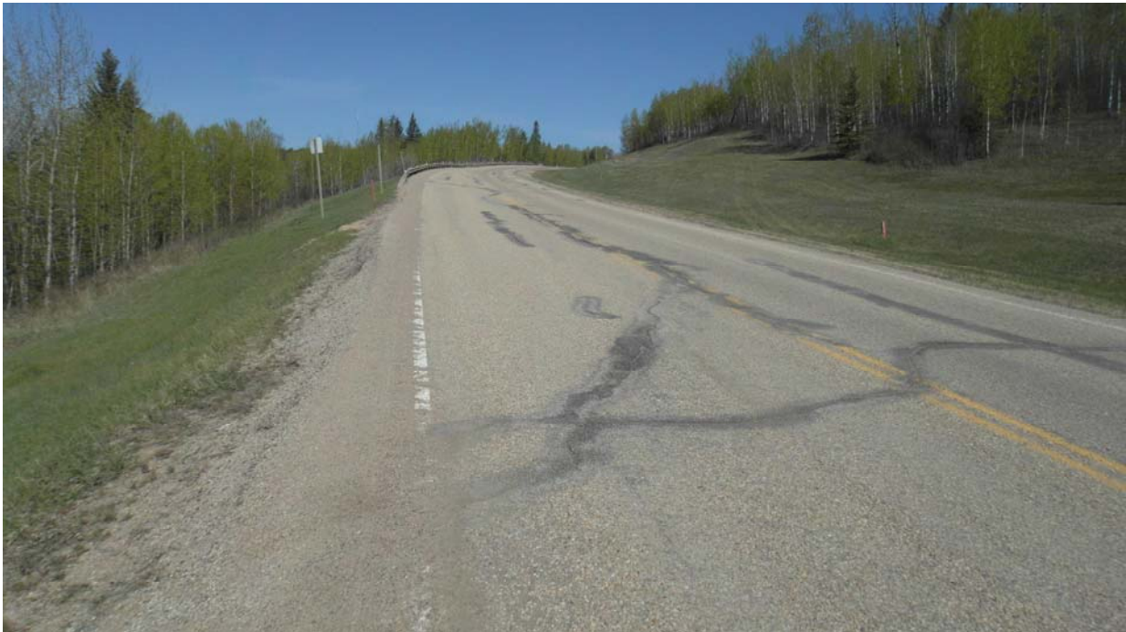
Photo #4 Open diagonal crack at the southern limit of Mid-Hill slope section (Looking northwest)
