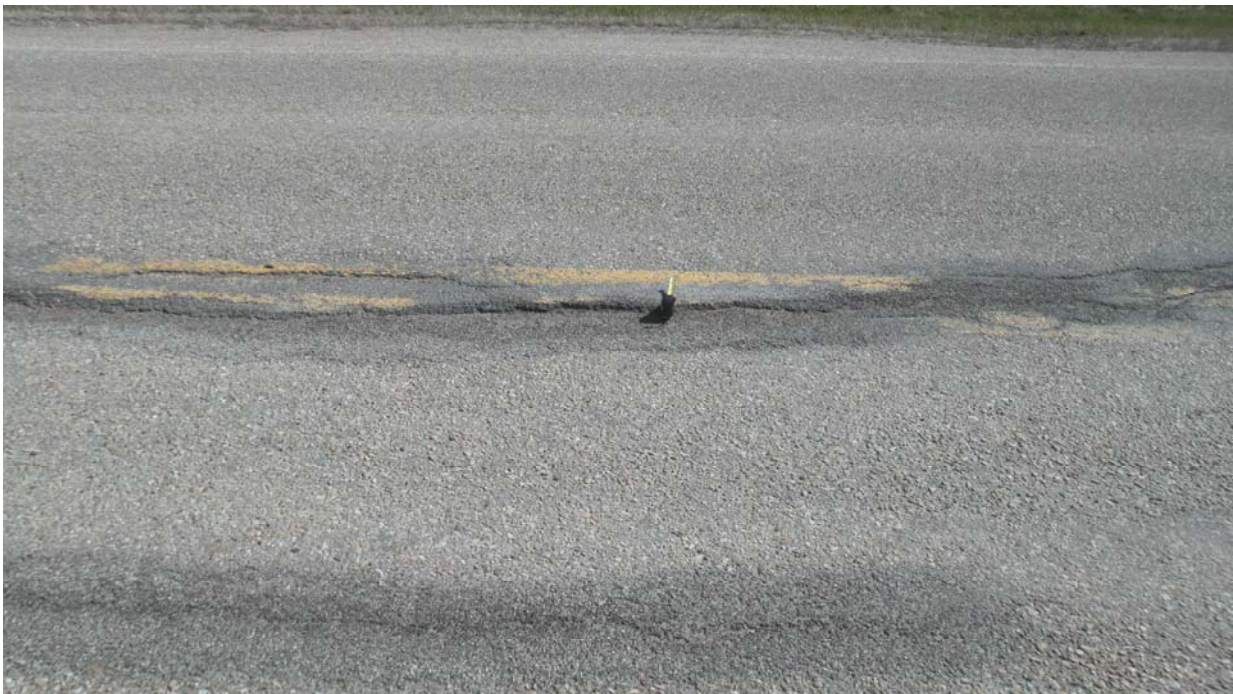
Photo #6 Open longitudinal crack within the Mid-Hill slope section; note the drop across the crack surface (Looking northeast)
