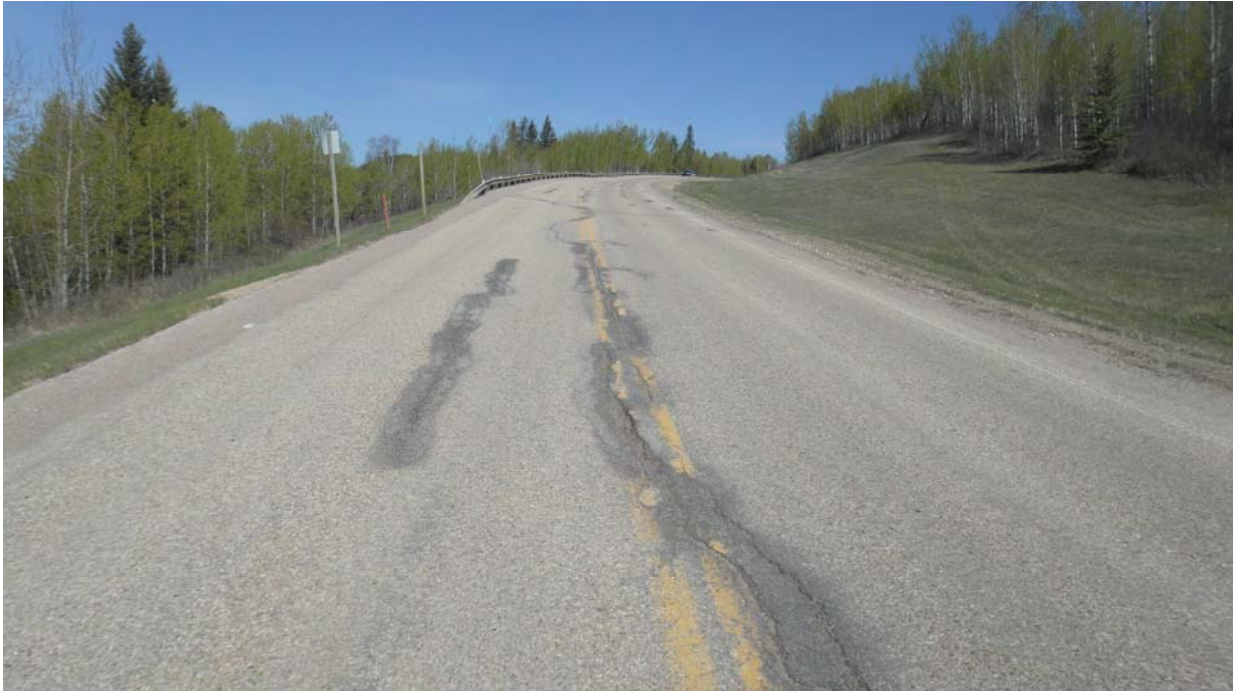
Photo #5 Open longitudinal crack within the Mid-Hill slope section (Looking northwest)
