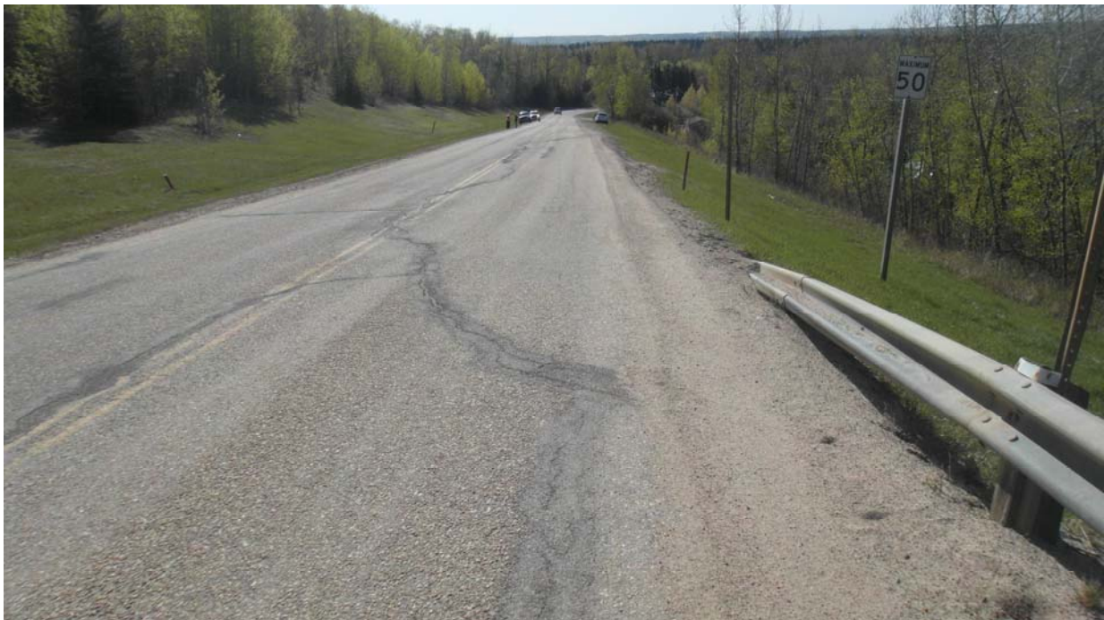
Photo #8 Looking southeast at the dip bounded by the cracks to the south of the speed sign on the highway Mid-Hill slope section
