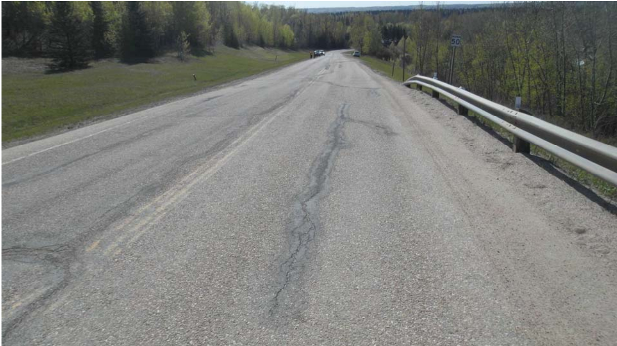
Photo #9 Looking southeast at a longitudinal crack northwest of the Mid-Hill slope section
