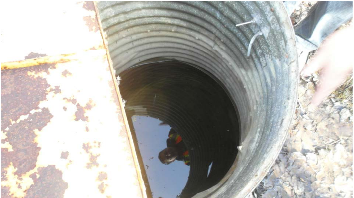
Photo #2 Standing water inside MH#1
