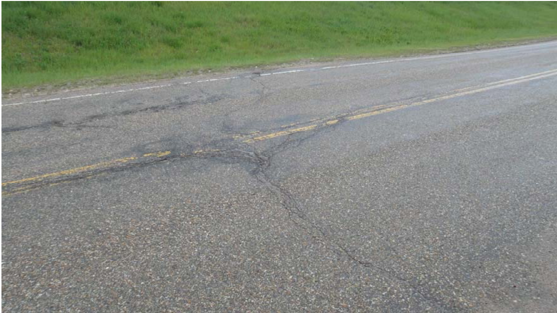
Photo #7 Diagonal open crack on the northern limit of highway uphill section, looking south
