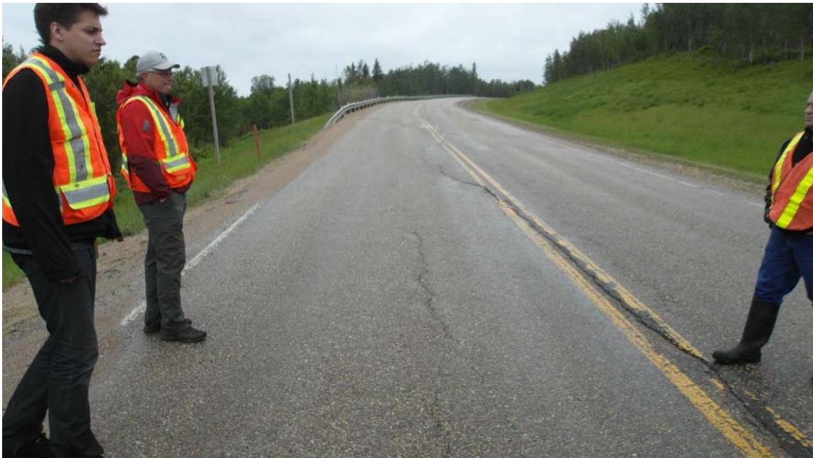
Photo #4 Open longitudinal crack within the Mid-Hill slope section (looking north)
