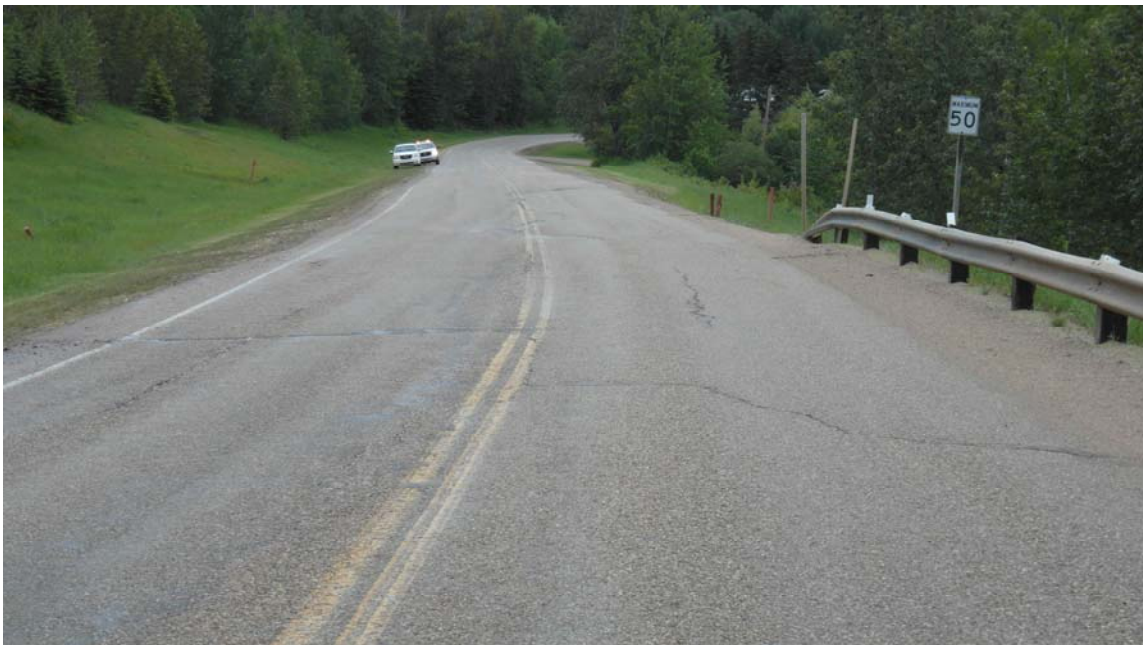
Photo #6 Looking south at the dip bounded by the cracks to the south of the speed sign on the highway Mid-Hill slope section
