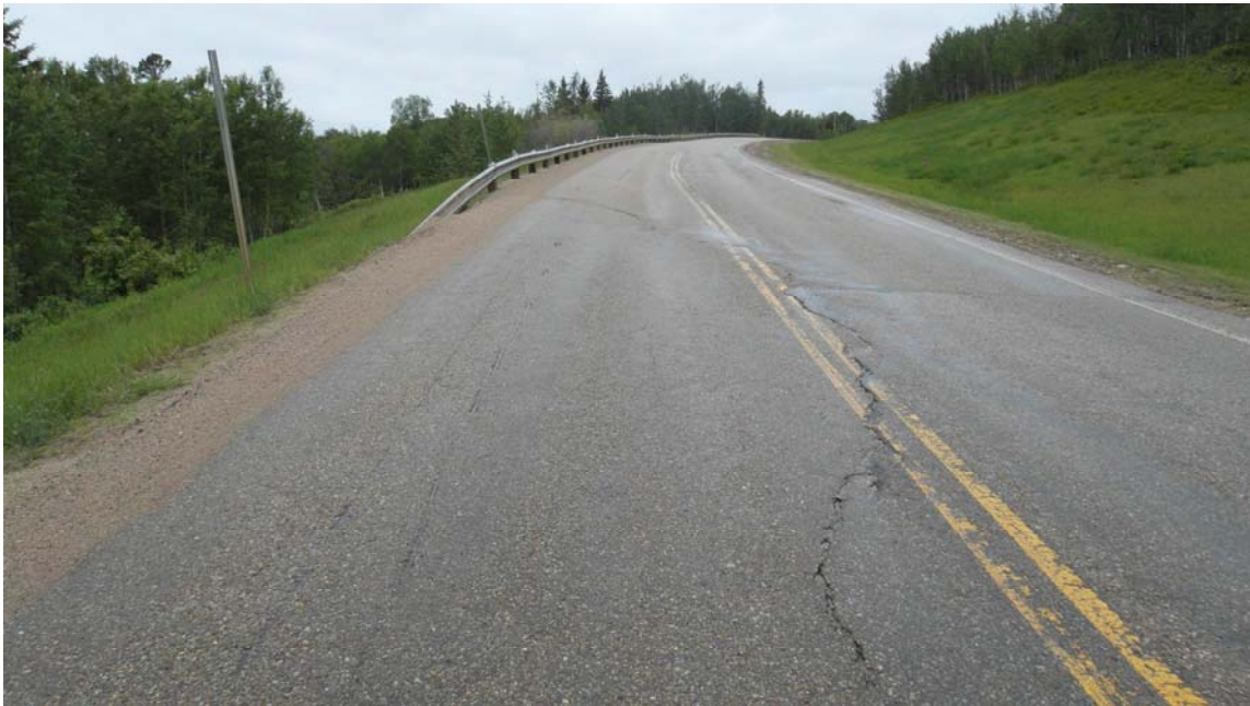
Photo #5 Open arc-shaped crack at the northern limit of Mid-Hill slope section (looking north)
