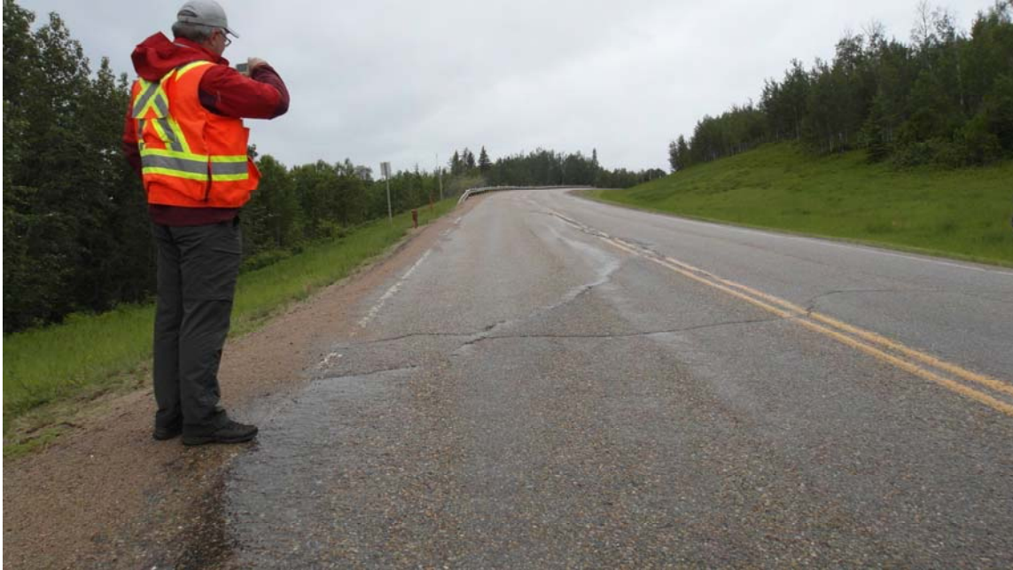
Photo #3 Open diagonal crack at the southern limit of Mid-Hill slope section (looking north)
