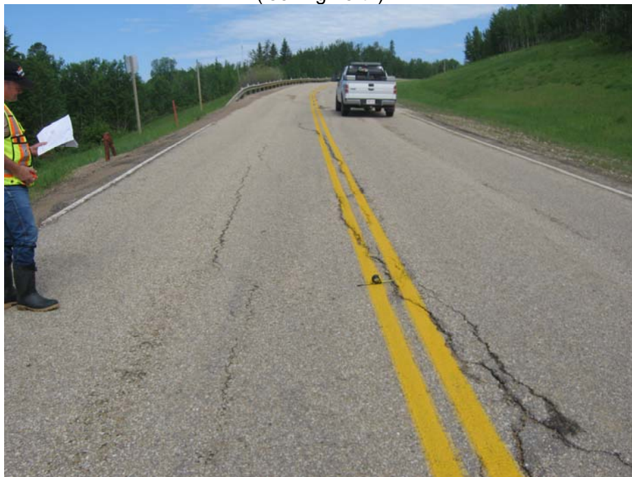
Photo #4 Open longitudinal crack within the Mid-Hill slope section (looking north)
