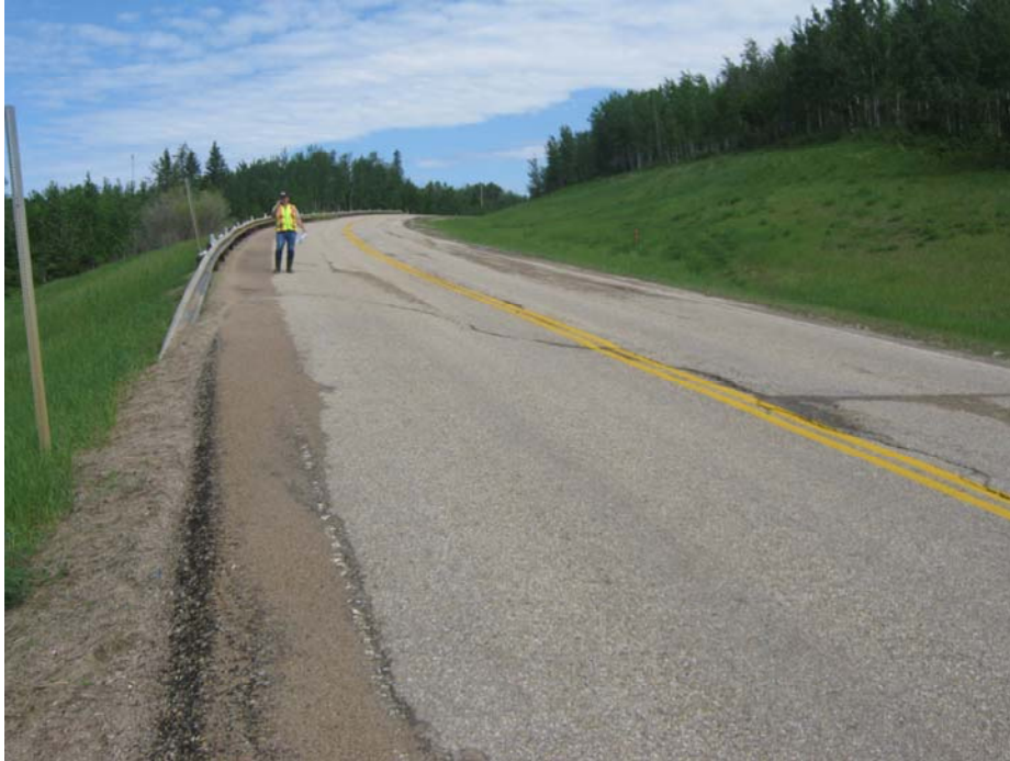
Photo #5 Open arc-shaped crack at the northern limit of Mid-Hill slope section (looking north)
