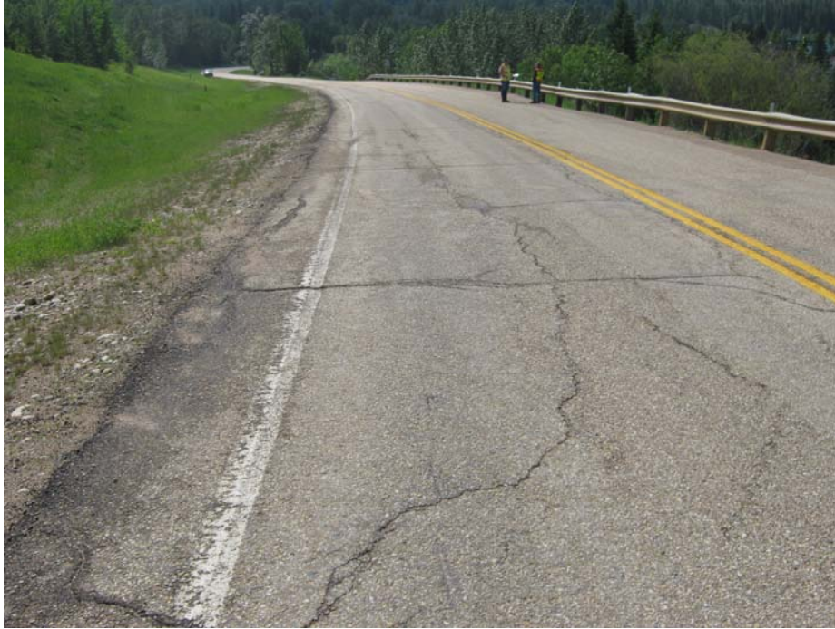
Photo #7 Diagonal and longitudinal open crack in the NBL of the highway within the highway uphill section (looking south)
