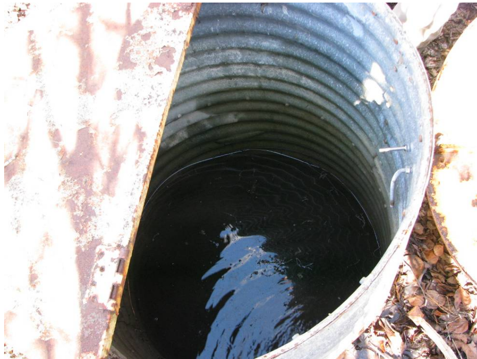
Photo #2 Standing water inside MH#1; note that the drain outlets are completely submerged under water
