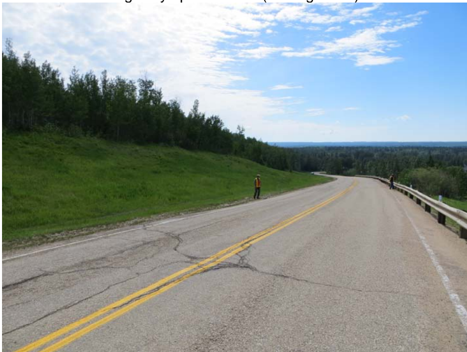
Photo #8 Diagonal open crack on the northern limit of highway uphill section, looking south
