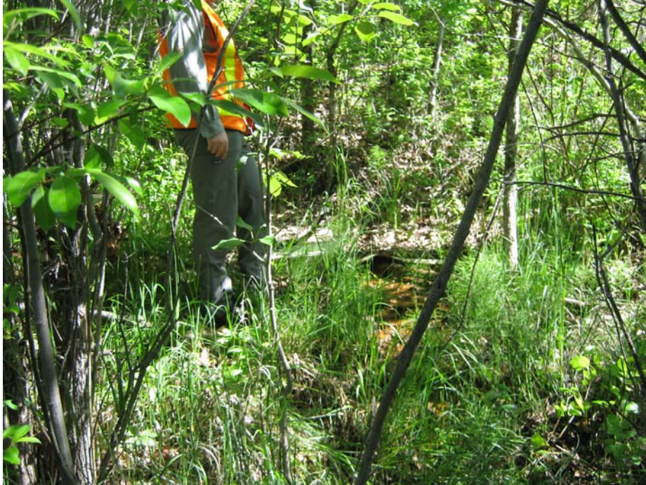
Photo #9 Looking at the metal cover above MH#2 location; note seeping water from below the cover
