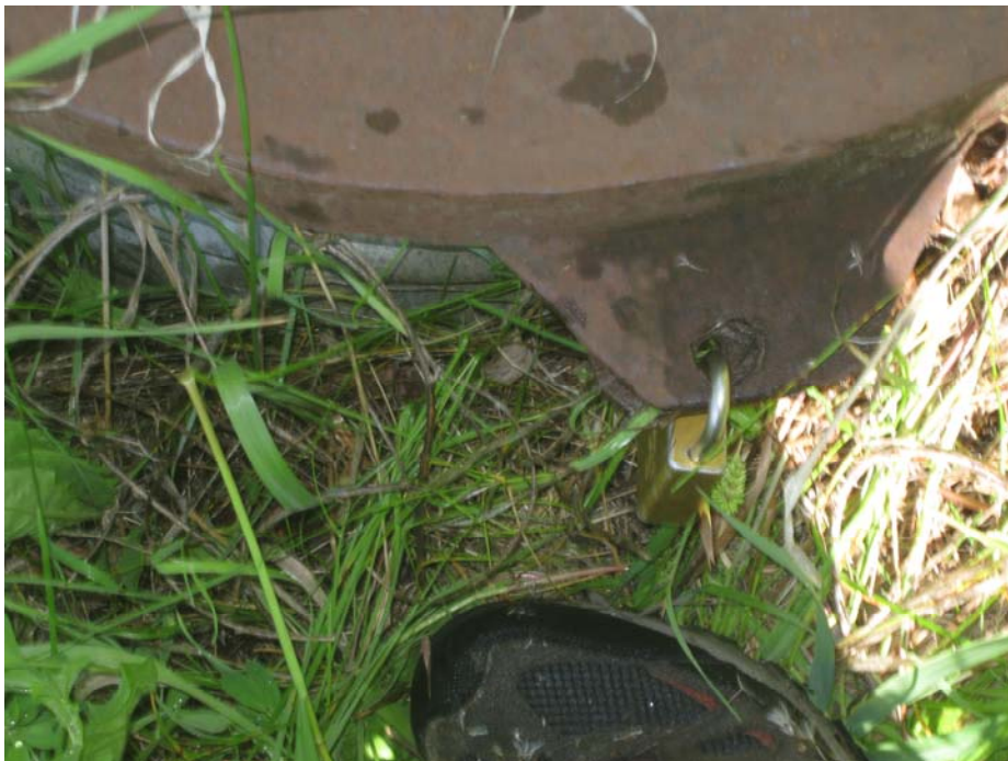
Photo #10 Looking at MH#2 cover; the manhole was locked by others which made it inaccessible for inspection
