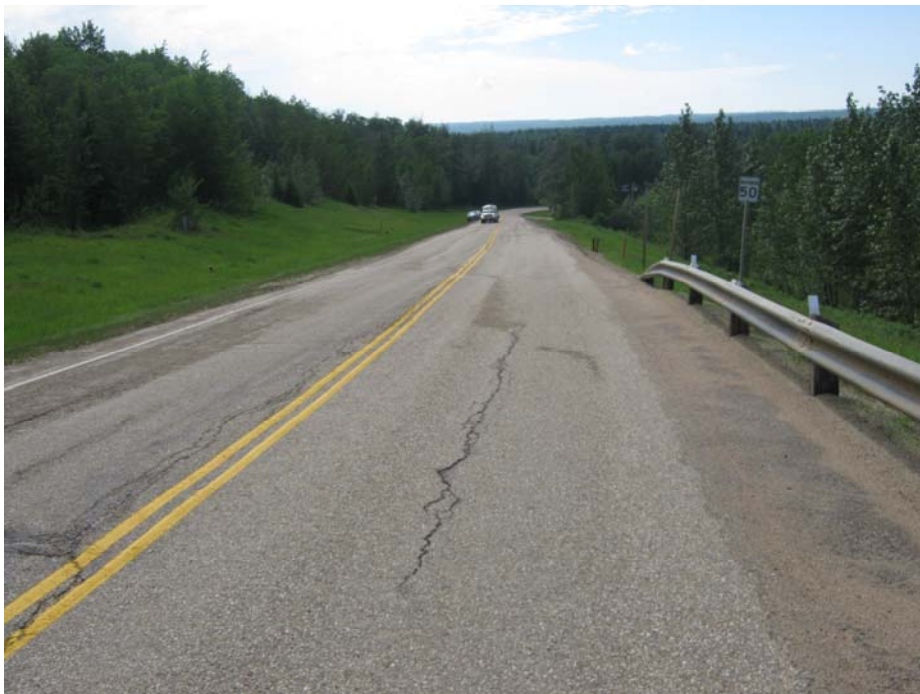
Photo #6 Looking south at the dip bounded by the cracks to the south of the speed sign on the highway Mid-Hill slope section
