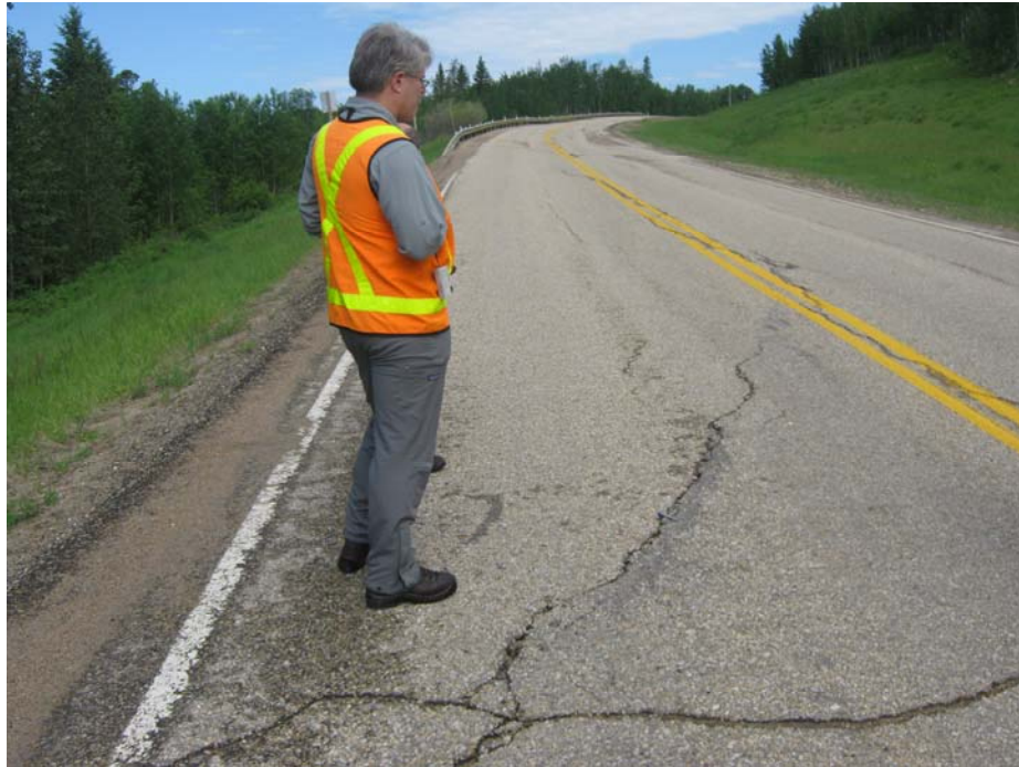
Photo #3 Open diagonal crack at the southern limit of Mid-Hill slope section (looking north)
