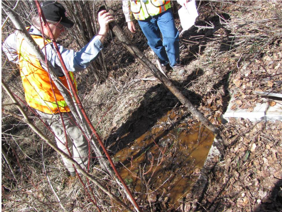
Photo #7 Existing metal cover in the top of the slope above MH#2; seepage came out when the cover was disturbed
