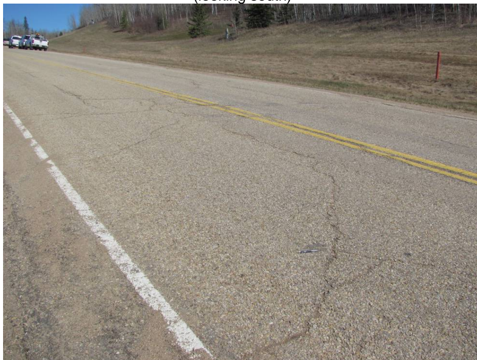
Photo #12 Open diagonal crack at the southern limit of Mid-Hill slope section (looking north)
