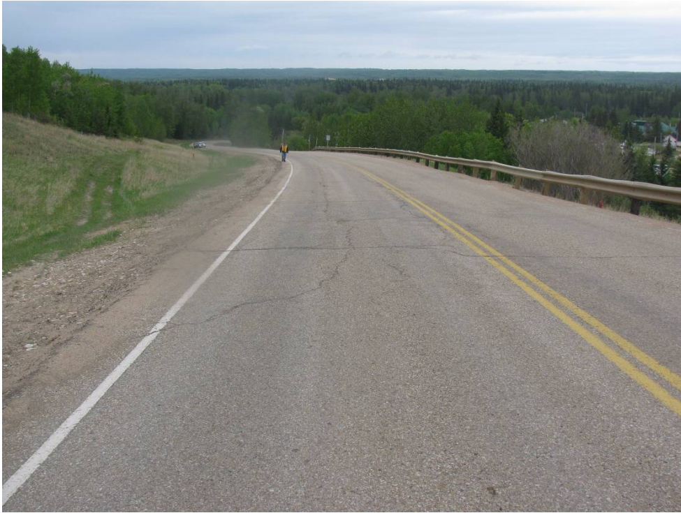
Photo #9 Diagonal and longitudinal open crack in the NBL of the highway within the highway uphill section (looking south)
