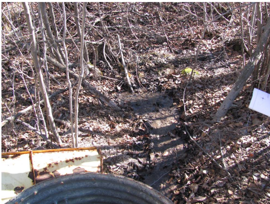
Photo #2 Trace of water around the Uphill CSP drainage collection manhole (MH#1)
