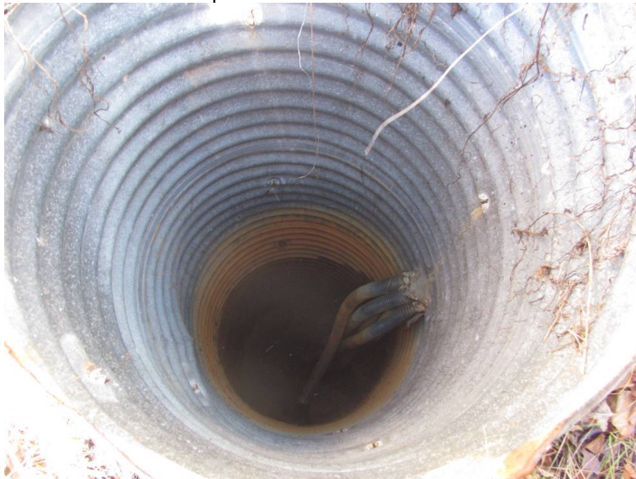
Photo #6 Looking inside MH#2; note the dry conditions and the rust inside the manhole. The manhole is about 0.6 m in diameter and 4.6 m deep below ground surface.
