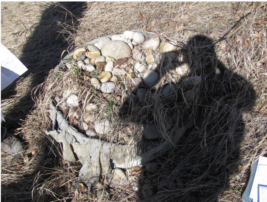
Photo #4 Looking at the manhole covered with cobbles located immediately downslope of MH#1.
