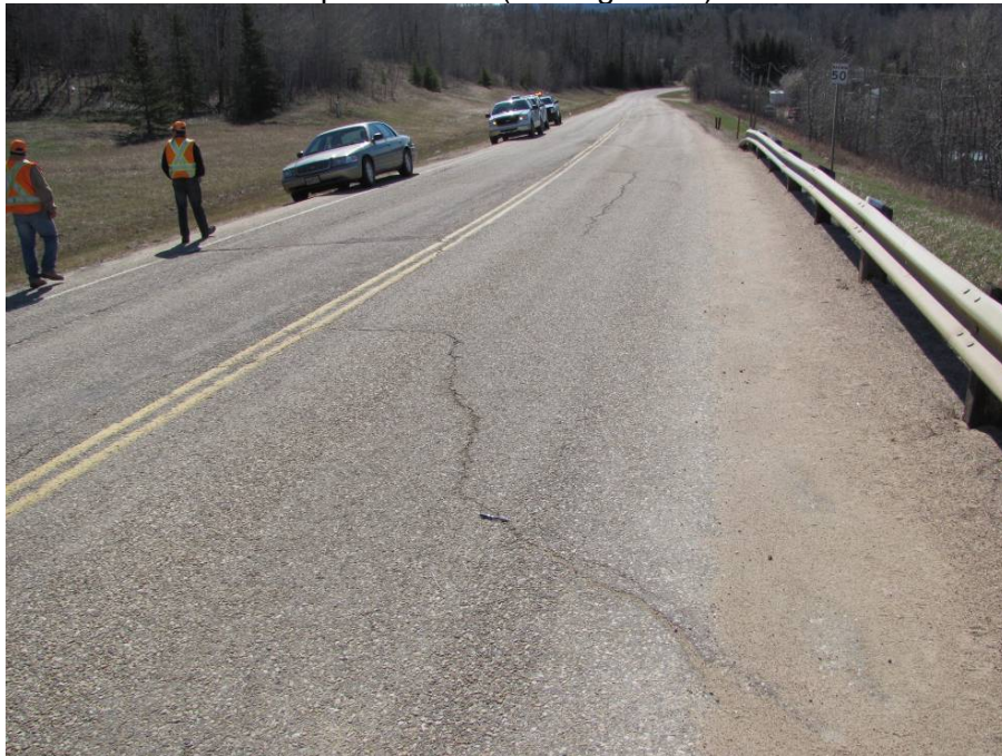
Photo #10 Open arc-shaped crack at the northern limit of Mid-Hill slope section, note dip in highway SBL (looking south)
