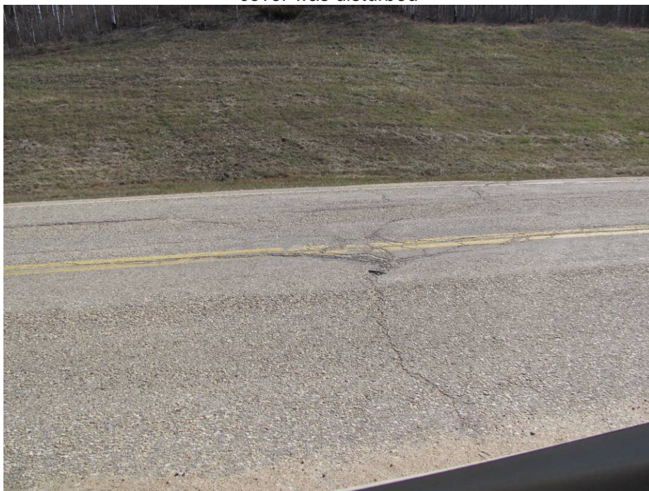
Photo #8 Diagonal open crack on the northern limit of highway uphill section, looking east
