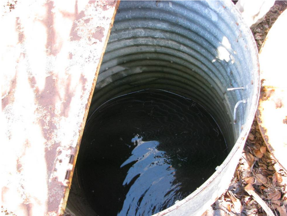
Photo #3 Standing water inside MH#1; note that the drain outlets are completely submerged under water
