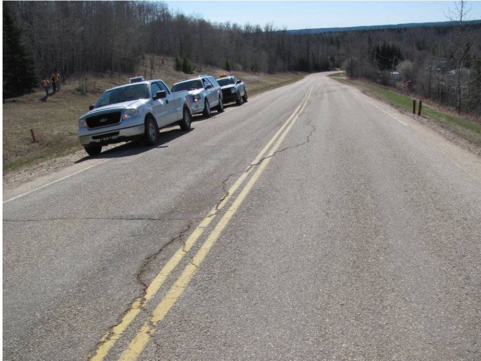
Photo #11 Cracks on the NBL and SBL surfaces within the Mid-Hill slope section (looking south)
