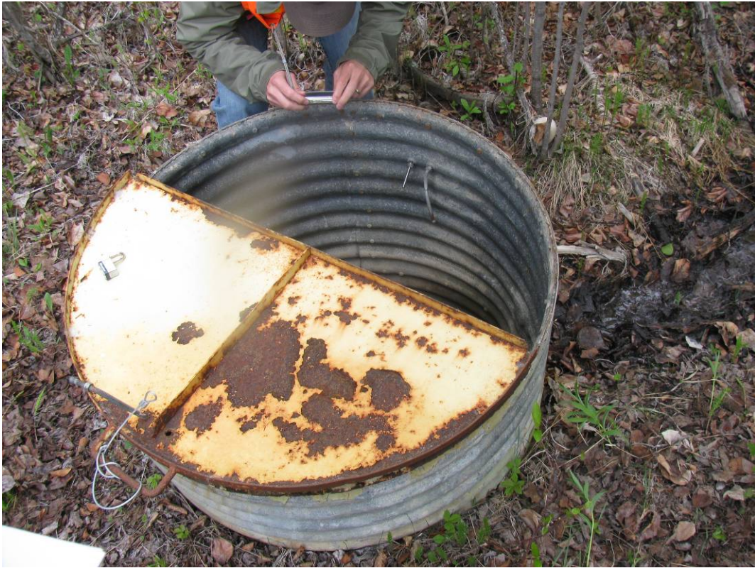
Photo #1 Trace of water around the Uphill CSP drainage collection manhole (MH#1)
