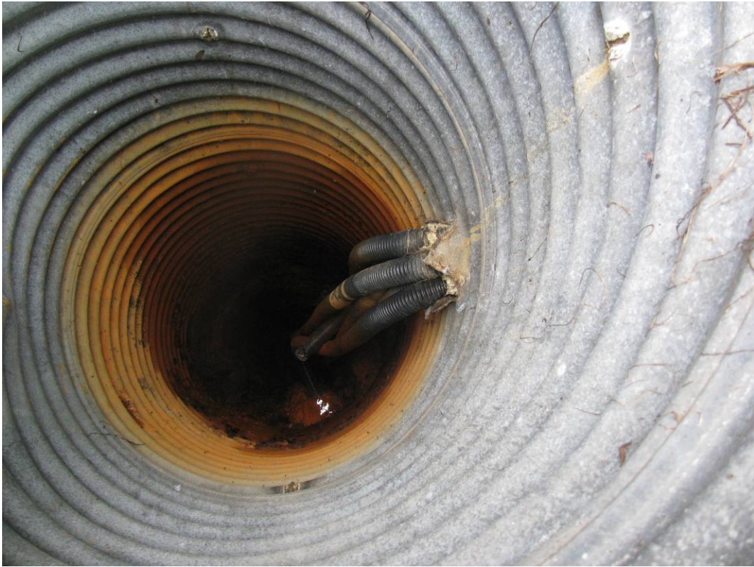
Photo #3 Looking inside MH#2; note the dry conditions and the rust inside the manhole. The manhole is about 0.6 m in diameter and 4.5 m deep below ground surface.
