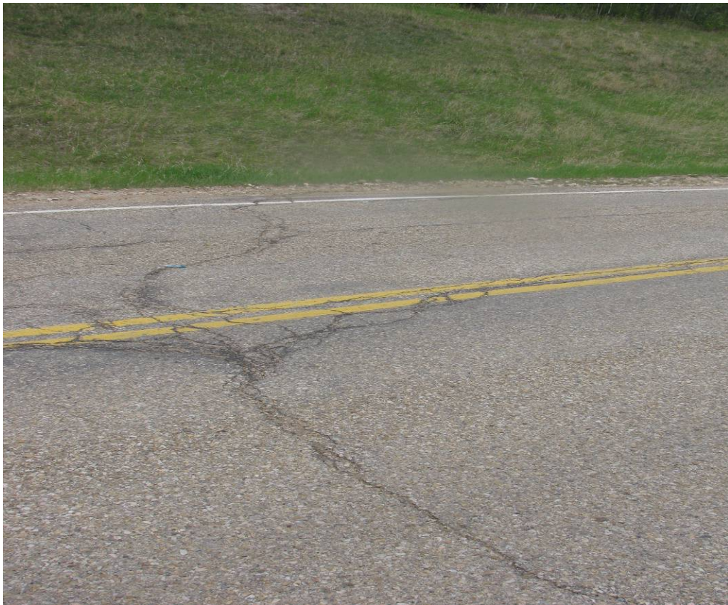
Photo #4 Diagonal open crack on the northern limit of highway uphill section, looking east
