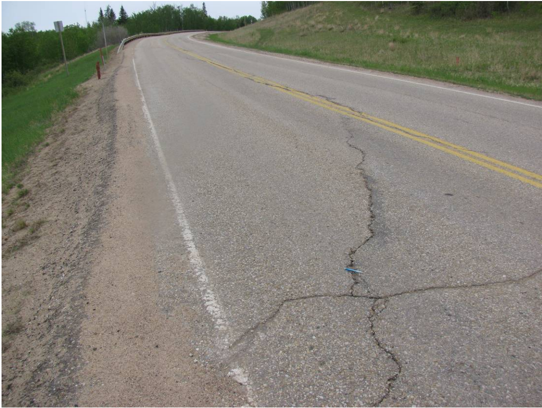
Photo #7 Open diagonal crack at the southern limit of Mid-Hill slope section, looking north
