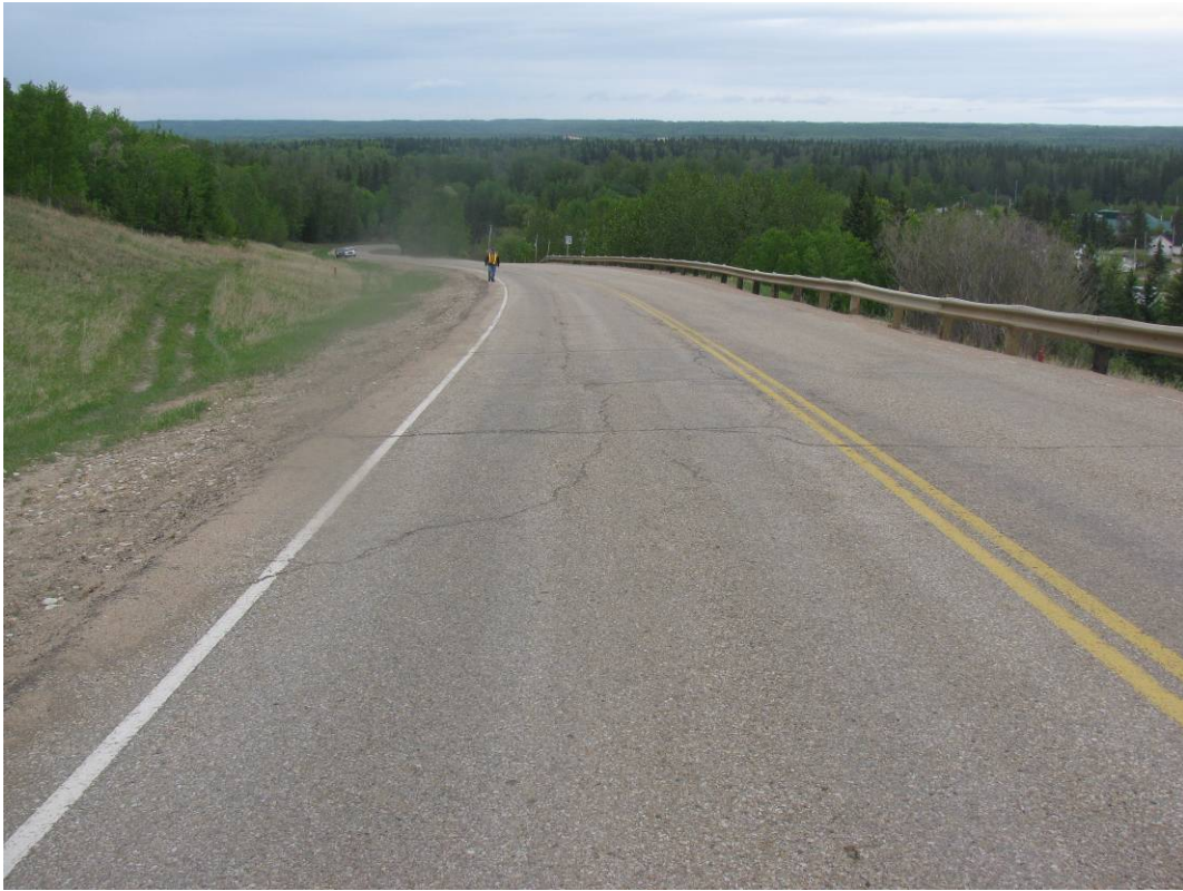
Photo #5 Diagonal and longitudinal open crack in the NBL of the highway within the highway uphill section, looking south
