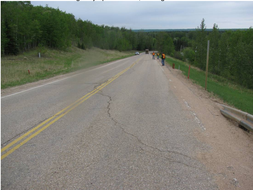
Photo #6 Open arc-shaped crack at the northern limit of Mid-Hill slope section, note dip in highway SBL (looking south)
