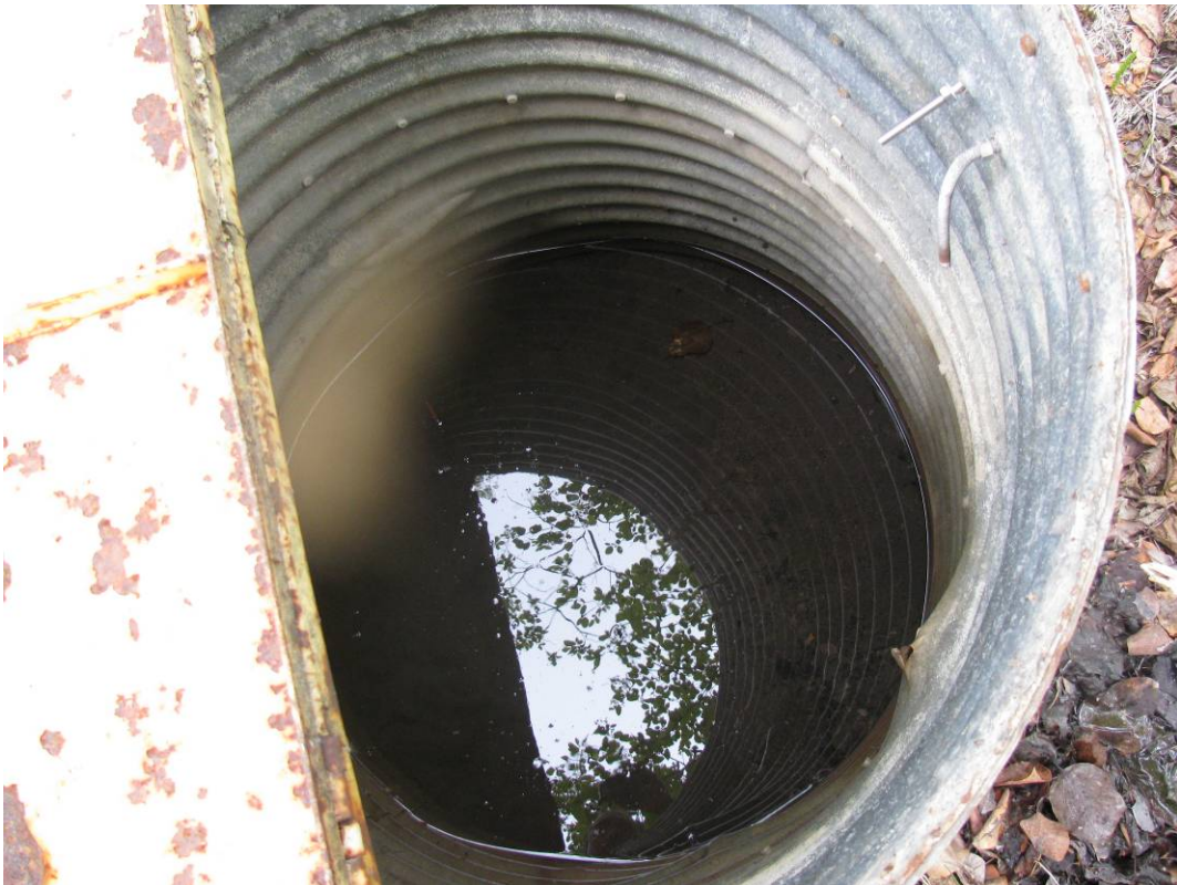
Photo #2 Standing water inside MH#1; note that the drain outlets are completely submerged under water
