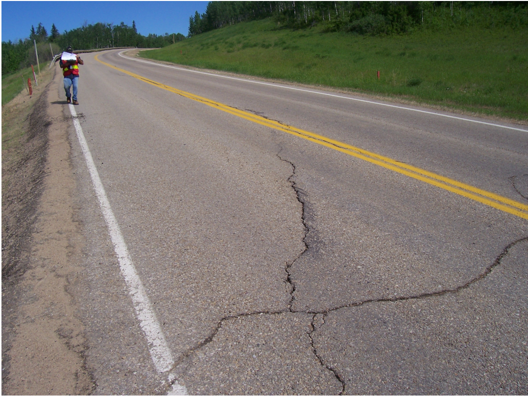
Photo #3 Open arc-shaped crack at the southern limit of Mid-Hill slope section, looking north
