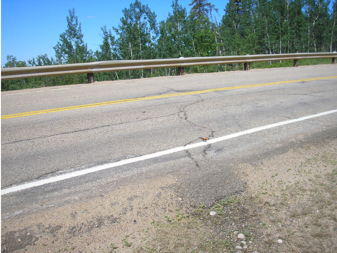
Photo #6 Diagonal open crack on the northern limit of highway uphill section, looking west
