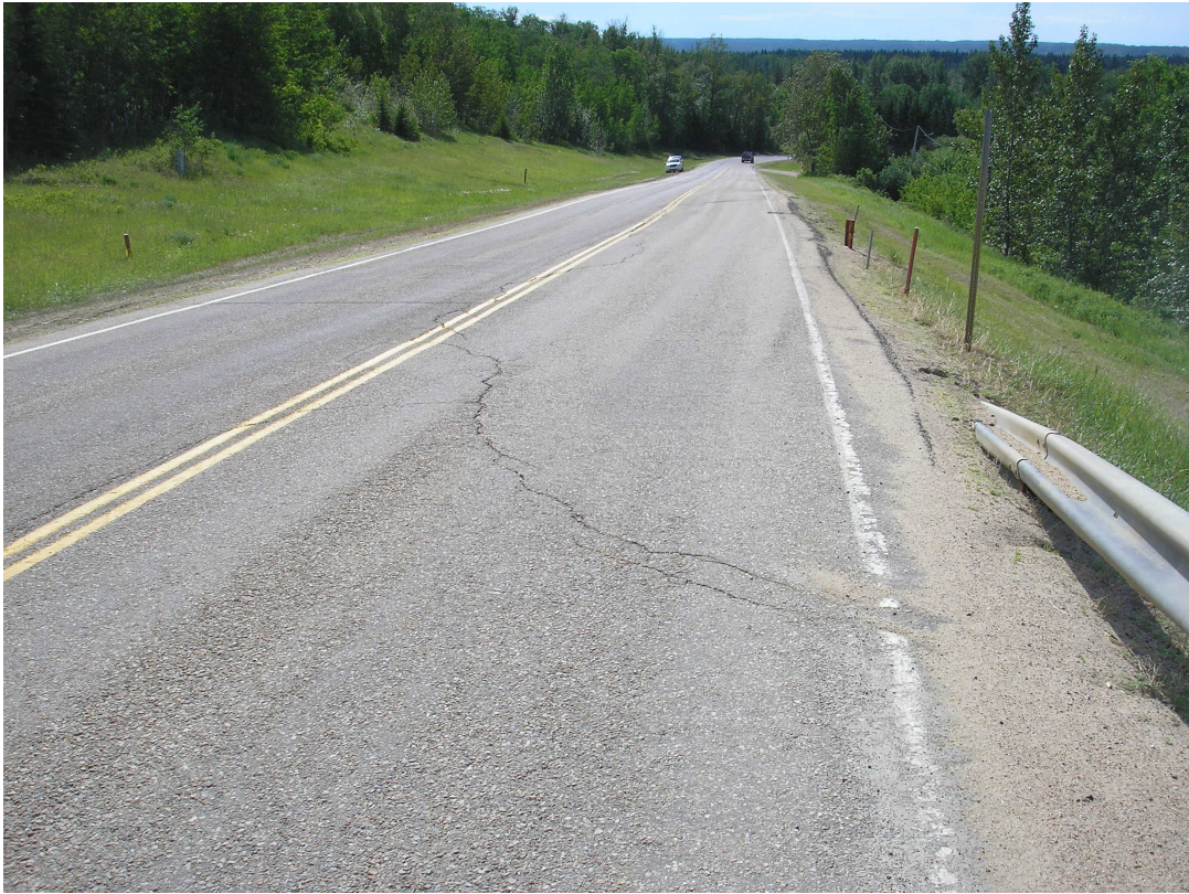
Photo #5 Open arc-shaped crack at the northern limit of Mid-Hill slope section, note dip on highway SBL (looking south)
