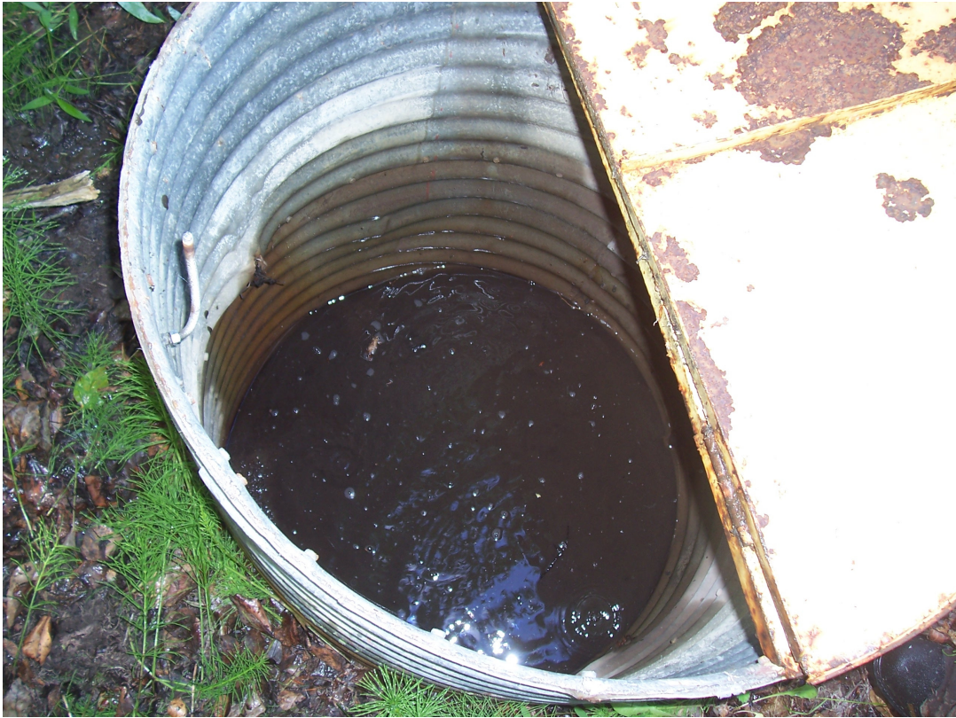
Photo #1 Water standing inside the Uphill CSP drainage collection manhole (MH#1)
