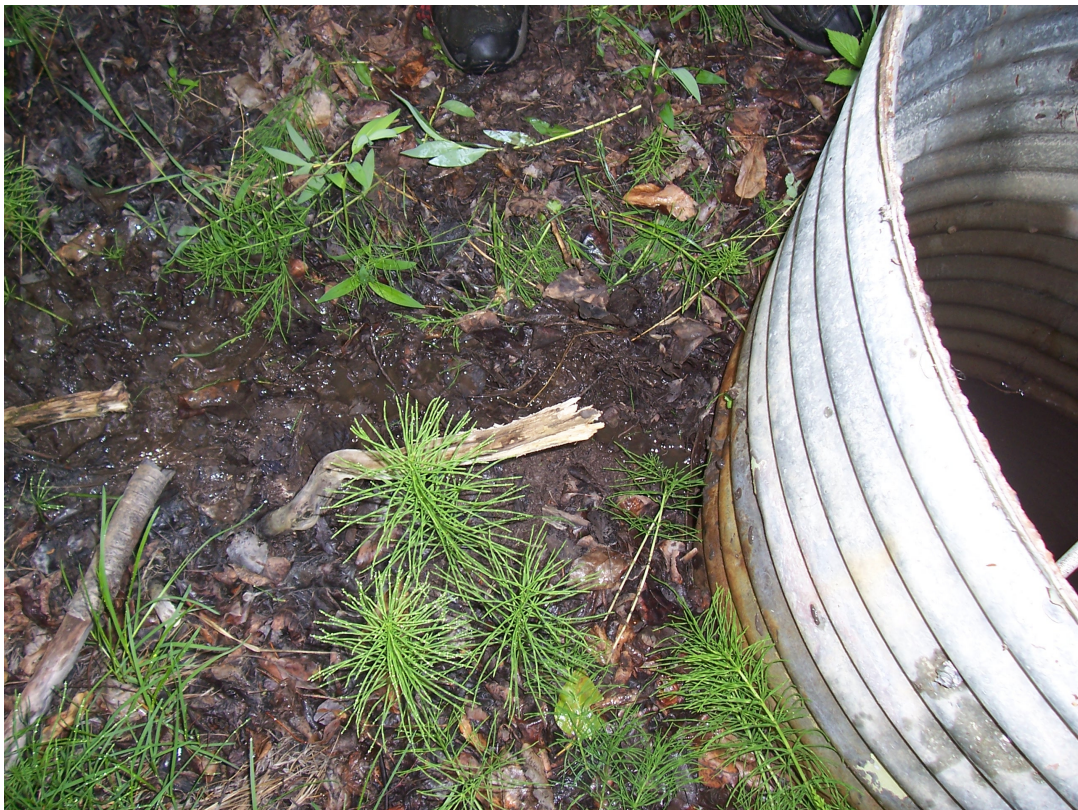
Photo #2 Water ponding around MH#1
