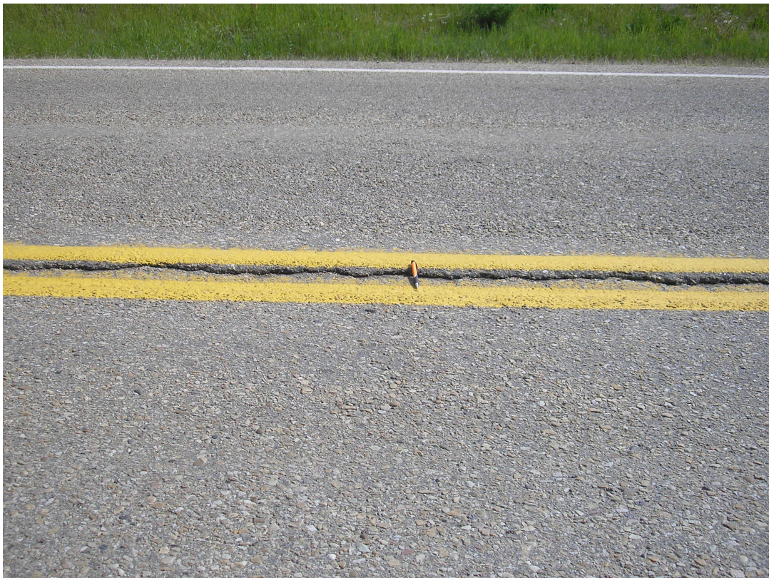
Photo #4 Dip on the highway SBL bounded by a centerline crack along the Mid-Hill slope section, looking east
