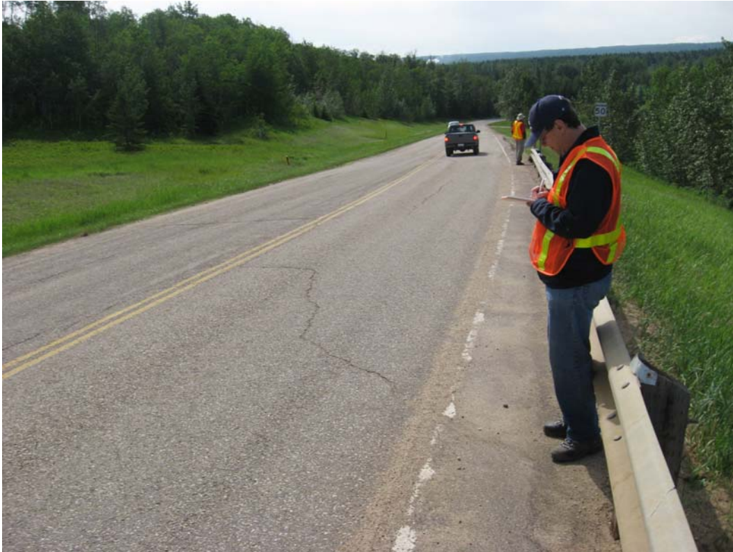
Photo 1 Up hill general pavement cracks.
