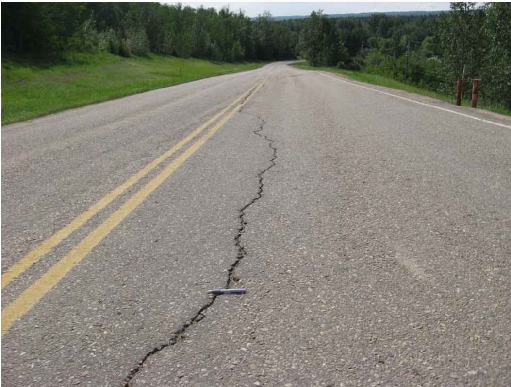
Photo 2 Mid-hill general pavement cracks.
