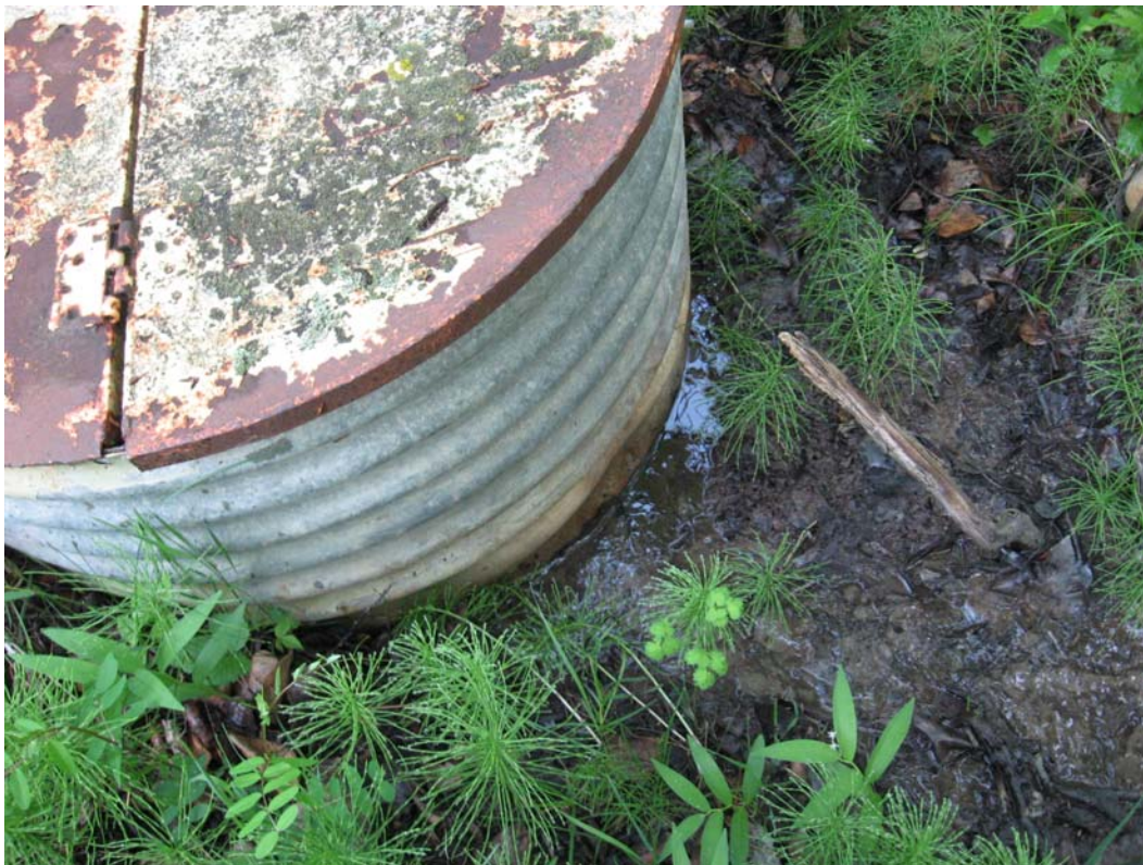
Photo 4 Water ponding at the backslope manhole.
