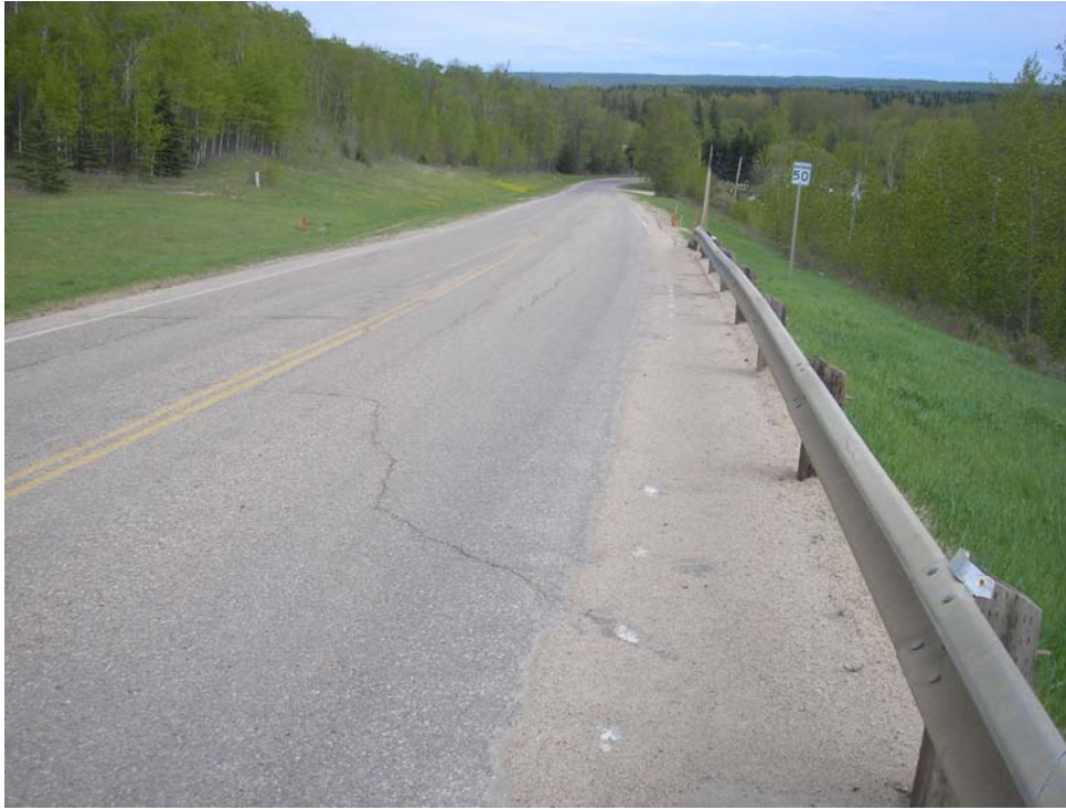
Photo 1 Up hill general pavement cracks.
