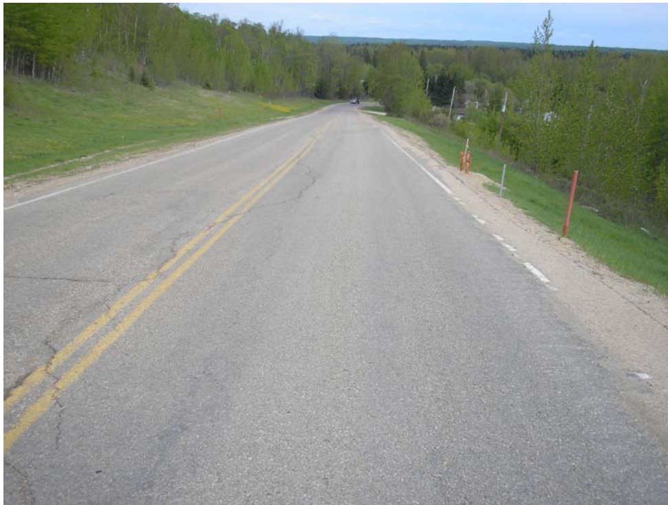
Photo 2 Mid-hill general pavement cracks.
