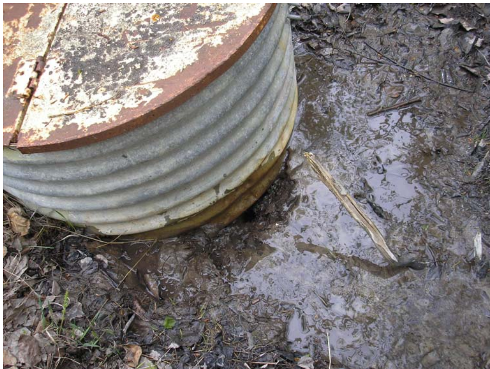
Photo 4. Water ponding at the backslope manhole.
