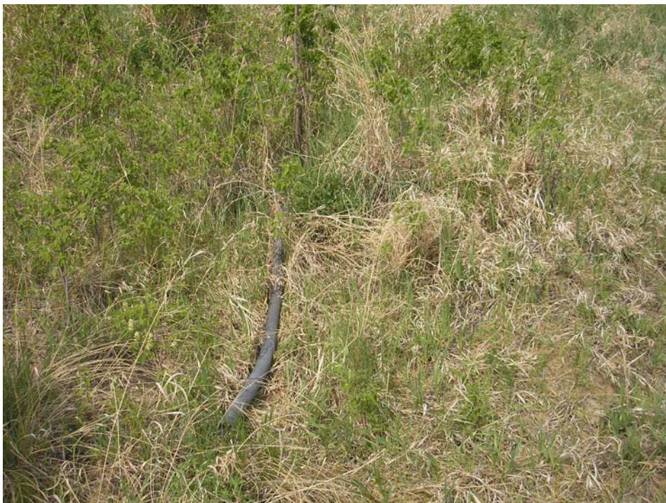
Photo 4. Subhorizontal drain outlet found in the side slope, May 19, 2006.
