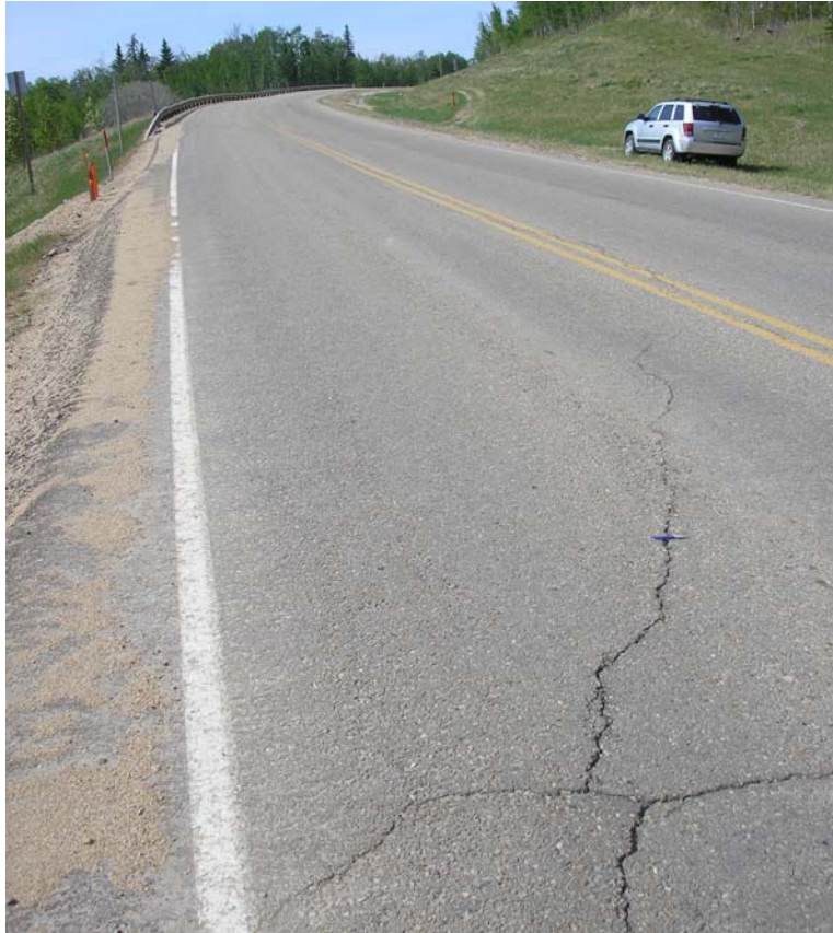
Photo 1. Up hill general pavement cracks, May 19, 2006.
