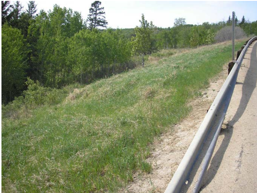
Photo 2. Scarp and graben feature on the sideslope unchanged, May 19, 2006.
