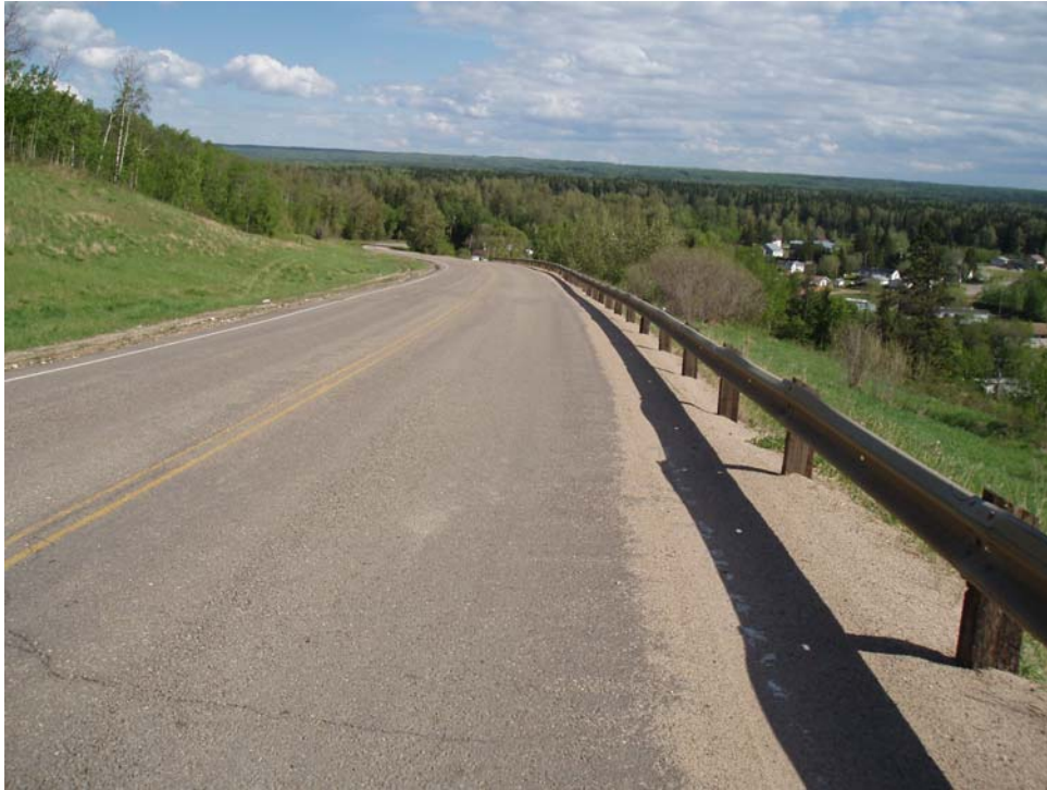
Photo 1. Up hill general view. Note on the foreground the cracking reappearing on the pavement patched in 2003.
