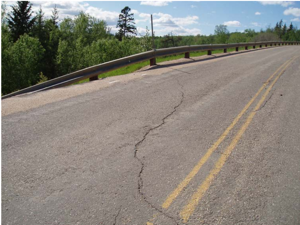
Photo 2. Mid-hill pavement distress.
