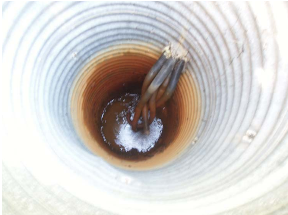
Photo 4 Collection point at the toe of the slope. Note the oxidation stain elevation
