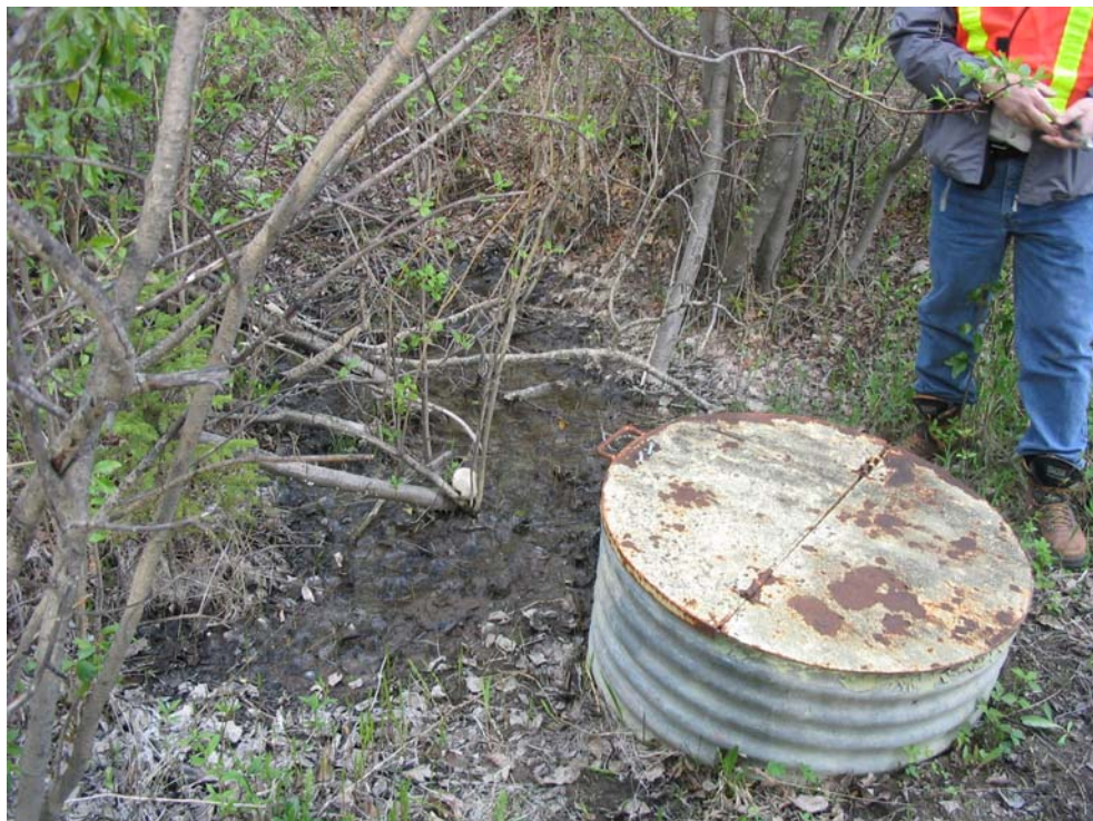
Spring flowing into vertical CSP well.
