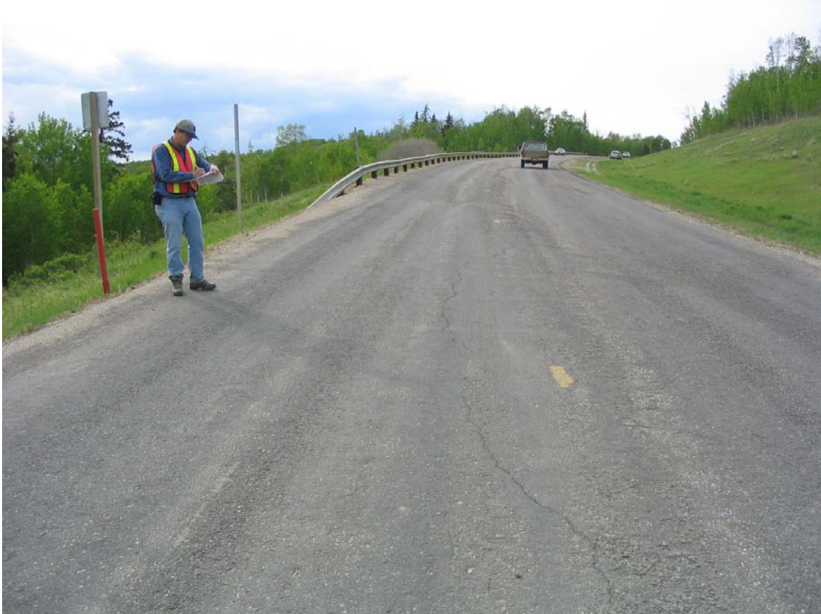
Mid-Hill - Faint crack re-appearing through the new path
