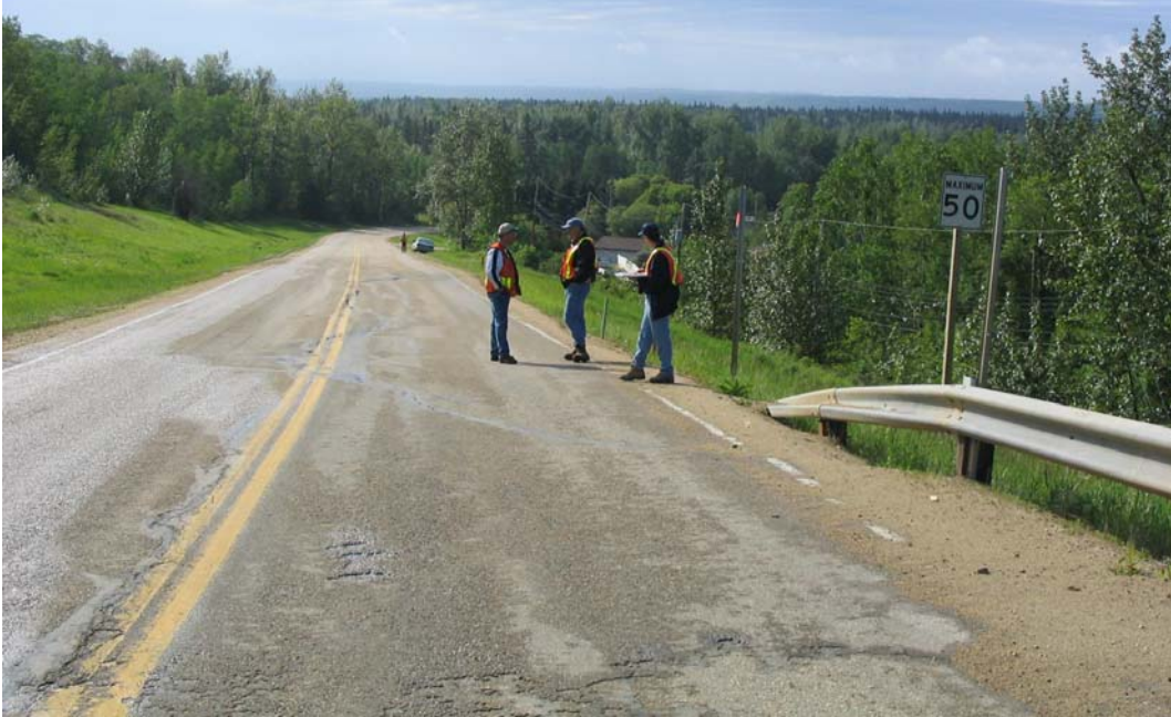
Mid hill slide looking east
