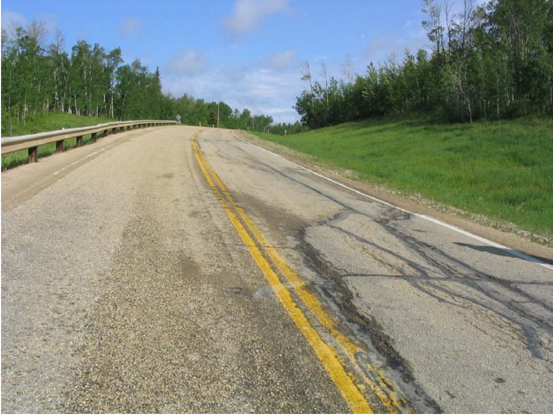
Upper hill area – looking west, pavement dip.
