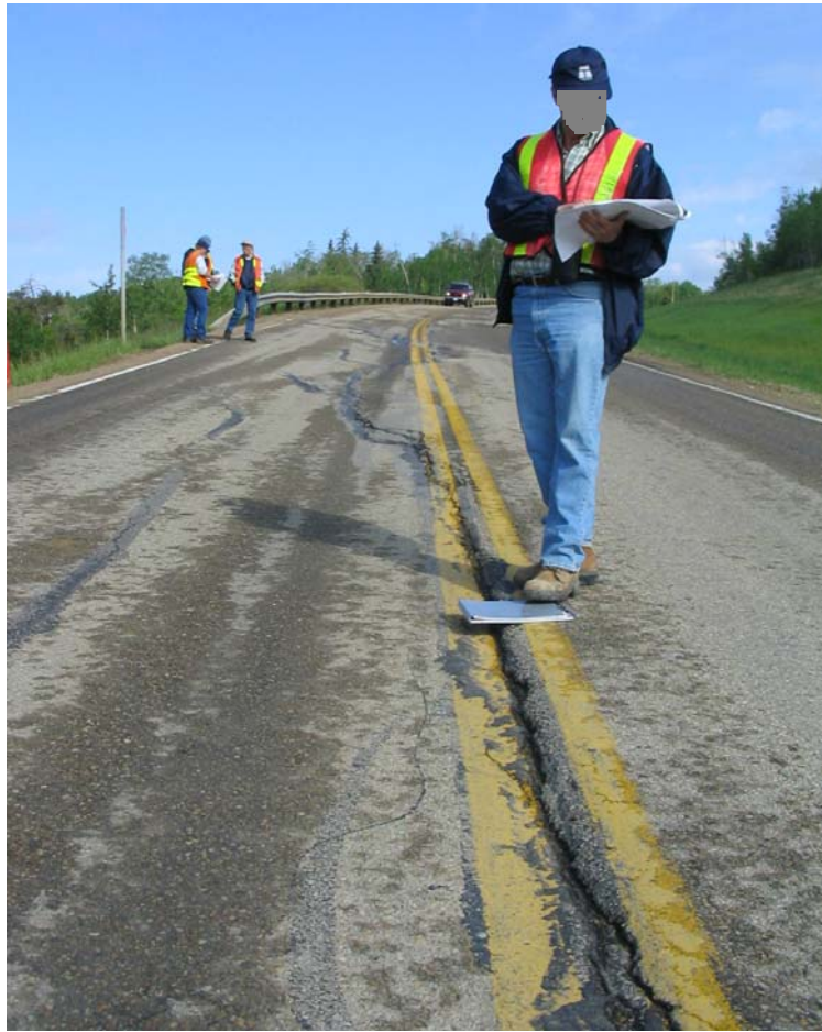
Mid-hill slide differential height across the crack.
