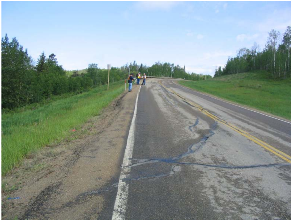
Mid hill slide – looking west.
