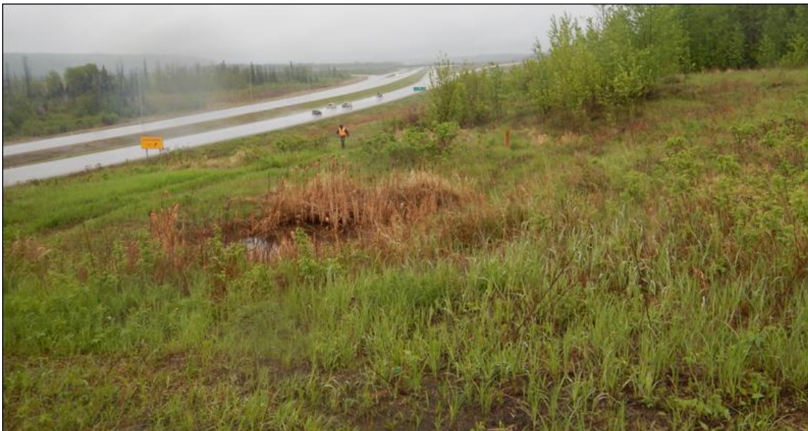
Photo No. 4 – Looking south at a vegetated scarp cack of the lower backslope slide
