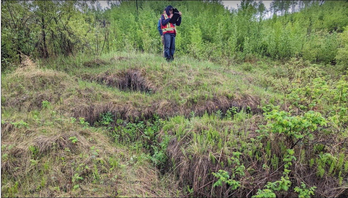
Photo No. 7 – Multiple tension cracks within the toe of the upper north slump
