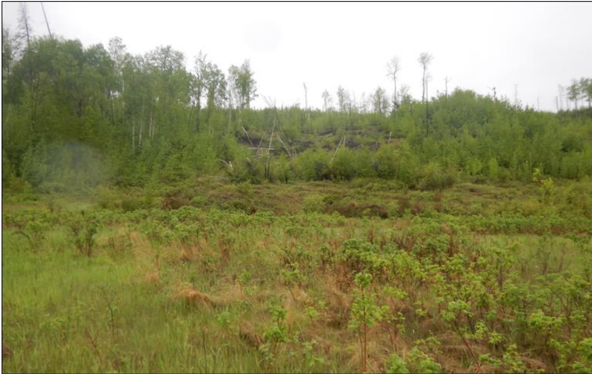
Photo No. 5 – Looking west at the upper backslope slump areas and toe rolls
