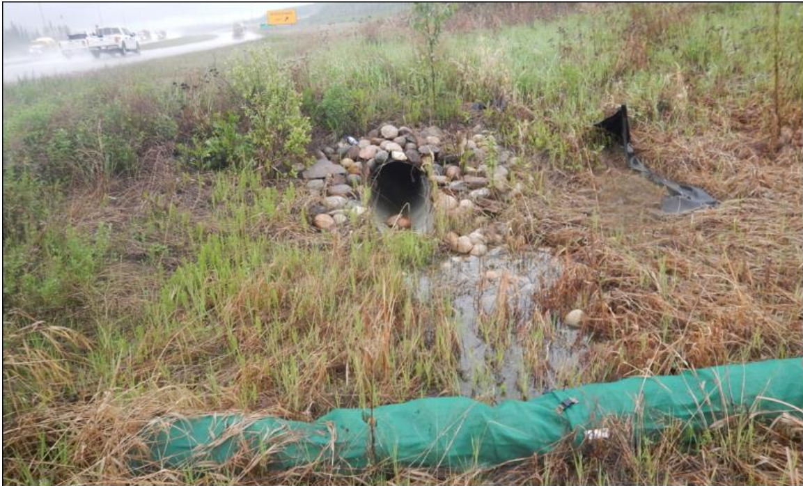
Photo No. 1 – Looking at the inlet of the culvert installed in the highway ditch below the lower landslide toe roll; water is slightly ponding at the culvert inlet location
