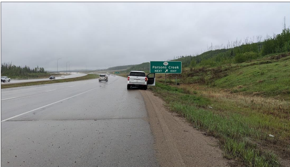
Photo No. 2 – Looking south at NC017A-2 landslide mass toppling over culvert in the ditch
