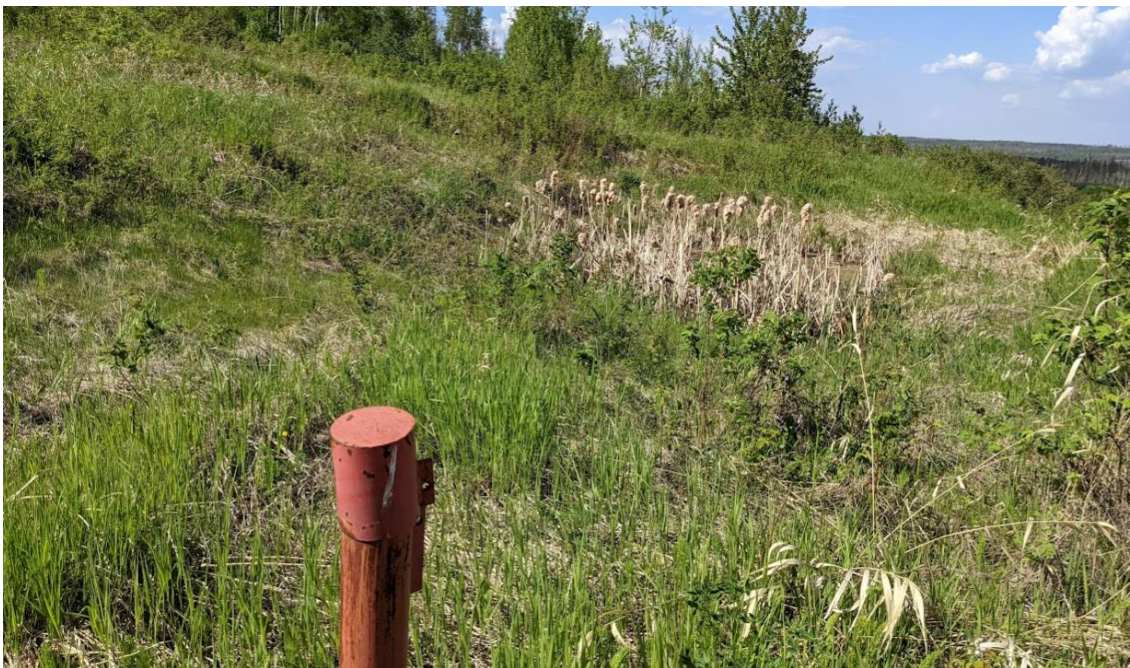
Photo No. 10 – Looking north at head scarp crack of the lower backslope landslide; more vegetation grew within the landslide mass
