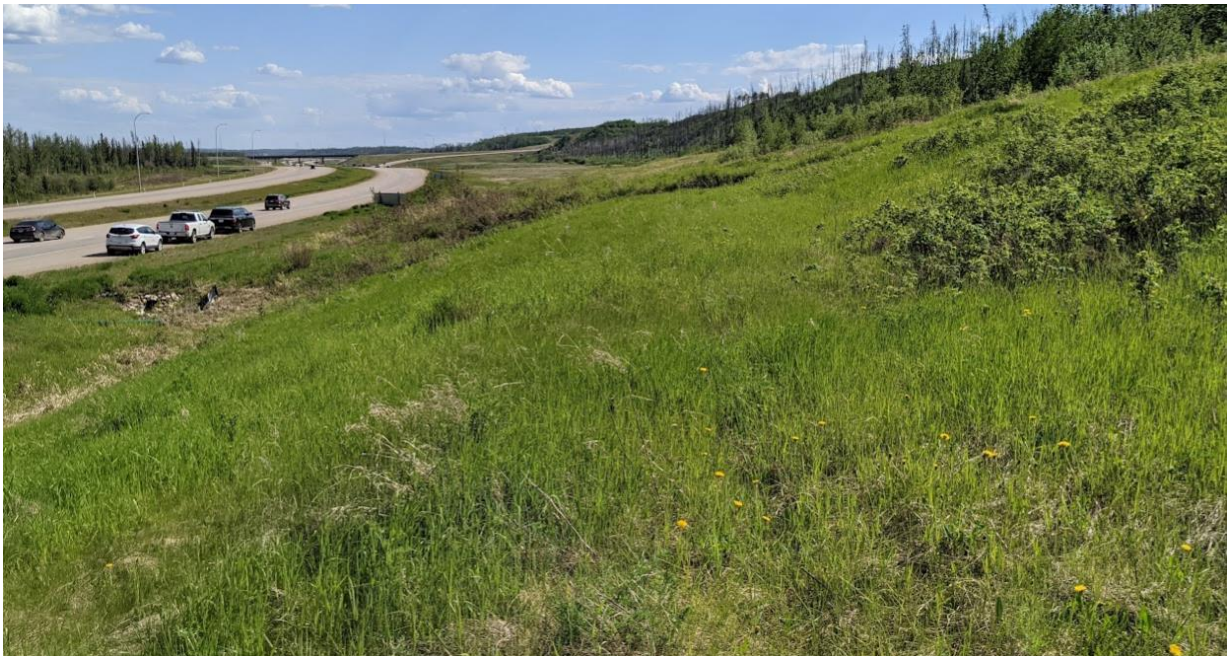
Photo No. 4 – Looking southeast at a scarp cack of the lower backslope slide
