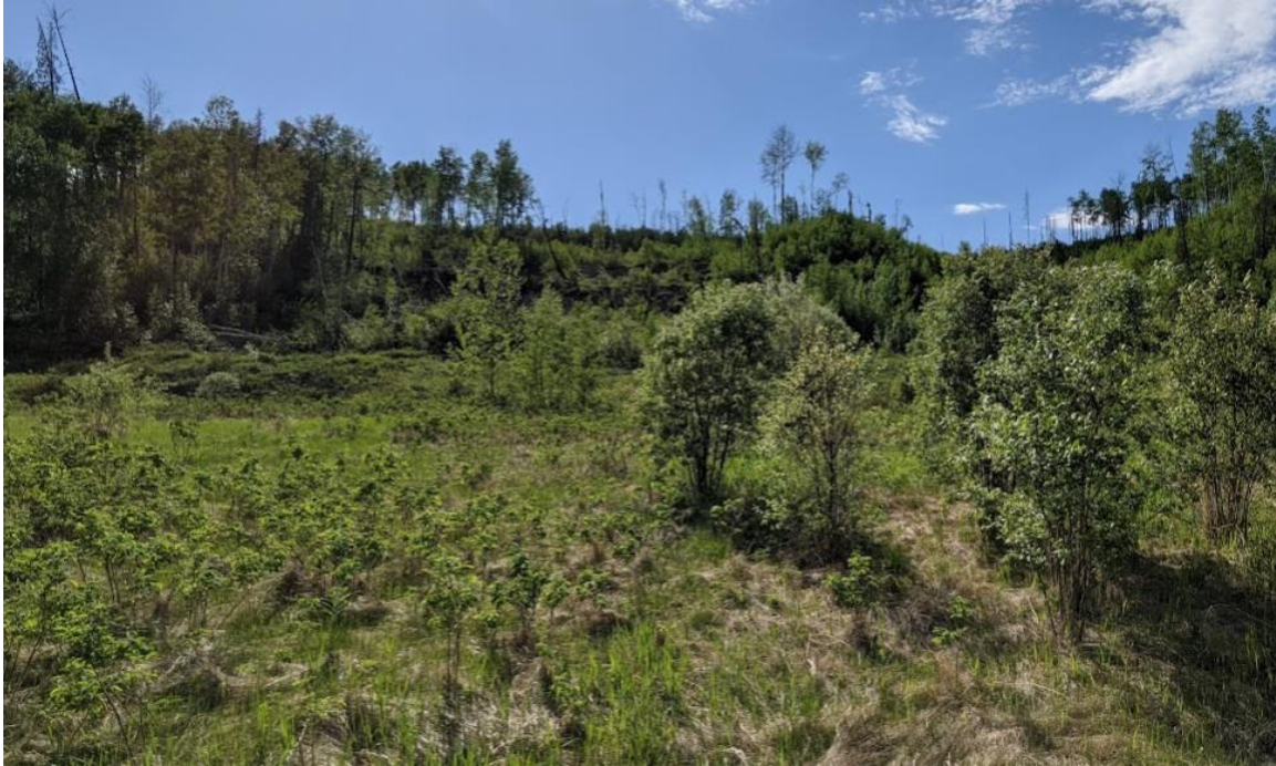
Photo No. 7 – Looking northwest at the head scarp cracks of the upper backslope slump
