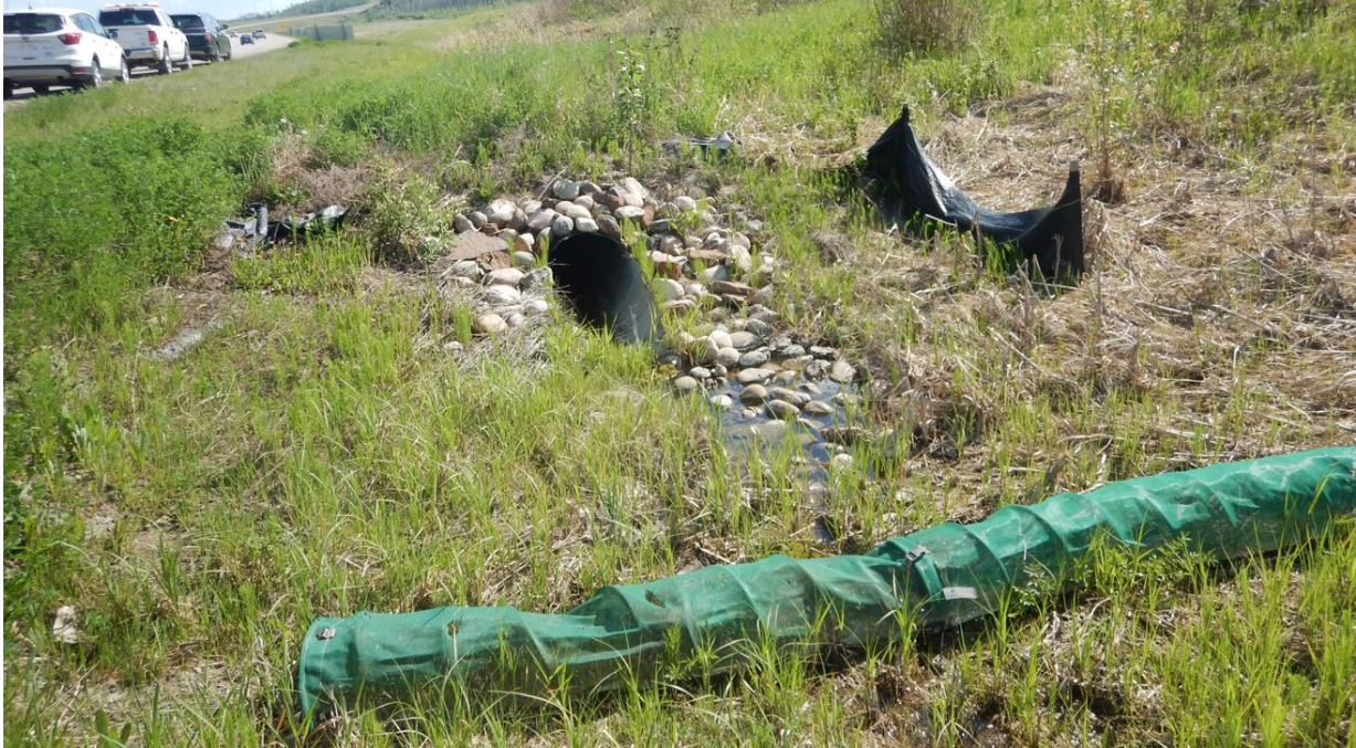
Photo No. 1 – Looking at the inlet of the culvert installed in the highway ditch below the lower landslide toe roll; water is slightly ponding at the culvert inlet location
