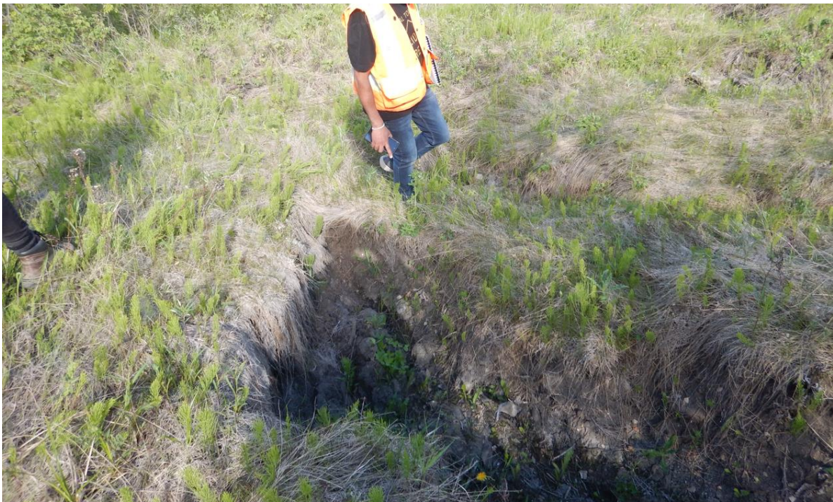
Photo No. 8 – Looking at a tension crack within the toe of the upper north slump; the tension crack is 1 m wide x 1 m deep; note seepage at depth of 0.5 m
