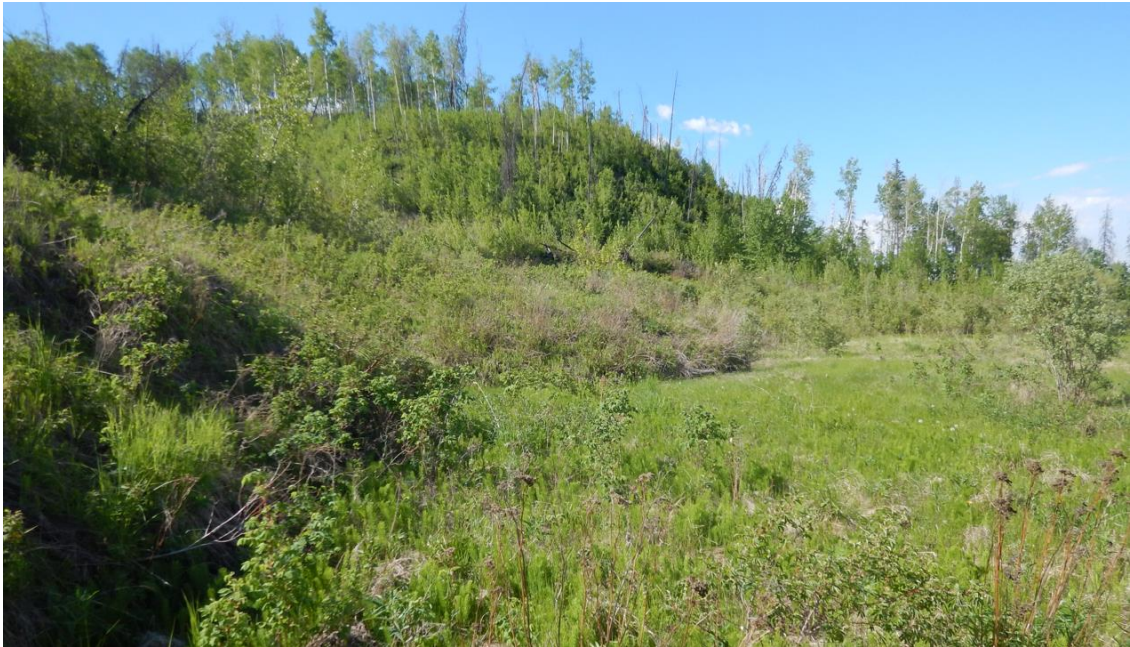
Photo No. 9 – Looking north at a 3 m high toe roll; the toe roll moved about 5 m to the east and buried TH99-12
