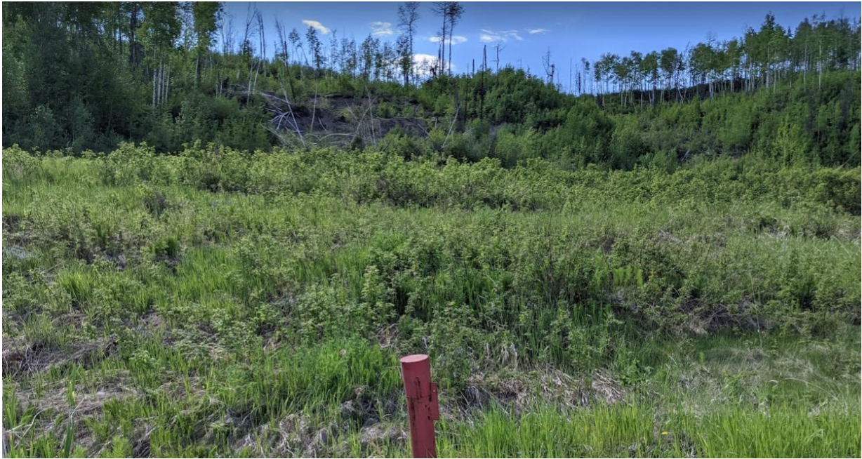
Photo No. 5 – Looking at the upper backslope slump areas and toe rolls
