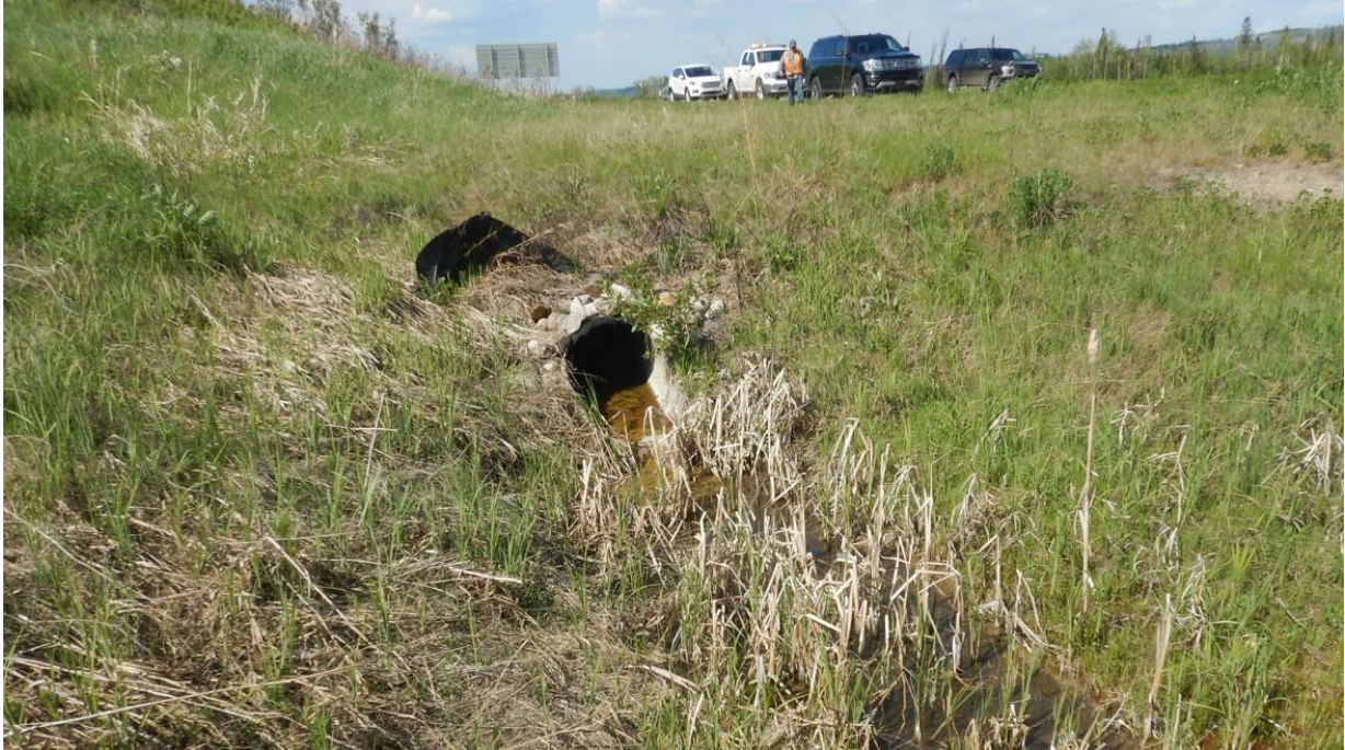
Photo No. 3 – Looking north at culvert outlet; more vegetation grew in ditch and water ponding at outlet in 2022
