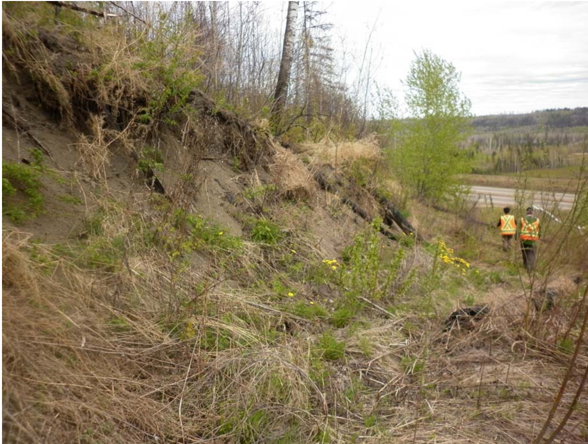
Photo 6 – Looking at the flank of the upper backslope north slump
