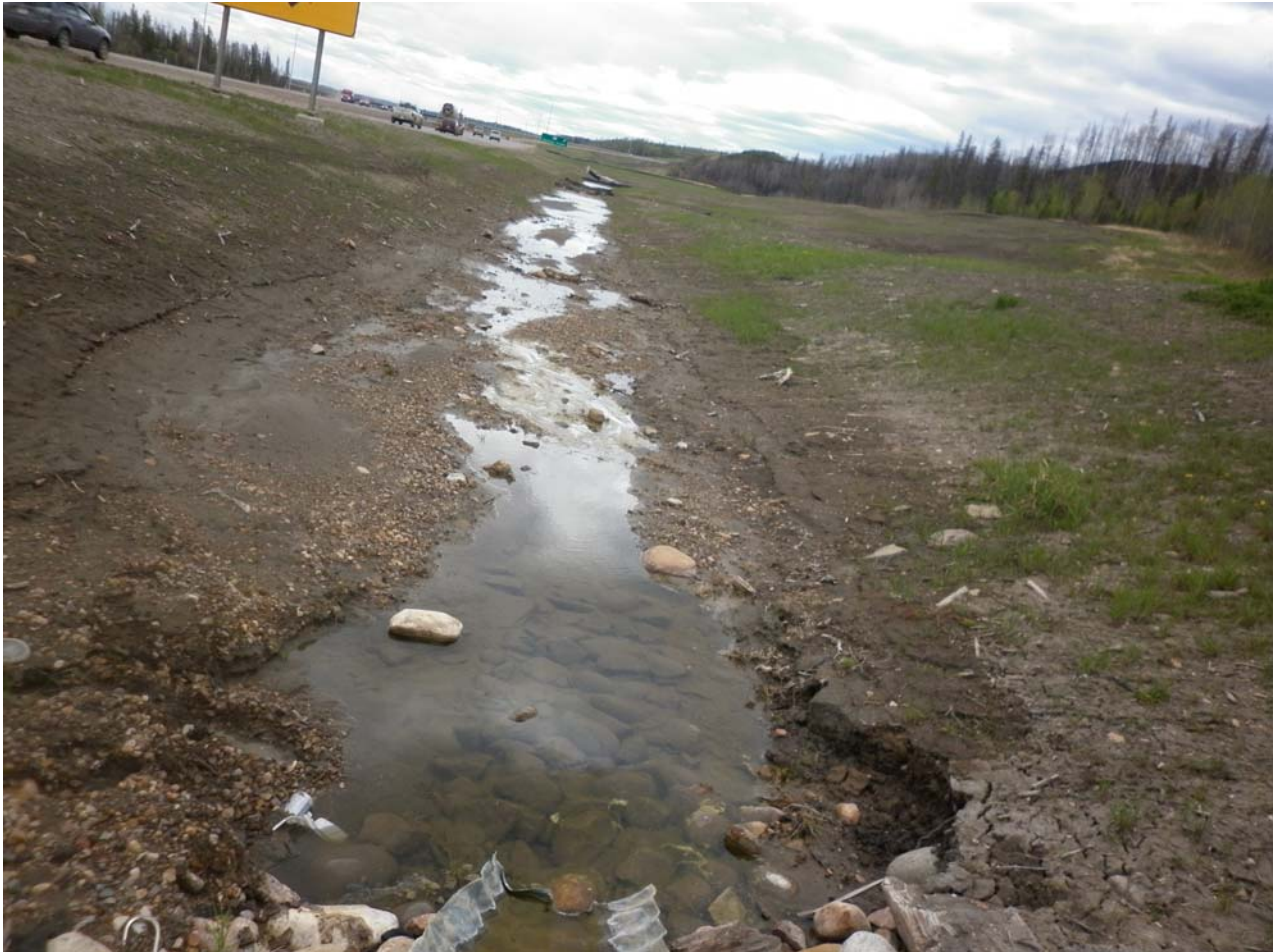
Photo 4 – Water ponding at the culvert outlet and along the ditch (Looking South)
