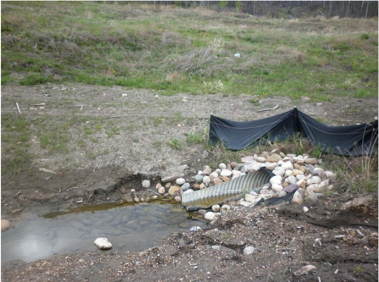
Photo 3 – Minor erosion and standing water around culvert outlet
