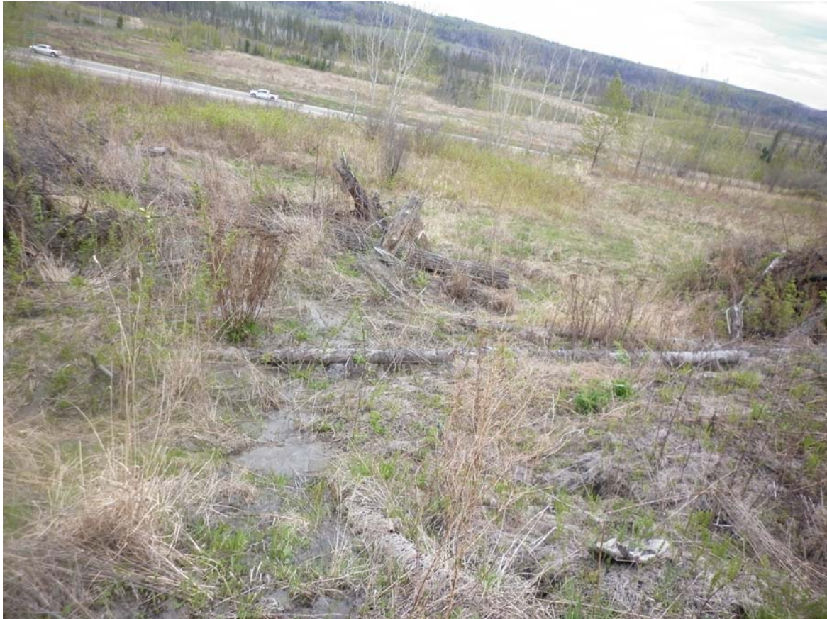
Photo 7 – Fast seepage near the northern flank of the upper backslope north slump (Looking East)
