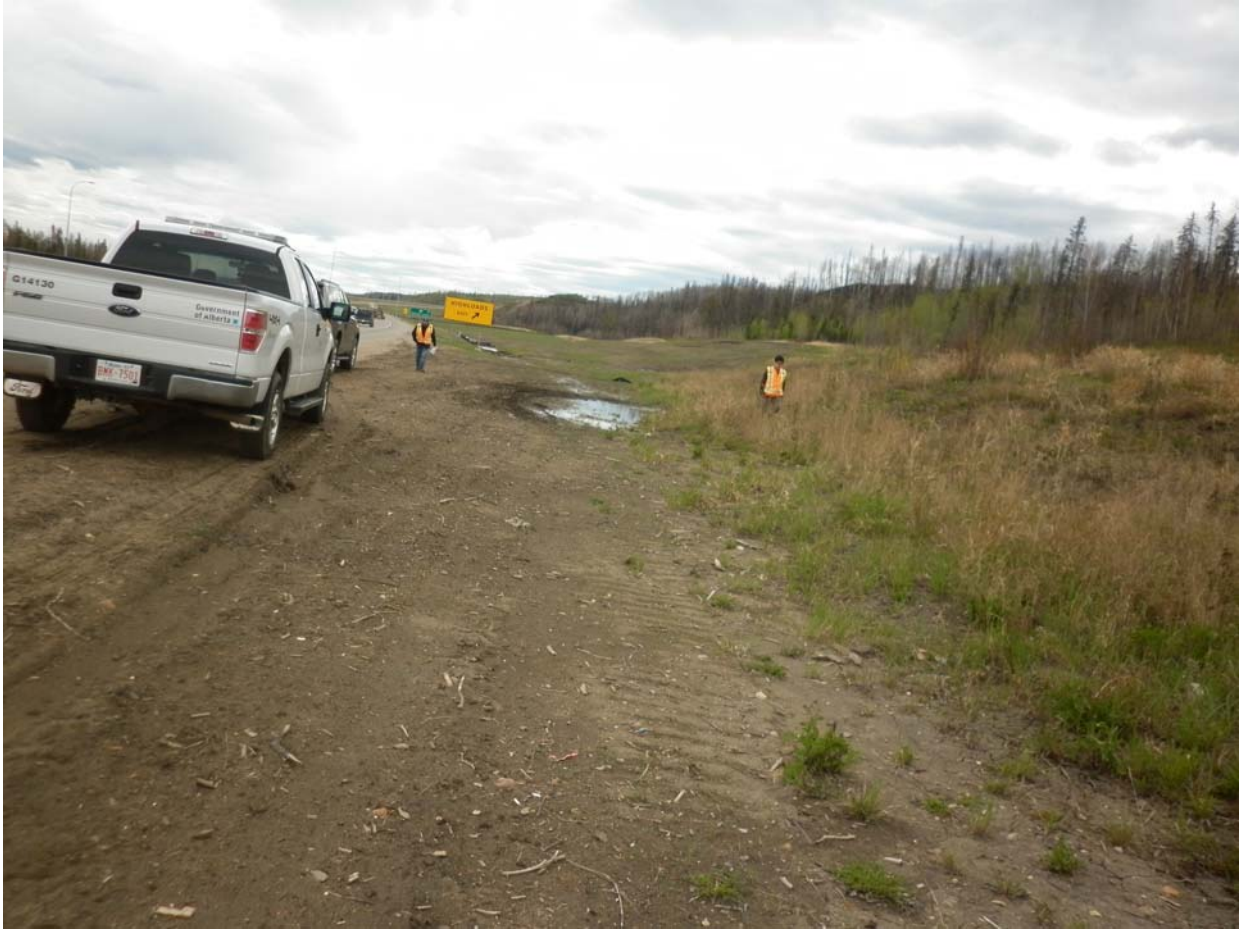
Photo 2 – Ponding water between the highway and the toe of the landslide (Looking South); note that the highway side slopes are bare of vegetation
