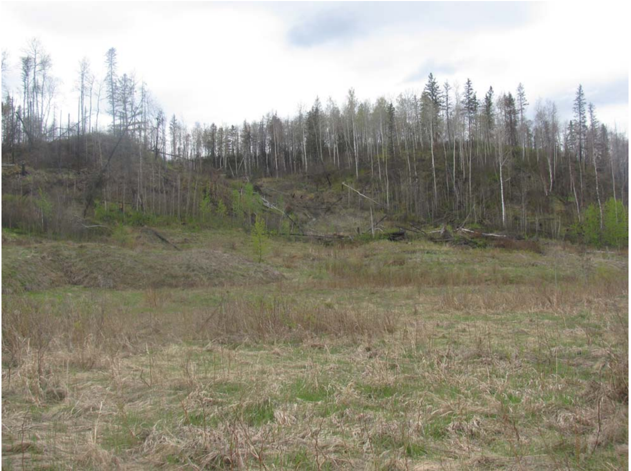
Photo 5 – Looking at the upper backslope slump areas and toe rolls
