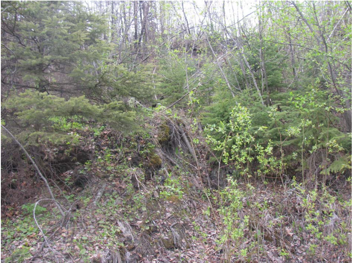
Photo 5a – Looking at the flank of the upper backslope south slump
