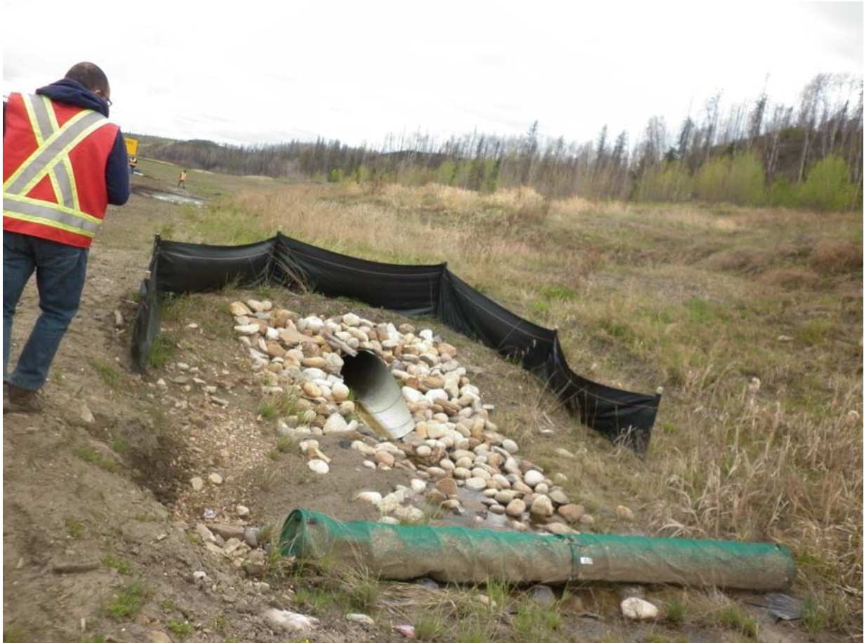
Photo 1 – Looking at the inlet of the culvert installed in the highway ditch below the lower landslide toe roll
