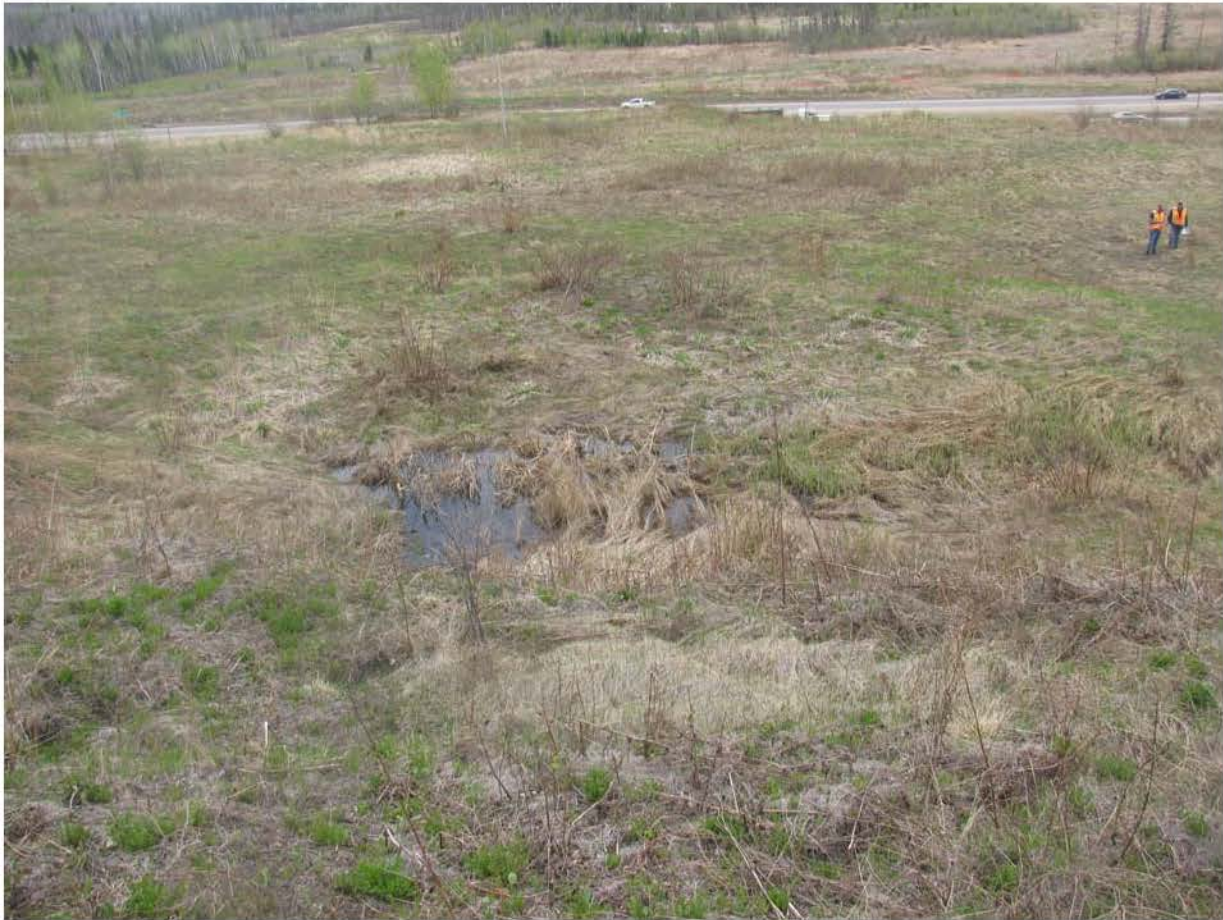
Photo 8 – Ponding water near the toe of the north slump (Looking East)
