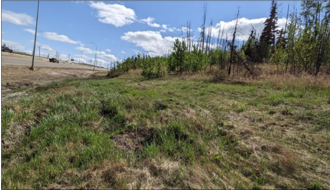
Photo 3. Looking south at the toe of the landslide; note tilting trees within the landslide mass
