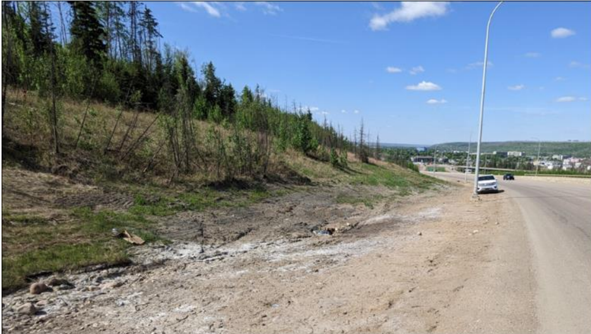
Photo 1. Looking north at the toe of the landslide; the landslide is toeing out above the ditch near culvert C6
