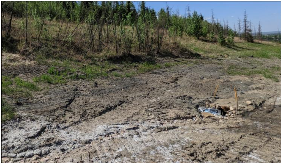
Photo 2. Previously noted erosion gully, downslope of the toe of the landslide at culvert inlet location, was filled and graded. Note garbage accumulation at the culvert inlet
