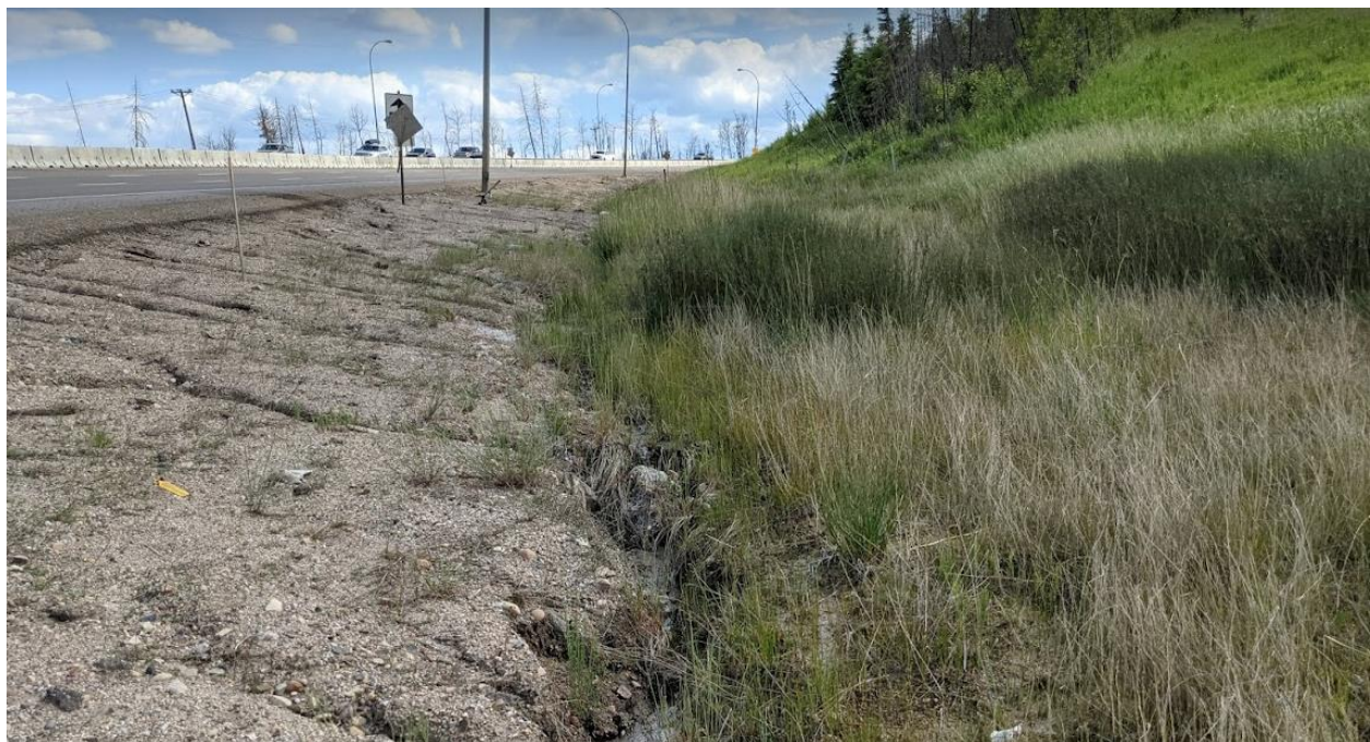
Photo No.3 –Looking south at the toe of the landslide; note tilting trees within the landslide mass
