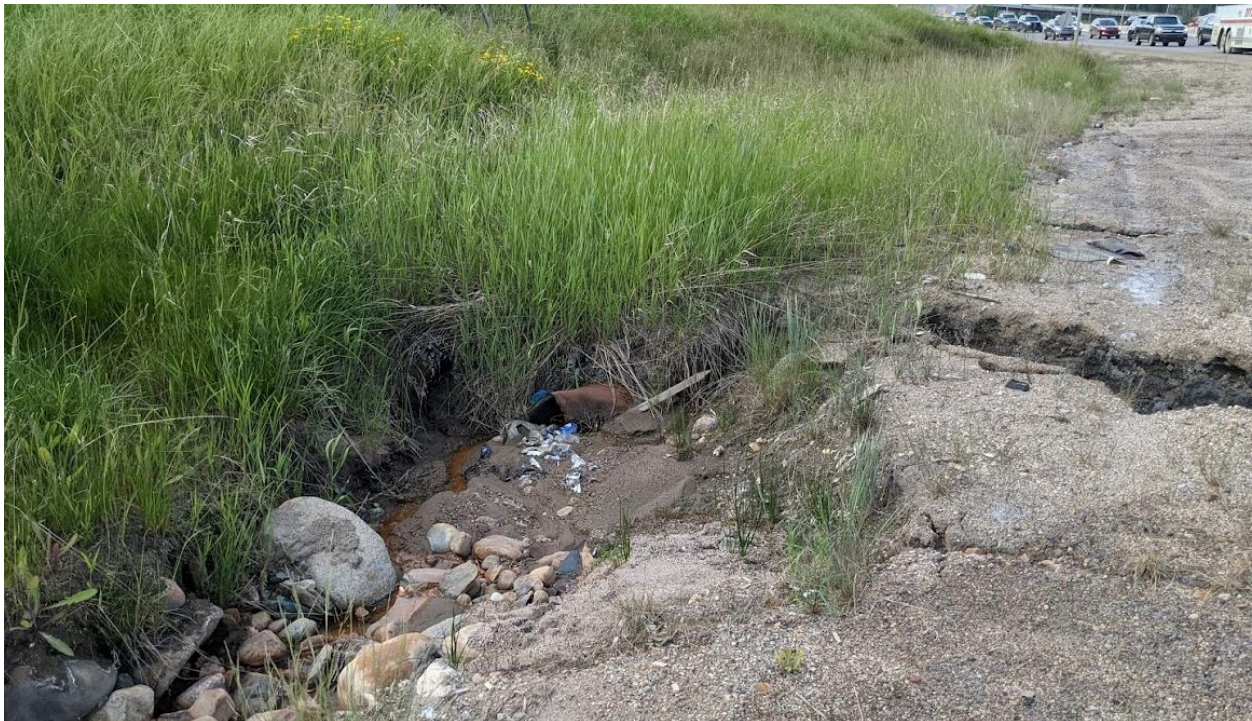
Photo No.2 – Erosion gully downslope of the toe of the landslide at culvert inlet location (Looking West)
