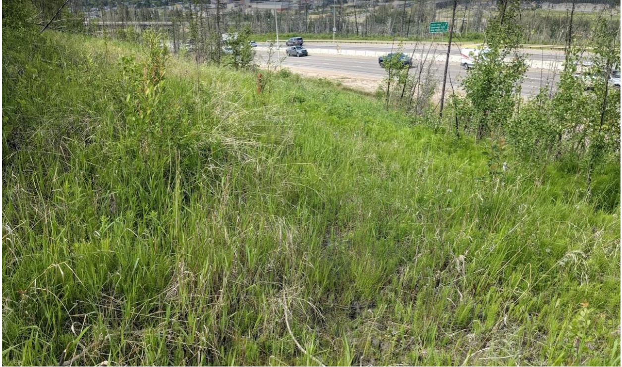
Photo No.4 –Looking north at S117-4; landslide mass is well vegetated
