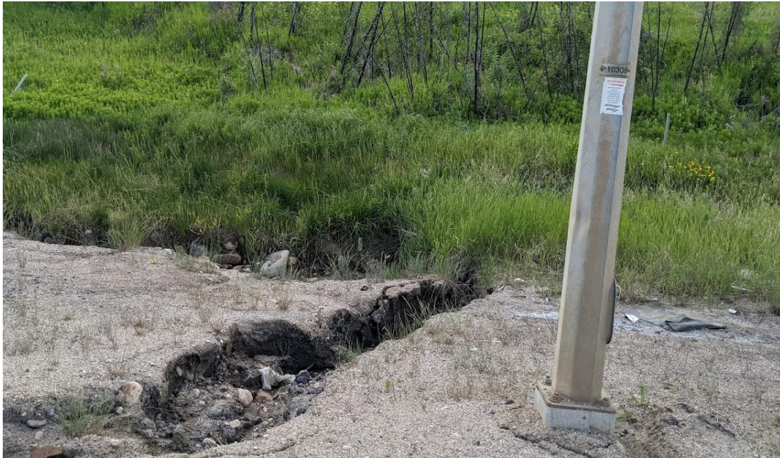
Photo No.2a – Severe erosion gully on the highway side slope to the east of the culvert inlet location (Looking east)
