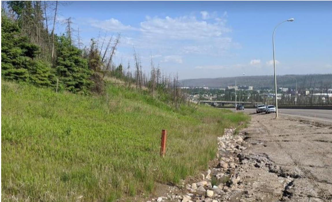
Photo No.1 – Looking north at the toe of the landslide; the landslide is toeing out above the ditch near culvert C6
