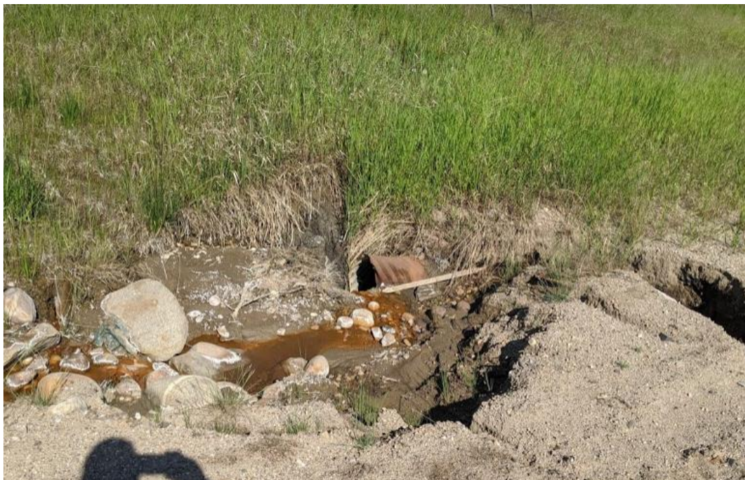
Photo No.2 – Erosion gully downslope of the toe of the landslide at culvert inlet location (Looking West)
