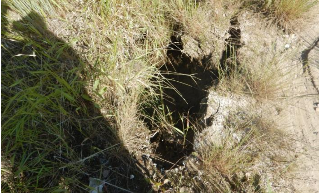
Photo No.6 –Sinkhole (1.3 m long x 0.8 m wide x 0.6 m deep) developed at the base of the backslope
