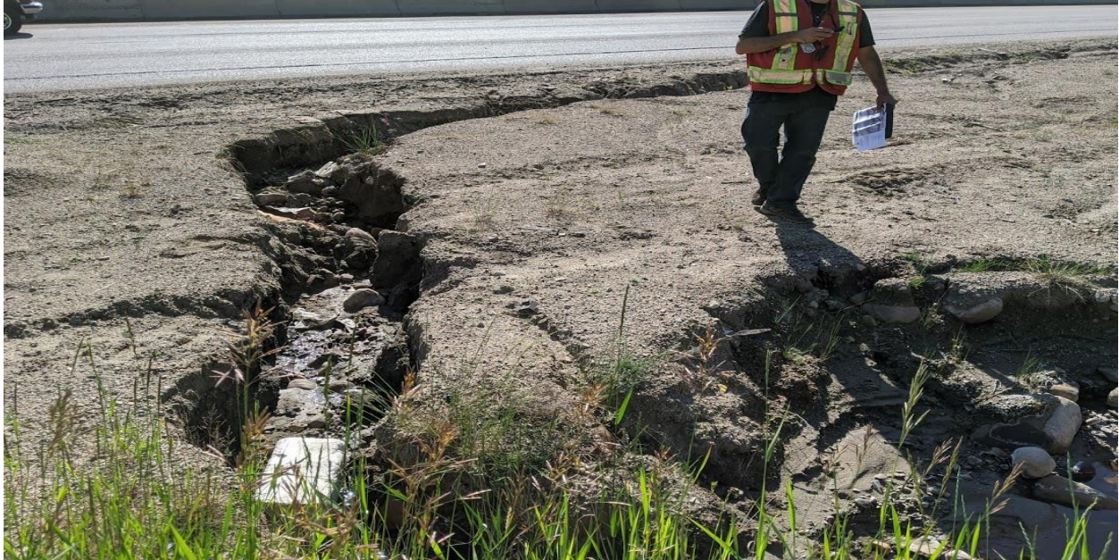
Photo No.2a – Severe erosion gully on the highway side slope to the east of the culvert inlet location (Looking east)
