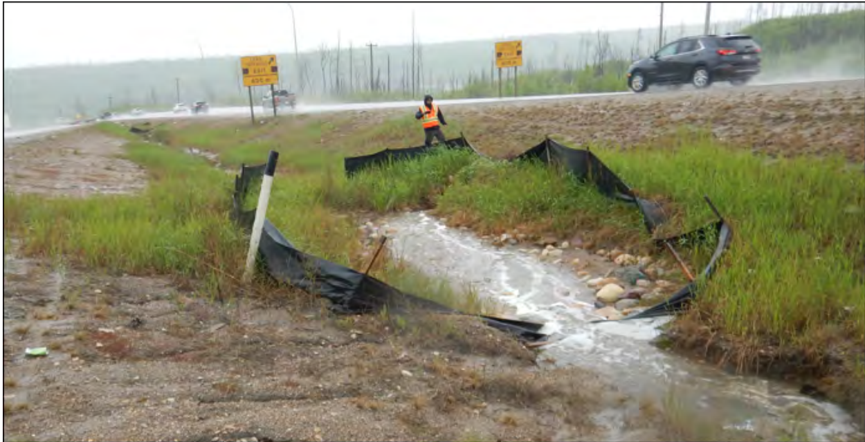
Photo 3 - 600 mm diameter SWSP culvert inlet (C5b; liner installed within the original C5b pipe).
