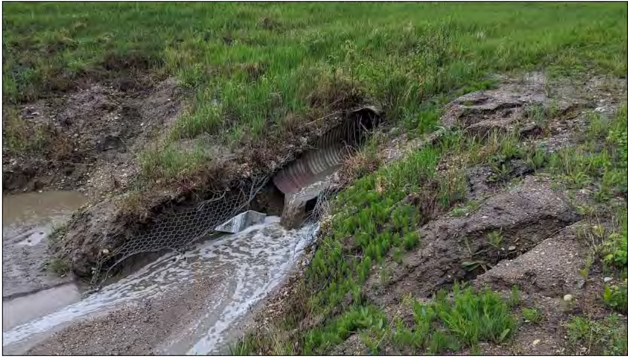
Photo 17 – Culvert C4 (1200 mm outlet); scour under the culvert; steady flow from the outlet.
