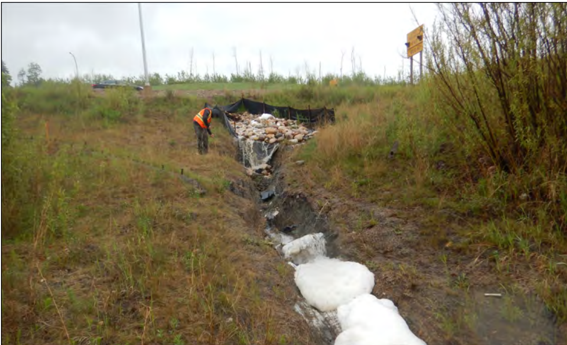
Photo 6 – Looking at a severe erosion gully downslope of the culvert C5b outlet location.
