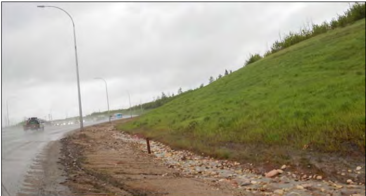
Photo 8c – Bare side slopes and minor erosion rills
