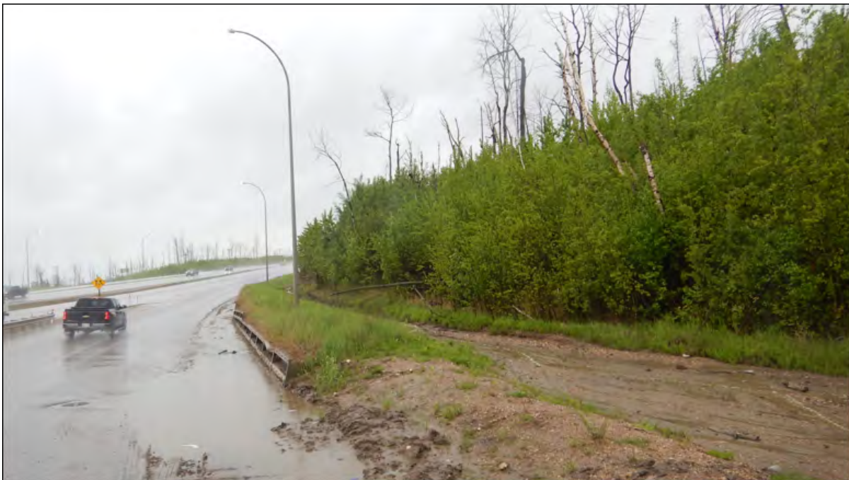
Photo 14 –Surface water from the road is ponding against the bin wall; roadway MHs 2 to 4 by the bin wall may have also been partially filled with sediment; sand and salt piles near the north end of the wall may have also dammed the water at this location.
