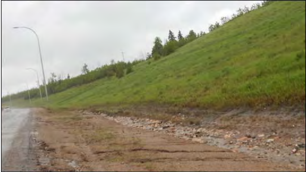
Photo 8b – Bare side slopes and minor erosion rills
