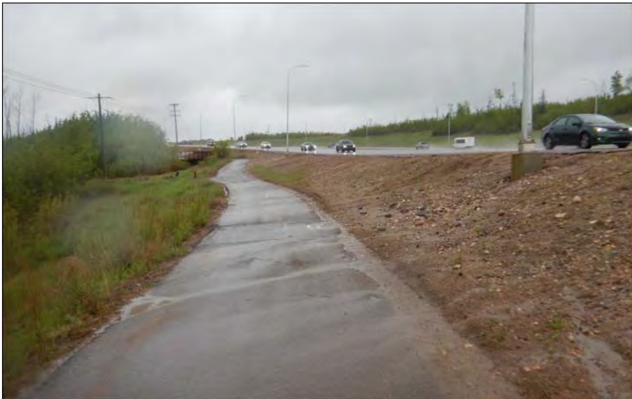
Photo 4 – Asphalt walking trail settlement/distress in response to the failed attempts to replace C5b.
