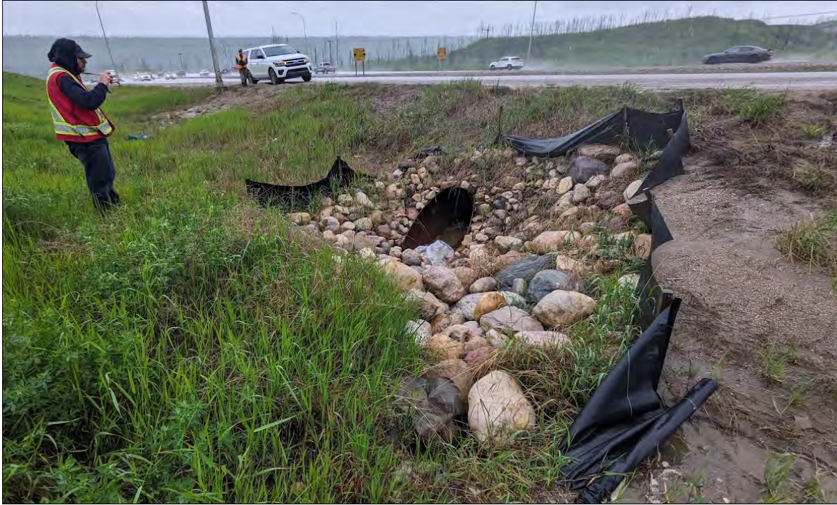
Photo 1 – Looking at the inlet of the 900 mm diameter SWSP culvert (C5a replacement).
