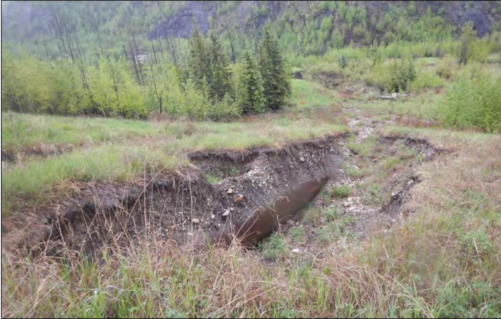
Photo 7 – Looking at erosion halfway down the hill exposing a buried SWSP trunk conveying the flow from the Culvert C5b to Saline Creek at the base of the valley
