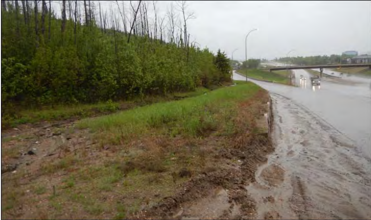
Photo No 13 – Manhole 5 is buried under sediment
