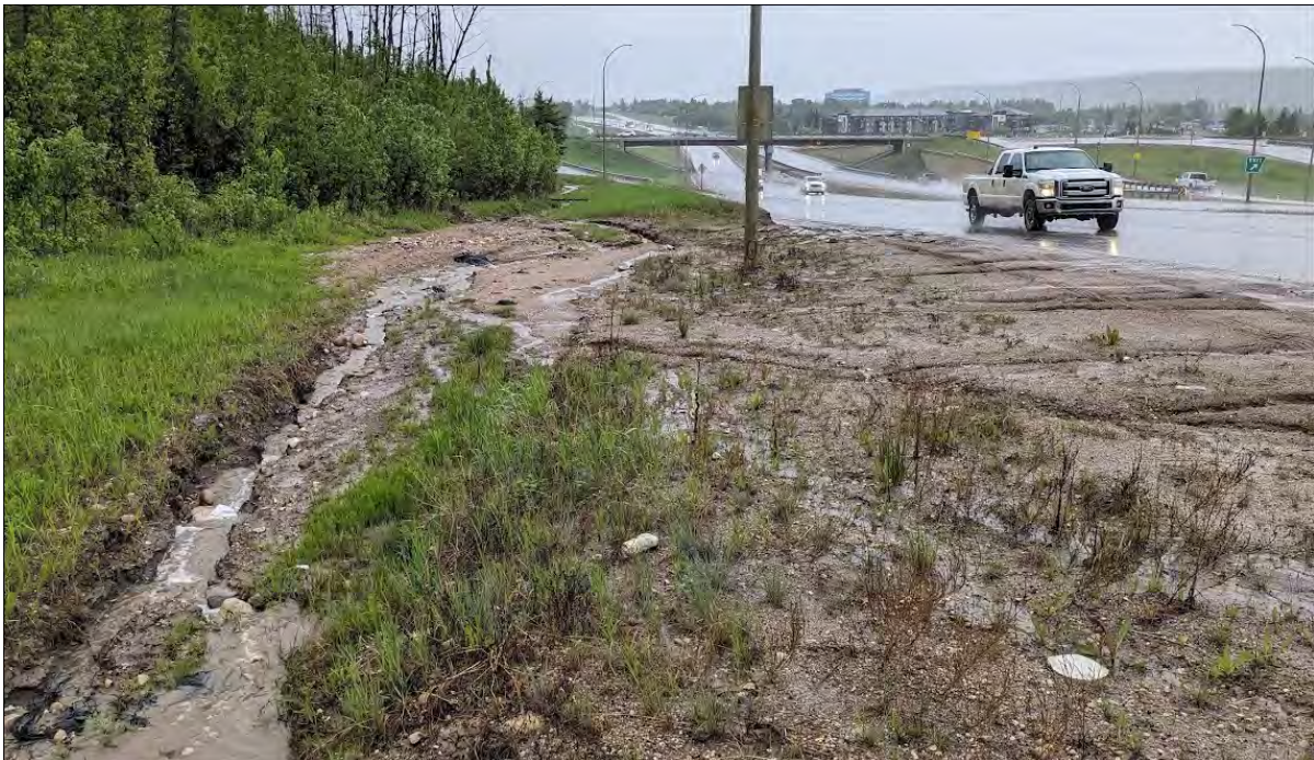
Photo 12 – Eroded ditch upstream of Jersey Wall
