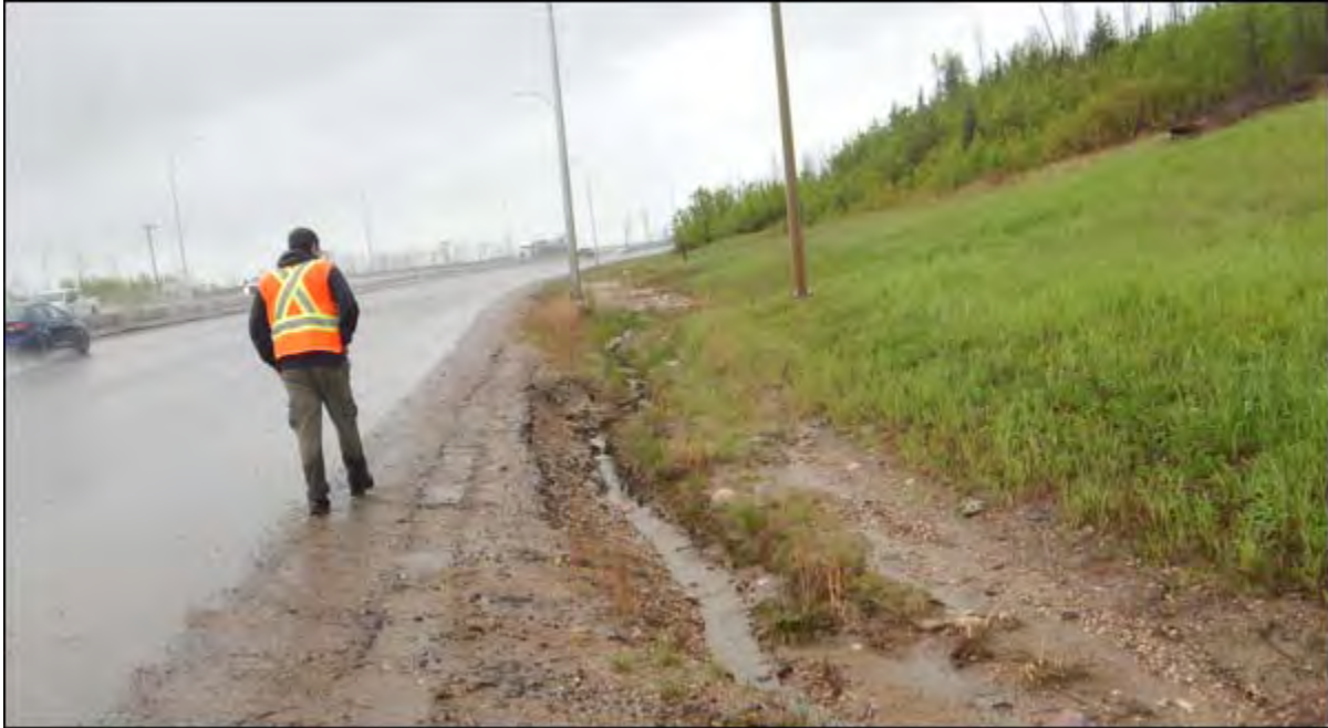
Photo 11 – Erosion gully less than 1.6 m wide by 0.9 m deep
