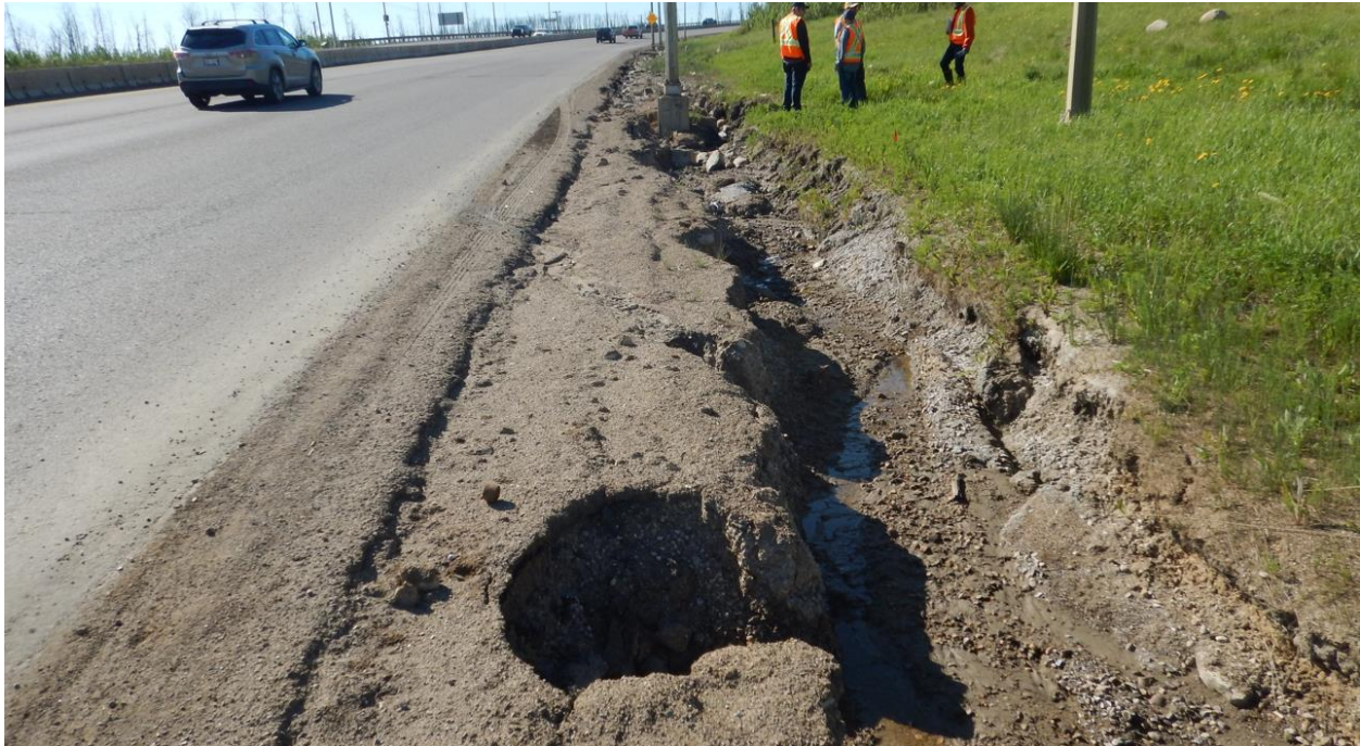
Photo 5 – Sinkhole 1m diameter by 0.6m deep and gully 3m wide by 1m deep.
