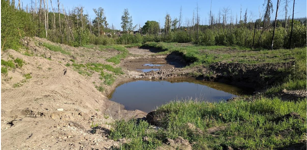
Photo 9 –AT cleaned the pond in the fall of 2021; substantial sediment removed to increase pond capacity.
