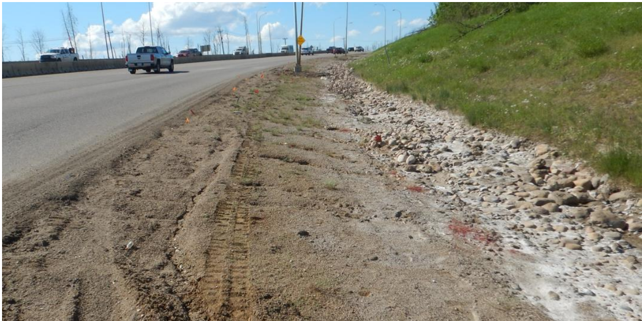
Photo 2c – Bare side slopes and erosion rills.
