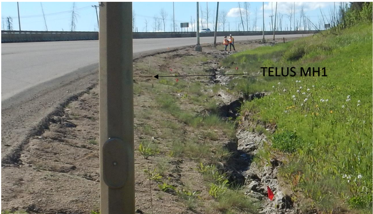
Photo 4 – Erosion, bare slopes. Drop structure DS2 completely buried under sediment.
