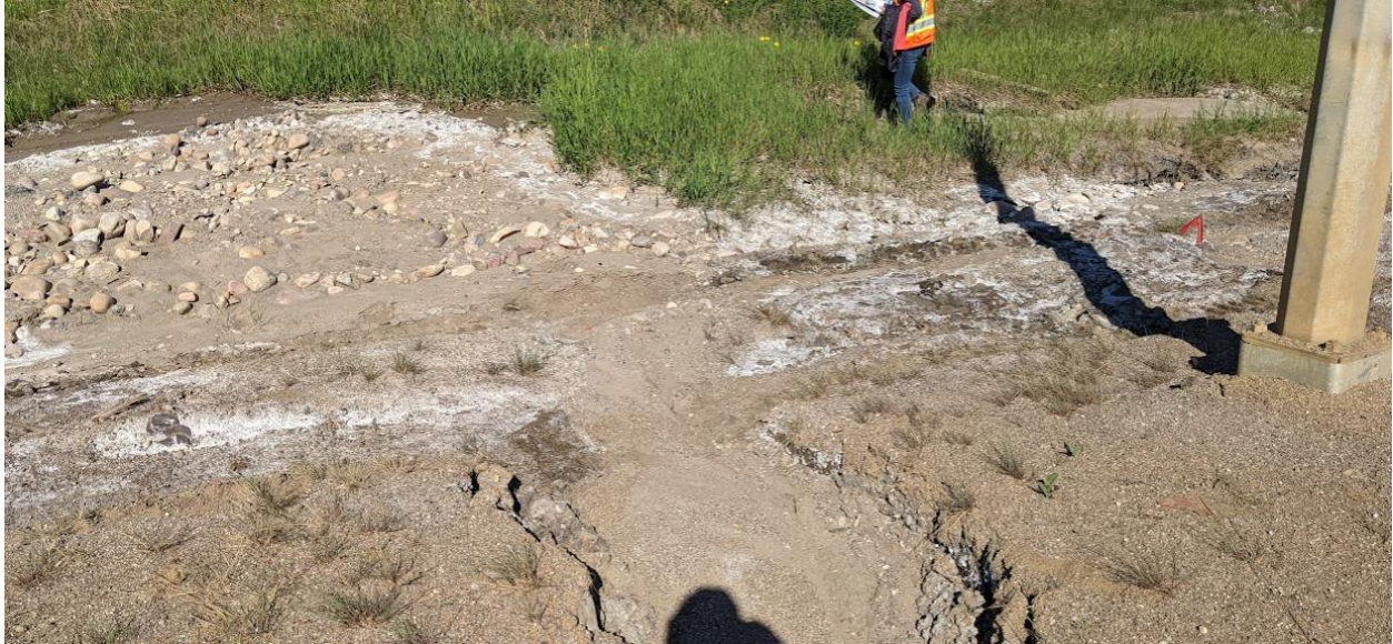
Photo 3 – Erosion developed on the highway side slope. Culvert C6 inlet buried under sediment.
