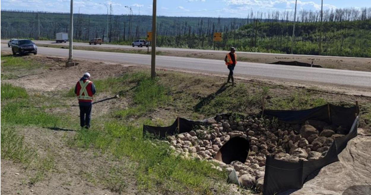
Photo 1 – Looking at the inlet of a new 900 mm diameter SWSP culvert (C5a replacement).
