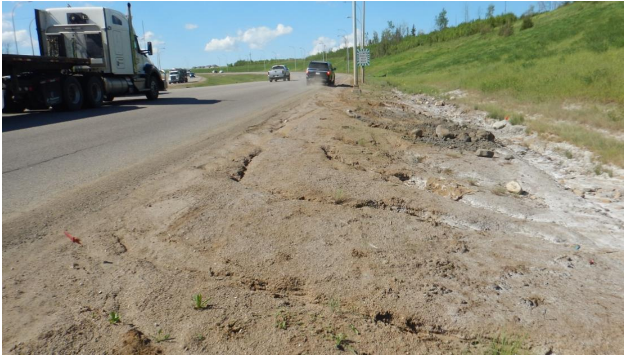
Photo 2b – Bare side slopes and erosion rills.
