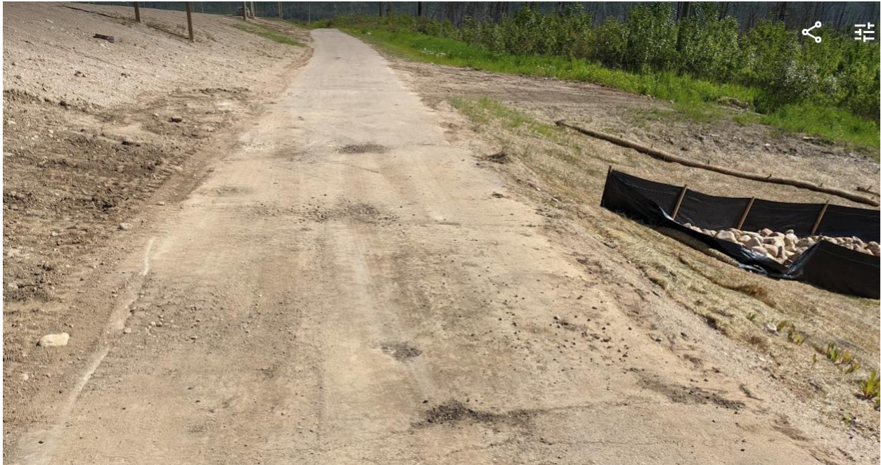
Photo 1e –Asphalt walking trail settlement/distress in response to the failed attempts to replace C5b.
