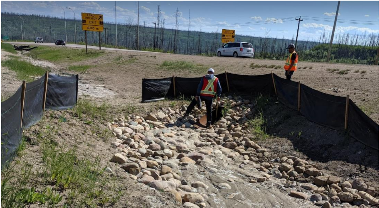
Photo 1c - 600 mm diameter SWSP culvert inlet (C5b; liner installed within the original C3b pipe).
