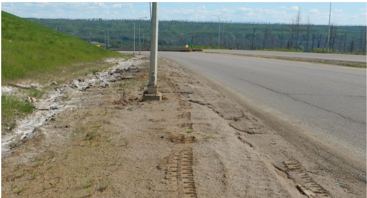
Photo 2 – Bare side slopes with erosion rills (looking north).
