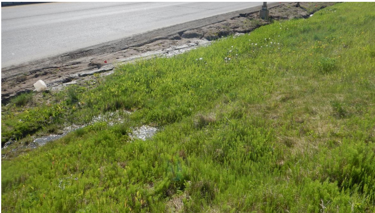
Photo 6 – Some seepage from the colluvium backslope flowing into eroded ditch.
