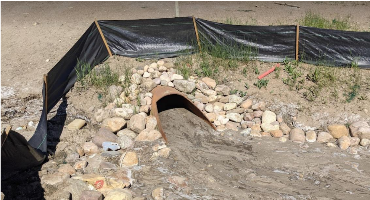
Photo 1b – Looking at the outlet of a new 900 mm diameter SWSP culvert (C5a replacement); Note the presence of sediment at the outlet of the new pipe; sediment covers a portion of the median ditch between the outlet of C5a and the inlet of C5b.
