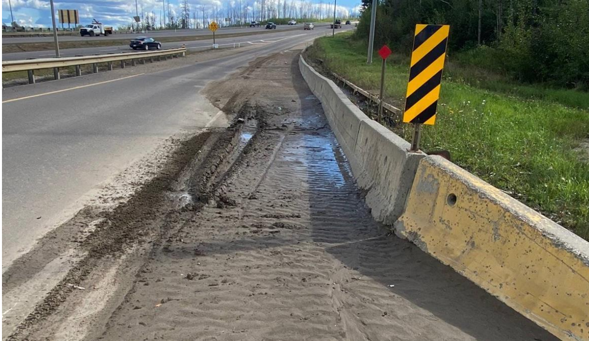
Photo 7 – Sediment accumulation on the highway by the Jersey barriers buried Manholes MH#1 and MH#5 (Photo received from AT after the June 8, 2022's site visit).
