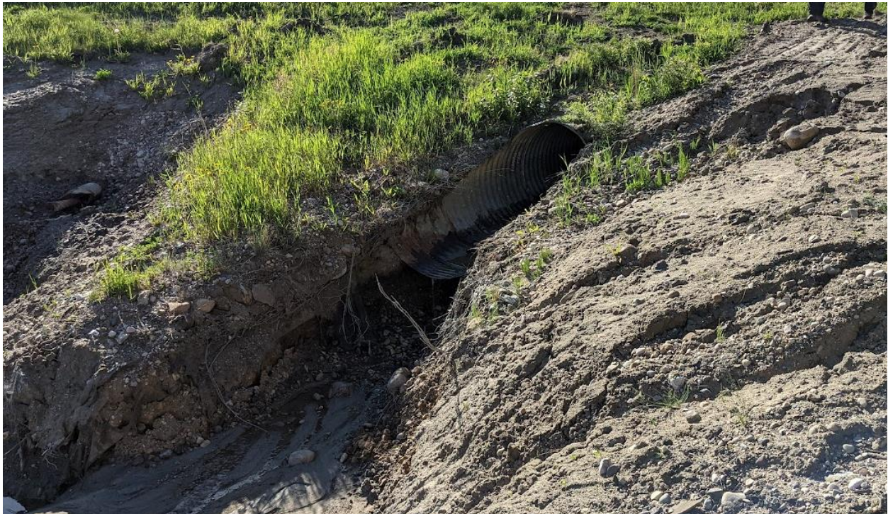
Photo 10 – Culvert C4 (1200 mm outlet); scour under the culvert; steady flow from the outlet.
