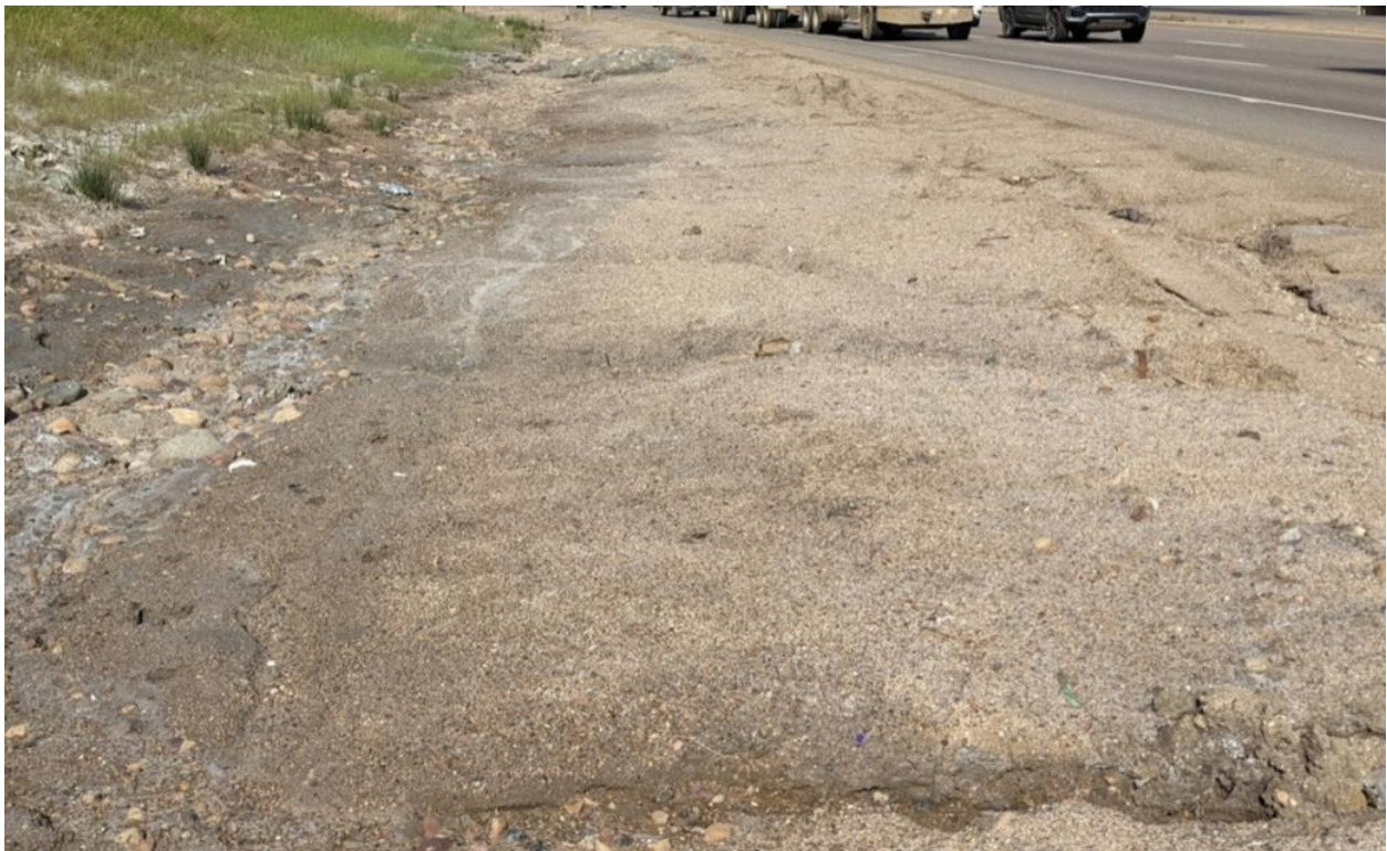
Photo 2b – Bare side slopes and erosion rills
