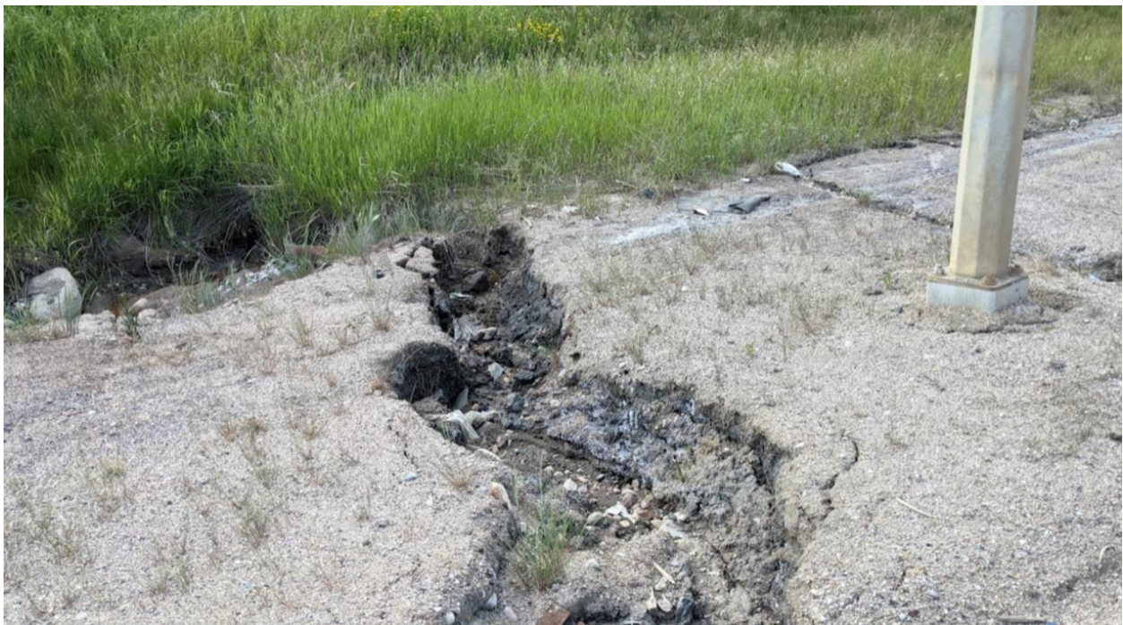
Photo 3 – Severe sediment accumulation and excessive erosion developed on the highway side slope near culvert C6 inlet location
