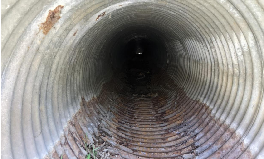
Photo 1c - 900 mm diameter CSP culvert (C5b) inlet. This culvert will be lined in 2021
