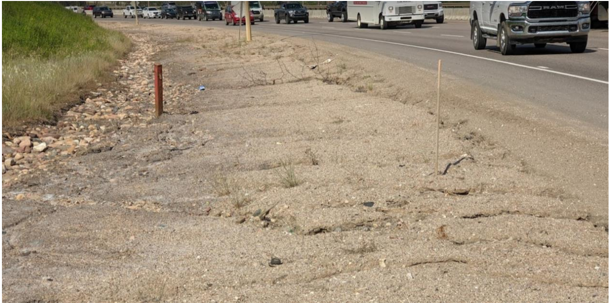
Photo 2c – Bare side slopes and erosion rills
