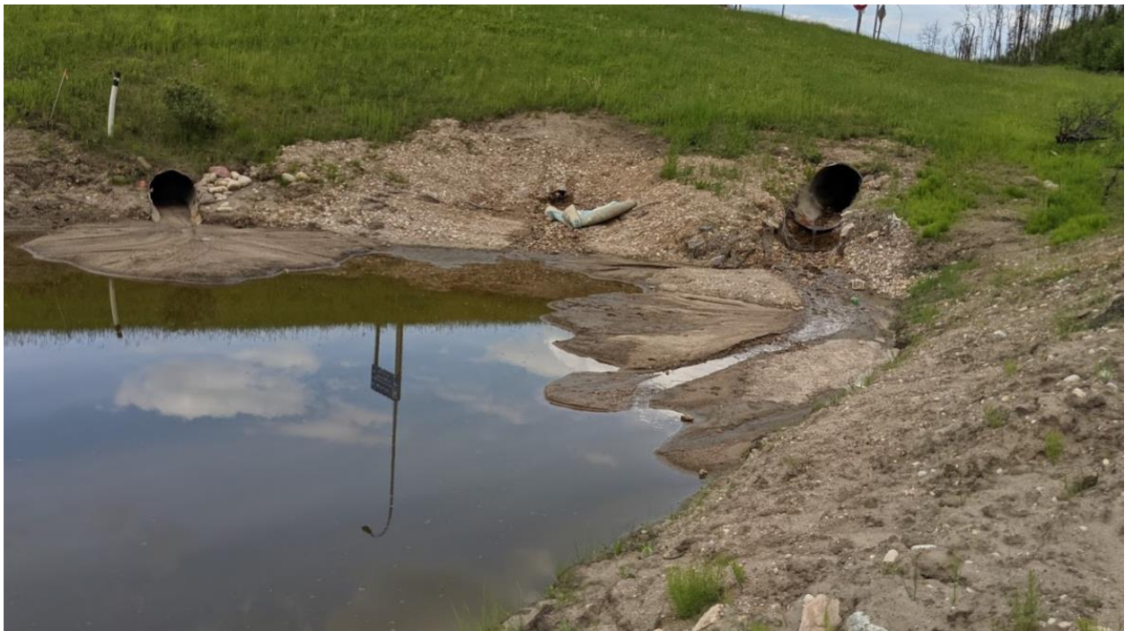
Photo 11 – Culvert C4 and C3 outlets; note sediment accumulation was partially removed from the inside of C4 (small culvert on the LHS of the photo); no flow on C4
