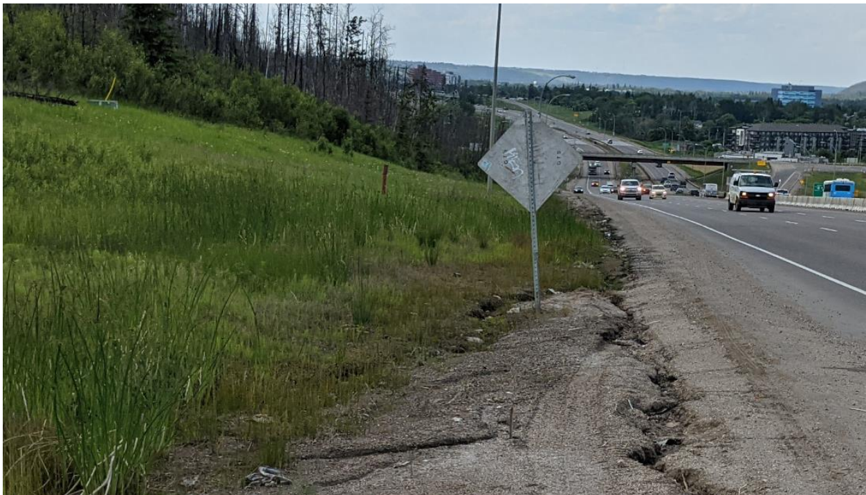
Photo 5 – Some seepage from the colluvium backslope flowing into eroded ditch
