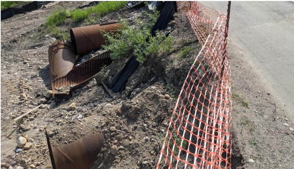
Photo 1d – 900 mm diameter CSP culvert (C5b) outlet. Inline Contracting had two unsuccessful attempts to replace the CSP culvert with a SWSP. The first attempt was to install the pipe 2m to the south of C5b, and the second attempt was to install the pipe 4 m to the north of C5b
