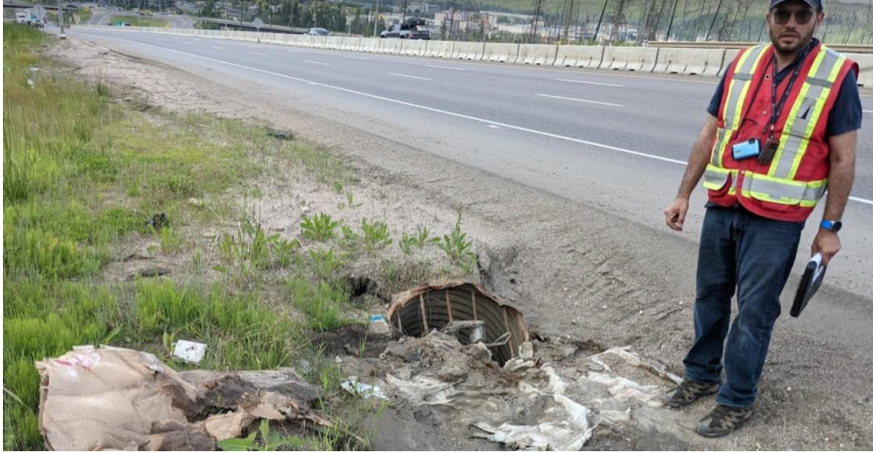
Photo 4 – Erosion , bare slopes, and debris near Drop structure DS2
