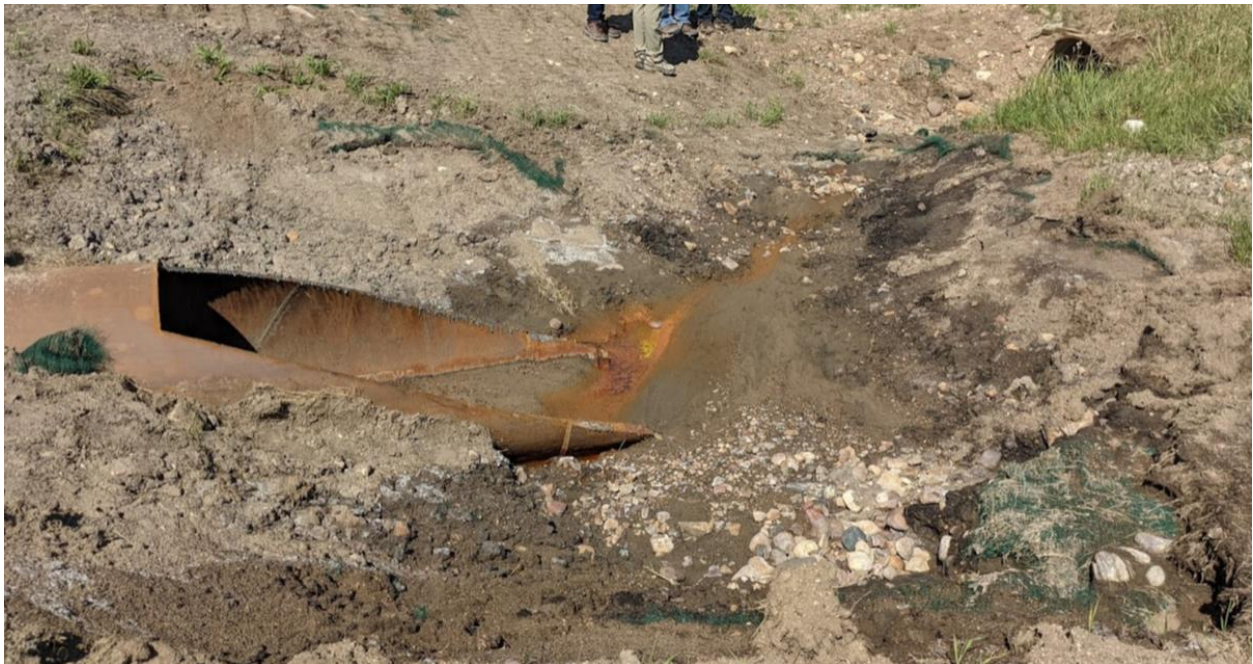
Photo 1b – Looking at the outlet of a new 900 mm diameter SWSP culvert (C5a replacement)
