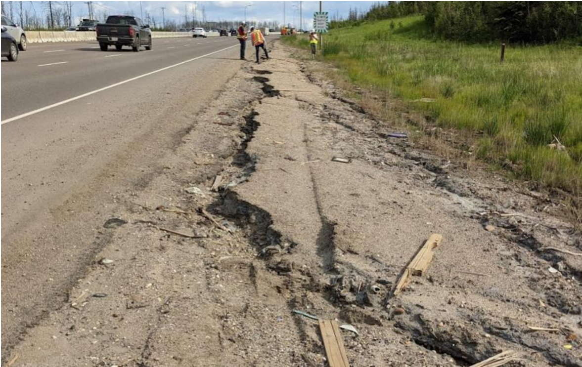
Photo 6 – Sediment accumulation in the highway side slope
