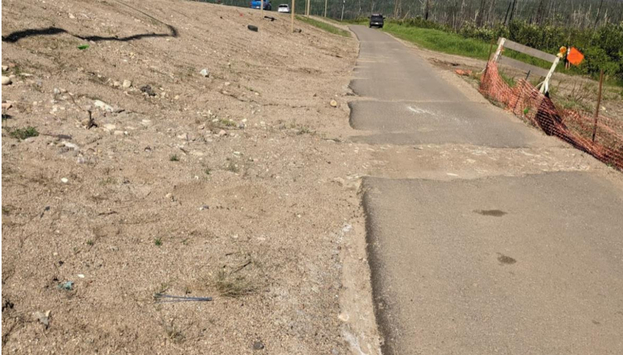
Photo 1e –Asphalt walking trail settlement/distress in response to the failed attempts to replace C5b
