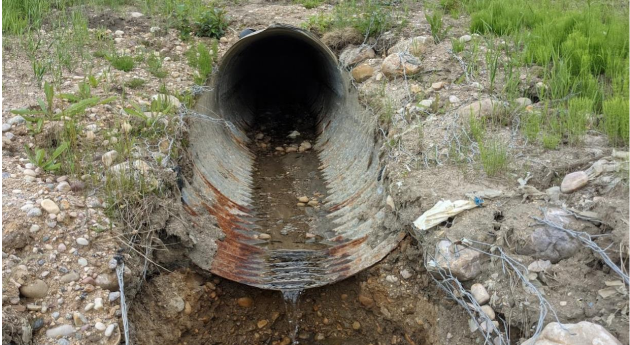
Photo 10 – Culvert C4 (1200 mm outlet); sediment removed from the culvert; steady flow from the outlet
