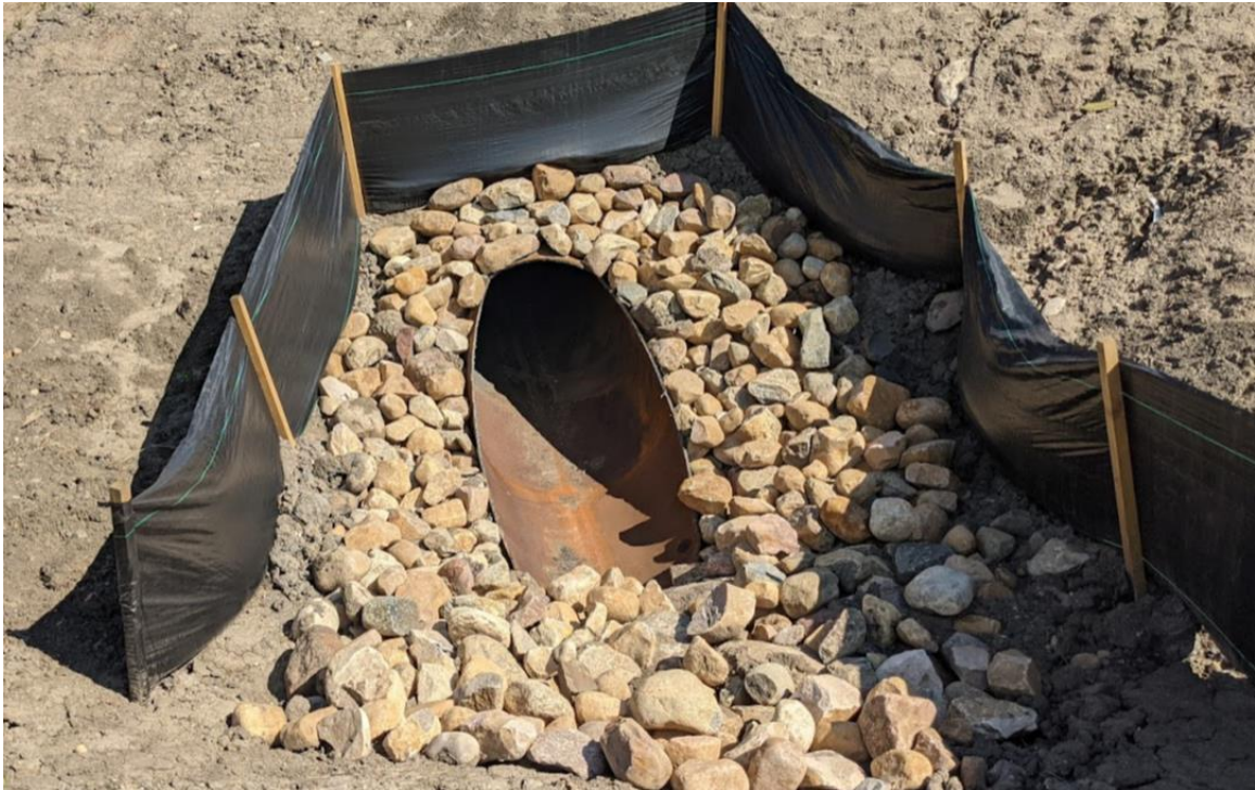
Photo 1 – Looking at the inlet of a new 900 mm diameter SWSP culvert (C5a replacement)
