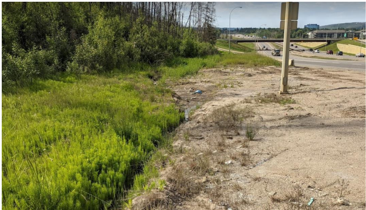
Photo 7 – Temporary berm and erosion gully along the back of bin and jersey walls
