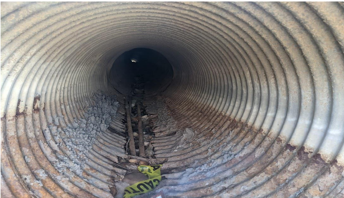
Photo 1f –Looking inside the C5b culvert from the outlet location; the culvert floor is excessively damaged, and rocks/debris are present within the culvert floor; the integrity of this culvert is questionable, and it will be lined in 2021 by Inline Contracting
