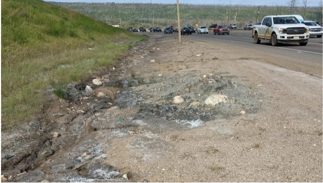
Photo 2 – Bare side slopes with erosion rills
