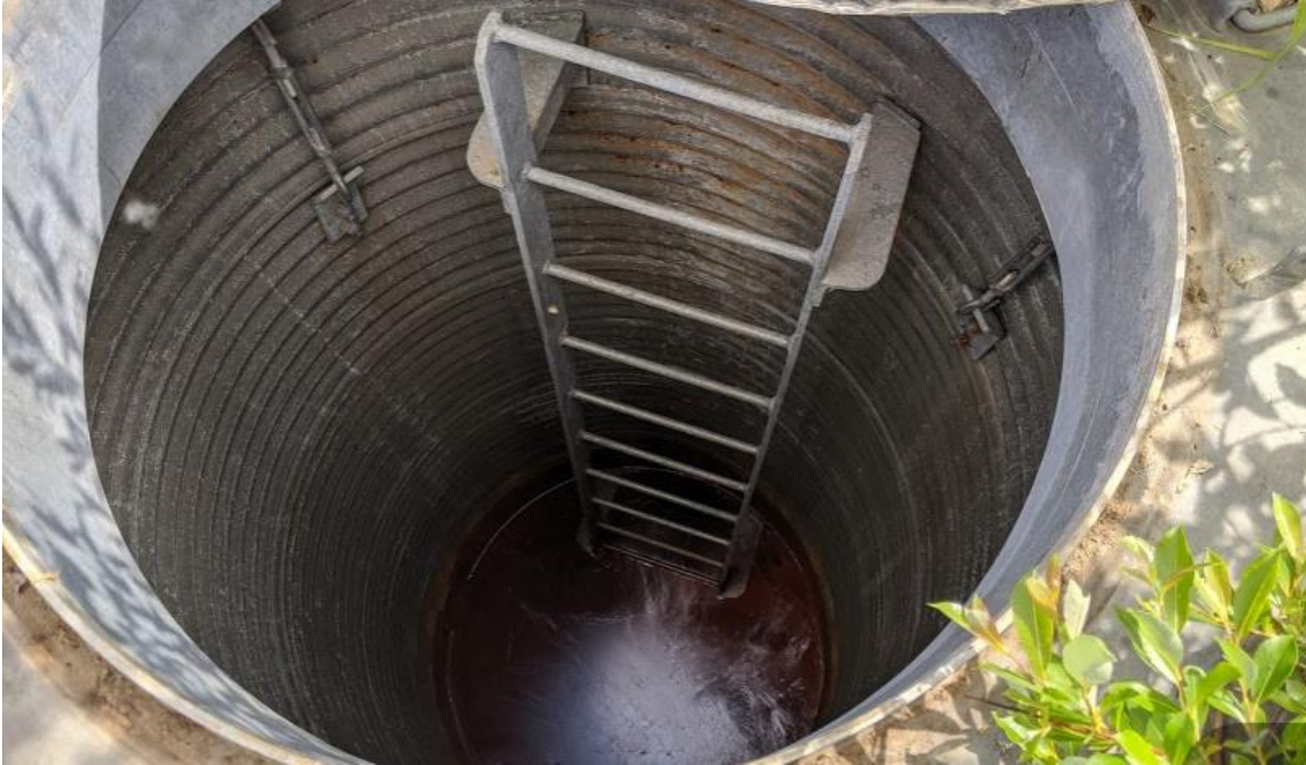
Photo No.3 – Manhole # 4; note that no flow was observed, and water was measured at 3 m from top of manhole
