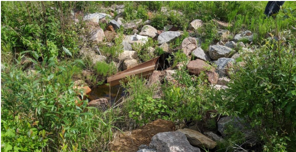
Photo No.10 – C3 culvert outlet; water is flowing out of the pipe but slightly ponding at outlet
