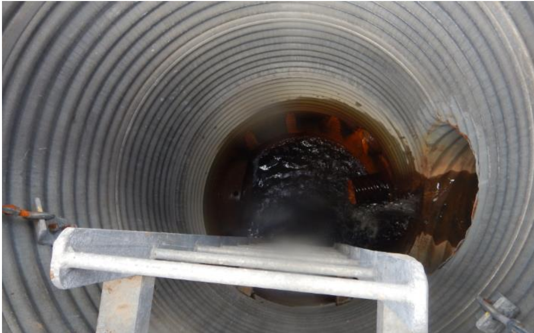
Photo No.5 – Manhole #3; note steady flow from the subdrain and culvert pipes
