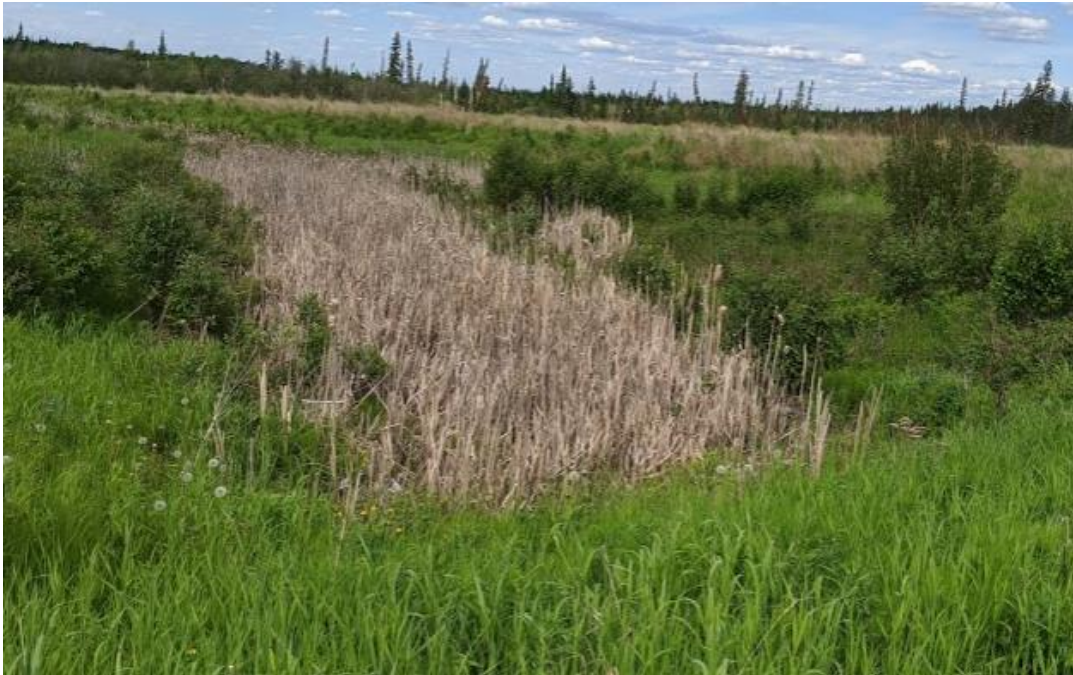
Photo No.7 – Water Ponding in the riprap channel located downslope of the 500 mm outflow pipe (Looking North)
