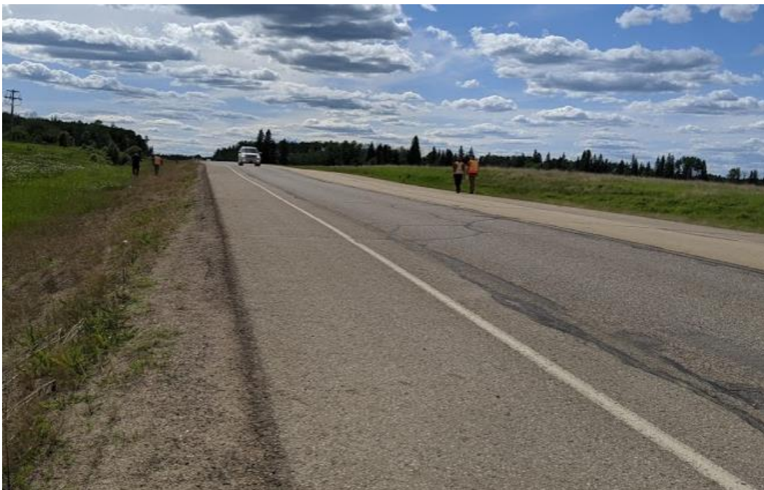
Photo No.6 – HWY 63 NBL; note presence of a hump and dip on highway lanes near the western flank of landslide (Looking West); highway cracks did not open since they were sealed in 2017
