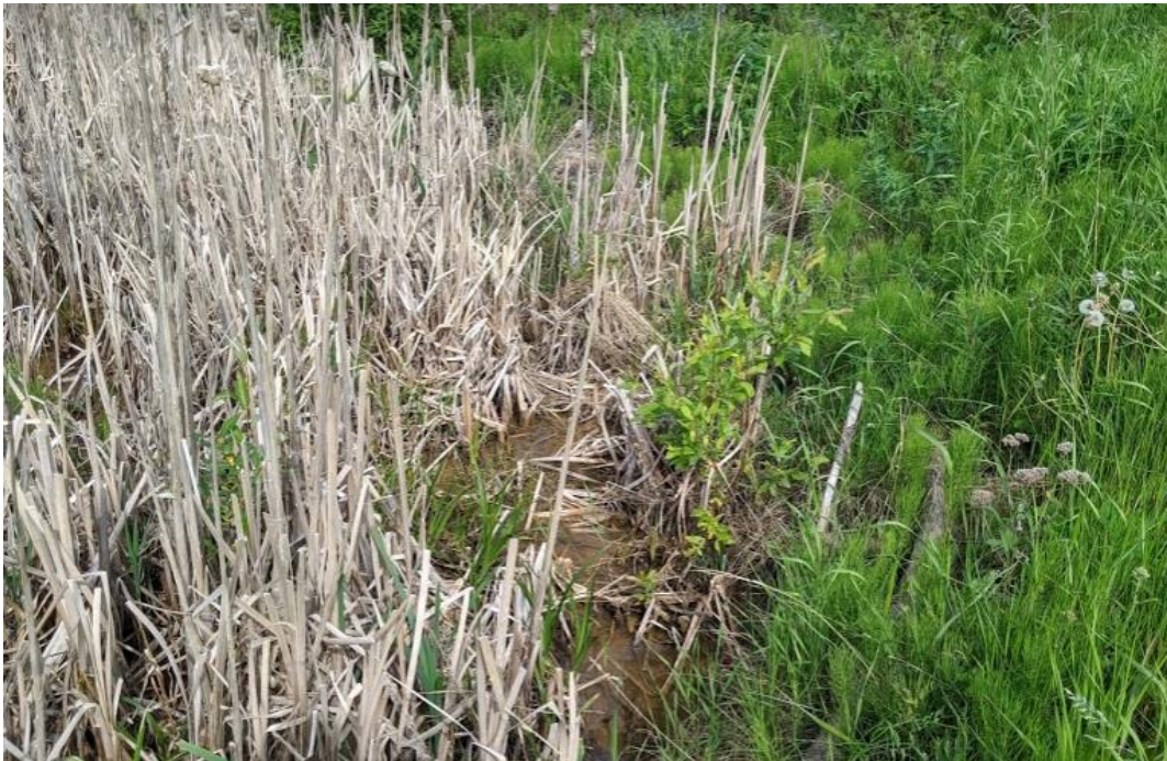
Photo No.8 – Ponding water, accumulated silt and debris at the outflow pipe outlet. Pipe is buried under sediment
