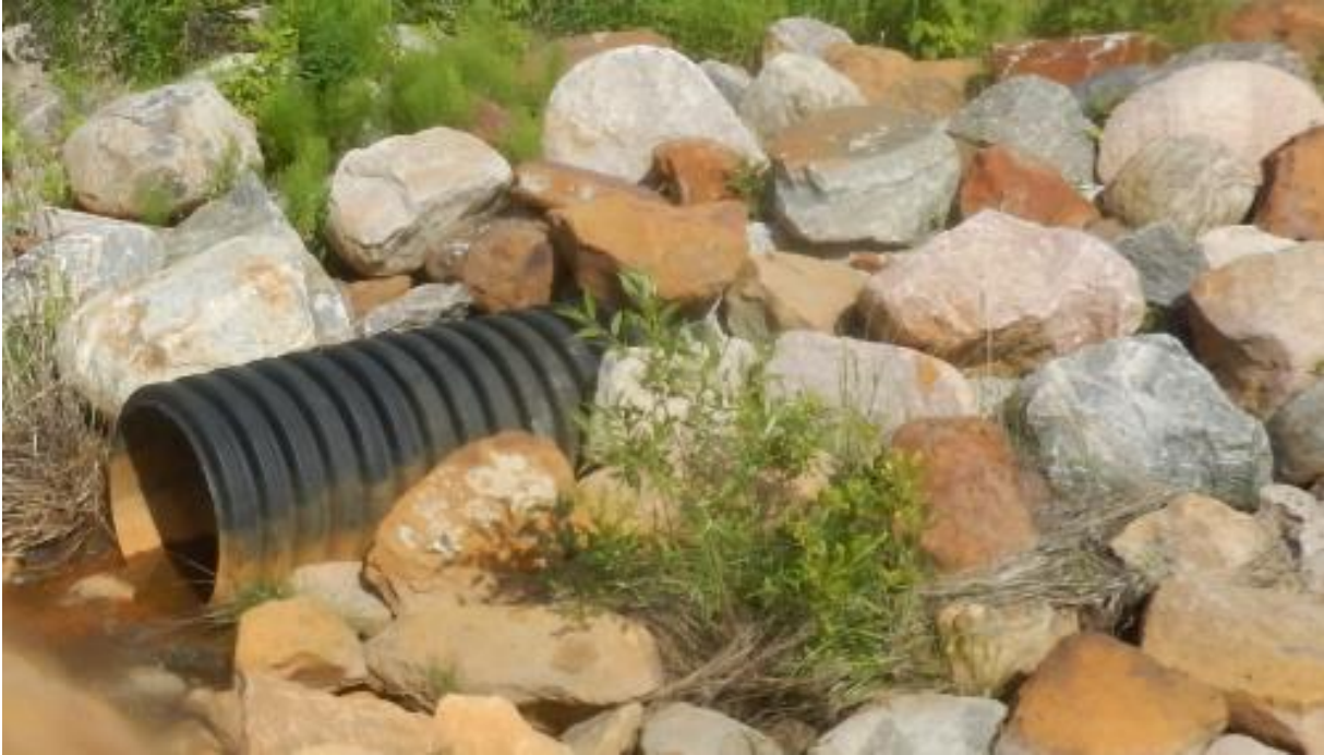
Photo No.9 – C2 extension (600 mm HDPE pipe outlet); water is flowing out of the pipe
