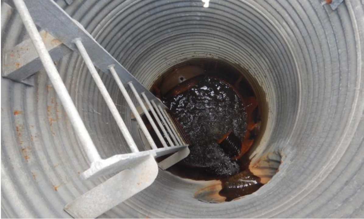
Photo No.5 – Manhole #3; note steady flow from the subdrain and culvert pipes
