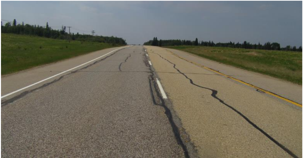
Photo No.8 – HWY 63 NBL; note presence of a hump and dip on highway lanes near the western flank of landslide (Looking West); highway cracks did not open since they were sealed in 2017
