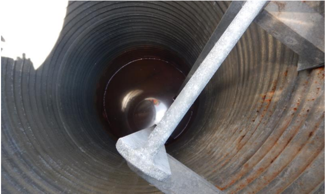
Photo No.3 – Manhole # 4; note that no flow was observed, and water was measured at 3 m from top of manhole
