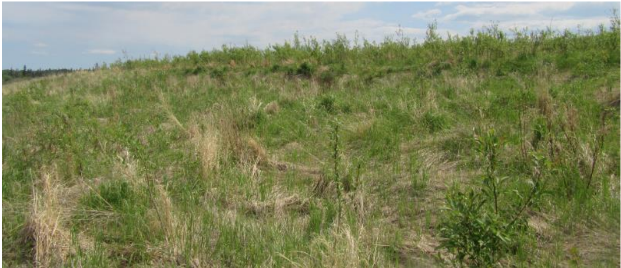
Photo No.14a – Vegetated head scarp crack of an old local slump on the north side of the western toe berm (Looking South)
