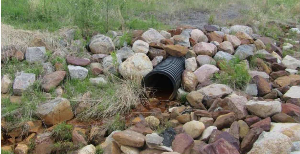
Photo No.14 – C2 extension (600 mm HDPE pipe outlet); water is flowing out of the pipe
