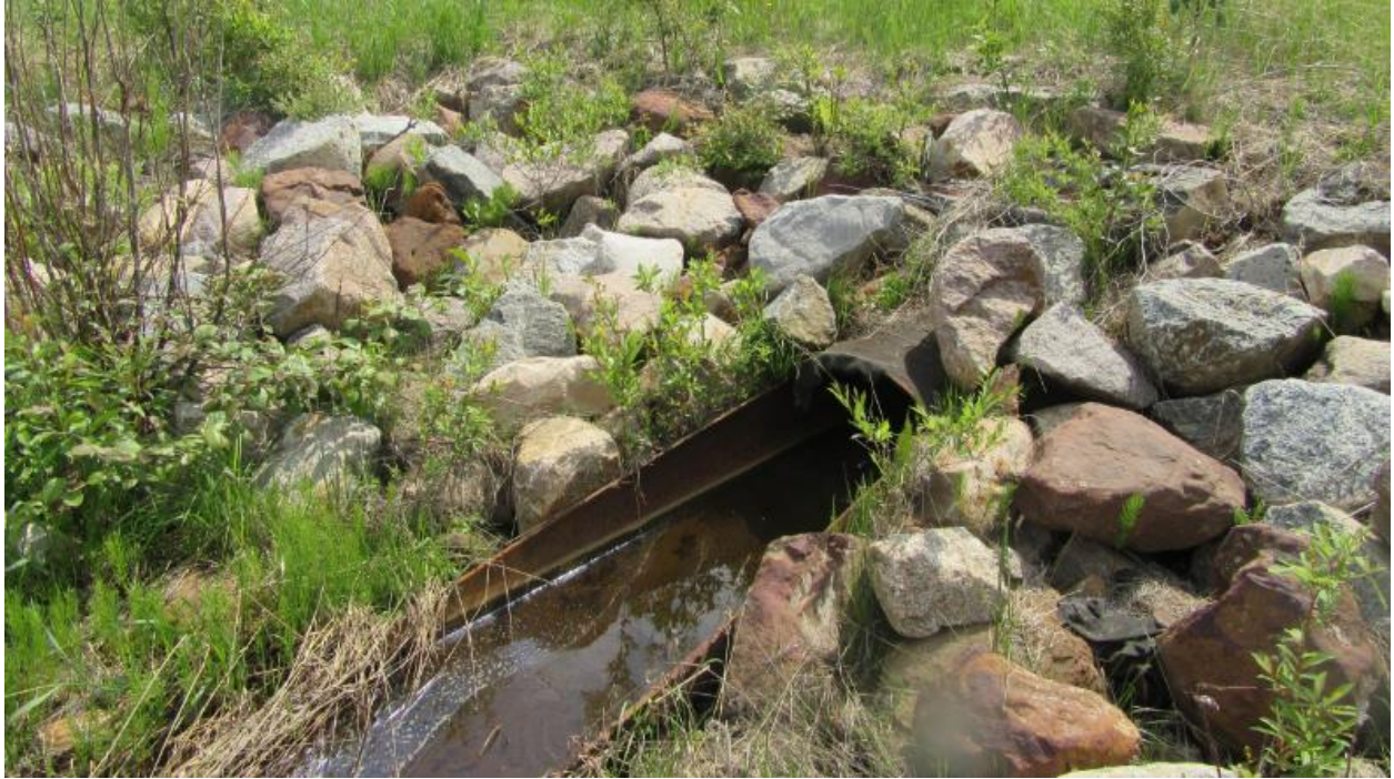
Photo No.15 – C3 culvert outlet; water is flowing out of the pipe
