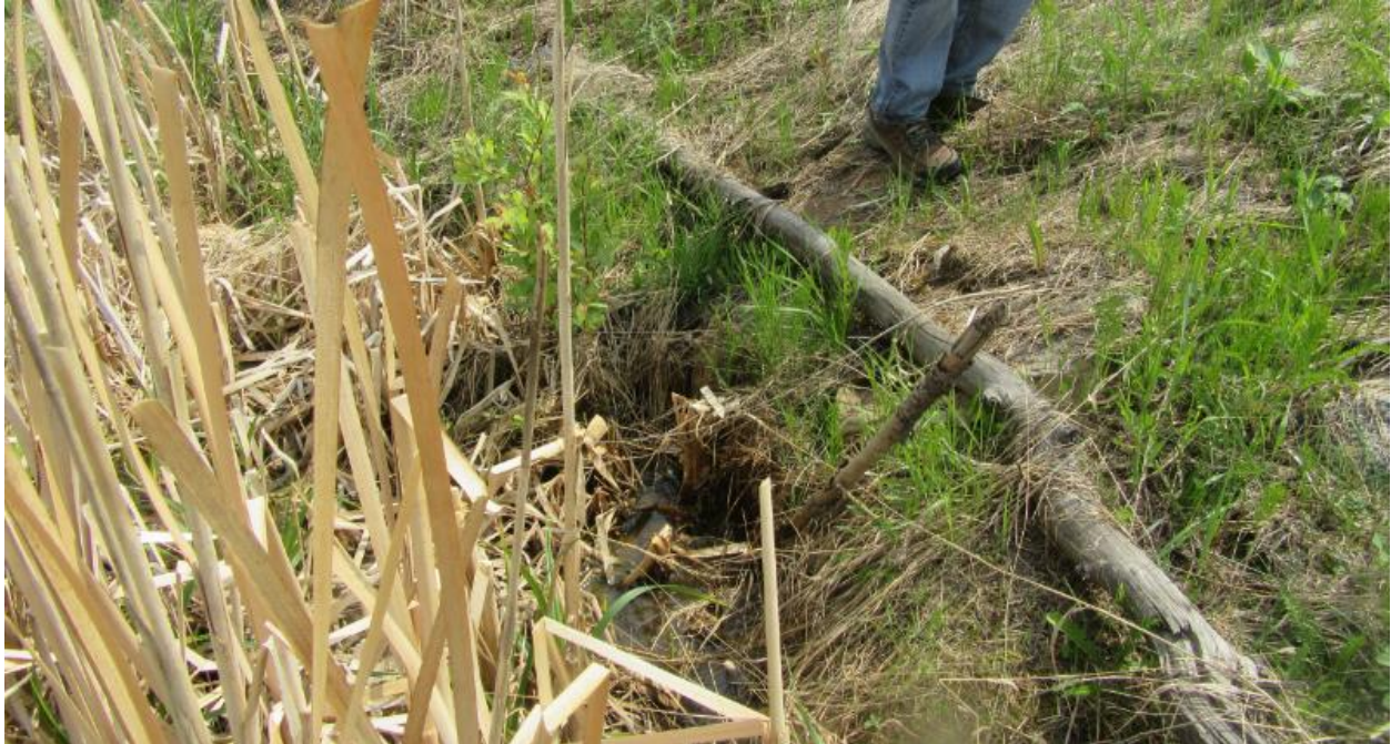
Photo No.10 – Ponding water, accumulated silt and debris at the outflow pipe outlet. Pipe is buried under sediment
