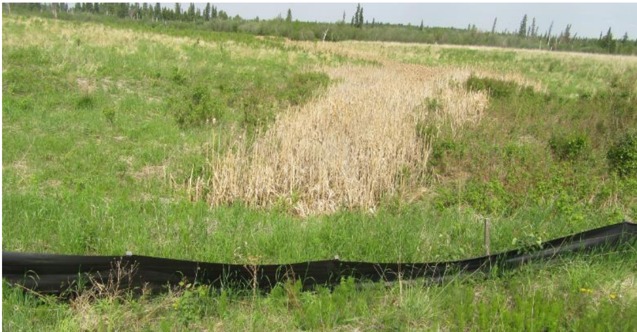
Photo No.9 – Water Ponding in the riprap channel located downslope of the 500 mm outflow pipe (Looking North)
