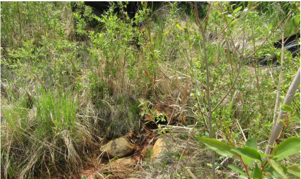
Photo No.13a – Subdrain pipe outlet S1; pipe was partially buried under silt; water was ponding at the outlet of the pipe
