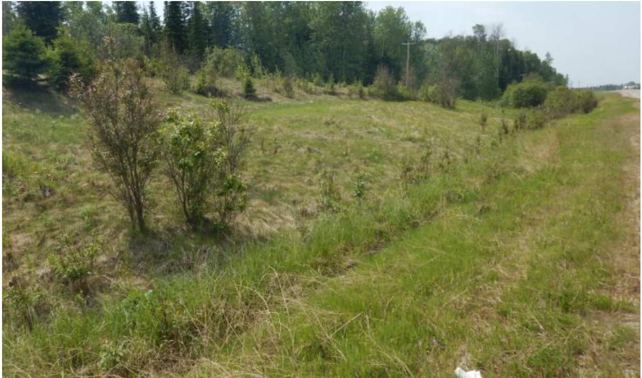
Photo No.16 – Looking south at the highway back slope slump; note that the toe is blocking the ditch flow
