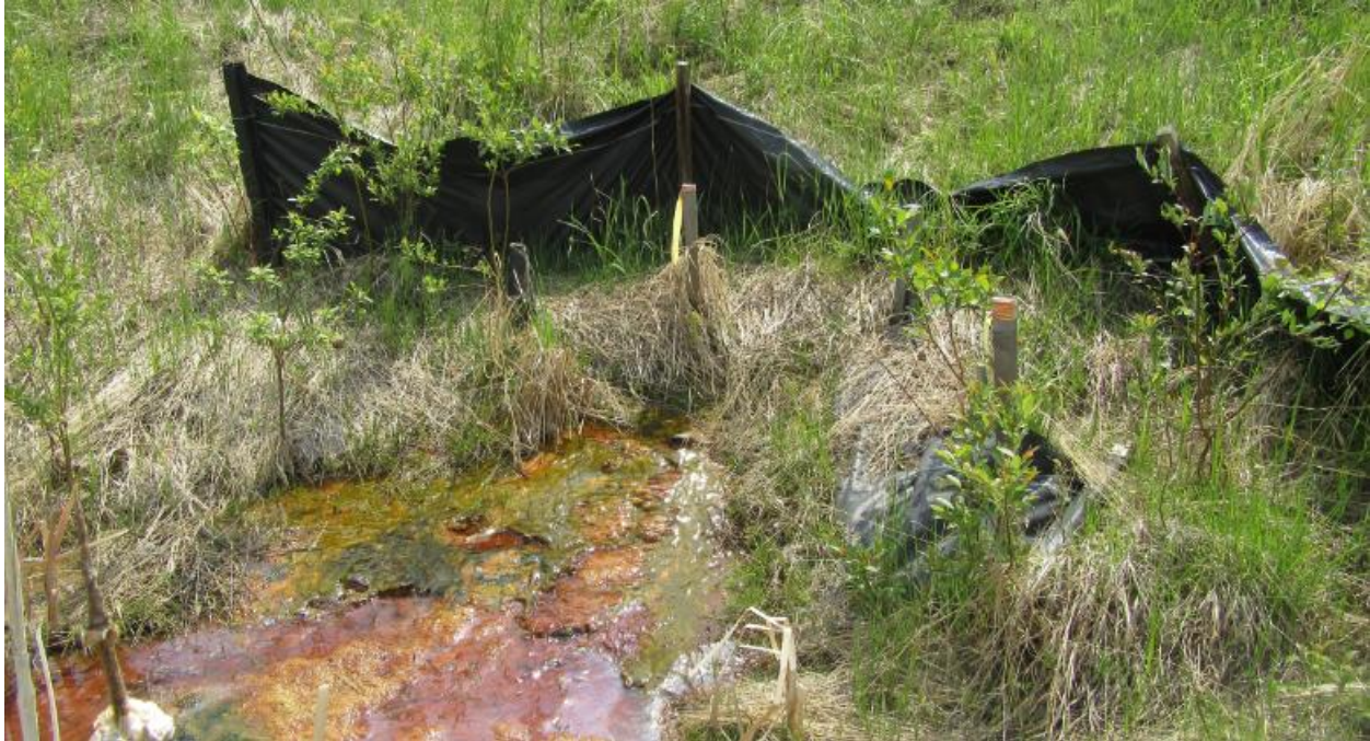
Photo No.13 – Subdrain pipe outlet S2; pipe was completely buried under silt; water was ponding at the outlet of the pipe
