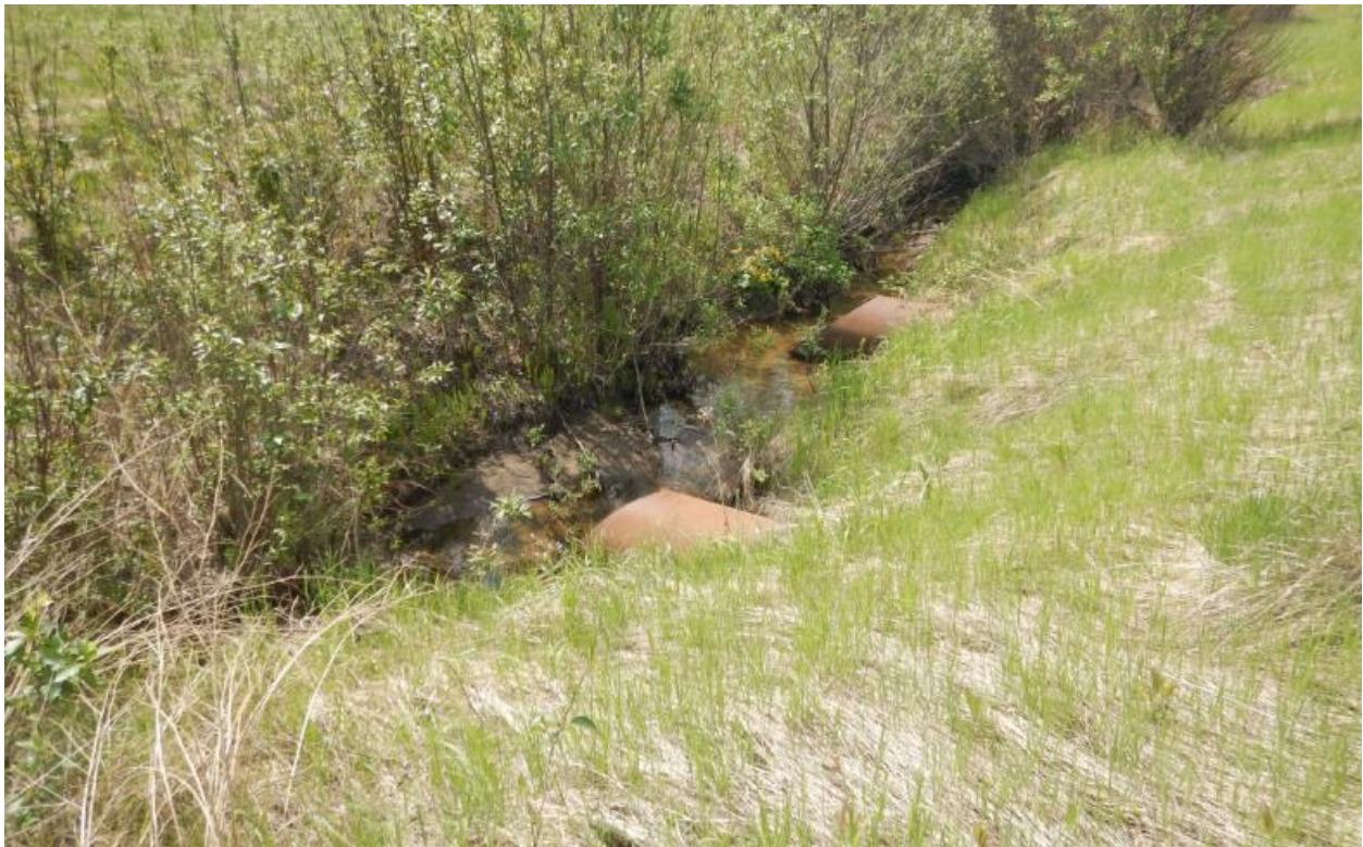
Photo No.17 – Two 800 mm SWSP culvert inlets; note existing erosion around the SWSP inlets (looking south)
