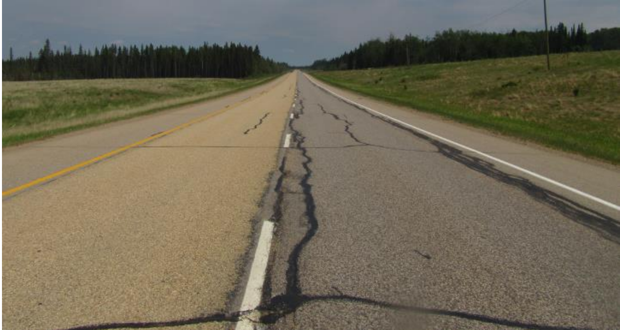
Photo No.8a – HWY 63 NBLs; not presence of a hump and dip on highway lands near the eastern flank of landslide (Looking East); highway cracks did not open since they were sealed in 2017
