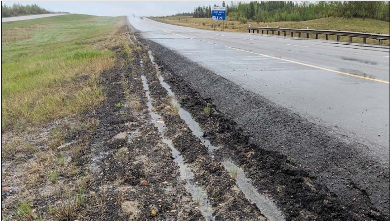
Photo No. 11 – Sharp Drop off 500 mm high on the NBL; significant thickness of ACP has been placed on the highway NBLs to remove the dip developed in response to slope movement
