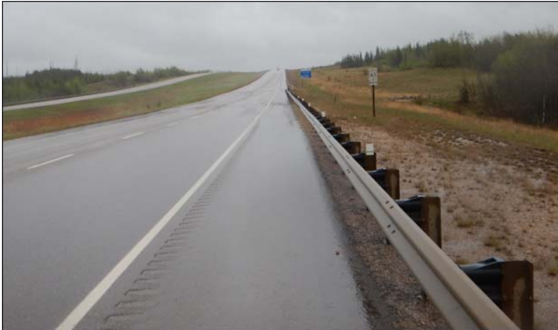
Photo No. 1 – Looking north at ACP patch recently placed along the north bound lanes (NBLs)
