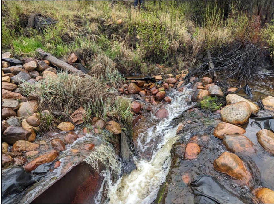
Photo No. 5a – Riprap channel erosion and debris accumulation near the 1.2 m SWSP culvert inlet
