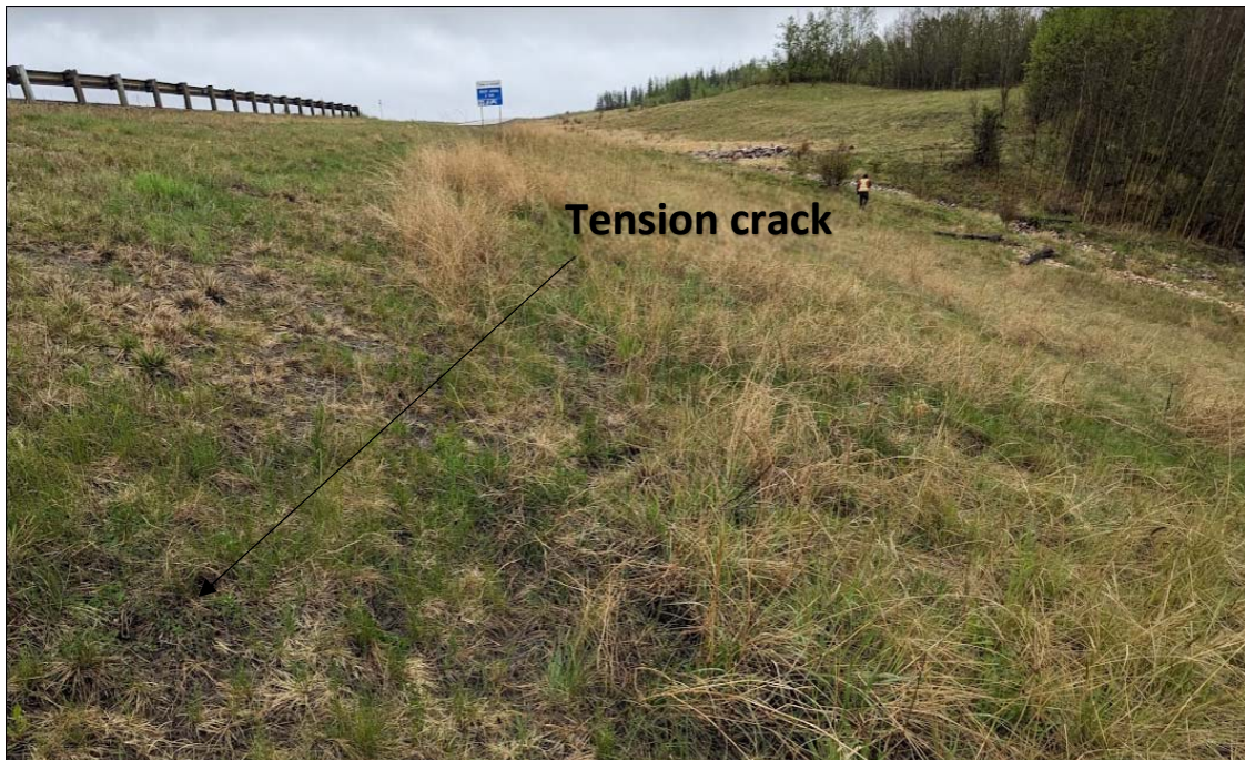
Photo No. 2 – Looking north at NBL embankment side slope. Note minor tension crack 50 mm wide and 50 mm deep
