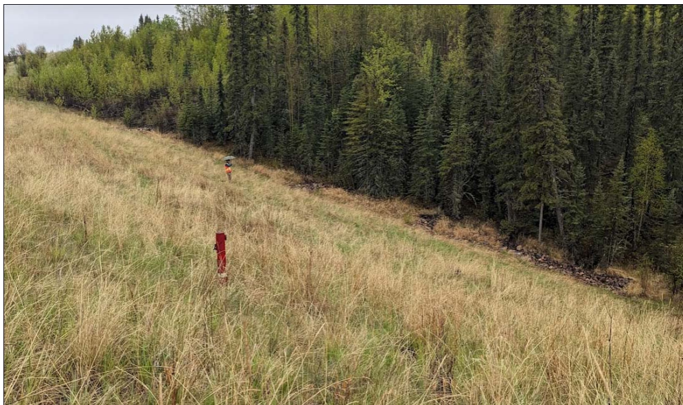
Photo No. 8 – Looking south at SBL west side slope; note good vegetation growth within repaired area
