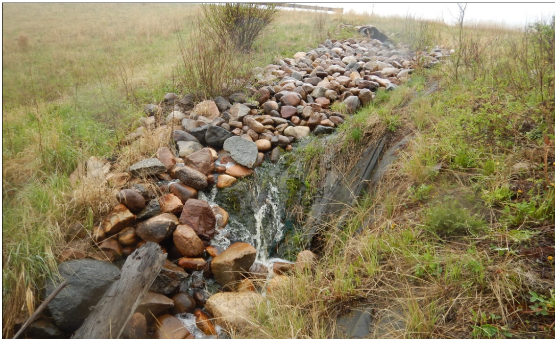
Photo No. 5 – Severe erosion within the riprap channel located downslope of the C3 culvert outlet
