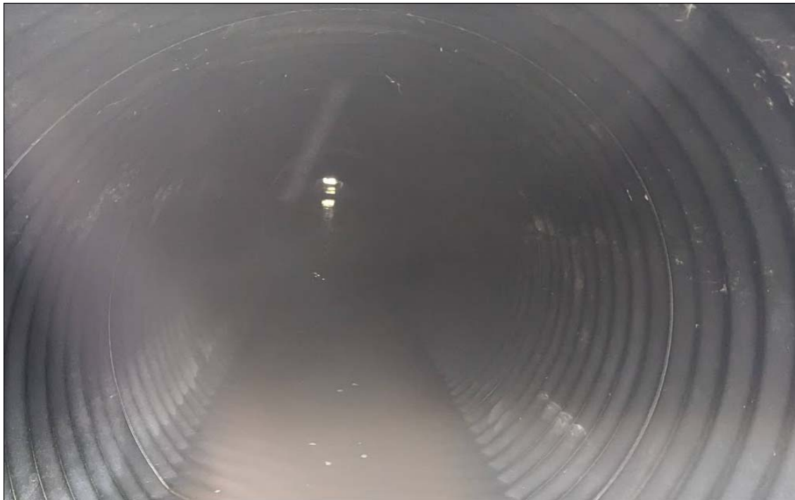
Photo No. 3 – CSP culvert C3 outlet showing heavy flow. Lower photo showing the condition inside the CSP culvert
