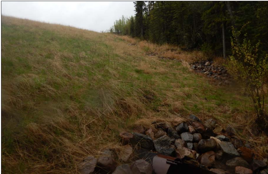
Photo No. 10 – North facing riprap channel along the SBL west side slope
