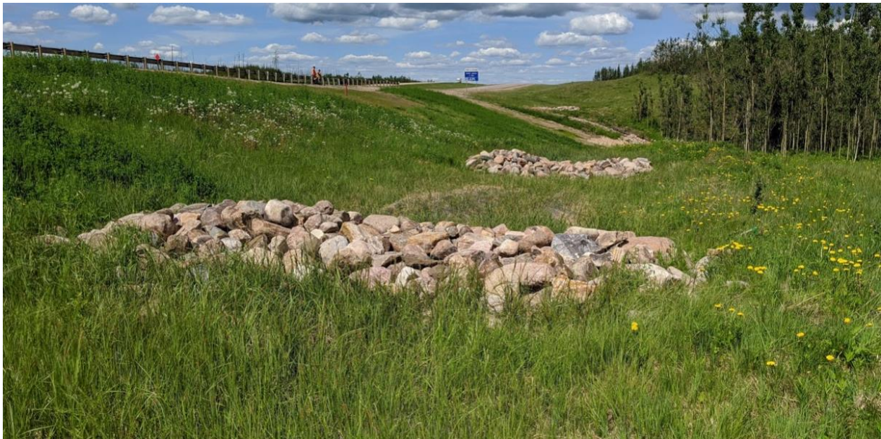
Photo No. 10 – Rock check dams located along NBL southeast ditch
