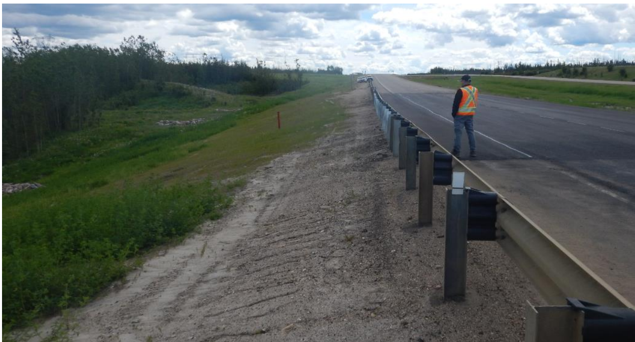
Photo No. 2 – Looking south at NBL embankment side slope; note minor rills near the guardrail
