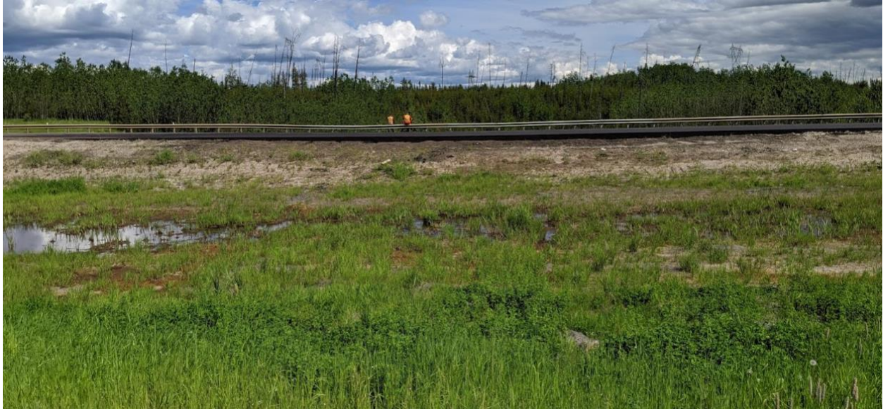
Photo No. 11 – Median ponding water; note recently placed ACP patch on the NBL
