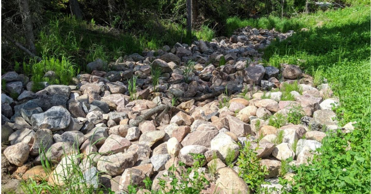
Photo No. 13 – New north facing riprap channel along the SBL west side slope
