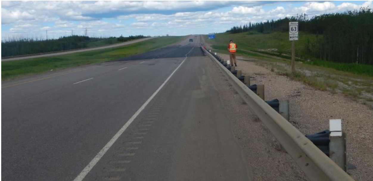
Photo No. 1 – Looking north at ACP patch recently placed along the north bound lanes (NBLs)
