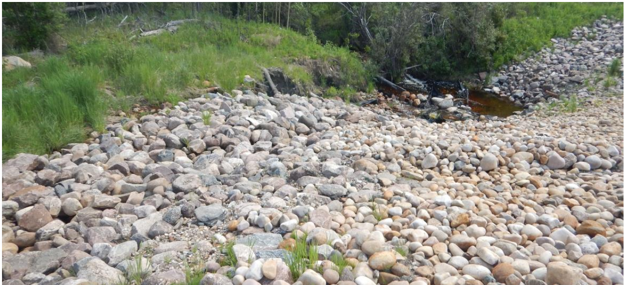
Photo No. 6 – Looking southeast toward the 1.2 m SWSP inlet; note erosion along the south facing riprap channel and deadfall accumulation near the inlet
