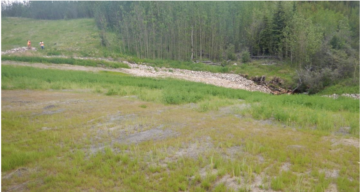
Photo No. 3 – NBL Embankment side slope; note vegetation growth and erosion of the creek bank at the toe of the slope
