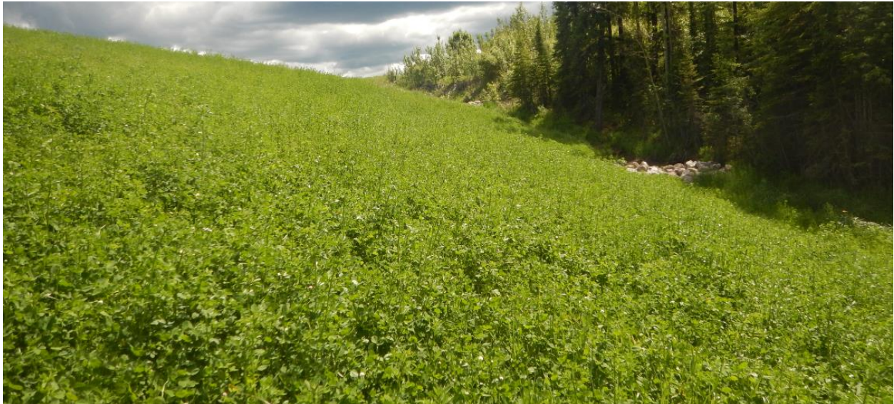
Photo No. 12 – Looking south at SBL west side slope; note good vegetation growth within recently repaired area
