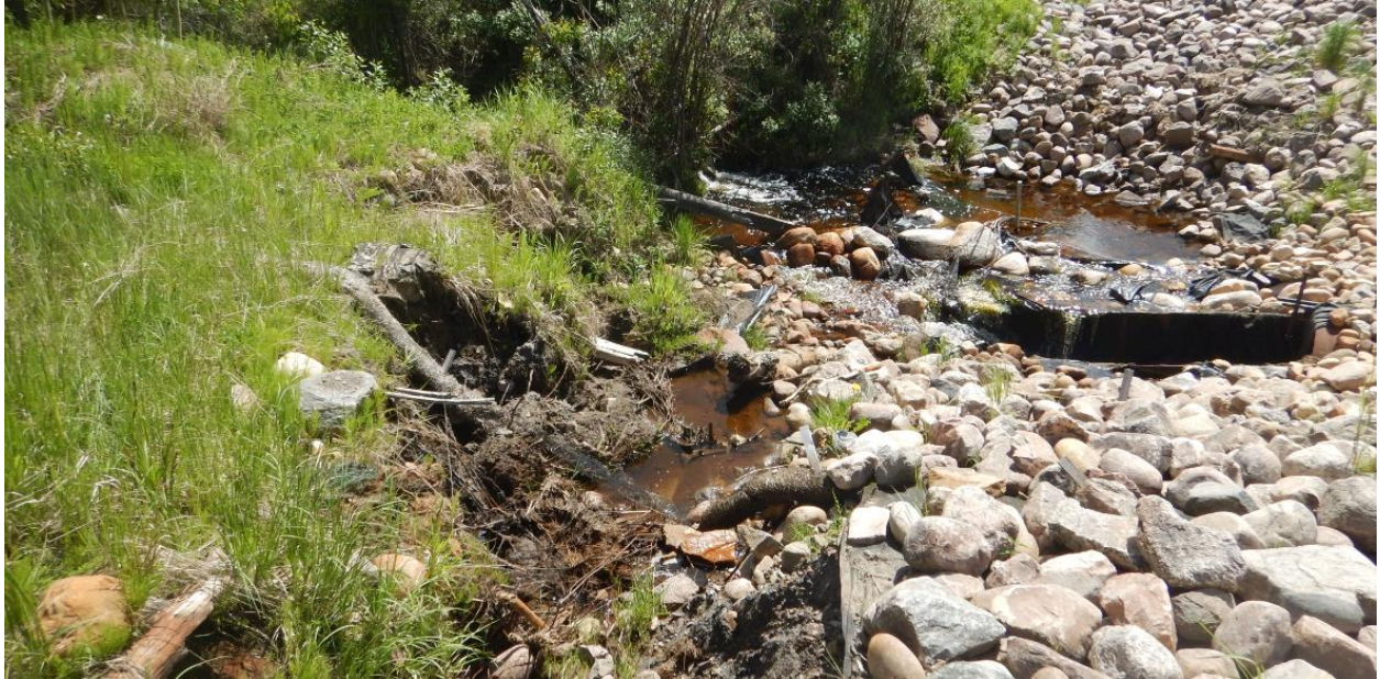
Photo No. 7 – Riprap channel erosion and debris accumulation near the 1.2 m SWSP culvert inlet
