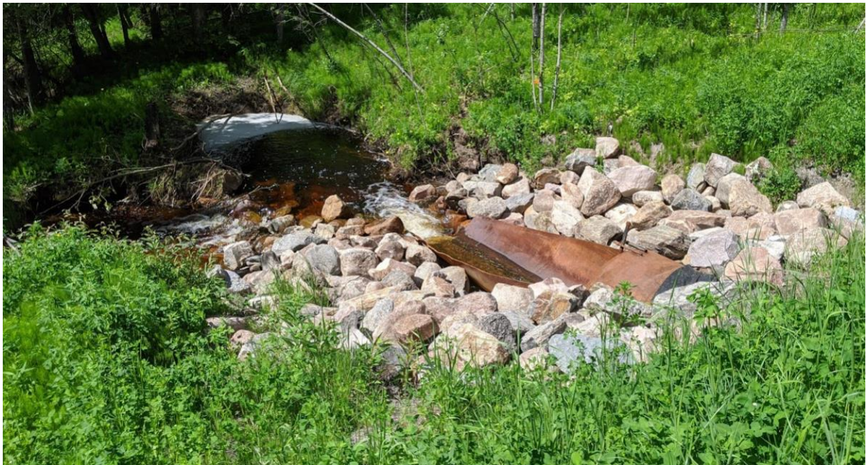
Photo No. 14 – New SWSP outlet; note water flow and minor erosion downstream of the outlet
