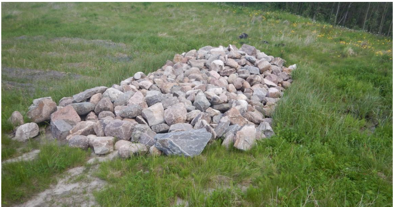
Photo No. 4 - New rock check dam located in the northeast ditch of the highway
