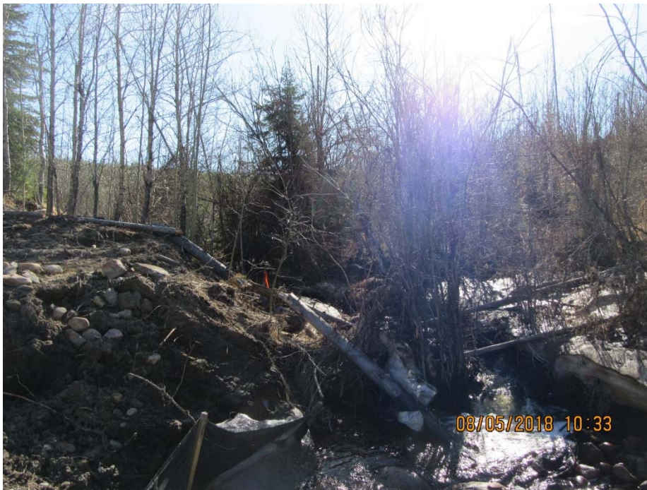
Photo No. 6 - Caved in Bank with trees partially blocking the new pipe
