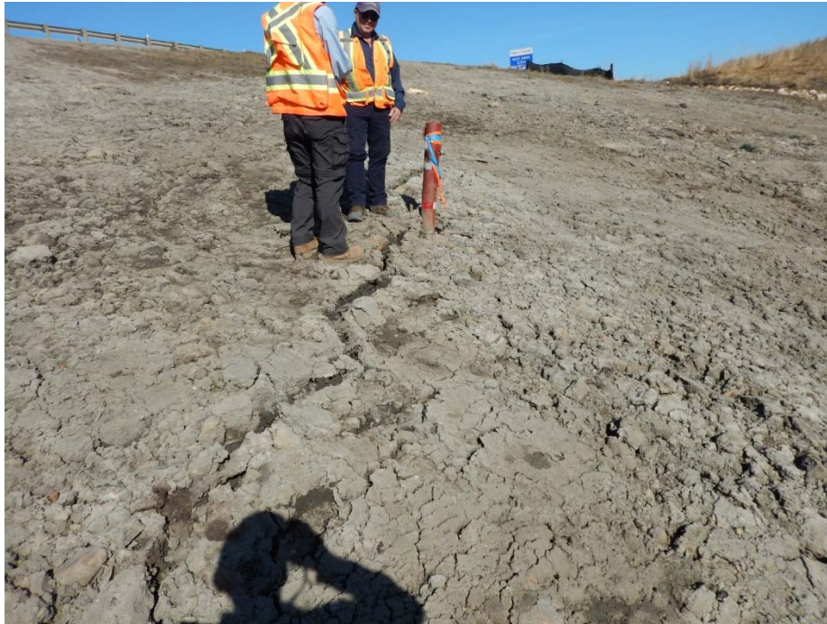
Photo No. 11 – Looking north at new cracks developed on the east embankment side slope (about 25 m above the culvert location)– Signs of localized slump above the culvert location
