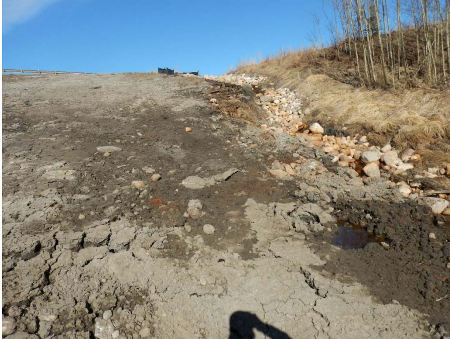
Photo No. 1 - North riprap lined channel leading to the inlet of the new pipe (looking north). Note the presence of disturbed riprap, seeping/ponding water into the slope beside and above the culvert inlet location, and existing cracks.
