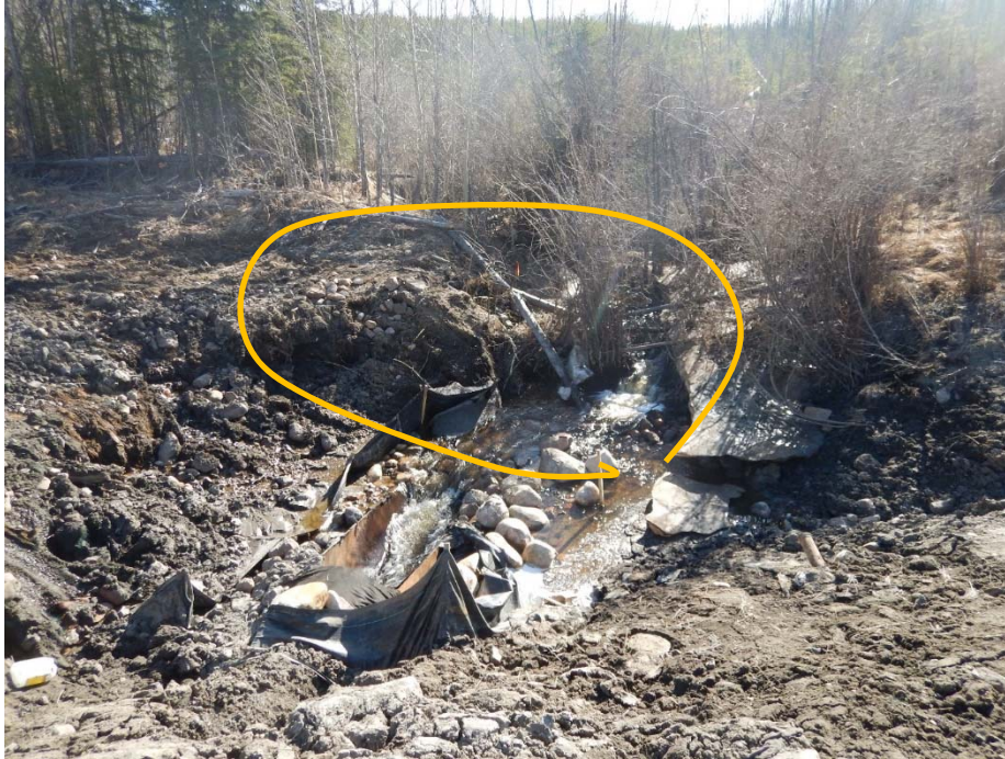
Photo No. 5 - New pipe Inlet Area (looking east) – Restricted flow to the culvert inlet, partially due to caved in bank slope (note the presence of deadfall). Creek flow is partially ponding to the south of the culvert inlet
