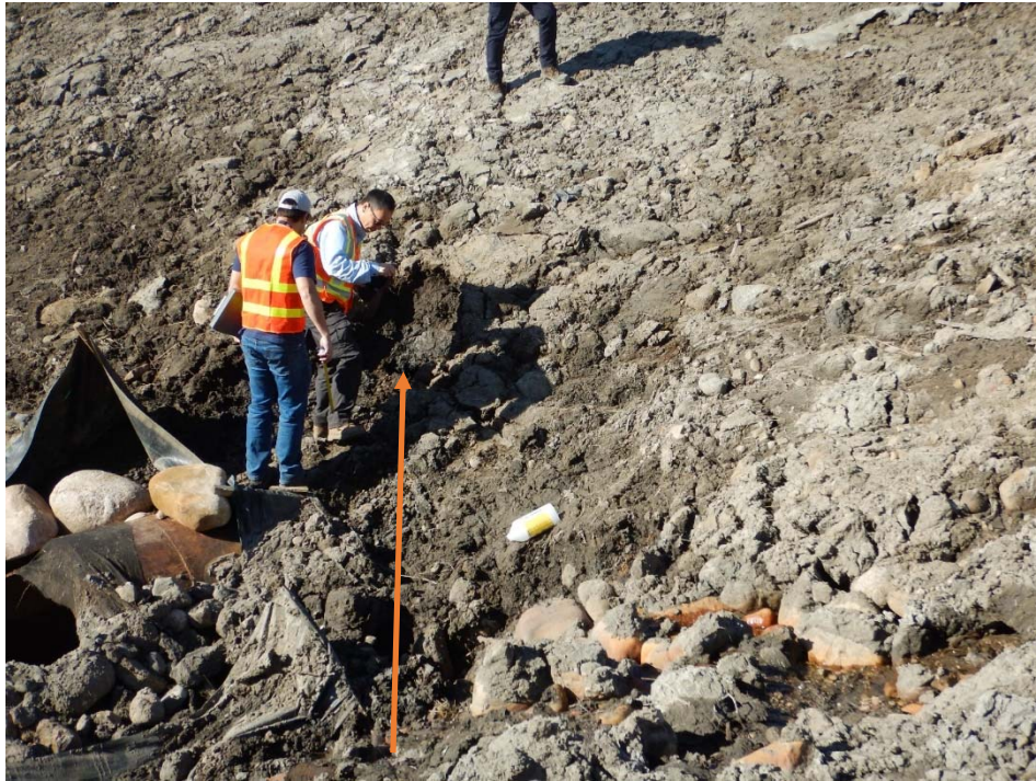
Photo No. 7 - Cavity noted above the crown of the new pipe.
