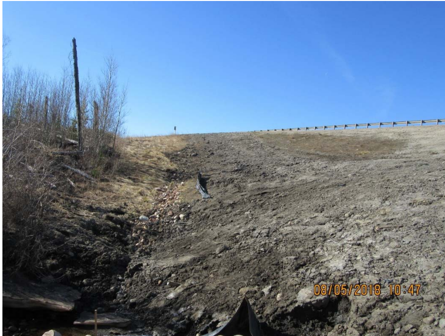
Photo No. 9 – Disturbed riprap in the south riprap lined channel leading to the new pipe inlet (looking south)
