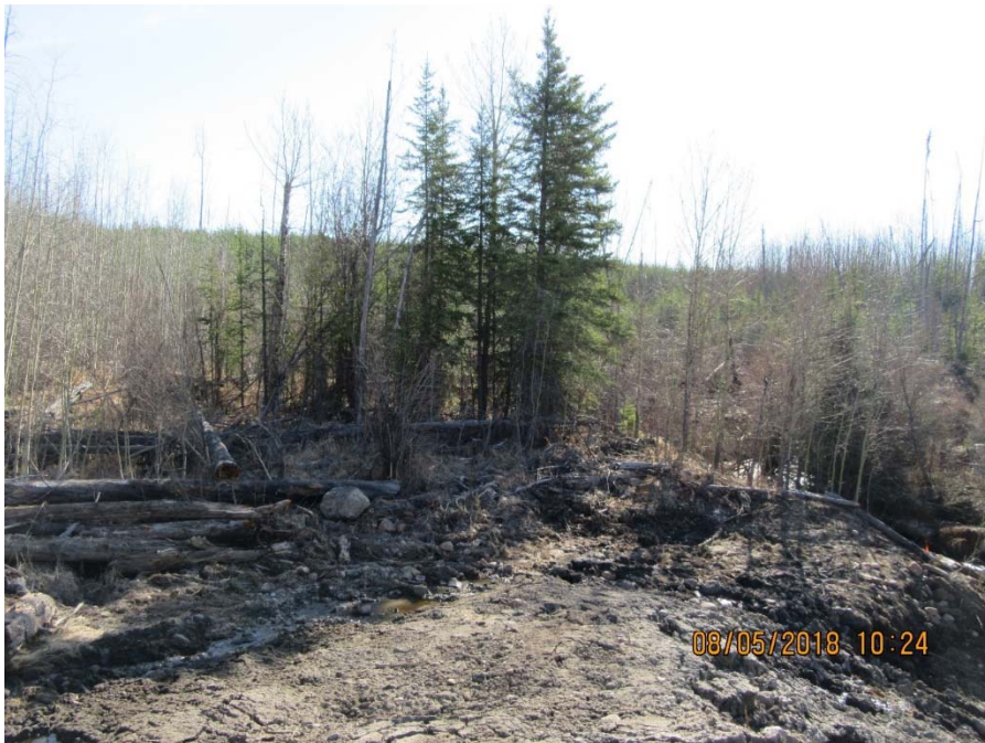
Photo No. 2 - Water Flowing in an uncontrolled manner from the mouth of the north riprap lined channel to the creek bank
