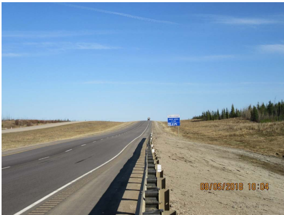
Photo No. 12 – Looking north at the highway surface. Note the pavement distress and the distortion of the guardrail within the dip area
