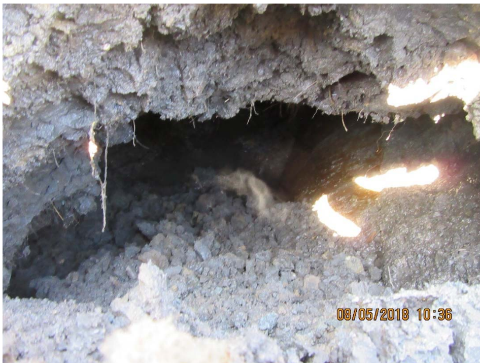
Photo No. 8 - Water seeping into the cavity
