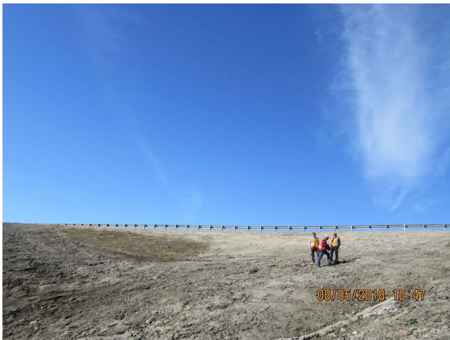
Photo No. 10 - Looking West at the highway embankment side slope. Note that the slope is bare of vegetation
