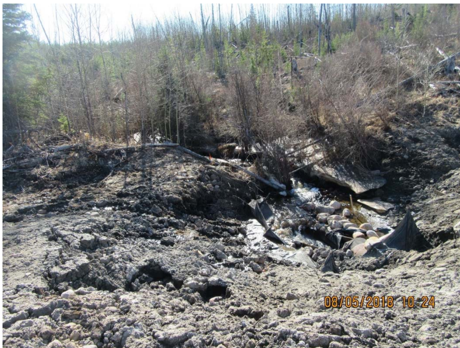
Photo No. 4 - New pipe Inlet Area (looking east) – Disturbed bank slopes, riprap, and silt fences. The banks are not armored and there is not enough riprap at the inlet location
