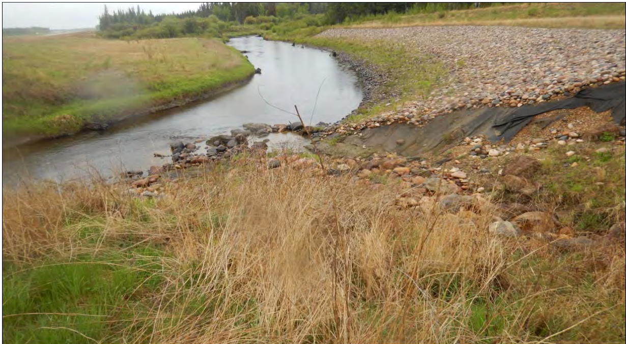
Photo No. 2 – Looking north at north facing riprap channel to the east of the bridge location. Note the deep erosion along the channel.
