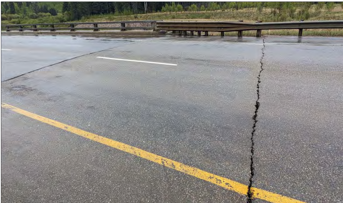
Photo No. 8 – Dip at the bridge south approach slab appears to have dropped more; and it is more noticeable within the western half between the yellow line and the edge of pavement above Slump 2
