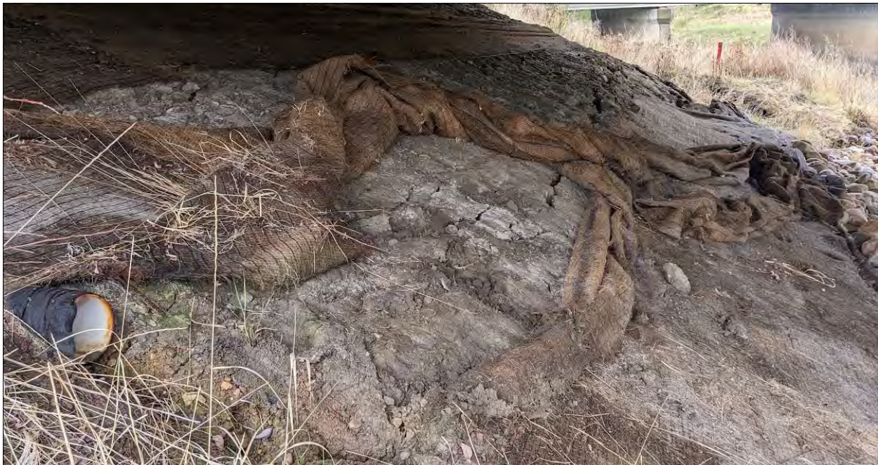
Photo No. 6 – Looking at Crack on head slope extending to the subdrain on the east side of the bridge. Crack is 5 mm wide at the subdrain and 700 mm wide at 10 m west of the subdrain.
