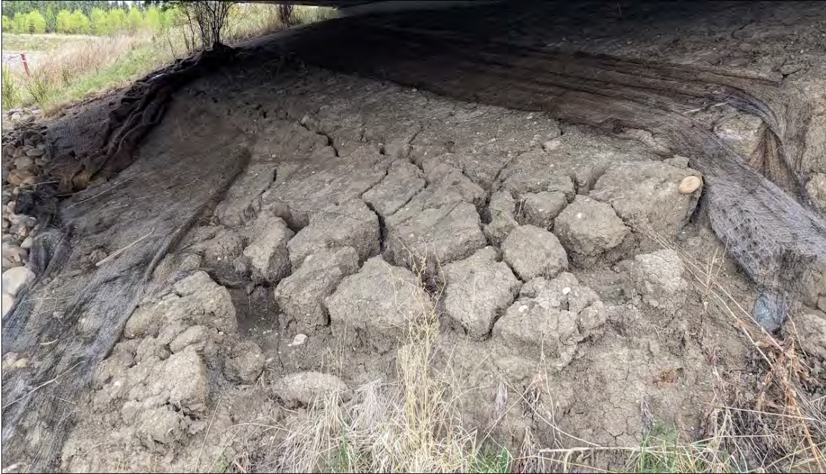
Photo No. 7 – Looking southeast at Slump No. 2 flank. Note: (a) eastern flank of slump extending below the bridge headslope and (b) extensive cracking and presence of a distinct longitudinal crack below bridge headslope
