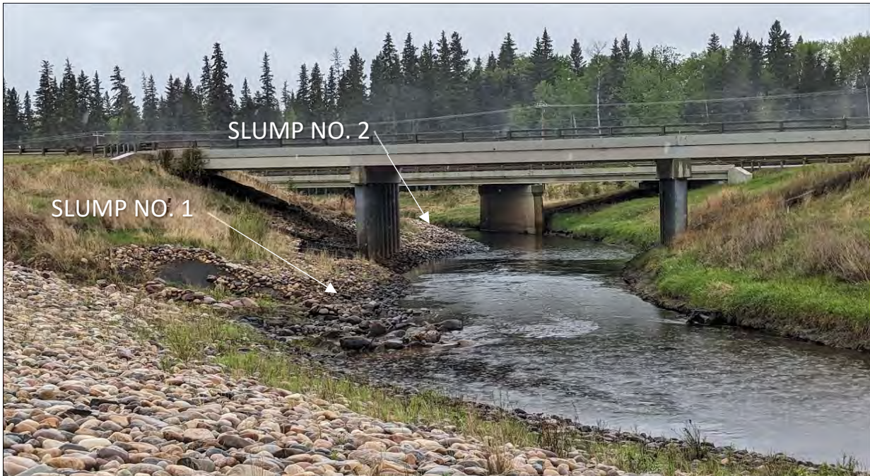
Photo No. 4 – Slumping within the riverbanks to the east of the Hwy (slump 1) and to the west of the Hwy (slump 2). Note distinct toe rolls in the river channel.
