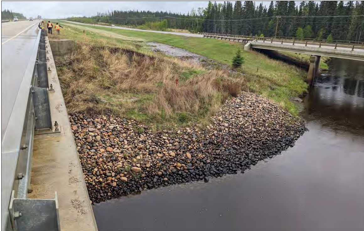
Photo No. 5 – Looking southwest at Slump No. 2. Vegetation has grown within the slump since the 2023 inspection.
