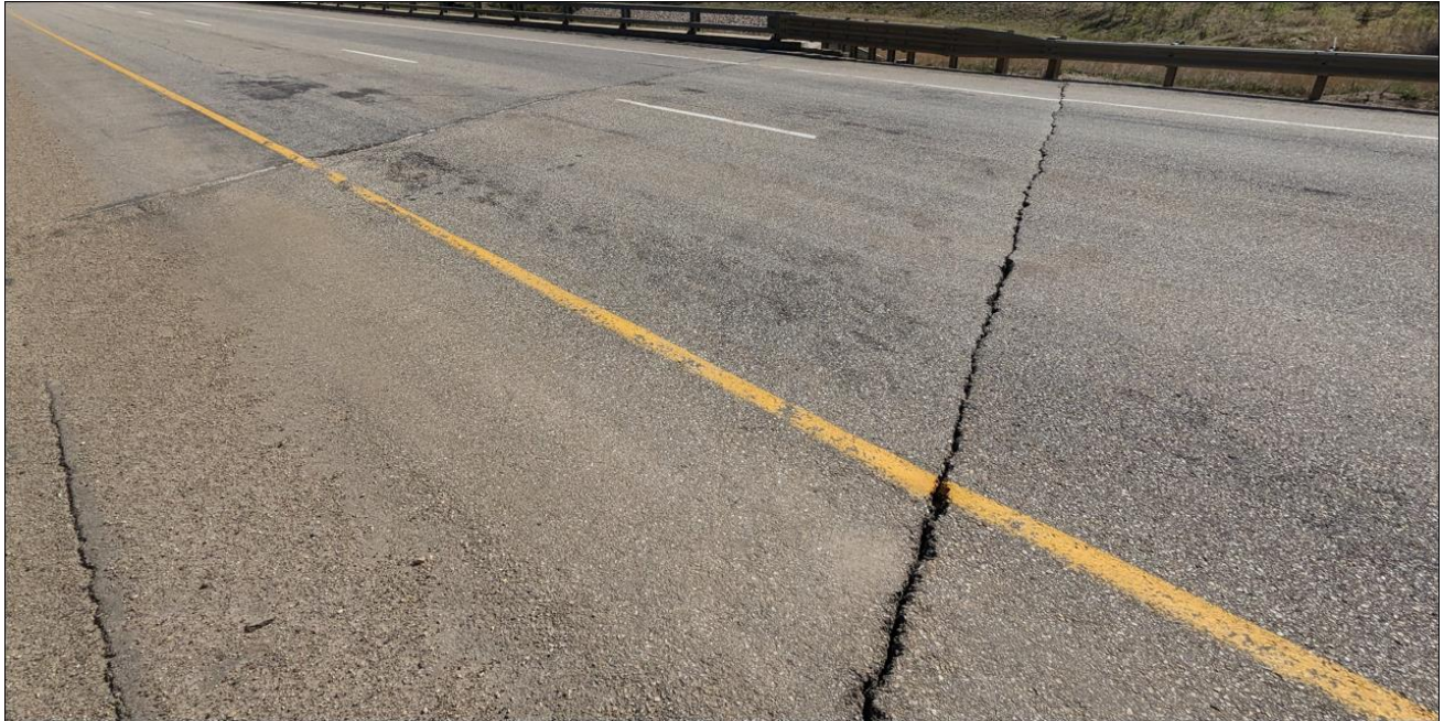
Photo No. 9 – Looking northeast at the bridge south approach slab; there is a slight dip in the highway surface, and it is more noticeable within the western half between the yellow line and the edge of pavement above Slump 2
