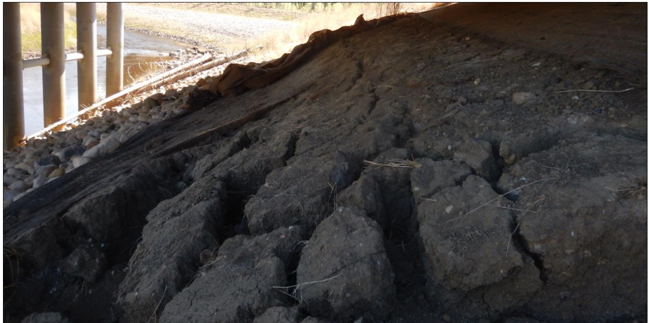
Photo No. 8 – Looking southeast at Slump No. 2 flank. Note: (a) void developed under wingwall, (b) change in soil type between the area under the bridge and the area beyond (west of) the wing wall, and (c) eastern flank of slump extending below the bridge headslope
