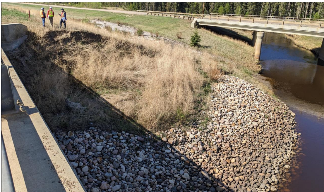
Photo No. 6 – Looking southwest at Slump No. 2
