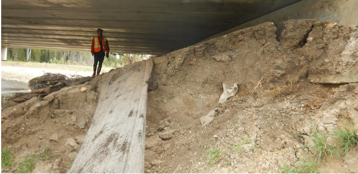
Photo No. 9 – Looking east at the portion of the head slope impacted by Slump No. 2
