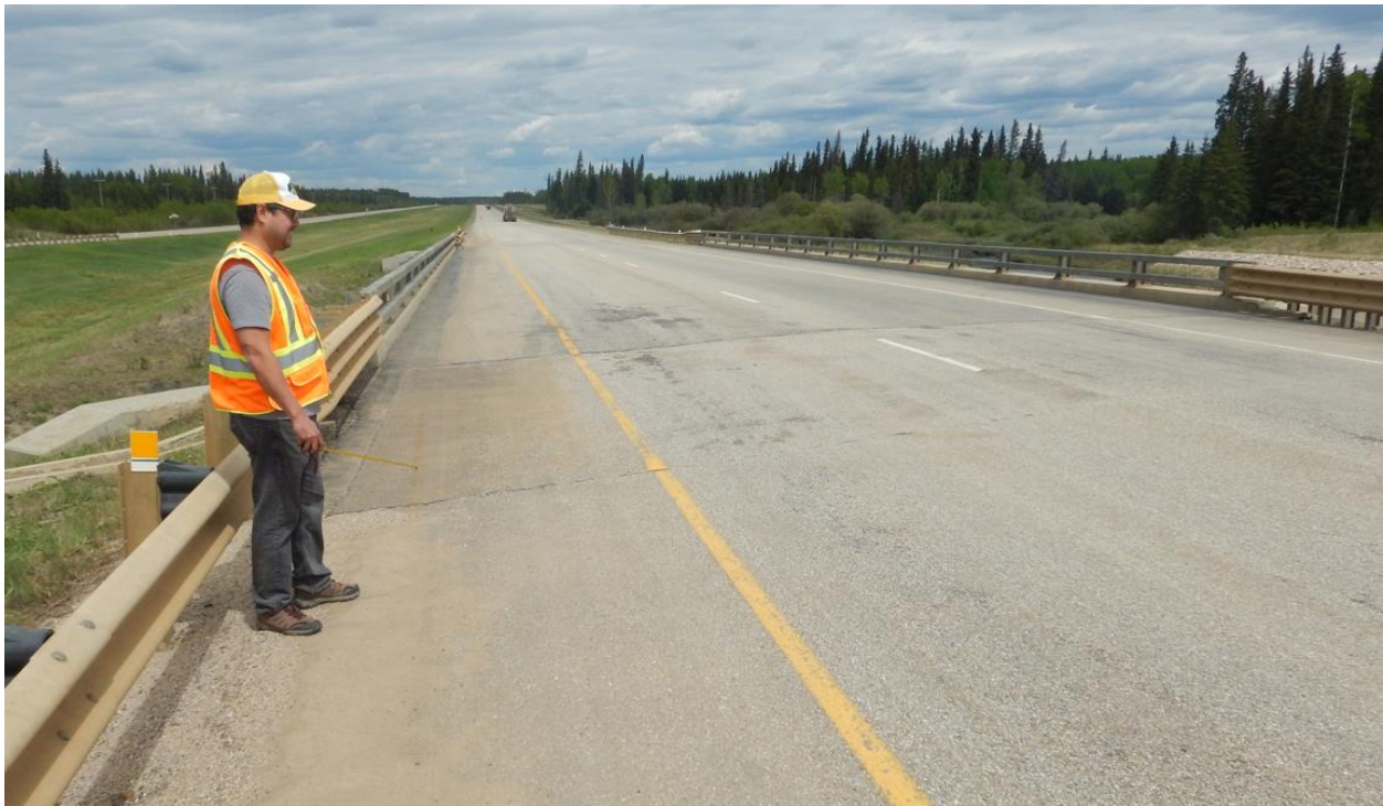
Photo No. 10 – Looking north at the bridge south approach slab; there is a slight dip in the highway surface, and it is more noticeable within the western half between the yellow line and the edge of pavement above Slump 2
