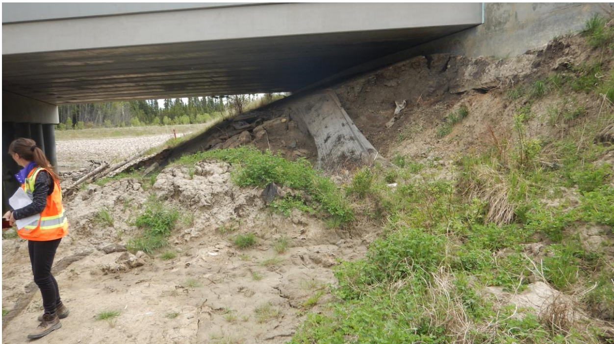
Photo No. 8 – Looking southeast at Slump No. 2 flank. Note: (a) void developed under wingwall, (b) change in soil type between the area under the bridge and the area beyond (west of) the wing wall, and (c) eastern flank of slump extending below the bridge headslope
