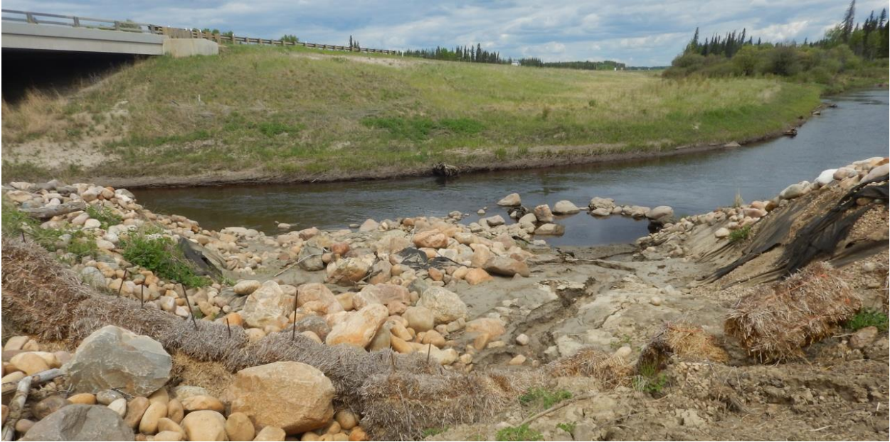
Photo No. 3 – Looking north at north facing riprap channel to the east of the bridge location. Note erosion along the channel.
