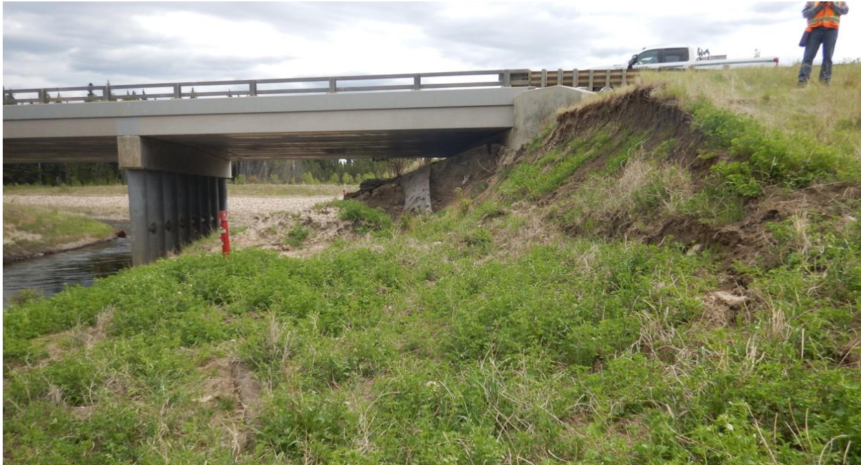
Photo No. 7 – Looking east at the head scarp crack of Slump No. 2
