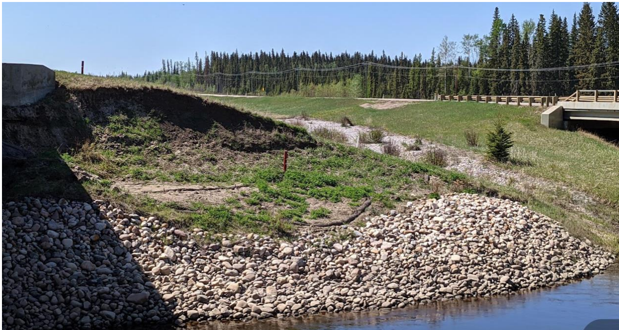
Photo No. 6 – Looking southwest at Slump No. 2
