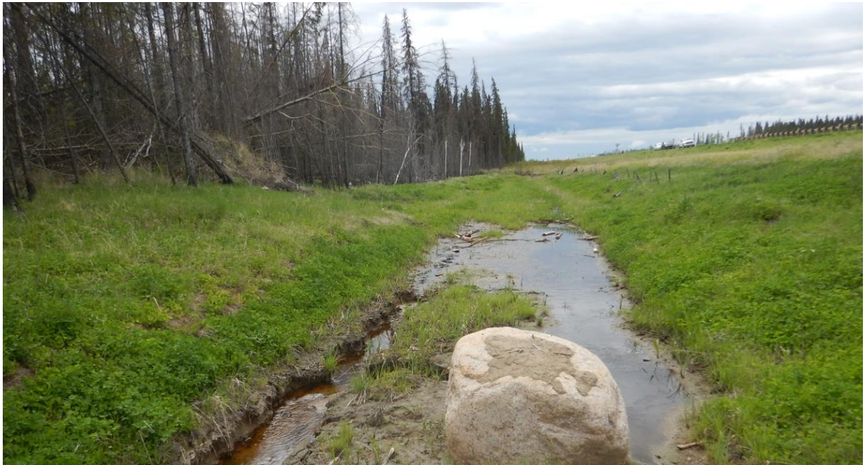
Photo No. 2 – Looking south at the highway west ditch; water is draining towards the eroded ditch to the east of the bridge location
