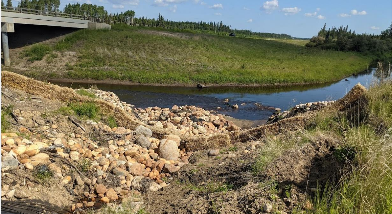
Photo No. 3 – Looking north at north facing riprap channel to the east of the bridge location. Note erosion along the channel. Beaver dam noted in this area in 2020 was removed.
