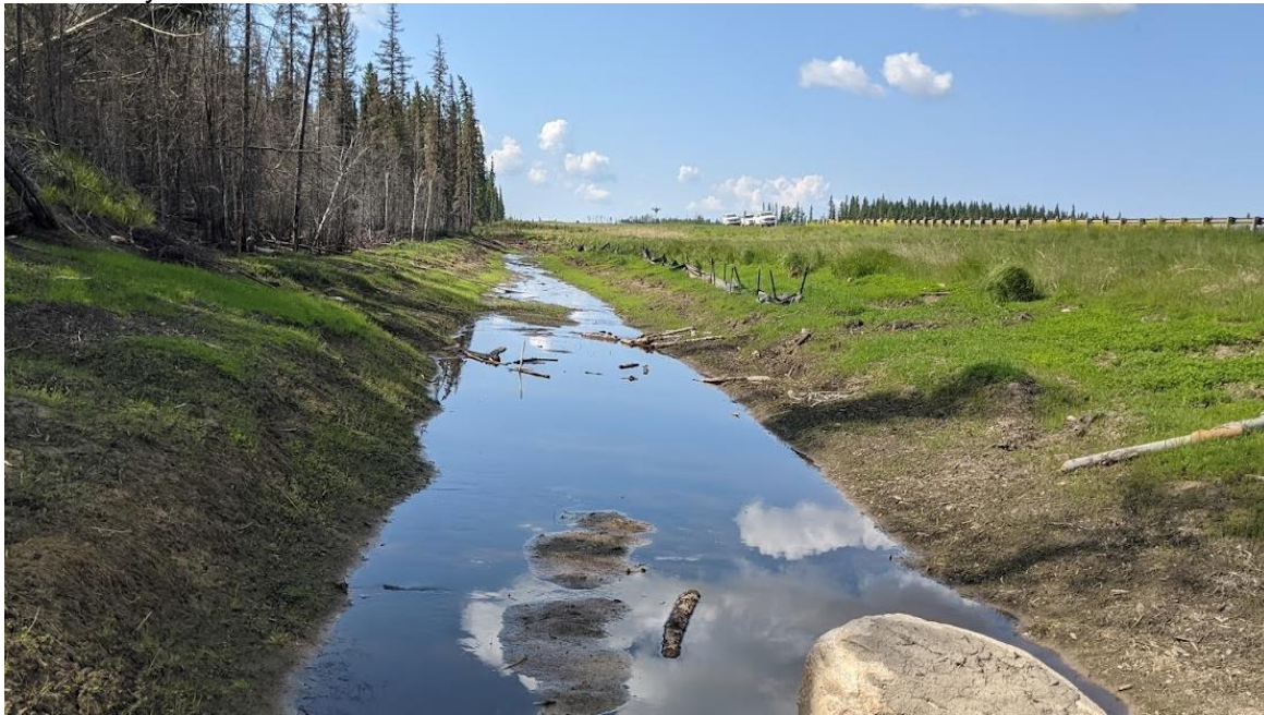
Photo No. 2 – Looking south at the highway west ditch; water is draining towards the eroded riprap channel to the east of the bridge
