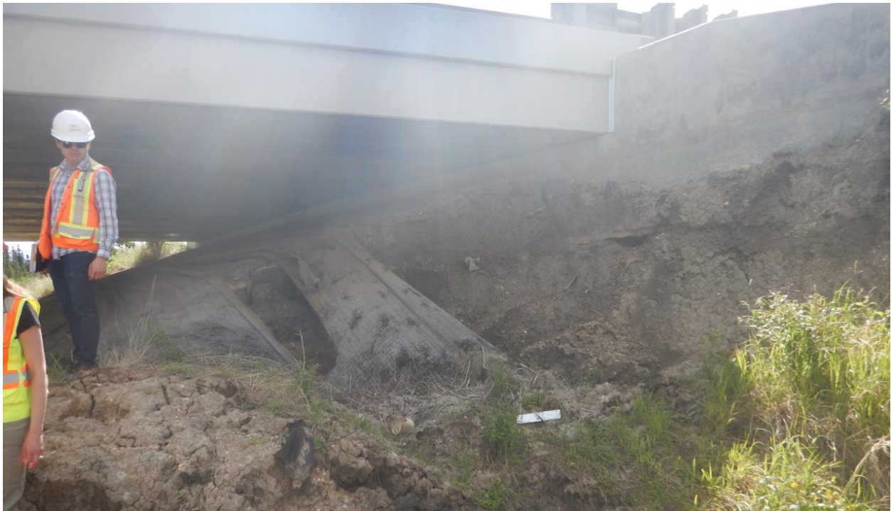
Photo No. 8 – Looking southeast at Slump No. 2 head scarp. Note (a) void developed under wing wall, (b) change in soil type between the area under the bridge and the area beyond (west of) the wing wall, and (c) eastern flank of slump extending below the bridge headslope
