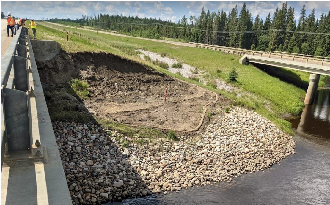
Photo No. 6 – Looking southwest at Slump No. 2
