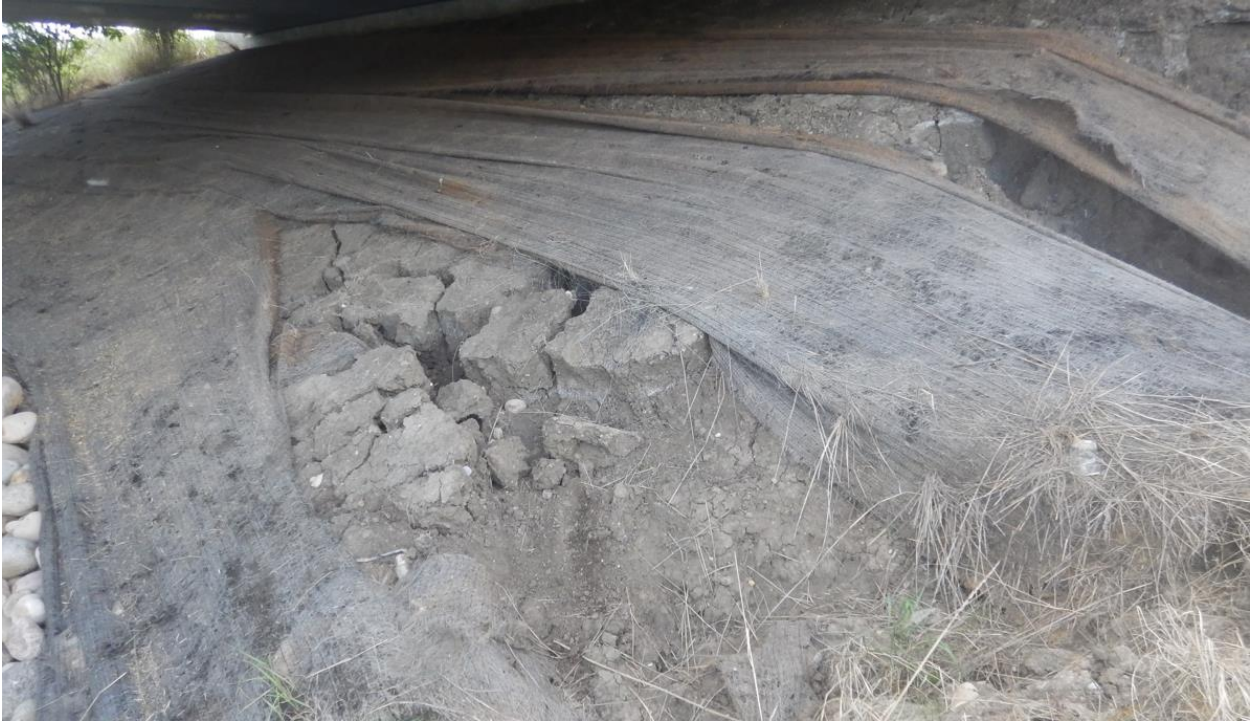
Photo No. 9 – Looking east at the portion of the head slope impacted by Slump No. 2
