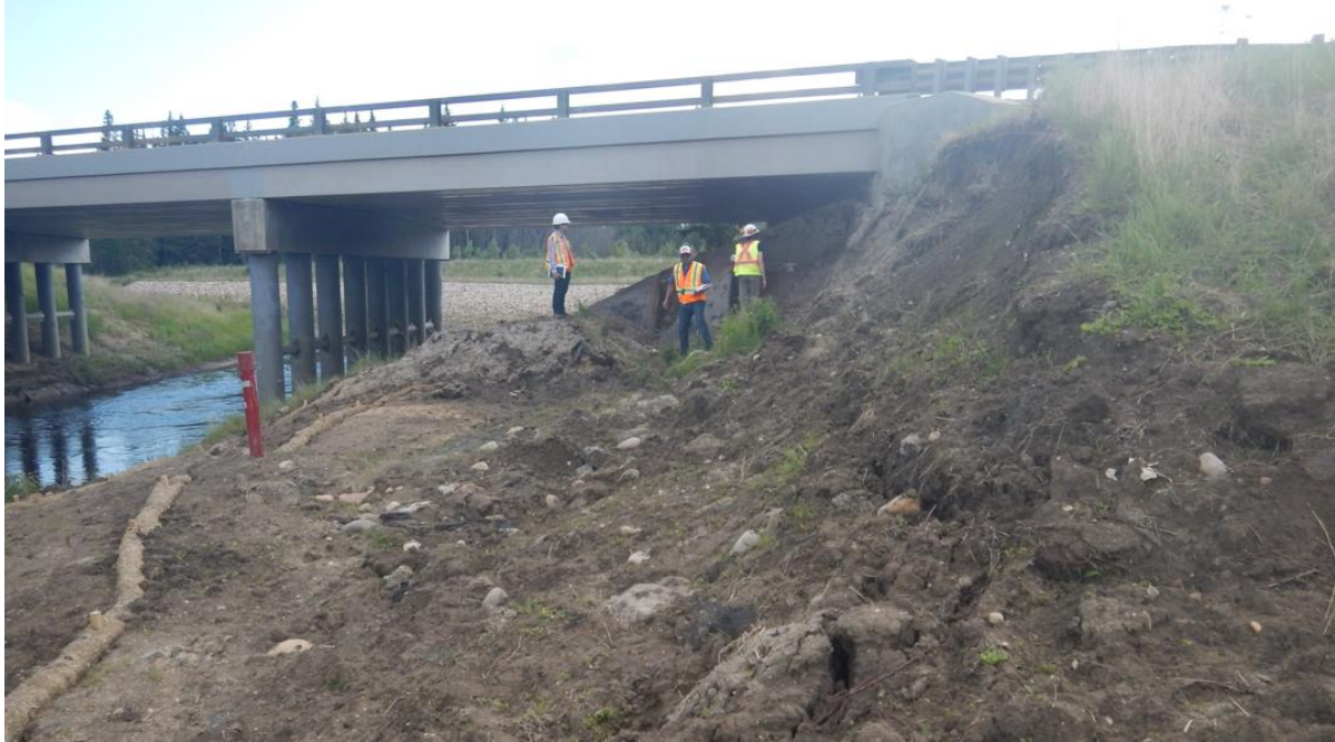
Photo No. 7 – Looking east at the head scarp of Slump No. 2
