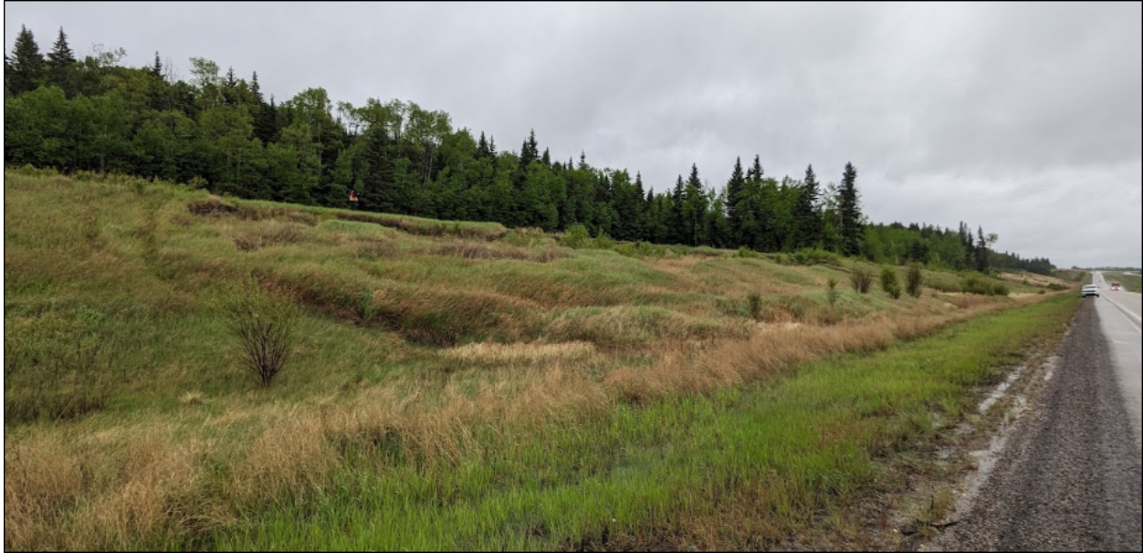
Photo No. 11 – NC091- 2: Looking south at landslide features; note the well-defined toe roll at the ditch and the presence of multiple tension cracks within the backslope
