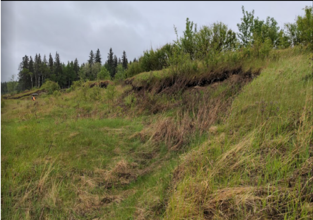
Photo No. 3- NC091-1: Looking north at landslide backscarp crack showing a 2.2 m drop approximately 5 m west of the upslope ditch
