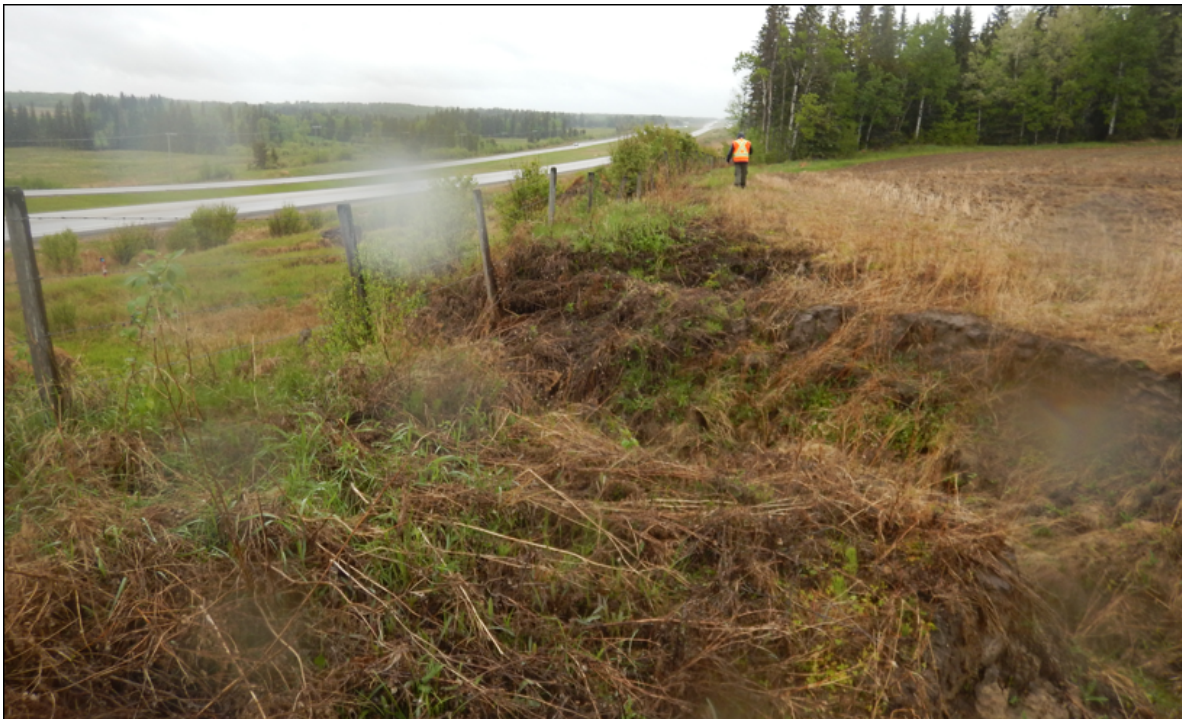
Photo No. 2- NC091-1: Looking north at an erosion gully developed within the farmer's field; vegetation grew within the gully
