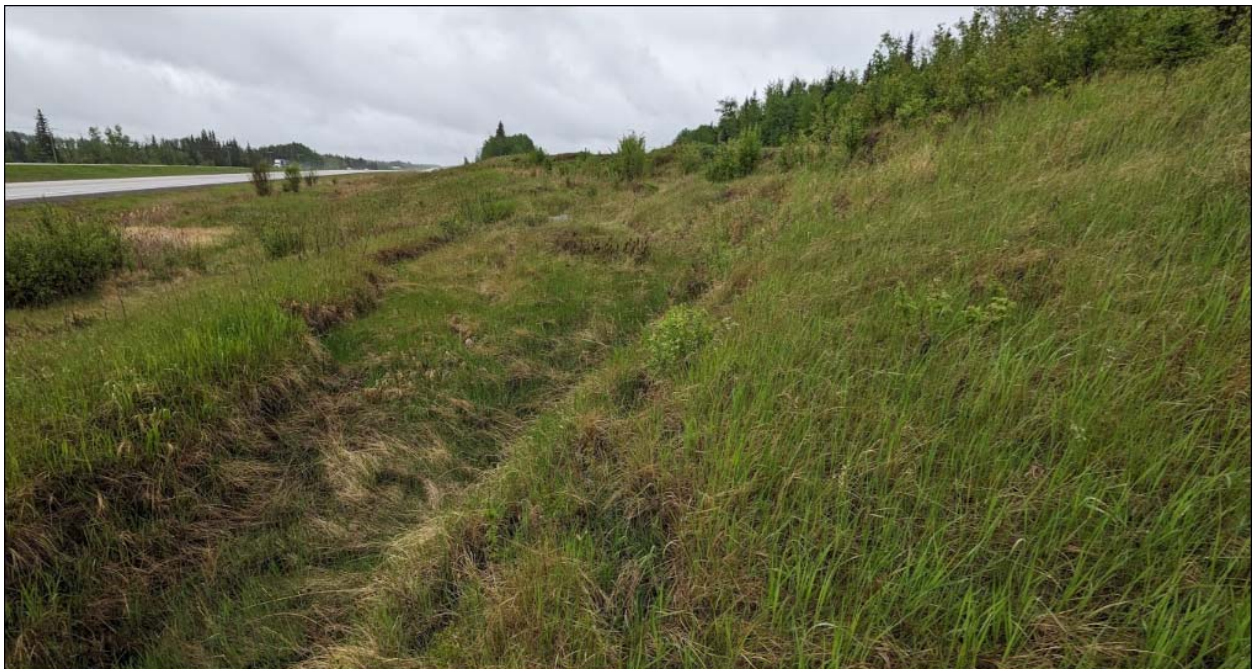
Photo No. 8 – NC091-2: Looking northeast at the southern flank of the landslide mass; note the presence of multiple tension cracks within the backslope
