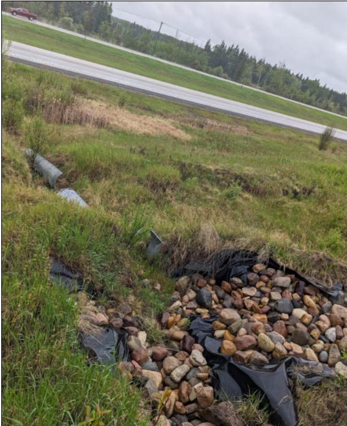
Photo No. 10 – NC091-2: Looking at the failed riprap apron
