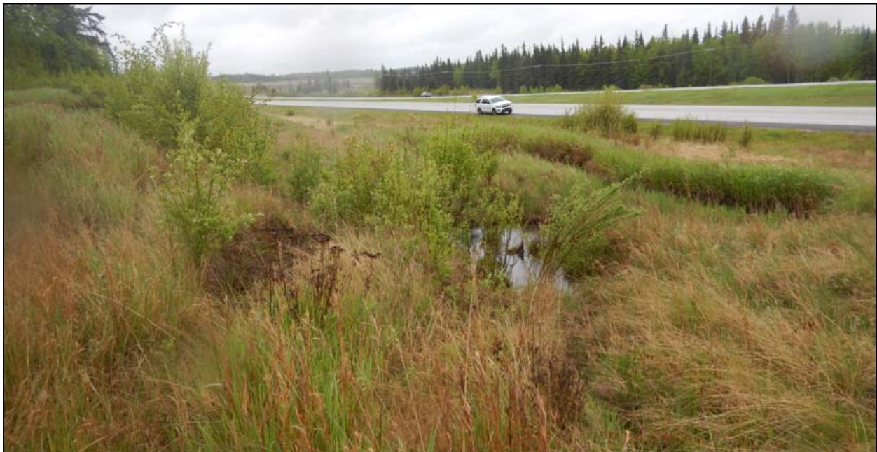
Photo No. 12 – NC091-2: Looking south at water ponding within the landslide mass
