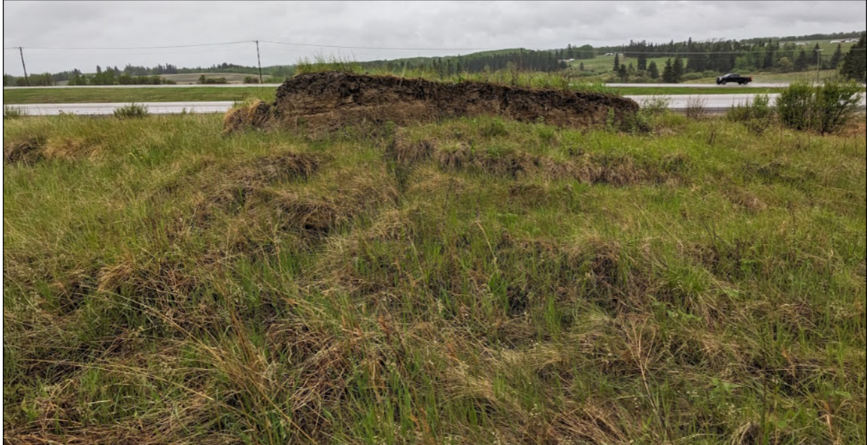
Photo No. 5 - NC091-1: Looking west at graben feature developed in the middle of the landslide mass
