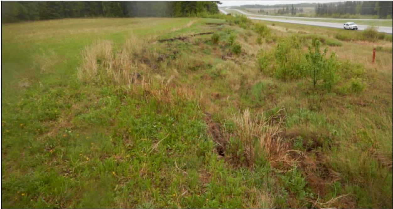
Photo No. 9 – NC091-2: Looking south at a scarp crack developed within the crest of the backslope
