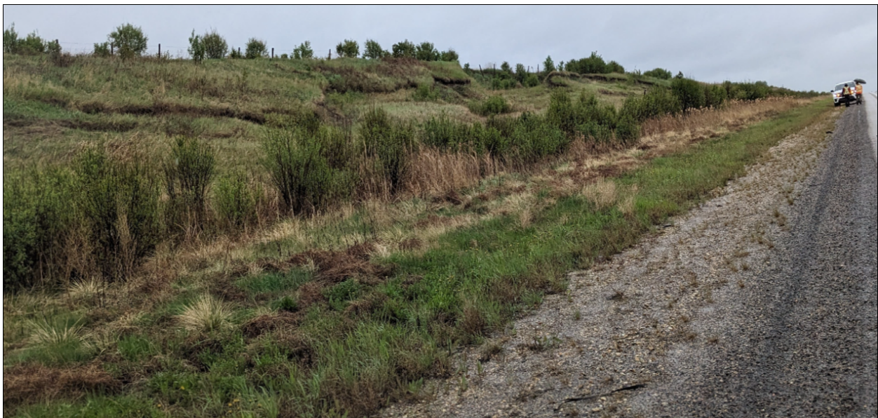
Photo No. 6 – NC091-1: Looking south at landslide features. The north flank extended further north in 2024
