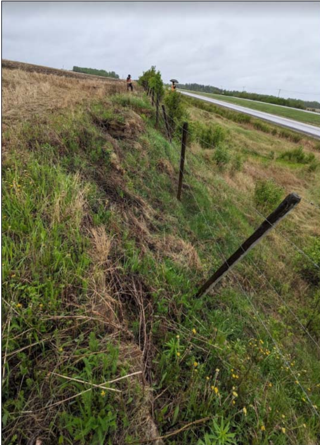
Photo No.4 - NC091-1: Looking south at a backscarp crack retrogressing into the farmer's field. Eight barbed wire posts were hanging in 2024.
