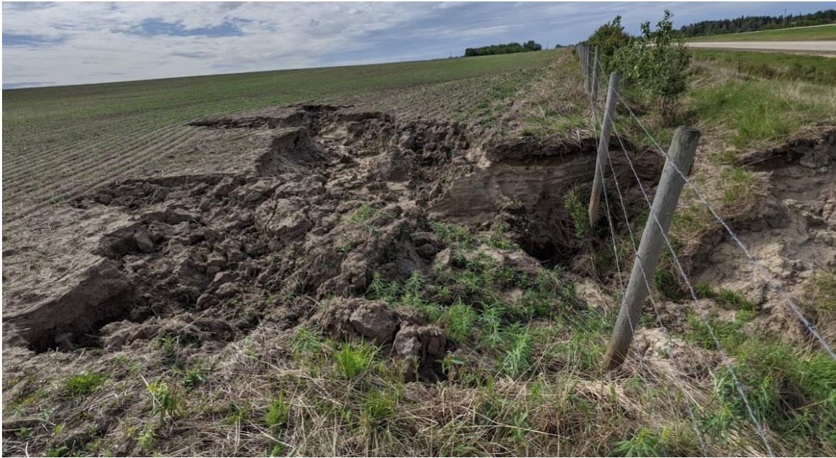
Photo No. 5 - NC091-1: Looking southwest at the head scarp crack and the erosion gully developed within the farmer's field
