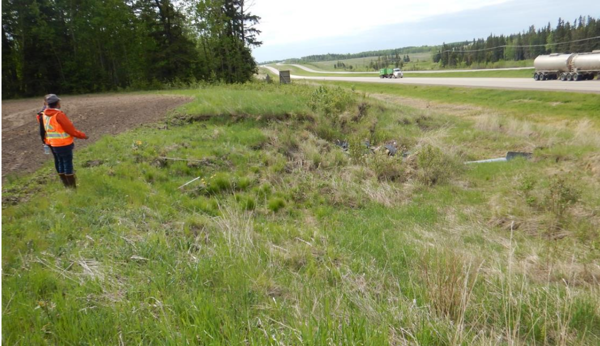
Photo No. 9 – NC091-2: Looking south at scarp crack developed within the crest of the backslope
