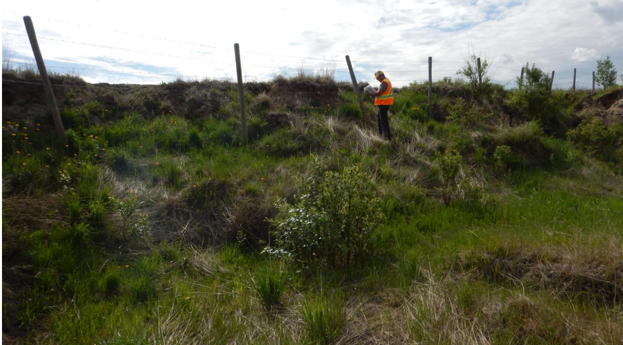
Photo No. 1- NC091-1: Looking southeast where the landslide cuts through catch water ditch; catch water ditch discharges water into the landslide mass
