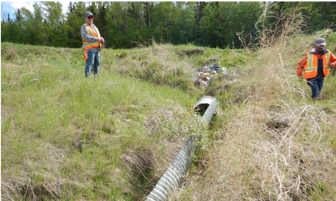
Photo No. 10 – NC091-2: Looking northeast at a scarp crack through the riprap apron and into the adjacent field (south scarp)
