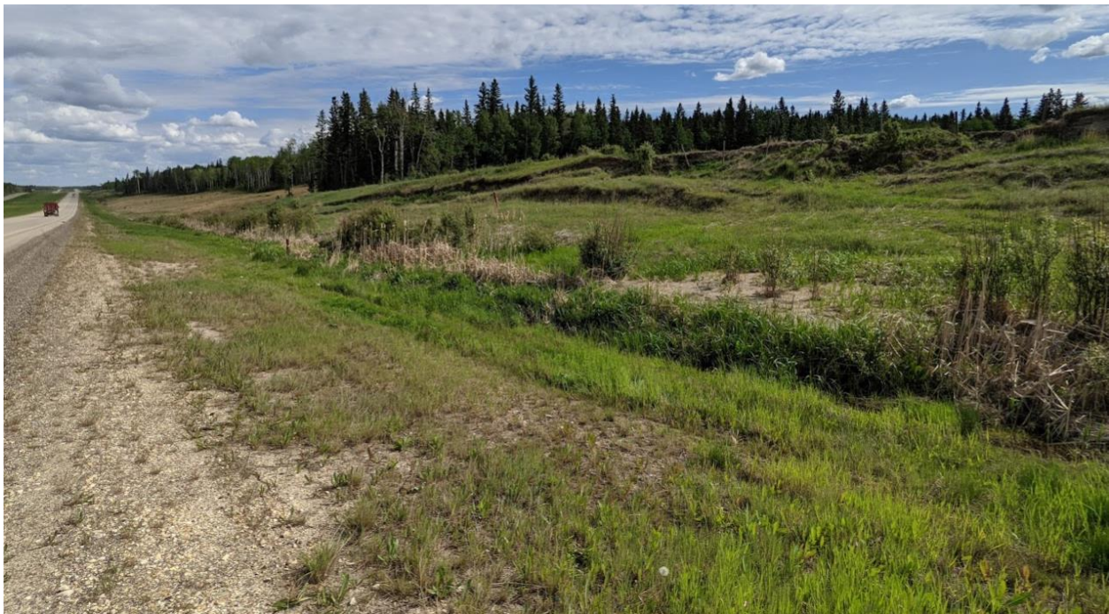
Photo No. 6 – NC091-1: Looking north at a distinct toe roll in the ditch
