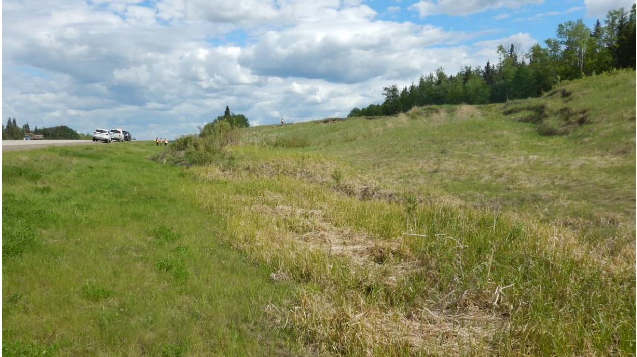
Photo No. 7 – NC091-2: Looking north at the landslide mass; note the presence of a distinct toe roll in the ditch
