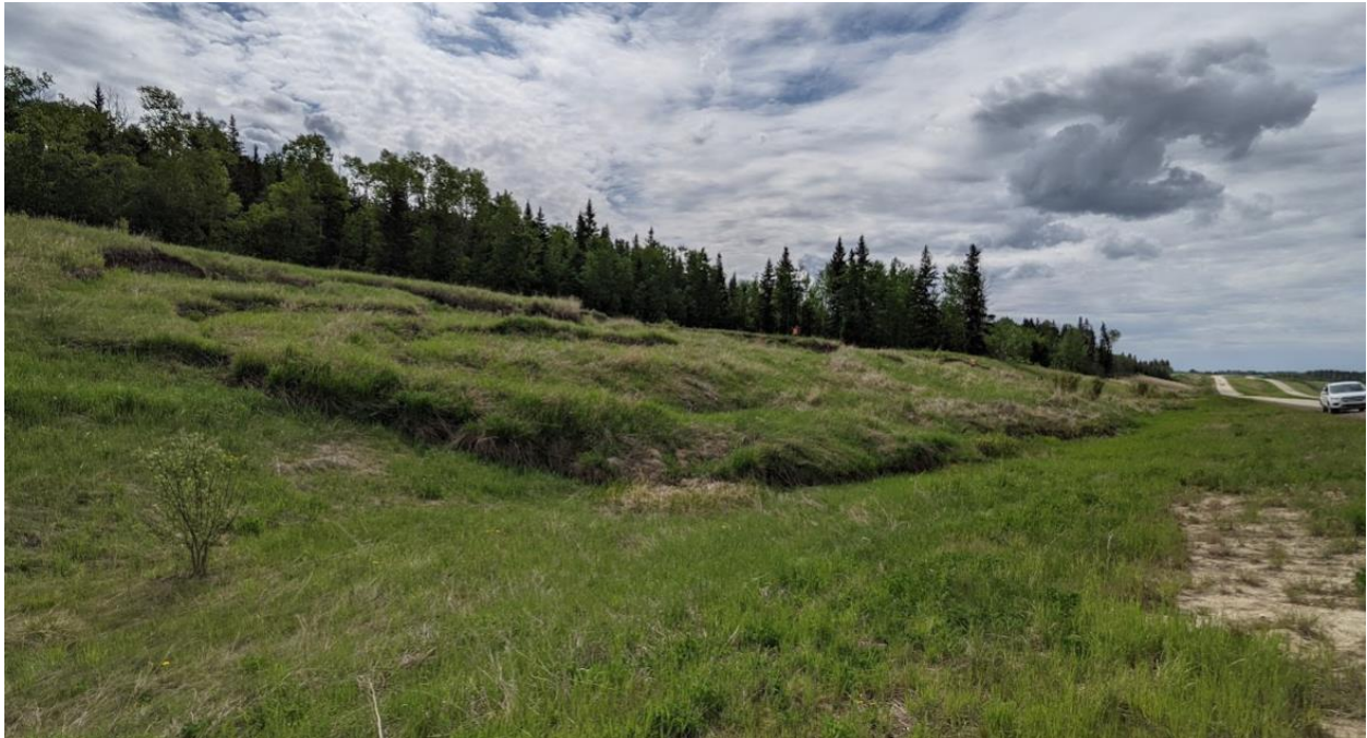
Photo No. 11 – NC091-2: Looking south at landslide features; note the well-defined toe roll at the ditch and the presence of multiple tension cracks within the backslope; landslide appears to be more vegetated than in 2020
