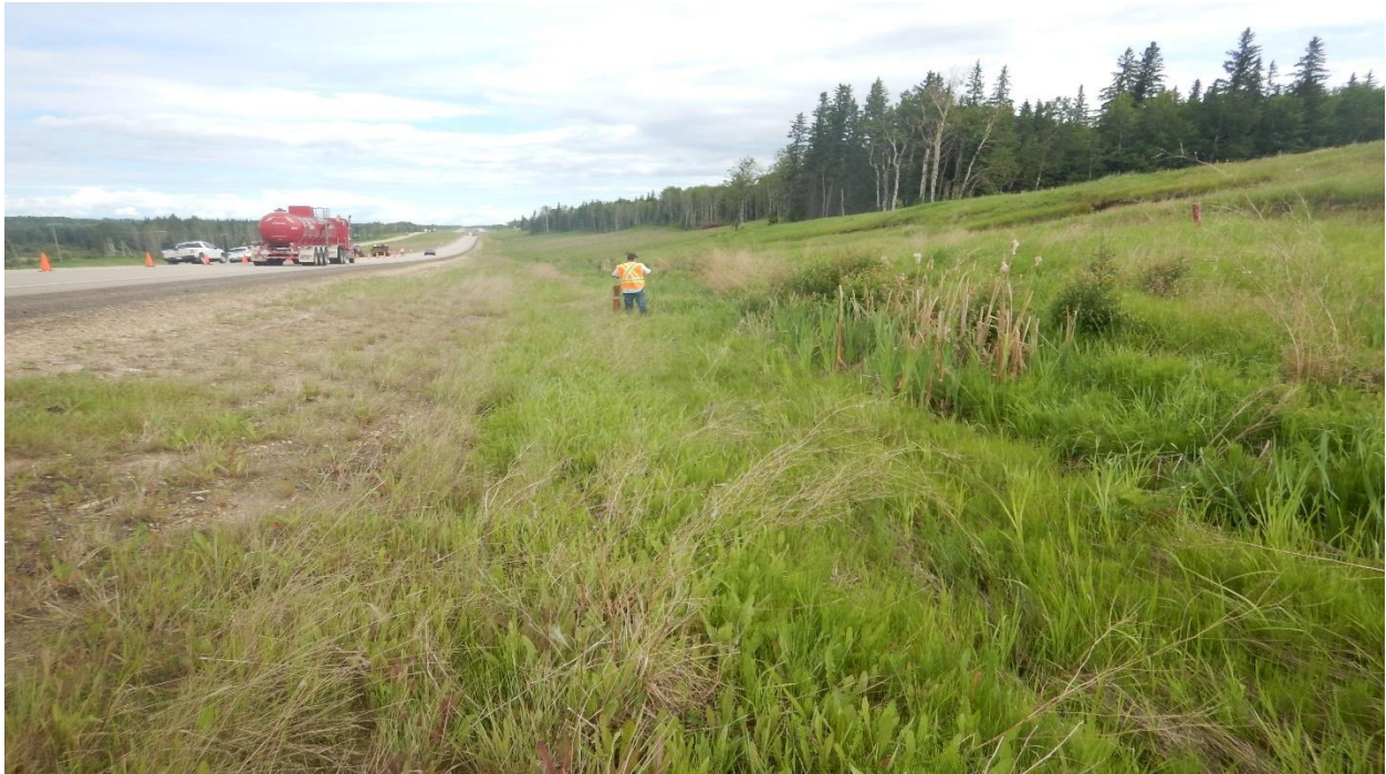
Photo No. 6 – NC091-1: Looking north at a distinct toe roll in the ditch
