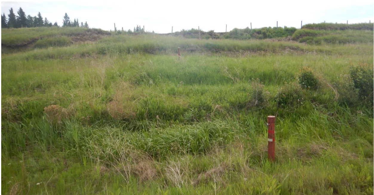
Photo No. 2- NC091-1: Looking east at multiple scarp cracks within the slope
