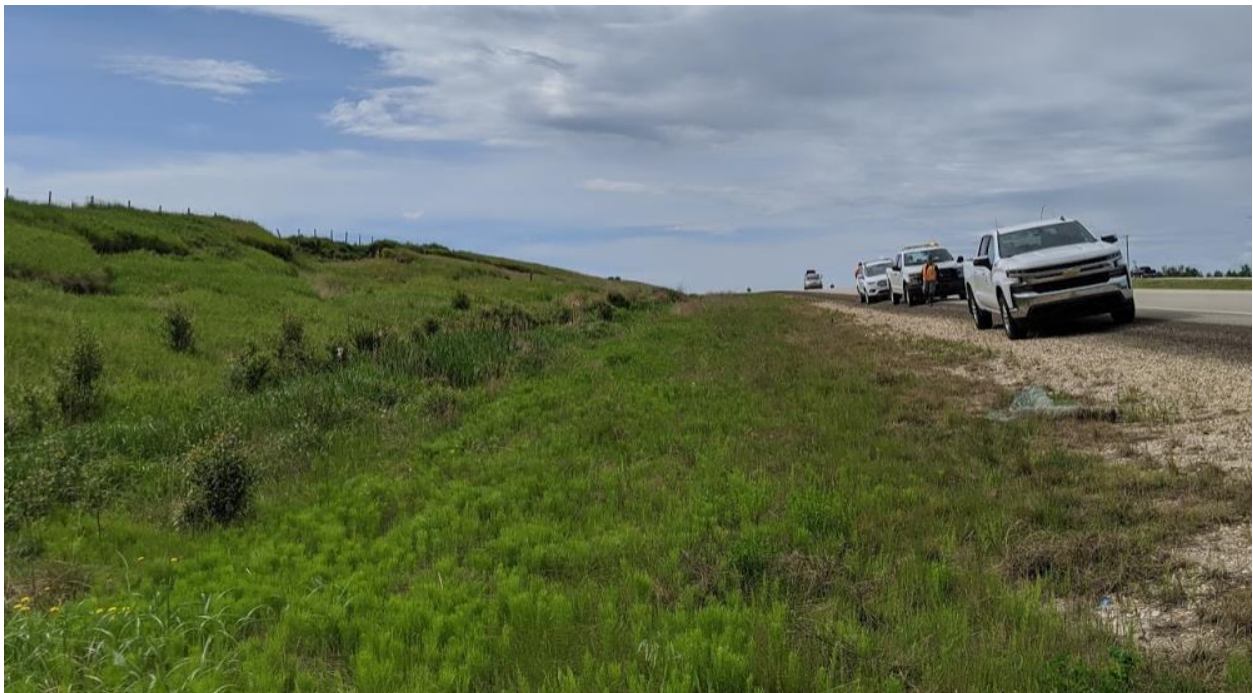
Photo No.3 - NC091-1: Looking south at the landslide mass
