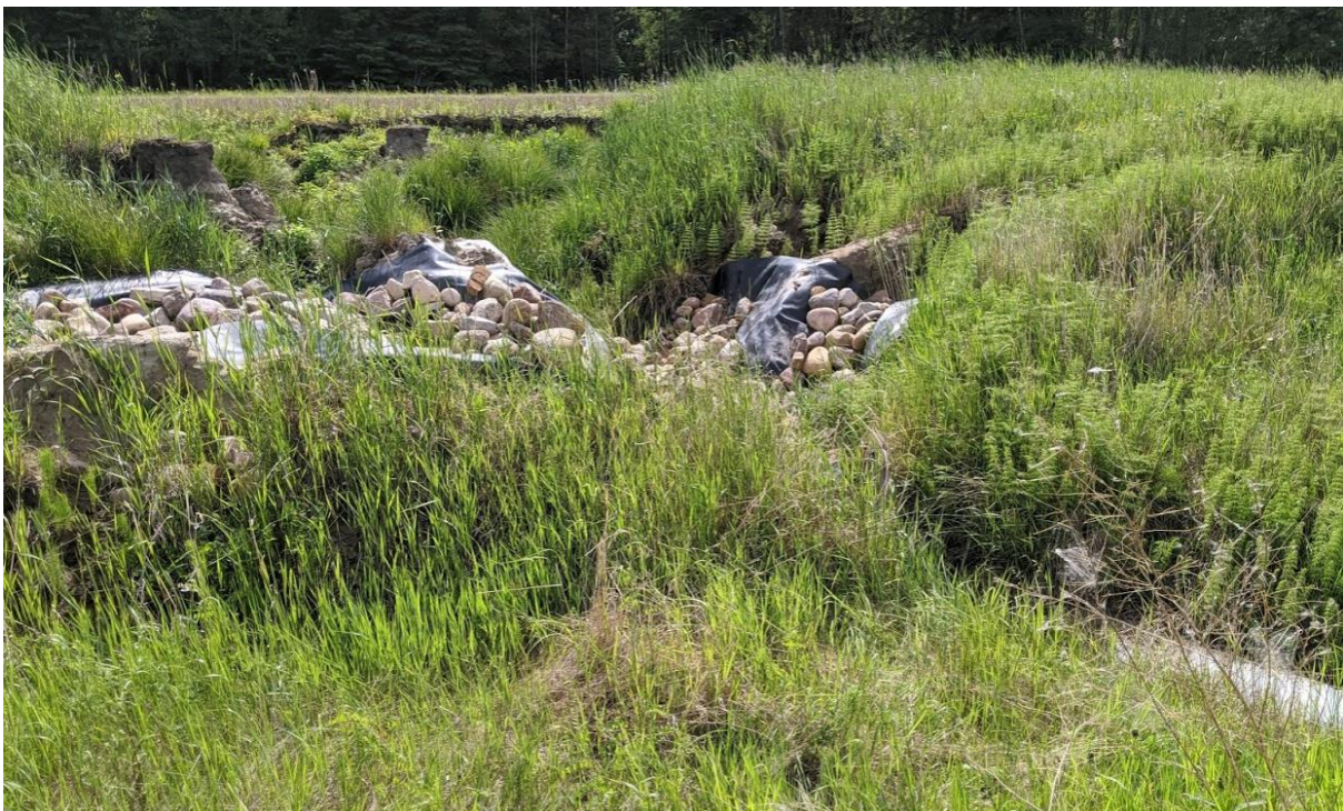
Photo No. 10 – NC091-2: Looking east at scarp through the riprap apron and into the adjacent field (south scarp).
