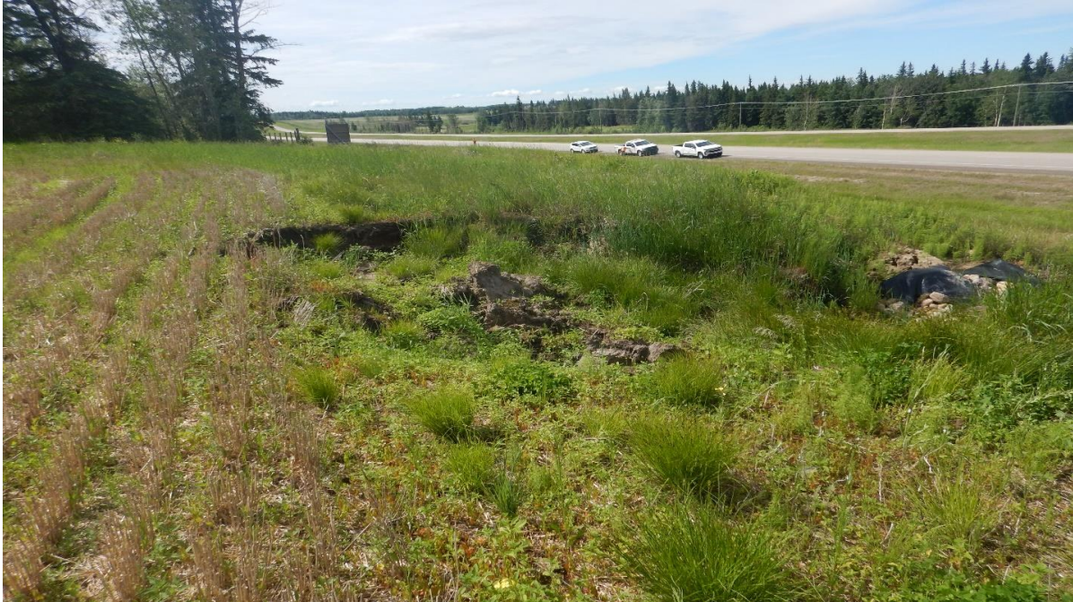
Photo No. 9 – NC091-2: Looking south at erosion developed within the crest of the slope at the riprap apron location
