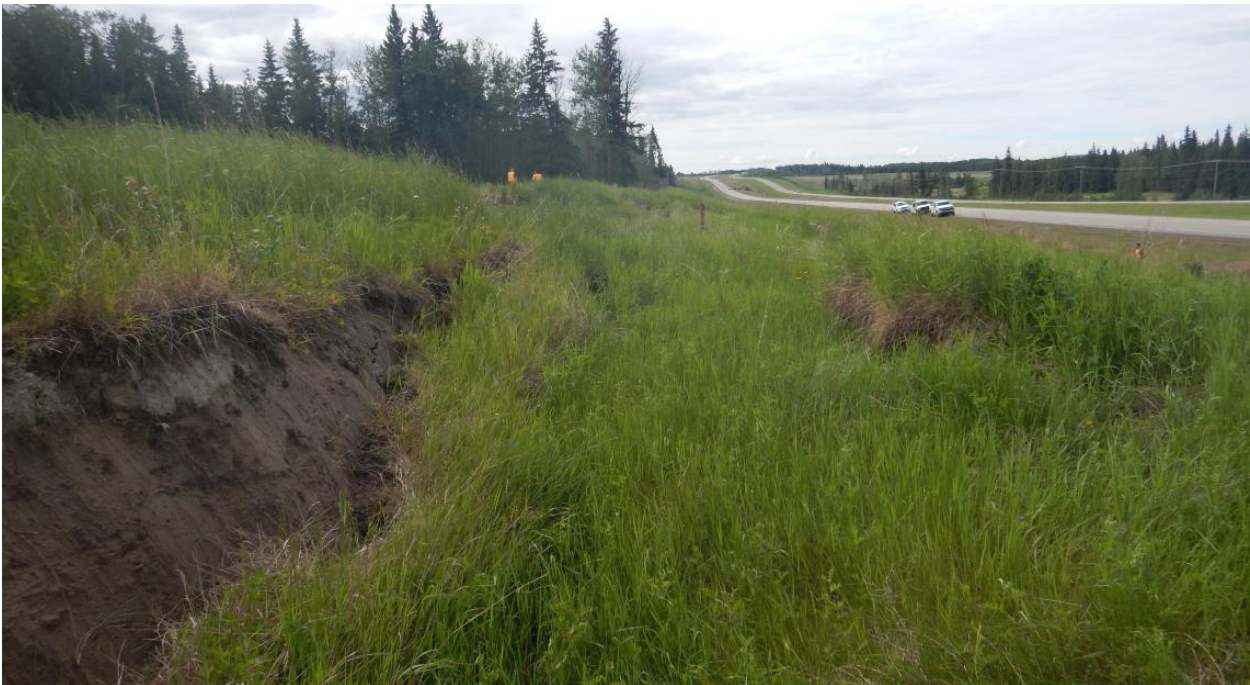
Photo No. 12 – NC091-2: Looking south from north portion at the graben block below the main scarp.
