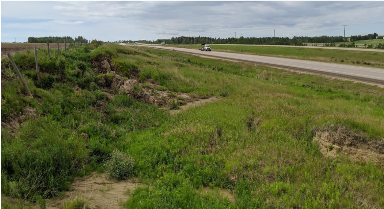
Photo No. 1- NC091-1: Looking south where the landslide cuts through catch water ditch; catch water ditch discharges water into the landslide mass
