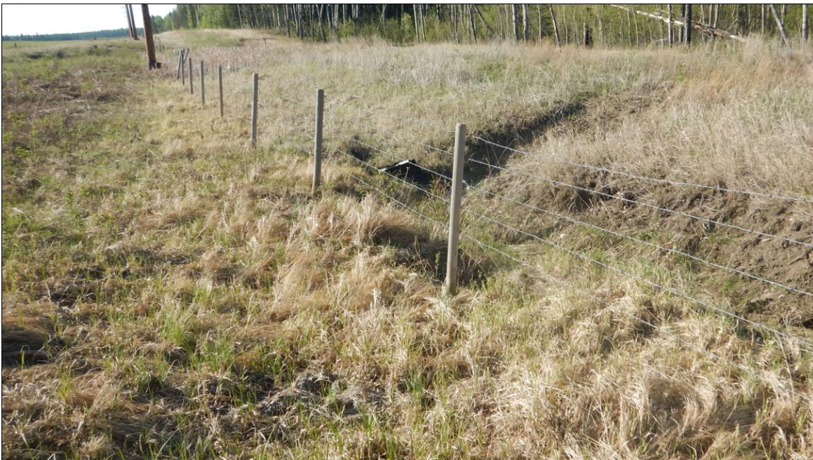
Photo No.2 – Sinkhole above the 800 mm diameter culvert; looking at the culvert inlet
