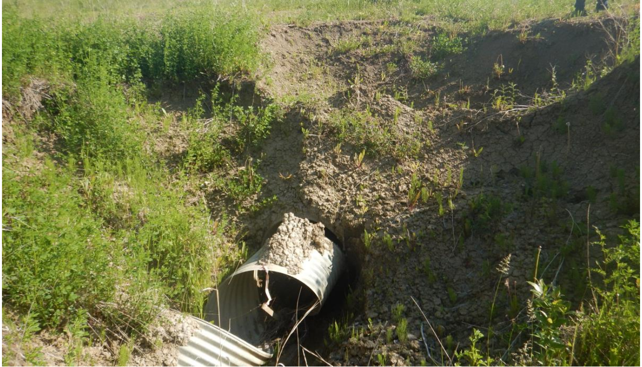
Photo No.5 – Looking at ruptured section of pipe at sinkhole location
