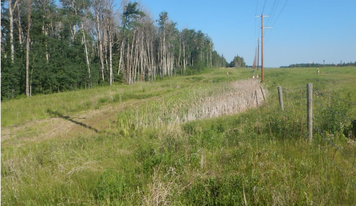
Photo No.7 – Southern flank of upper and lower landslide blocks (Looking North); note standing water within the flank and lateral shifting of existing fence
