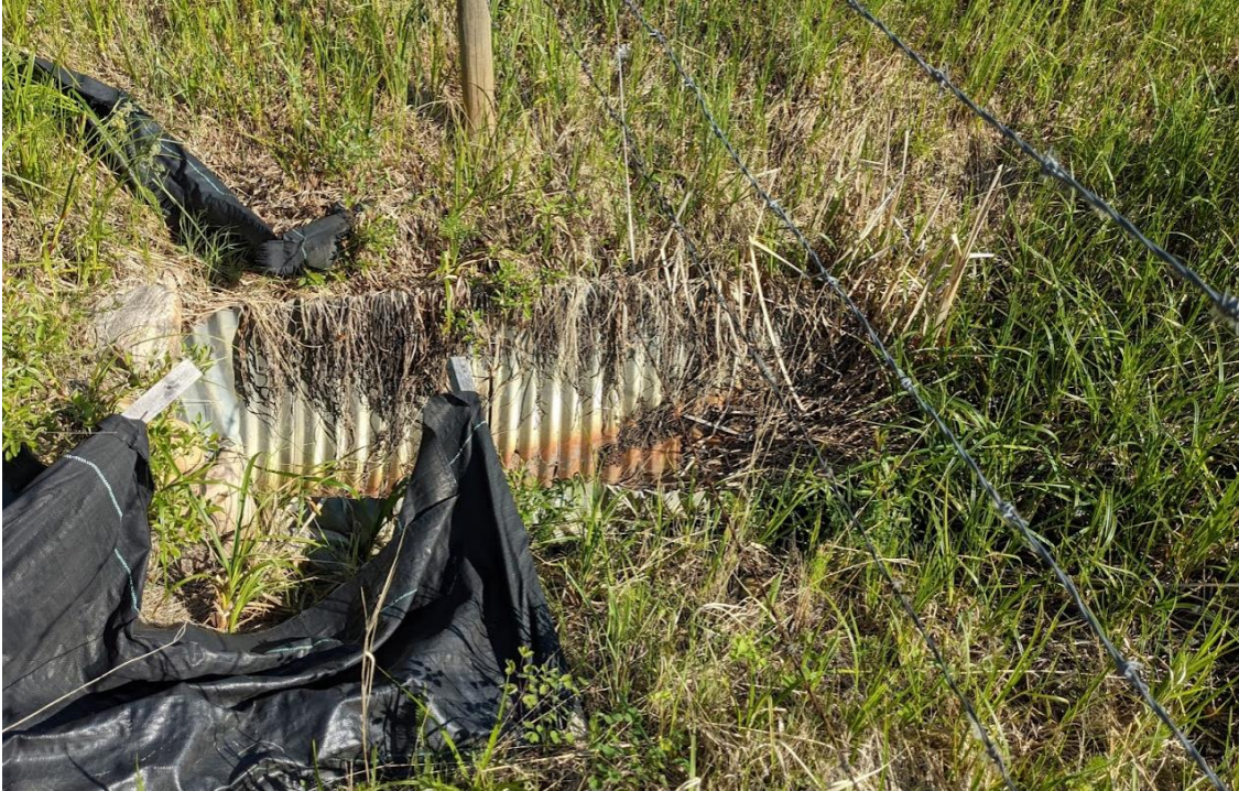
Photo No. 9 – 700 mm diameter CSP culvert C3 inlet; water is flowing under culvert
