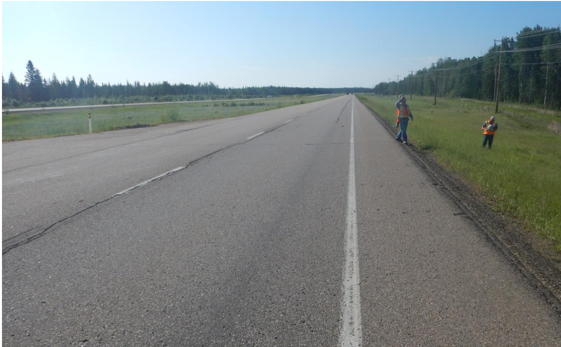
Photo No. 11 – Looking south at highway southbound lanes; landslide is not currently impacting the highway surface; head scarp crack is about 6.5 m away from the edge of pavement
