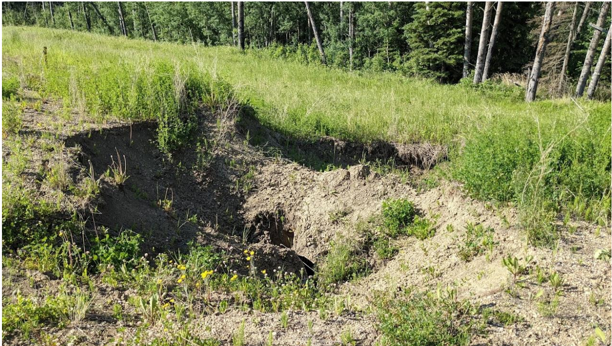
Photo No.4 – Sinkhole above the 800 mm diameter culvert; looking at the culvert separation area near the outlet location (6 m diameter x 1.5 m deep)
