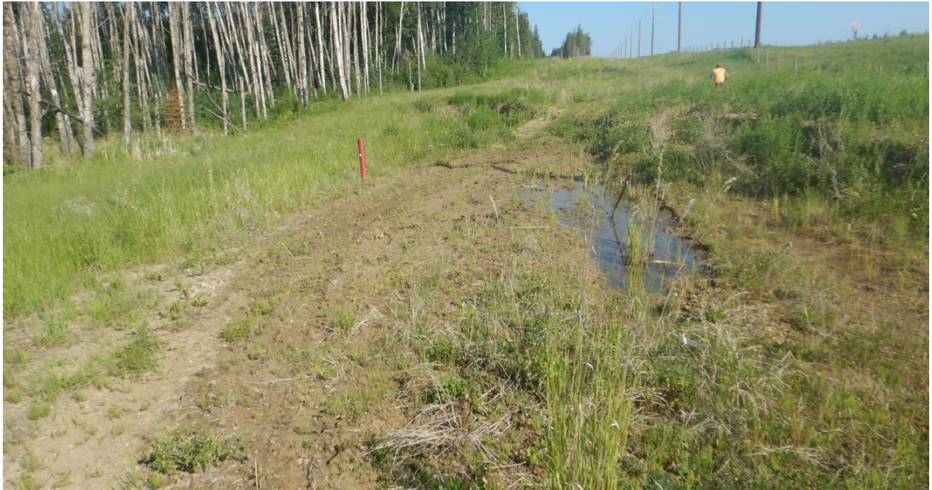
Photo No.6 – Looking north at lower landslide block; water is ponding beside the 1 m deep head scarp crack
