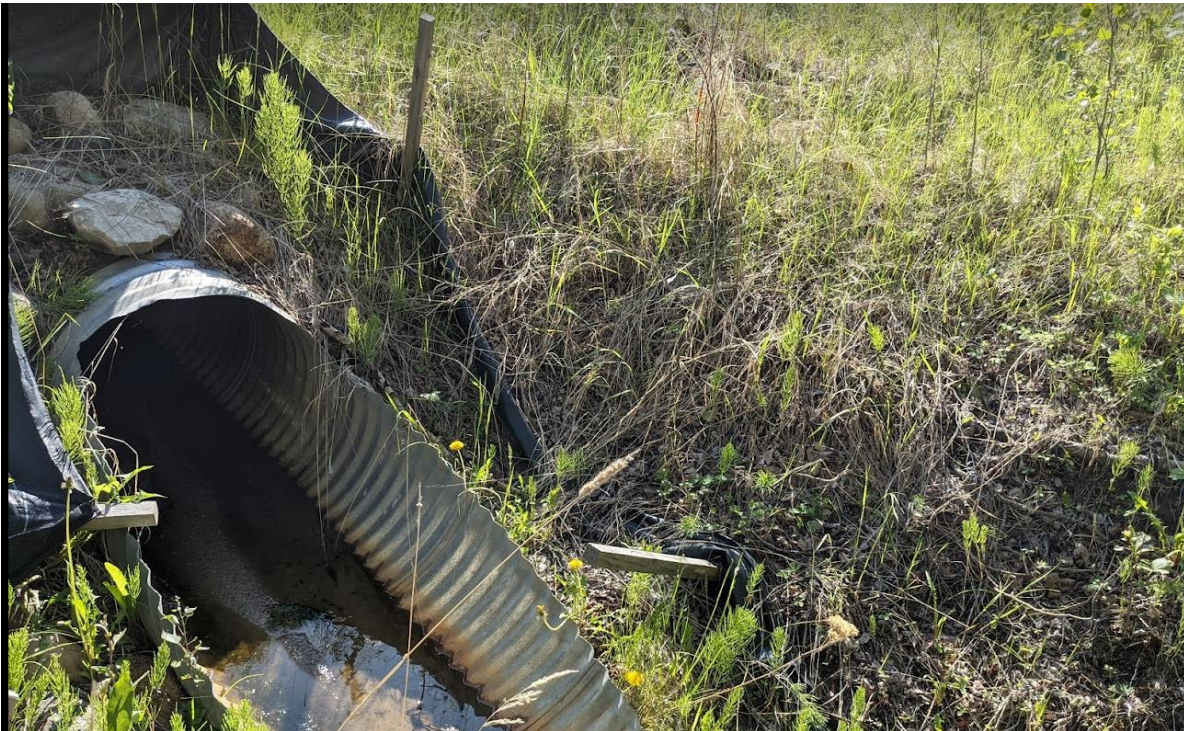
Photo No.8 – 700 mm diameter CSP culvert C3 outlet; note sediment accumulation inside the culvert; minor flow from the outlet of the culvert was noted in 2021
