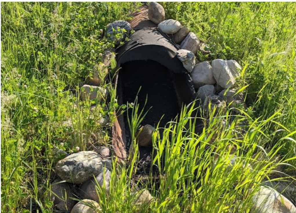
Photo No.10 – Outlet of 800 mm diameter culvert C1; note sediment at the culvert outlet; ground surface is a bit higher than the culvert invert at outlet
