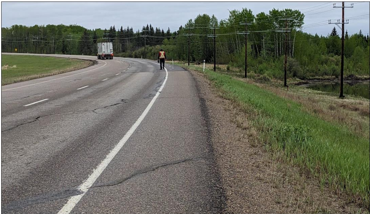
Photo No. 8 – Looking south at the southern flank cracks of the NC08-1 repaired landslide
