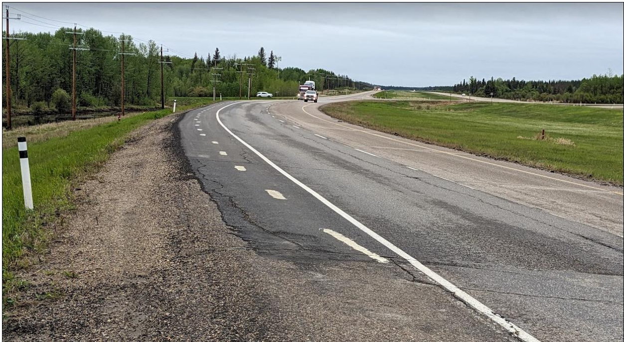
Photo No. 12 – Looking north at reflective cracks, 30-70 mm wide with 10 mm drop, near the southern flank of the NC08-2 landslide
