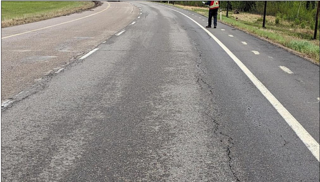
Photo No. 10 – Looking south at reflective cracks within the middle section of the NC08-2 landslide
