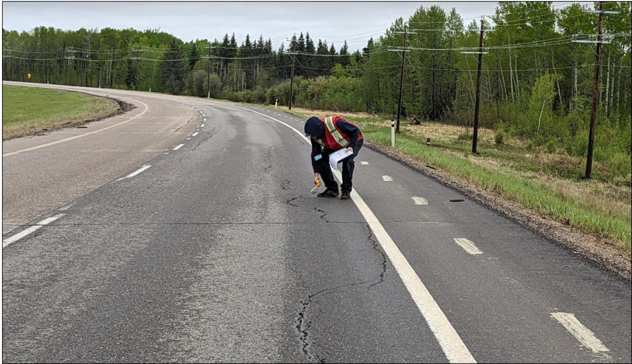
Photo No. 11 – Looking south at, 30-40 mm wide with no drop, reflective cracks near the southern flank of the NC08-2 landslide
