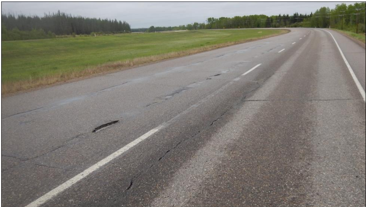
Photo No. 6 – Looking south at highway open cracks and potholes within the limits of the NC08-1 repaired area
