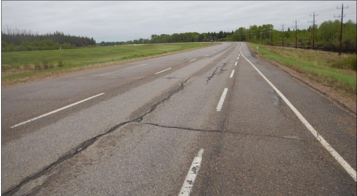
Photo No. 5 – Looking south at highway open cracks within the limits of the repaired area in 1997 (previously known as NC08-1)
