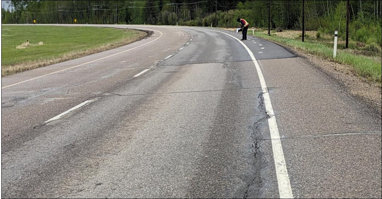
Photo No. 9 – Looking south at the northern flank of the new landslide (NC08-2); new ACP patch placed in 2022 showing reflective cracks (20 mm to 70 mm wide)
