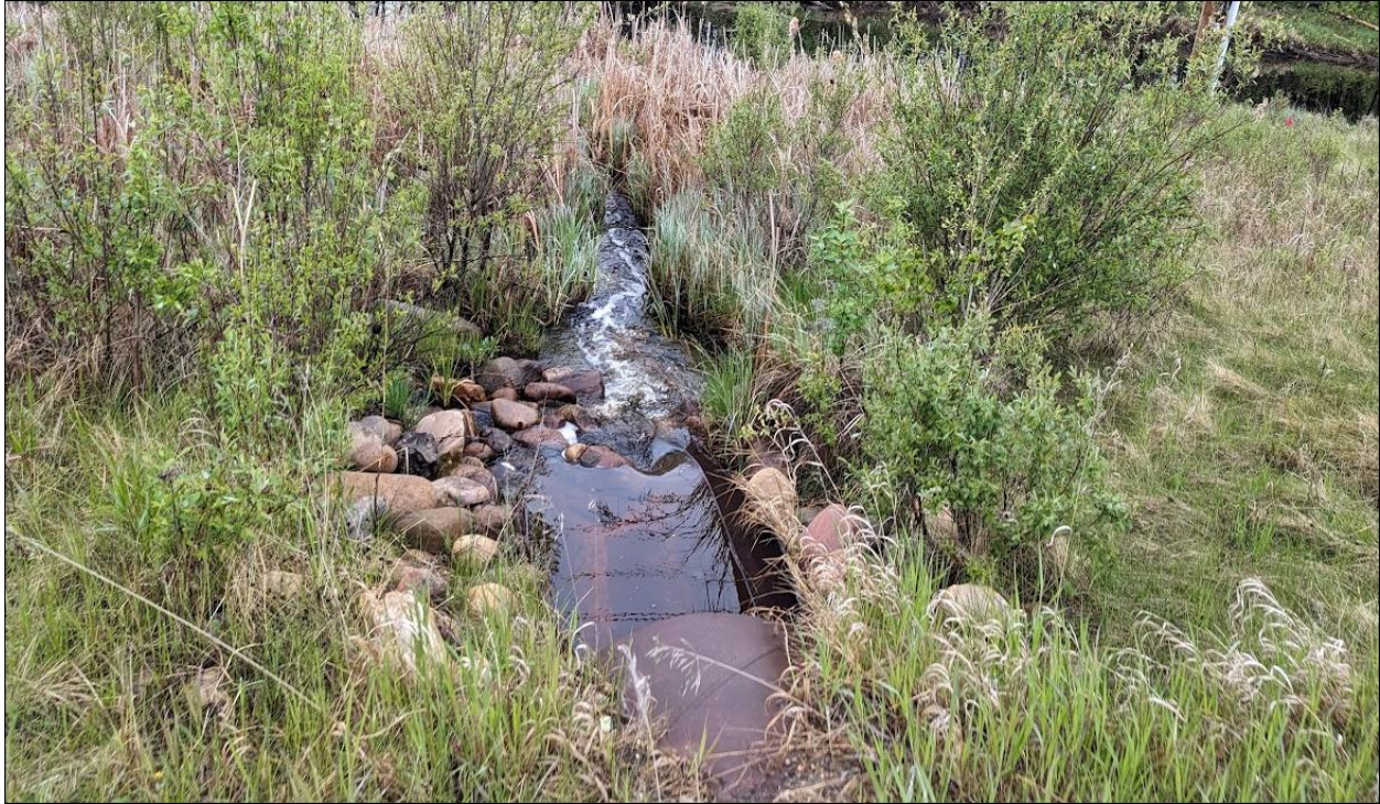
Photo No. 7 – Looking at the 900 mm diameter SWSP Culvert C2 outlet; heavy flow in 2024
