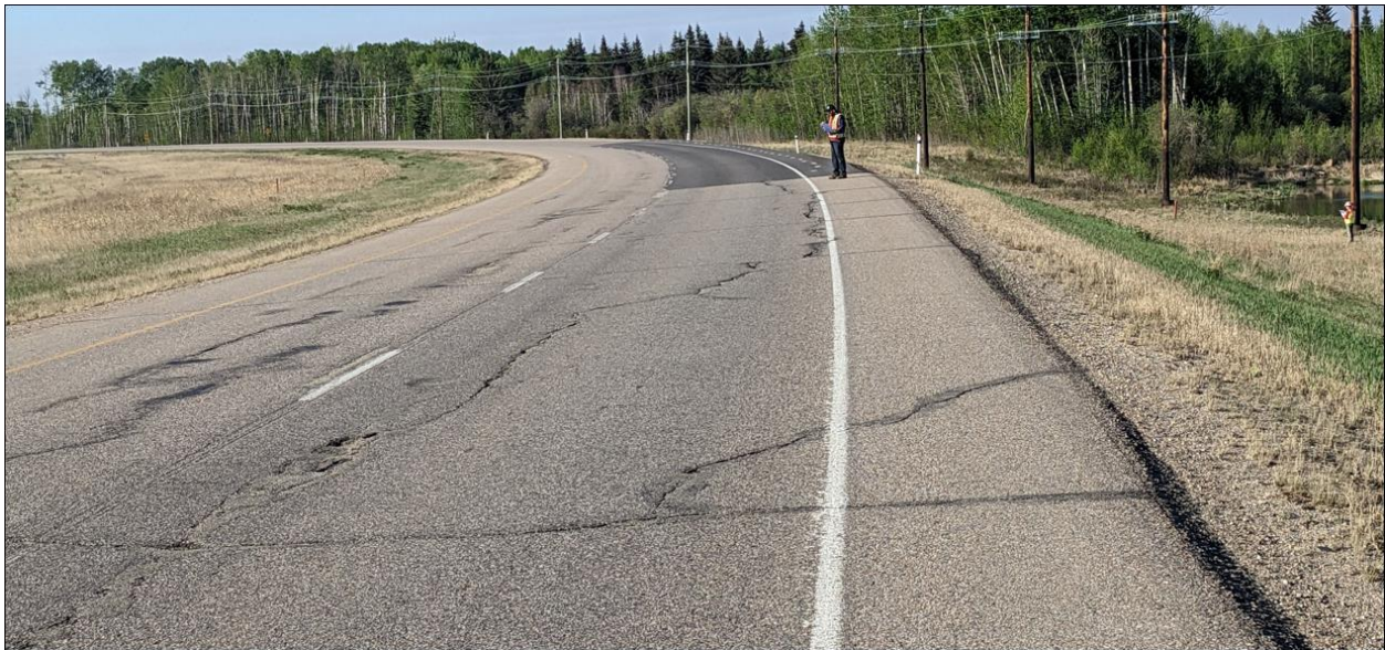
Photo No. 8 – Looking south at the southern flank cracks of the NC08-1 repaired landslide
