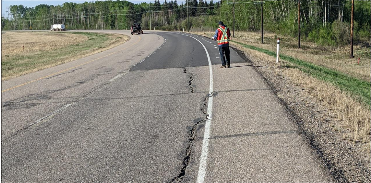
Photo No. 9 – Looking south at the northern flank of the new landslide (NC08-2); note new ACP patched placed in 2022 already showing reflecting cracks
