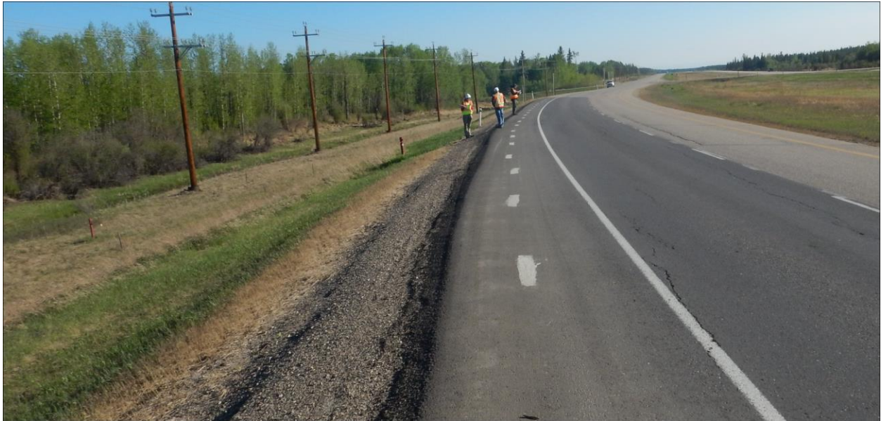
Photo No. 12 – Looking north at reflective cracks near the southern flank of the NC08-2 landslide
