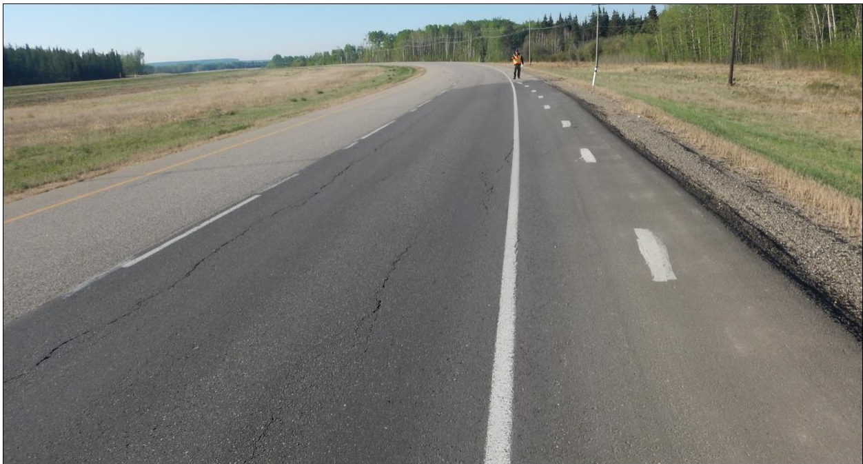
Photo No. 10 – Looking south at reflective cracks within the central portion of the NC08-2 landslide
