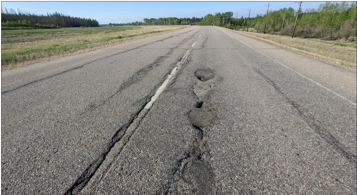
Photo No. 6 – Looking south at highway open cracks and potholes within the limits of the NC08-1 repaired area
