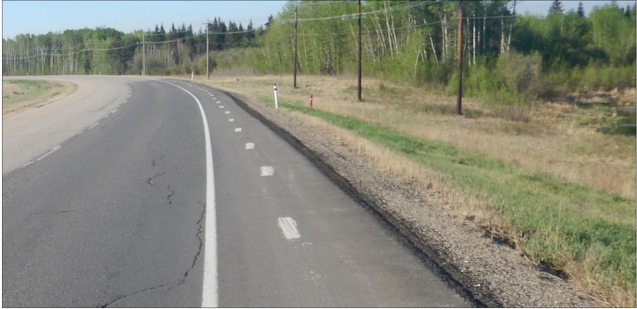
Photo No. 11 – Looking south at reflective cracks near the southern flank of the NC08-2 landslide
