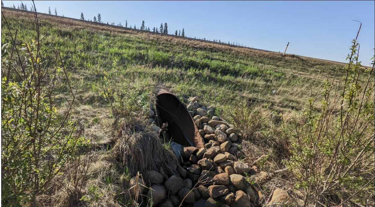
Photo No. 7 – Looking at 900 mm diameter SWSP Culvert C2 outlet; heavy flow in 2023
