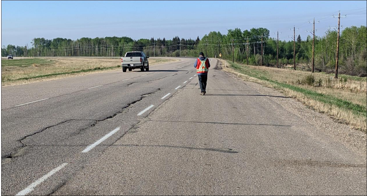
Photo No. 5 – Looking south at highway open cracks within the limits of the repaired area in 1997 (previously known as NC08-1)
