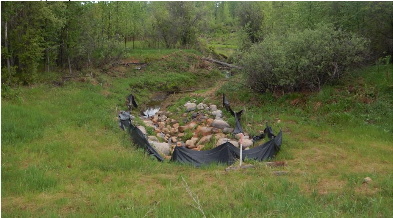
Photo No. 2 – Looking northeast at Culvert C1 outlet; water continues to flow freely along the channel
