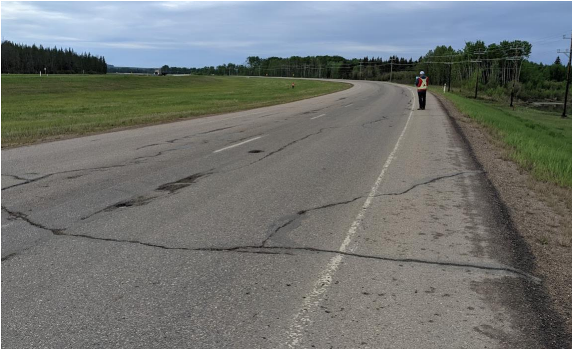
Photo No. 9 – Looking south at the southern flank cracks of the NC08-1 repaired landslide
