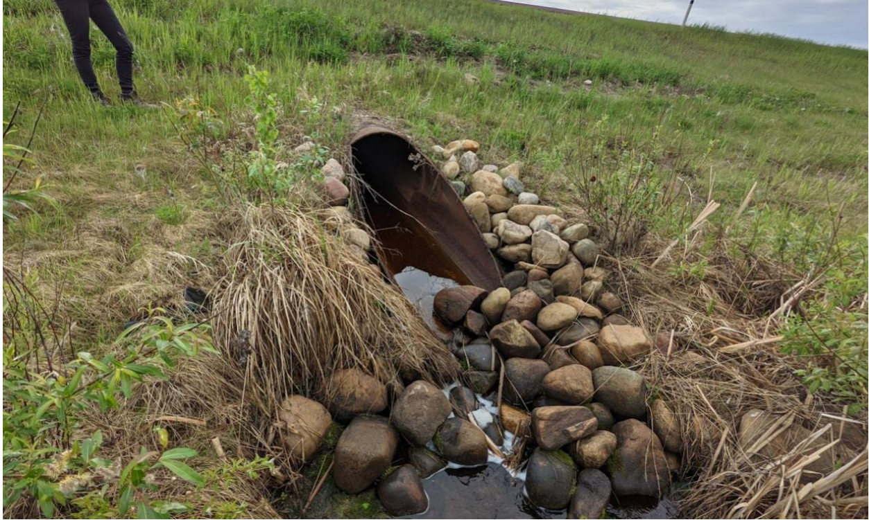
Photo No. 7 – Looking at 900 mm diameter SWSP Culvert C2 outlet; heavy flow in 2022
