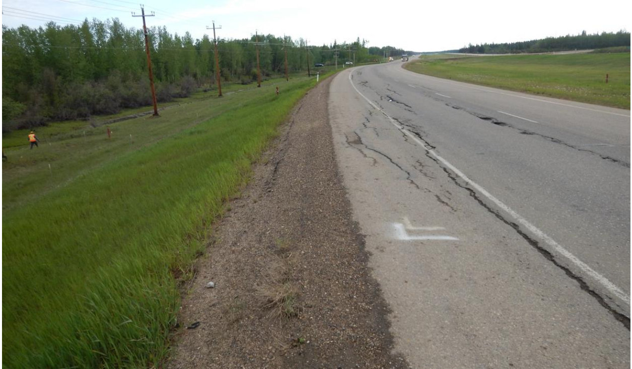
Photo No. 13 – Looking north at highway cracks near the southern flank of the NC08-2 landslide
