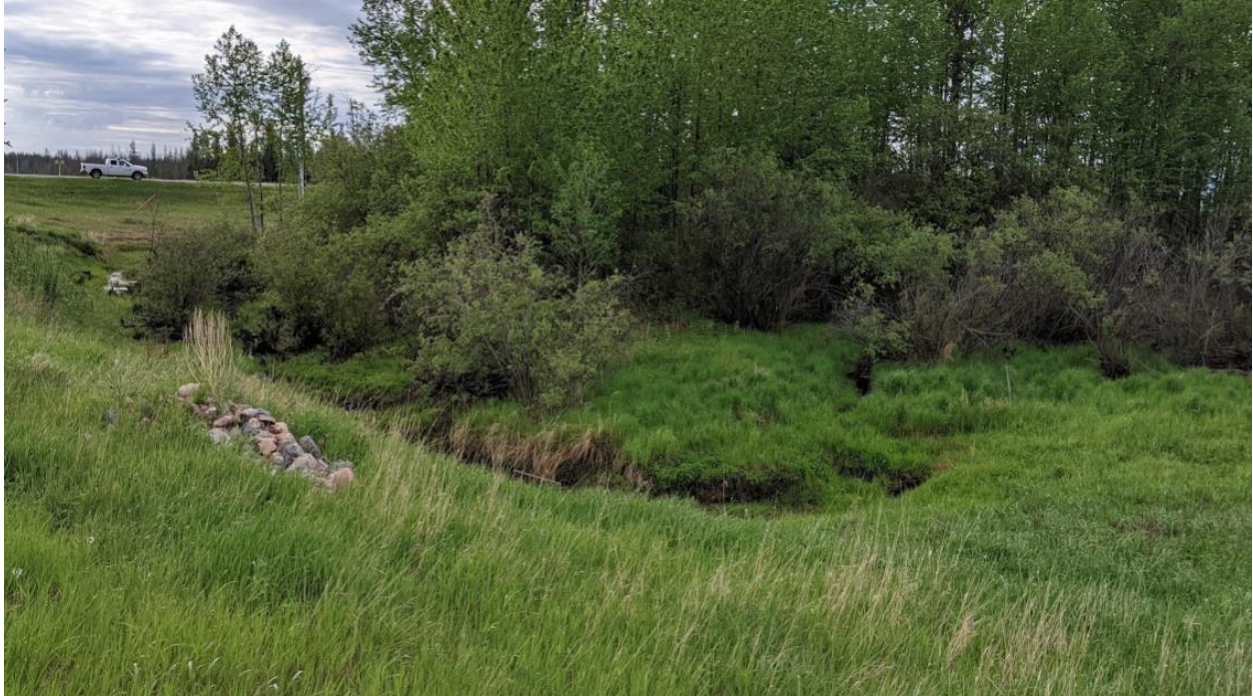
Photo No. 3 – Looking east towards CSP culvert C1 outlet; note that this area was submerged under water in 2020
