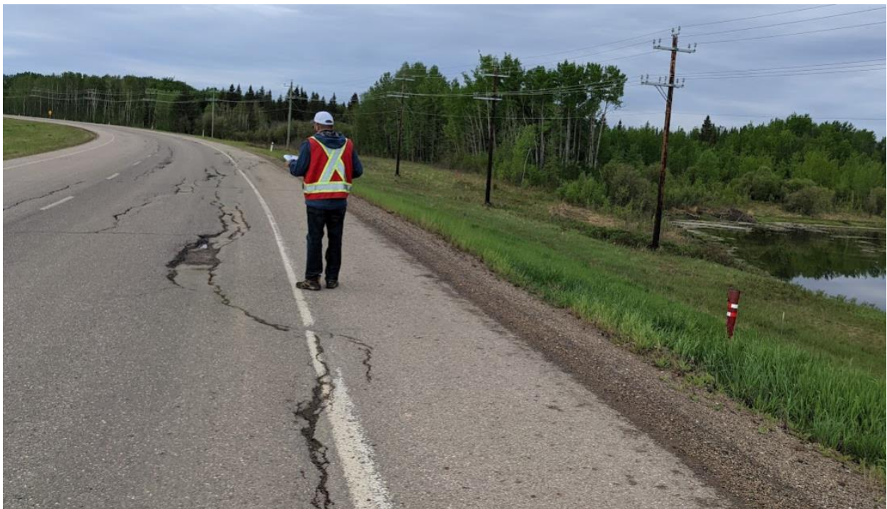
Photo No. 12 – Looking south at highway cracks near the southern flank of the NC08-2 landslide
