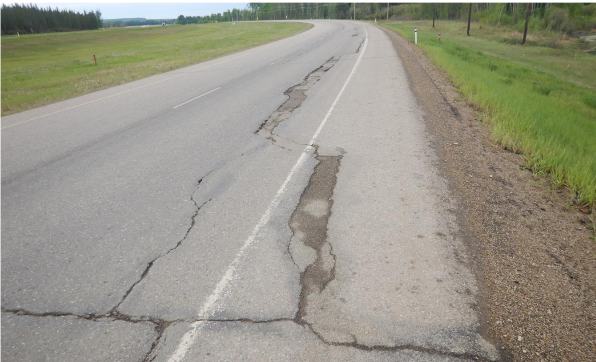
Photo No. 10 – Looking south at the northern flank of the new landslide (NC08-2); note exiting drop within the highway lane
