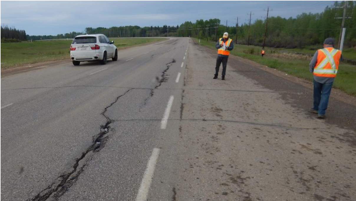
Photo No. 5 – Looking south at highway open cracks within the limits of the repaired area in 1997 (previously known as NC08-1)
