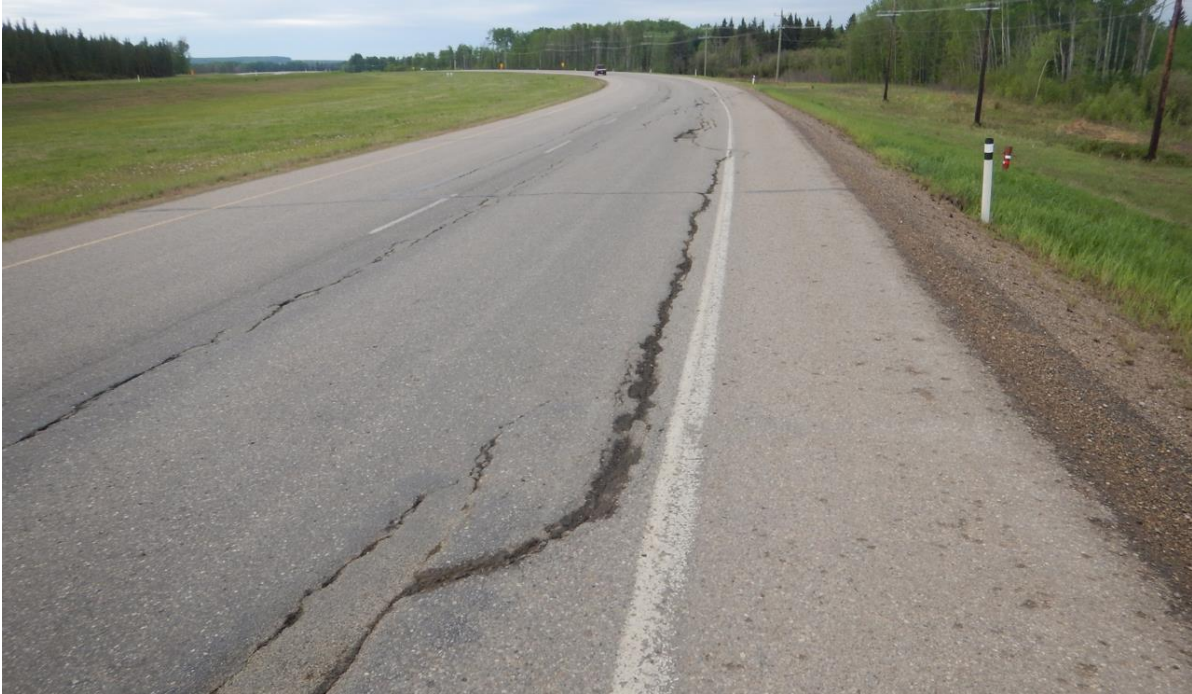
Photo No. 11 – Looking south at highway cracks within the central portion of the NC08-2 landslide
