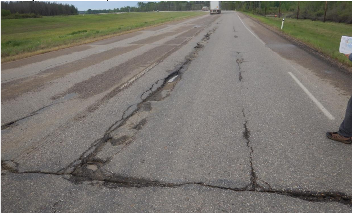
Photo No. 6 – Looking south at highway open cracks and potholes within the limits of the NC08-1 repaired area
