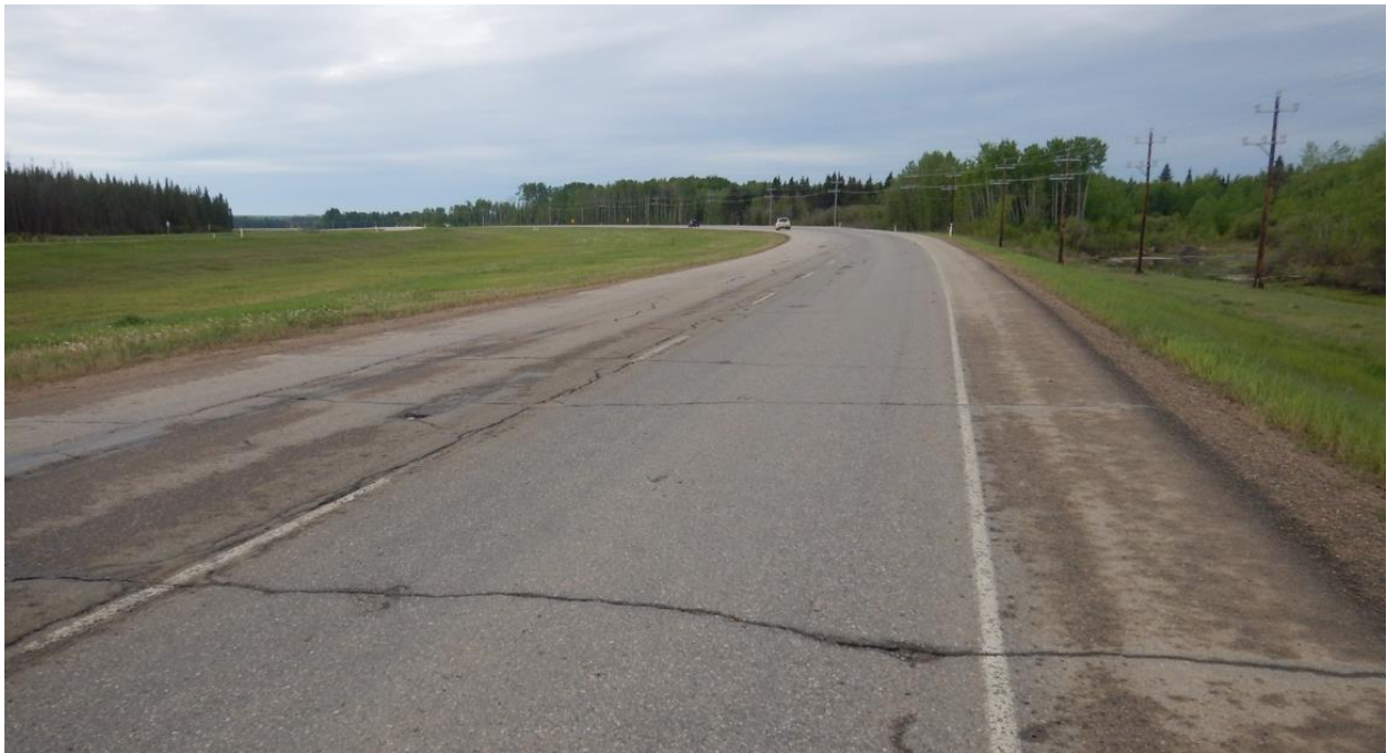
Photo No. 8 – Looking south at highway open cracks within the limits of the repaired area in 1997 (NC08-1)
