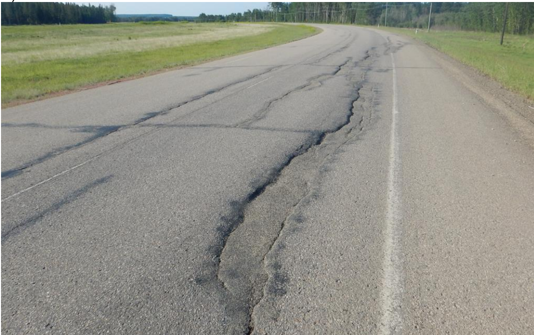
Photo No. 12 – Looking south at highway cracks near the southern flank of the south landslide (NC08-2)
