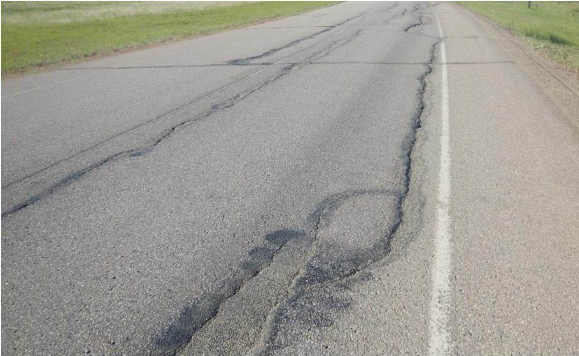
Photo No. 11 – Looking south at highway cracks at the central portion of the south landslide (NC08-2)
