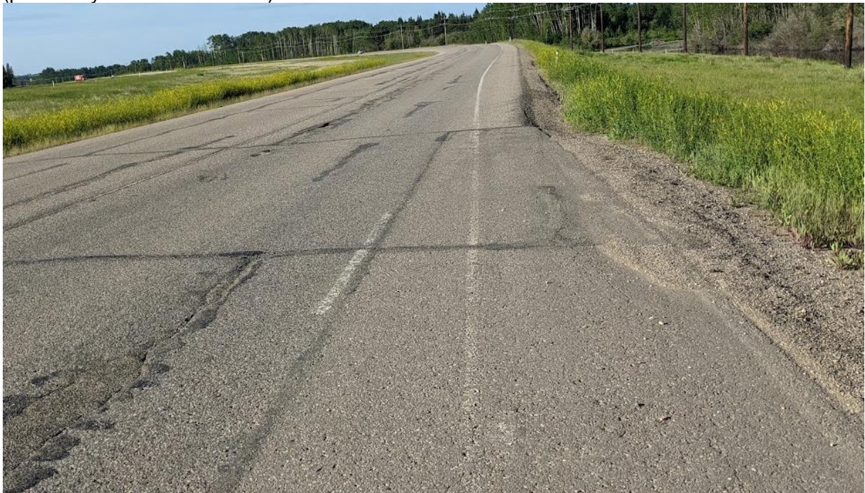
Photo No. 6 – Looking south at highway open cracks and potholes within the limits of the NC08-1 repaired area
