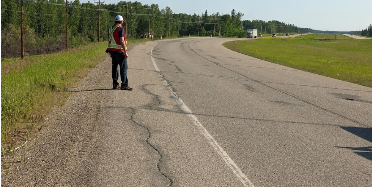
Photo No. 13 – Looking north at highway cracks near the south flank of the south landslide (NC08-2)
