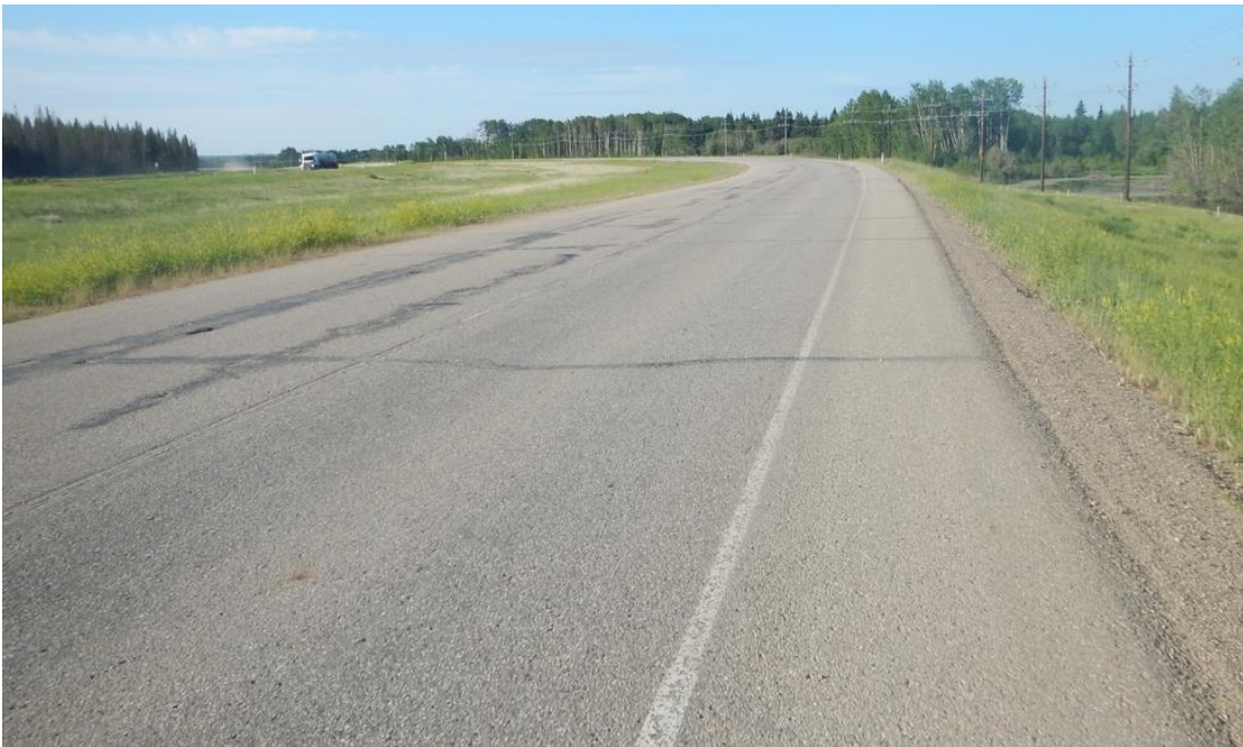
Photo No. 8 – Looking south at highway open cracks within the limits of the repaired area in 1997 (NC08-1)
