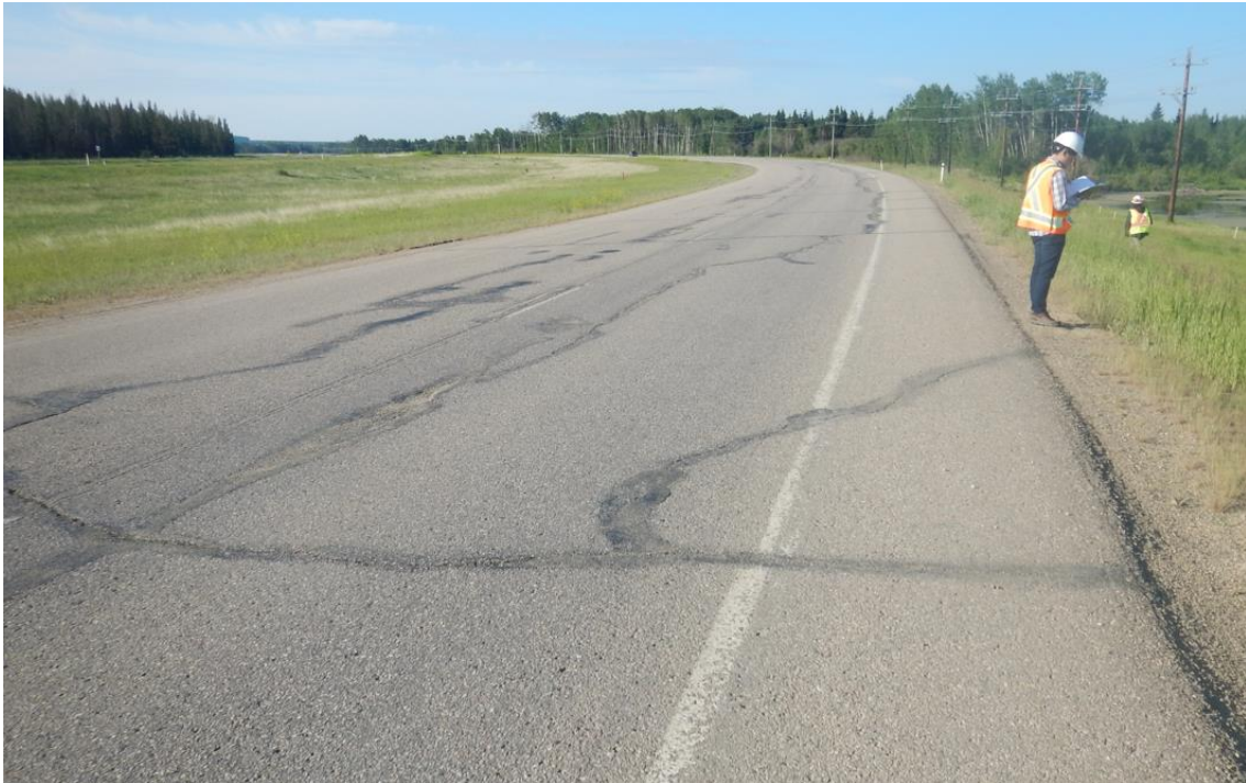
Photo No. 9 – Looking south at the southern flank cracks of the NC08-1 repaired landside. Note that cracks were spray patched in 2020
