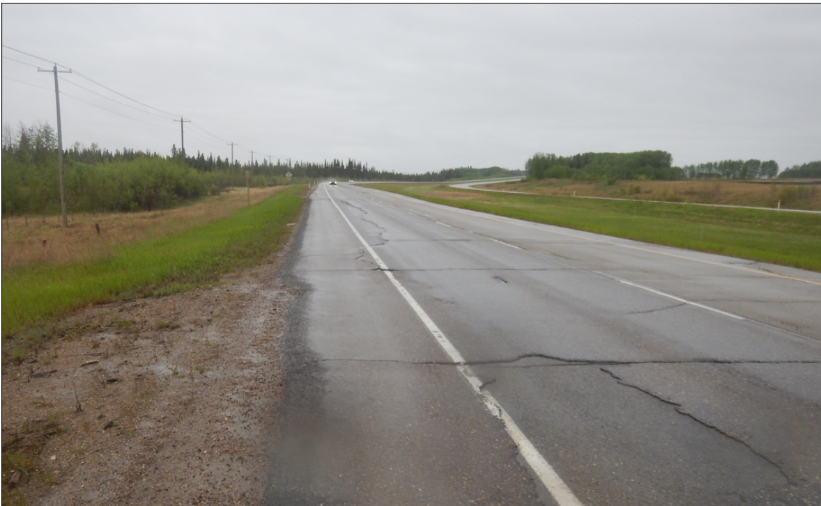
Photo No. 4 – West landslide (looking north from the southern limit of the landslide); note the dip developed on the highway surface within the limits of the landslide
