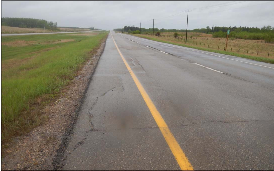
Photo No. 1 – Looking south at open diagonal and longitudinal cracks on the former highway NBL surface from the north limit of the east landslide
