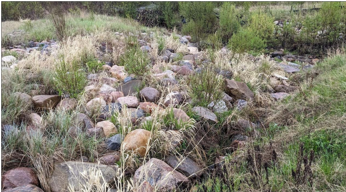
Photo No. 12 – South facing channel: Erosion gully developed on the west edge of the channel has been filled with riprap
