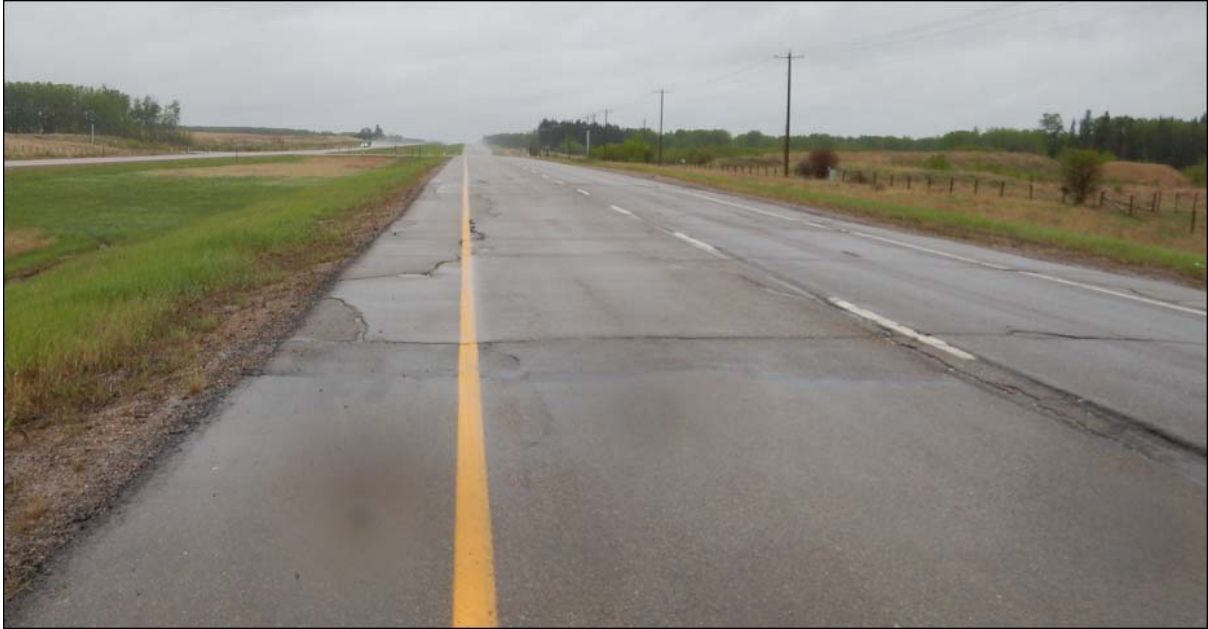
Photo No. 3 – Looking south from the southern limit of the east landslide at reflective diagonal crack on the existing patch
