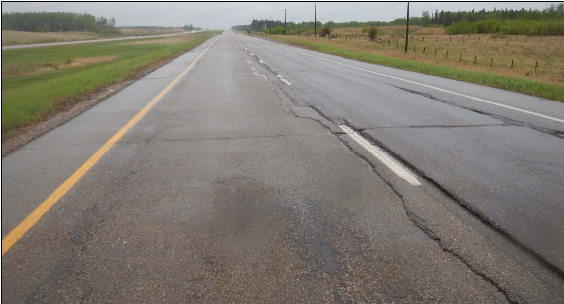
Photo No. 2 – Looking south at an open longitudinal reflective crack within the middle section of the east landslide; note the presence of a 40 mm elevation difference between the two lanes
