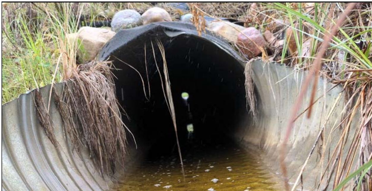
Photo No. 8 – Looking inside the outlet of the 600 mm diameter CSP culvert installed below the NBLs; water is still ponding inside the pipe
