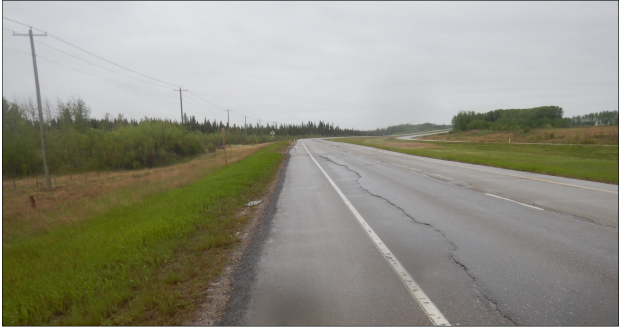
Photo No. 5 – Looking north at the west landslide reflective cracks on the highway surface
