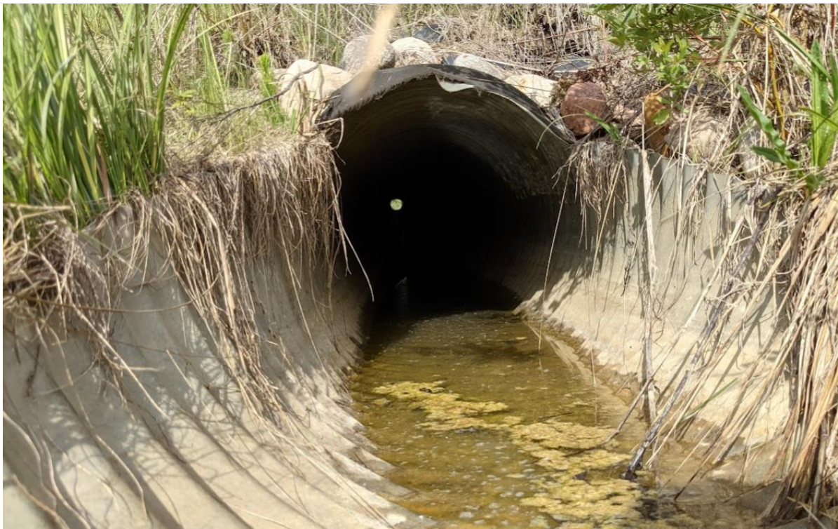
Photo No. 8 – Looking inside the outlet of the 600 mm diameter CSP culvert installed below the NBLs; water is ponding inside the pipe
