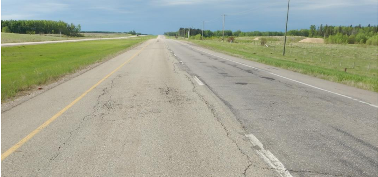
Photo No. 3 – Looking south at an open longitudinal reflective crack within the middle section of the east landslide; not the presence of a 40 to 50 mm elevation difference between the highway lanes (2015 patch created a lip between the lanes)
