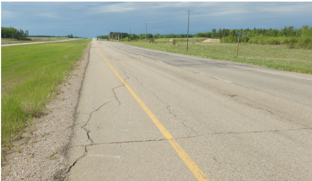
Photo No. 2 – Looking south at open diagonal and longitudinal cracks on the former highway NBL surface from the north limit of the east landslide
