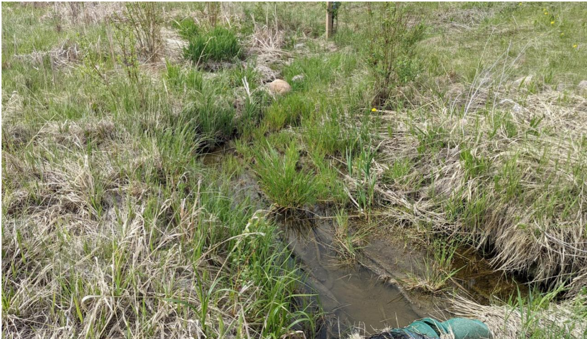
Photo No. 12 – South facing channel: erosion along the ditch (4 m long x 2 m wide x 0.6 m deep) has not significantly grown since 2020
