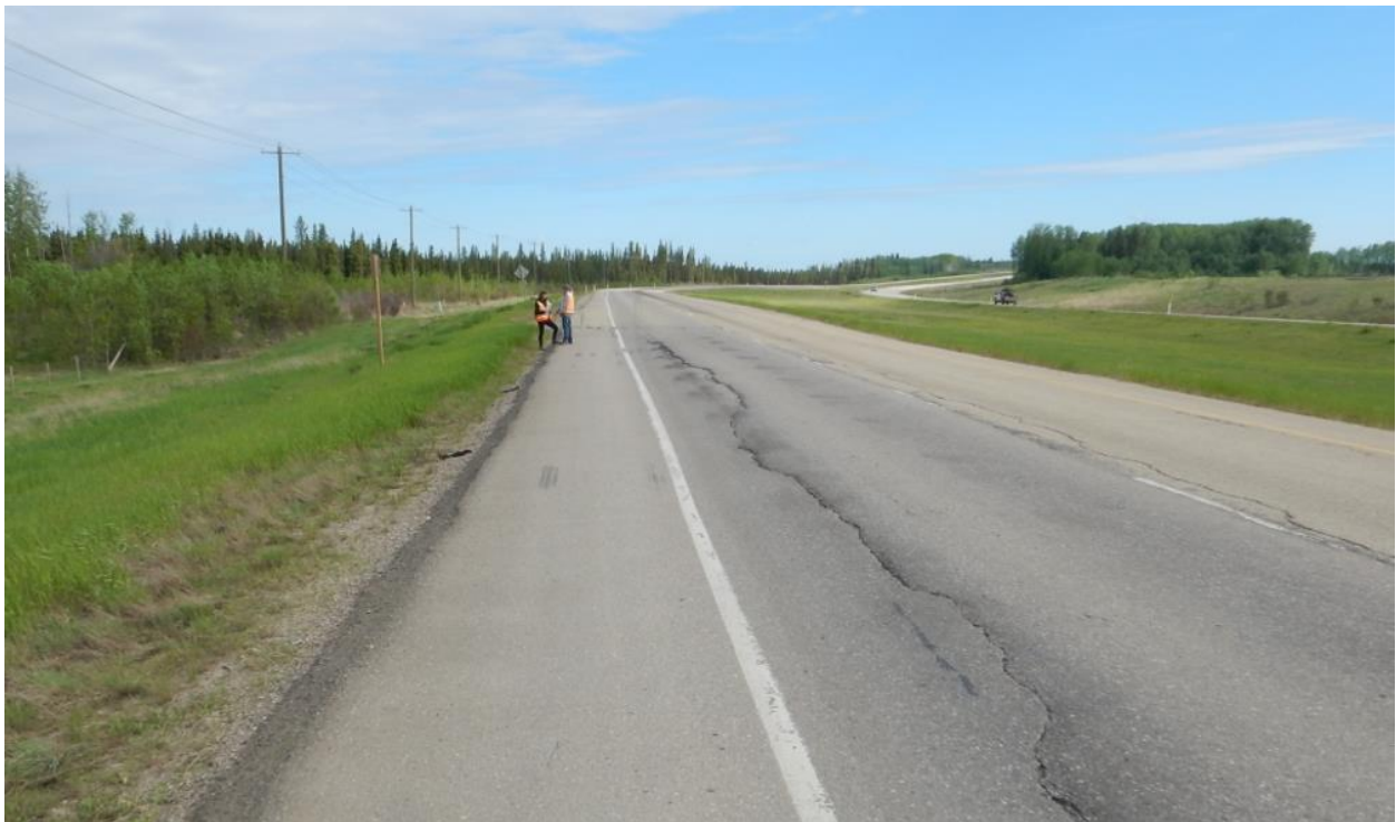
Photo No. 6 – Looking north at the east landslide reflective cracks on the highway surface
