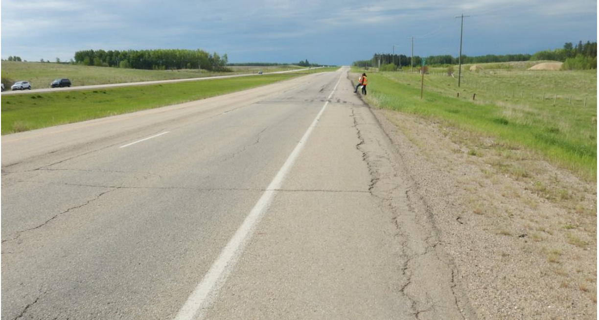
Photo No. 1 – General view of the highway SBLs condition (looking south); note presence of highway cracks (on former highway SBL) to the northern limit of the west landslide
