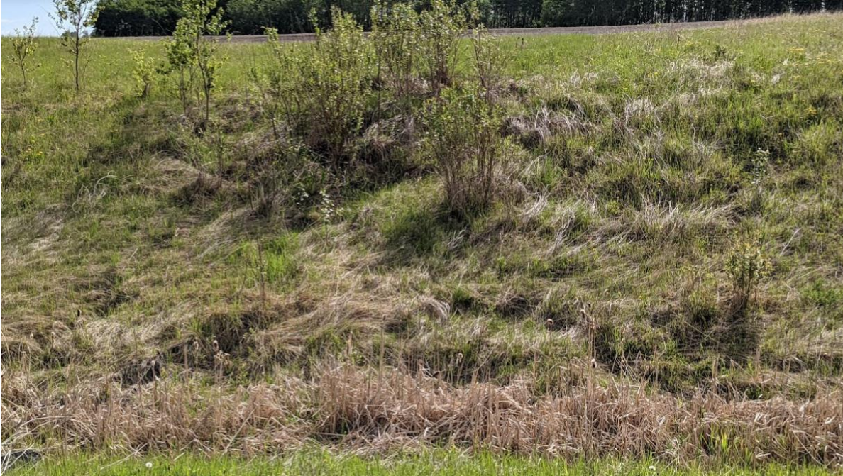
Photo No. 9 – Looking northeast at the backslope slump area observed in 2017; vegetation has grown within the slump area
