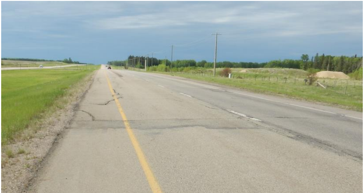
Photo No. 4 – Looking south from the southern limit of the east landslide at reflective diagonal crack on the existing patch
