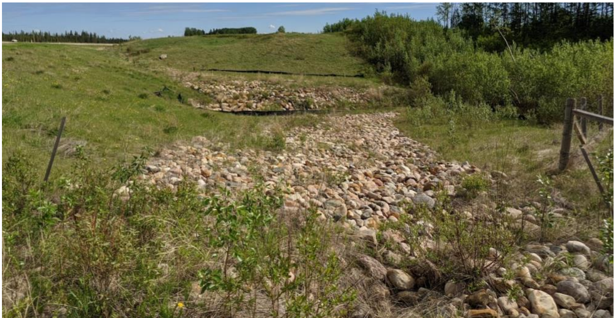
Photo No. 14 – looking northeast along the riprap lined north facing drainage channel
