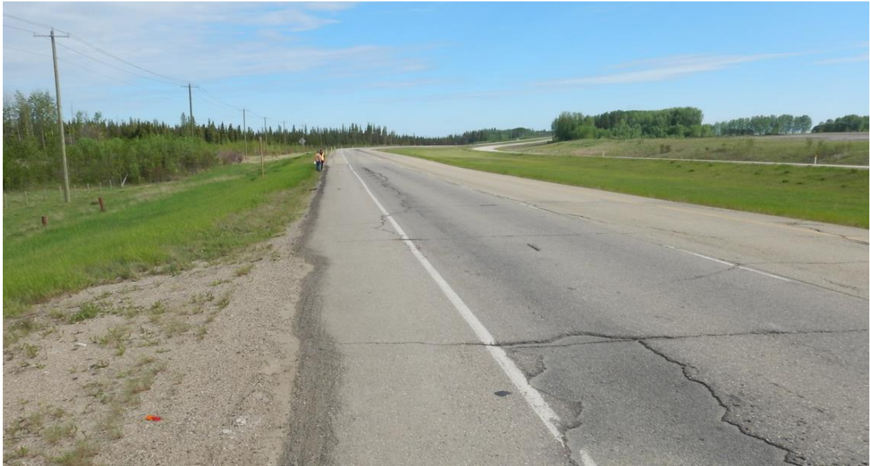
Photo No. 5 – East landslide (looking north from the northern limit of the landslide)
