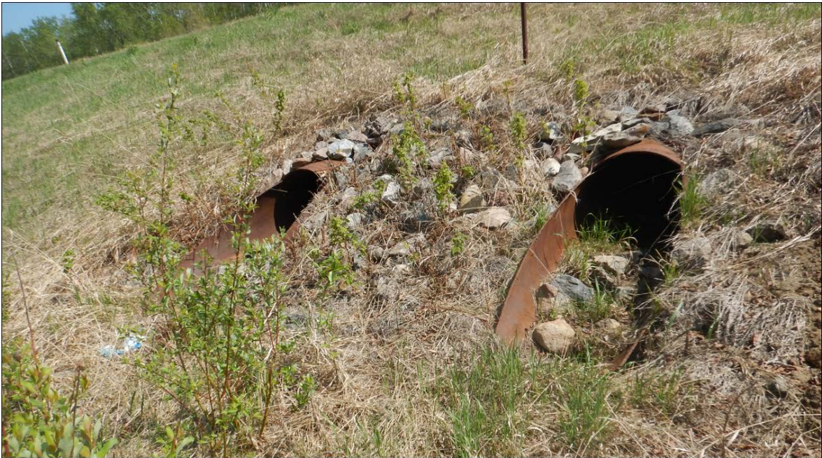
Photo No.2 - Looking northeast at the twin culverts outlets; Sediment and silt fence cleared; no flow in 2023
