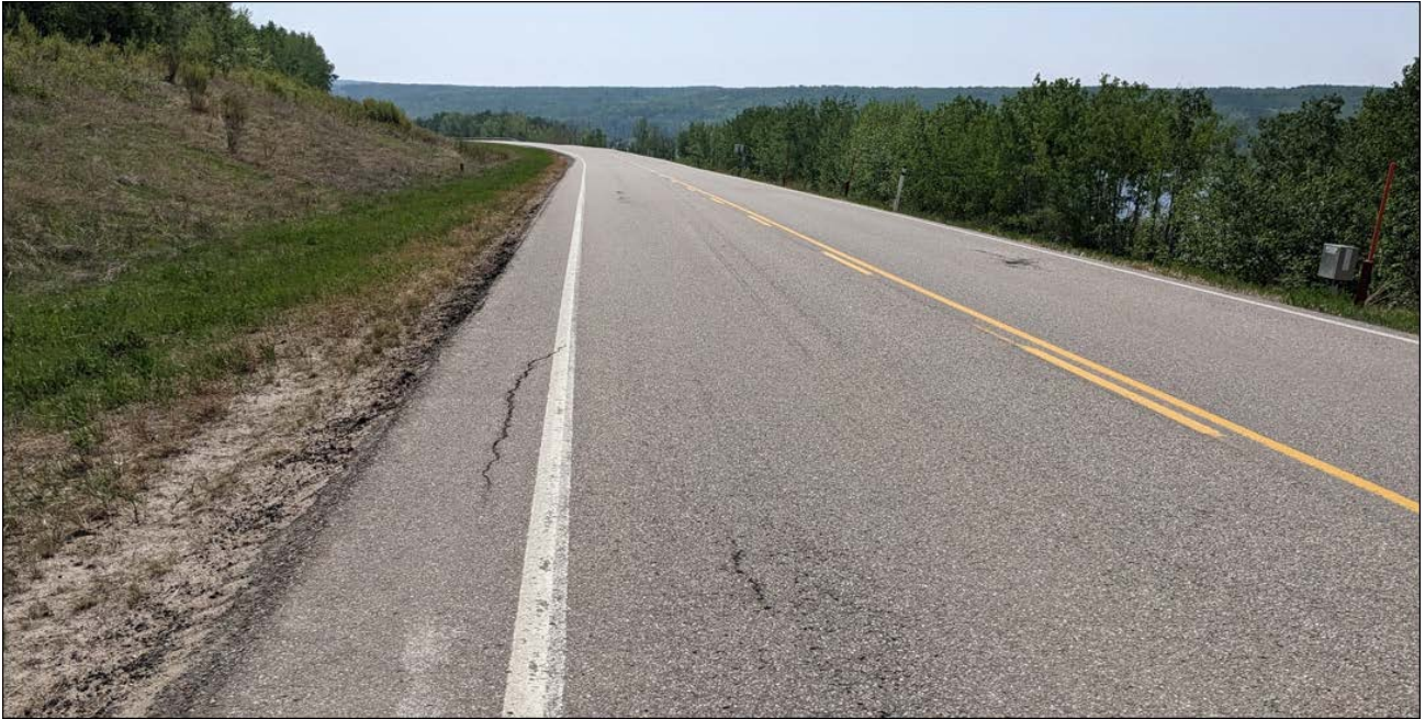
Photo No.7 – Looking south at reflective cracks 10 to 20 mm wide, no drop
