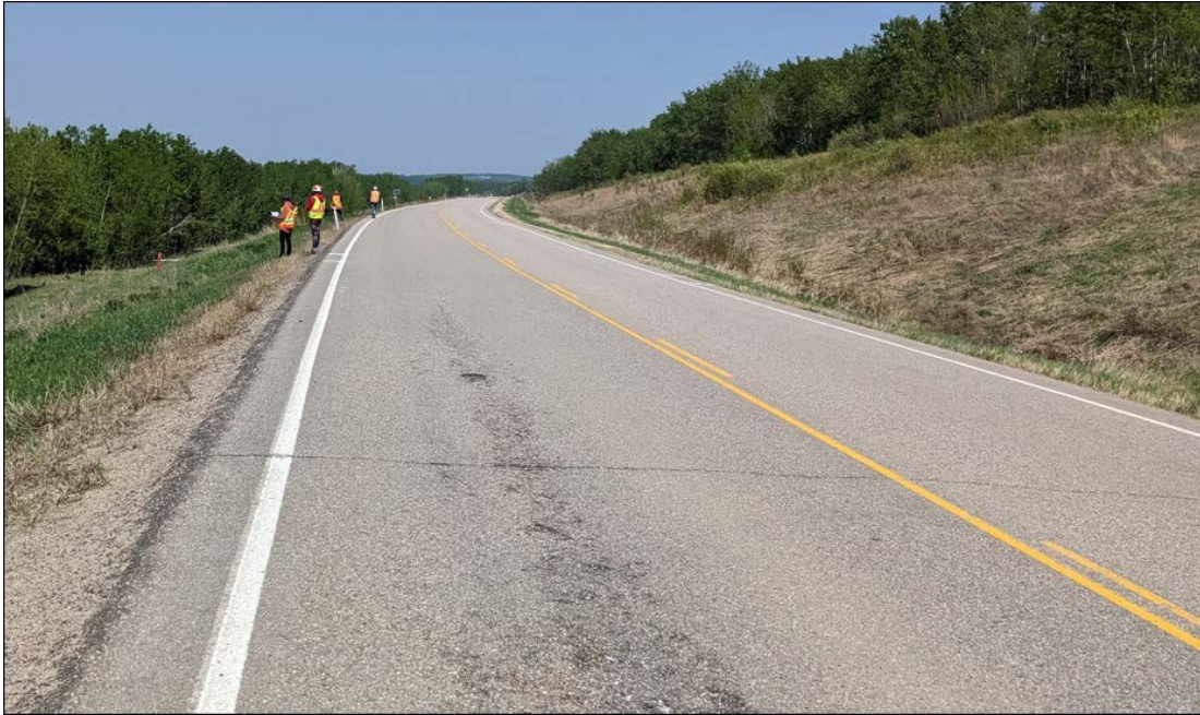
Photo No. 1 - Looking north at highway surface; no reflective cracks or dips noted at the south end of the site
