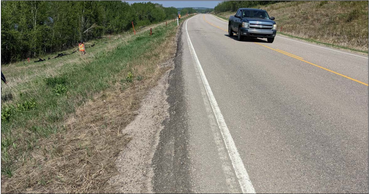
Photo No.5 – Looking north at sharp shoulder drop off on the west side slope
