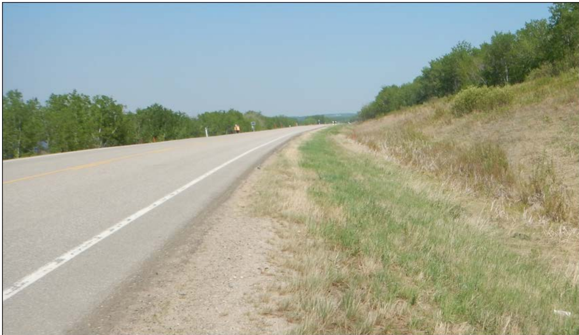
Photo No.4 - Looking north at the TRM lined ditch; no water flowing; note cattails in the ditch area
