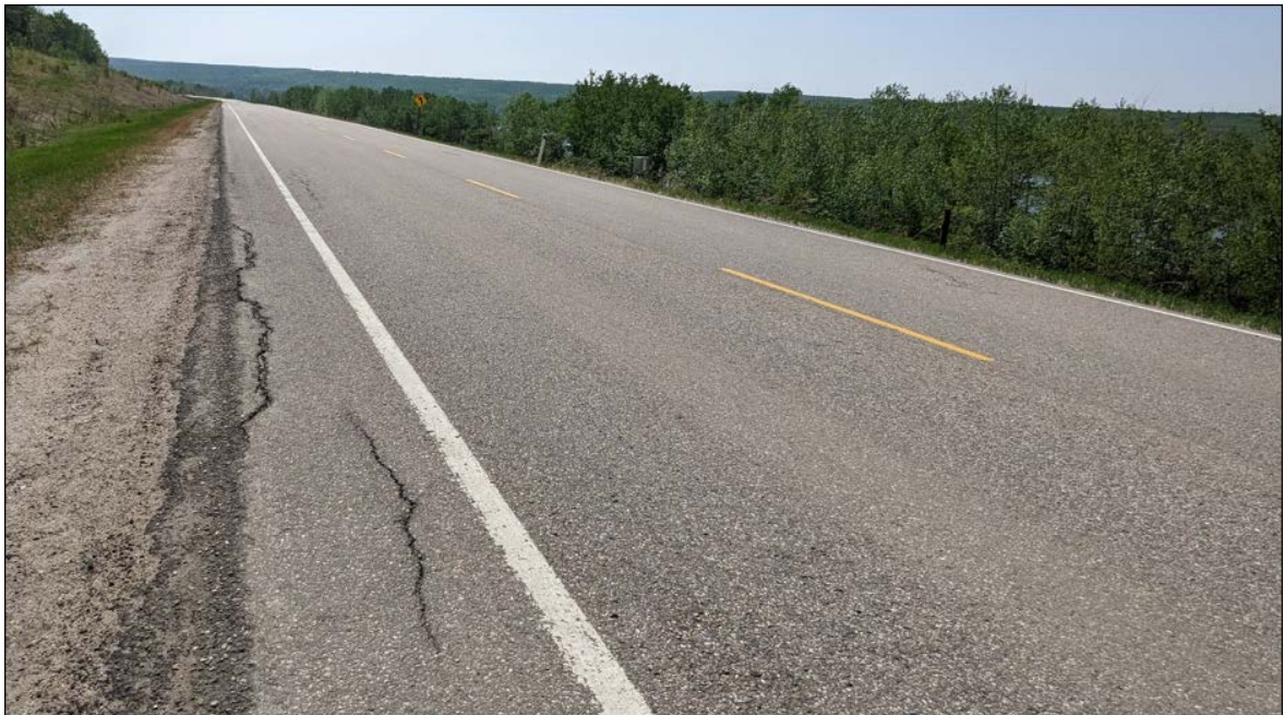
Photo No. 8 – Looking south at reflective cracks 10 to 20 mm wide, no drop
