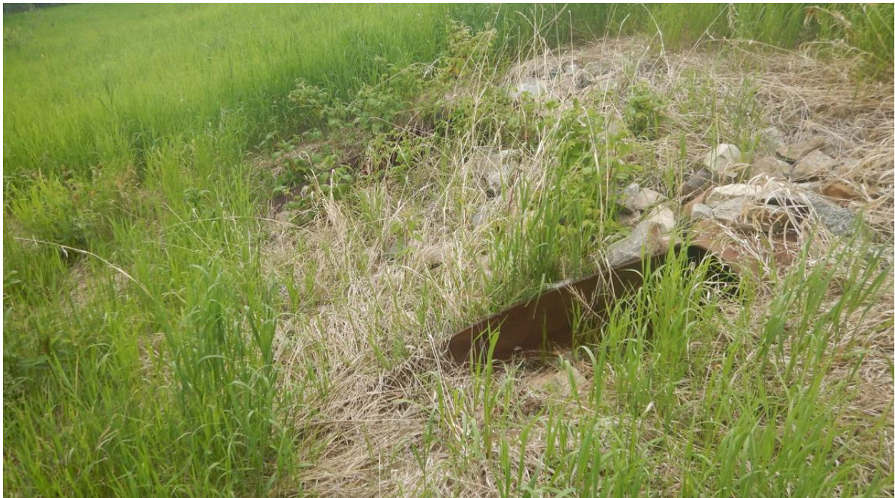
Photo No.2 - Looking northeast at the twin culverts outlets; Sediment and silt fence cleared; no flow in 2021
