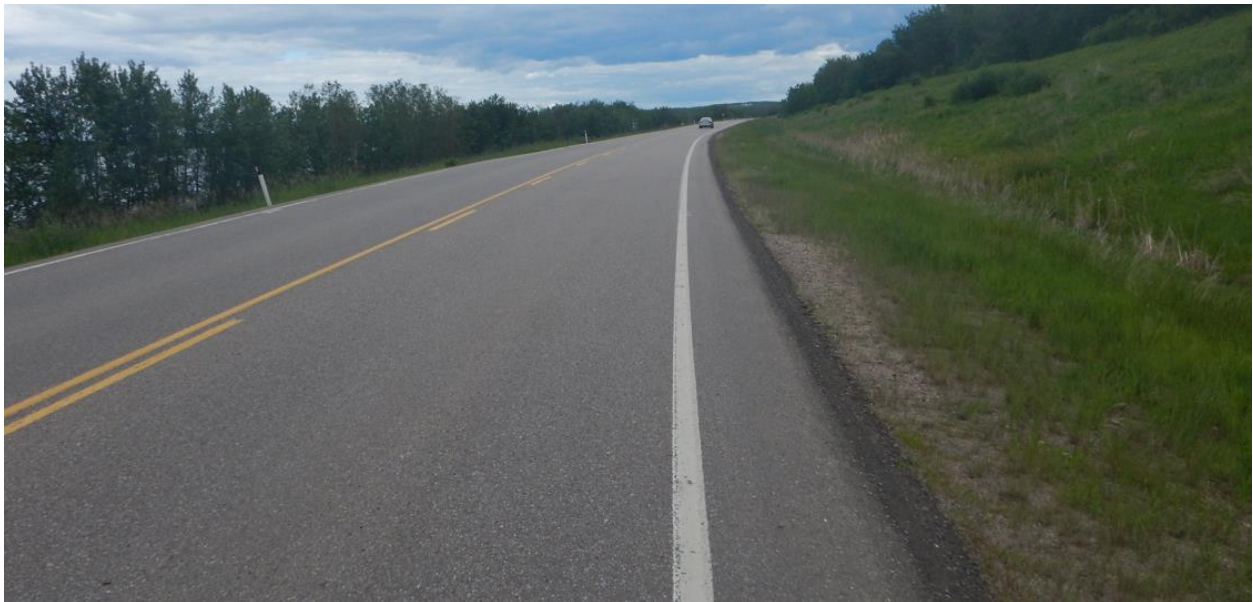
Photo No.4 - Looking north at the TRM lined ditch; no water flowing; note cattails in the ditch area
