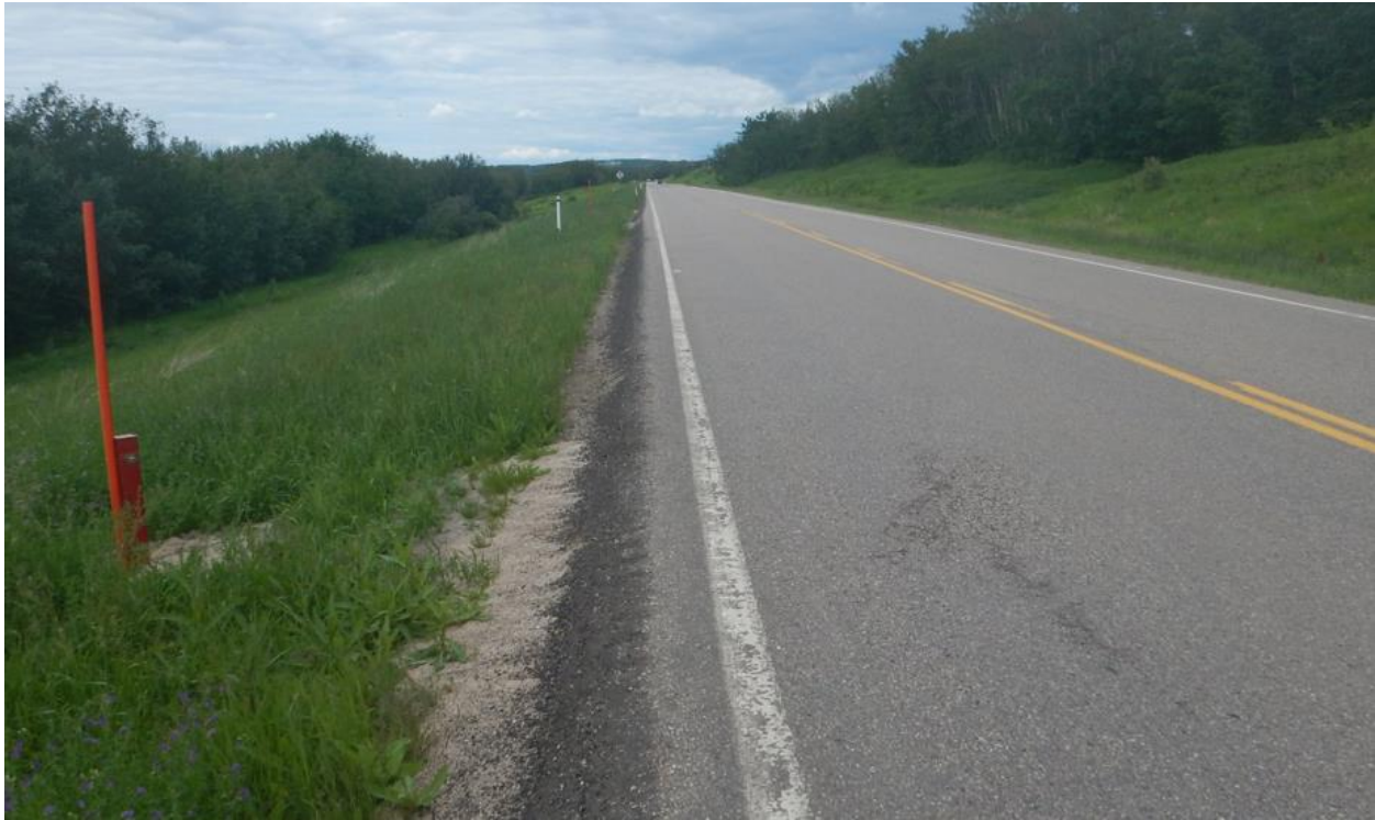
Photo No.7 – Looking north at sharp drop off shoulder on the west side slope
