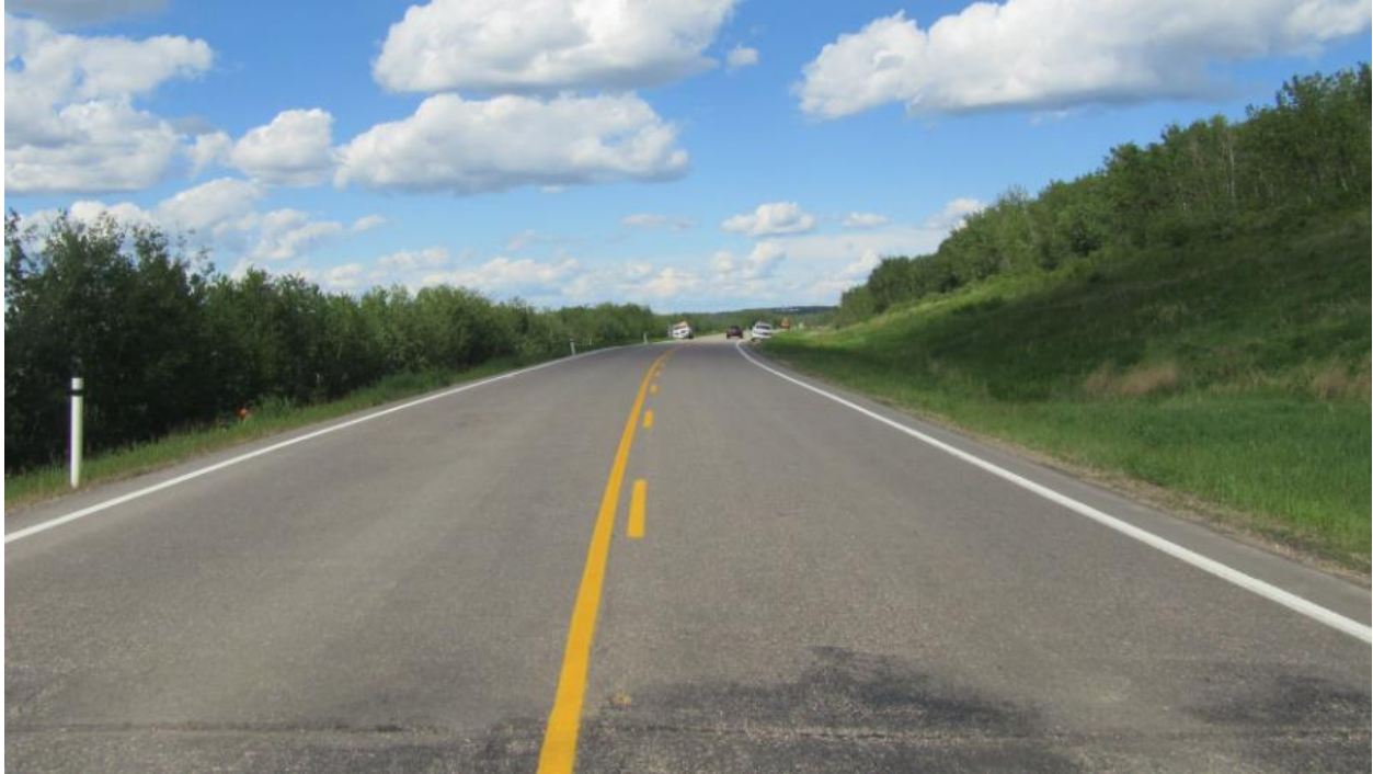
Photo No. 1 - Looking north at highway surface; no reflective cracks or dips noted in 2019
