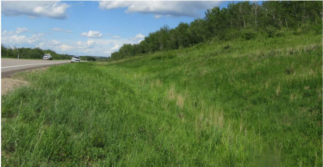
Photo No.3 - Looking north at the TRM lined ditch; water flows south towards the twin culverts and vegetation grew in the ditch and backslope
