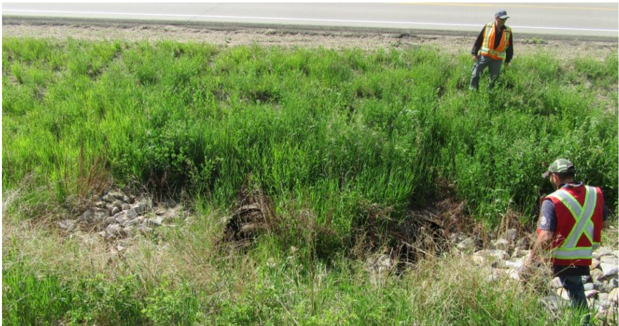
Photo No.2 - Looking at twin culverts (northwest); water flows into most eastern pipe
