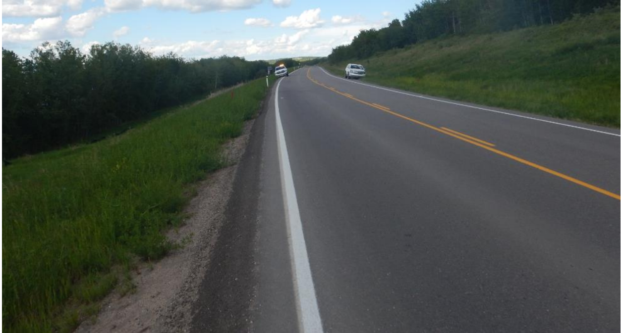
Photo No.5 - Looking north at a sharp drop off along the western edge of the road; vegetation grew on the highway side slope
