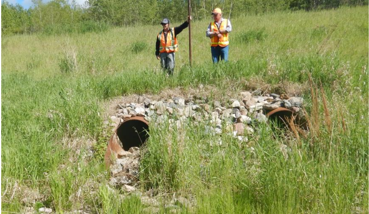
Photo No.7 - Looking at the outlets of the twin culverts; water flows downstream of the pipes toward the bush
