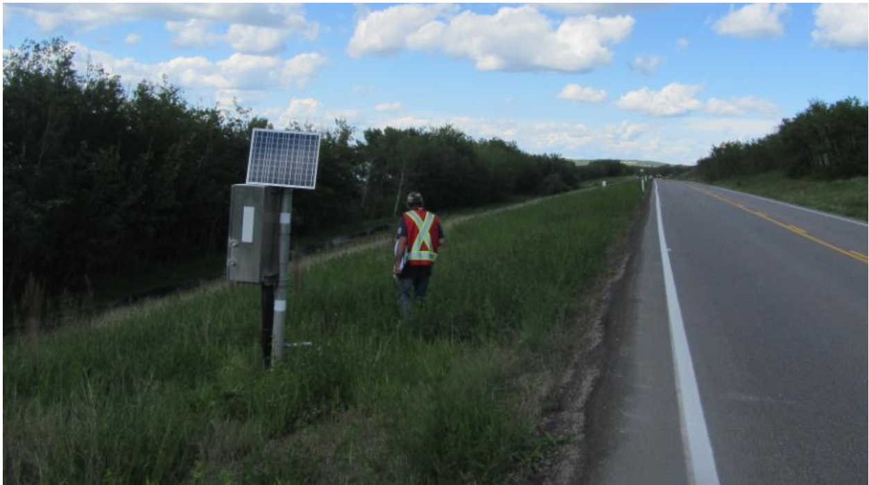
Photo No.6 - Looking at data logger DT1 installed at pile 146 location; vegetation grew at previously noted subsidence at the base of the data logger
