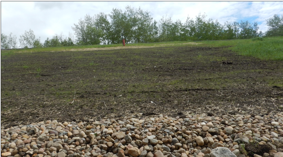
Photo No. 5 – Looking east at the area of the 2024 slump repairs downslope of the pile wall location.
