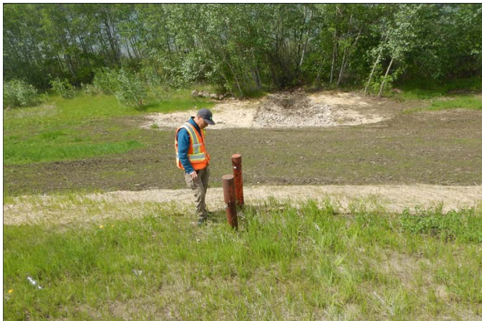
Photo No. 3 – Looking west at the area of the 2024 slump repairs downslope of the pile wall location. Note vegetation starting to grow between the pile wall and the riprap channel
