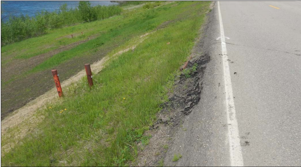
Photo No. 2a – Looking at the highway northwest side slope upslope of the 600 mm CSP culvert outlet location. Asphalt surface outside of the white line was likely damaged during construction
