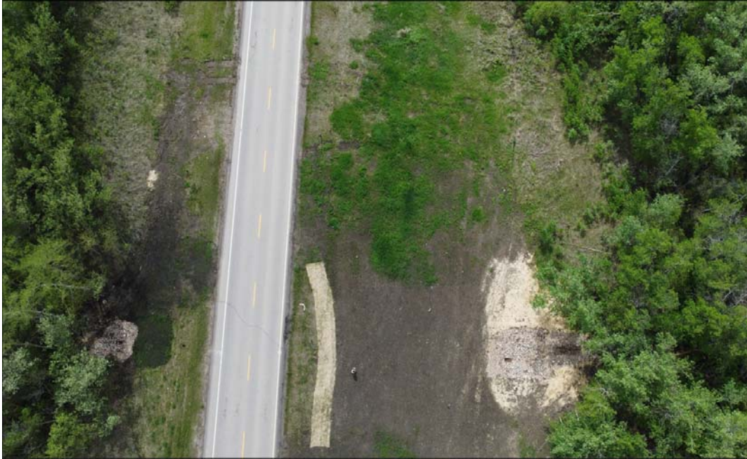
Photo No. 6 – Aerial photo covering both sides slopes of the highway and the extent of the 2024 repairs completed by In-Line Construction
