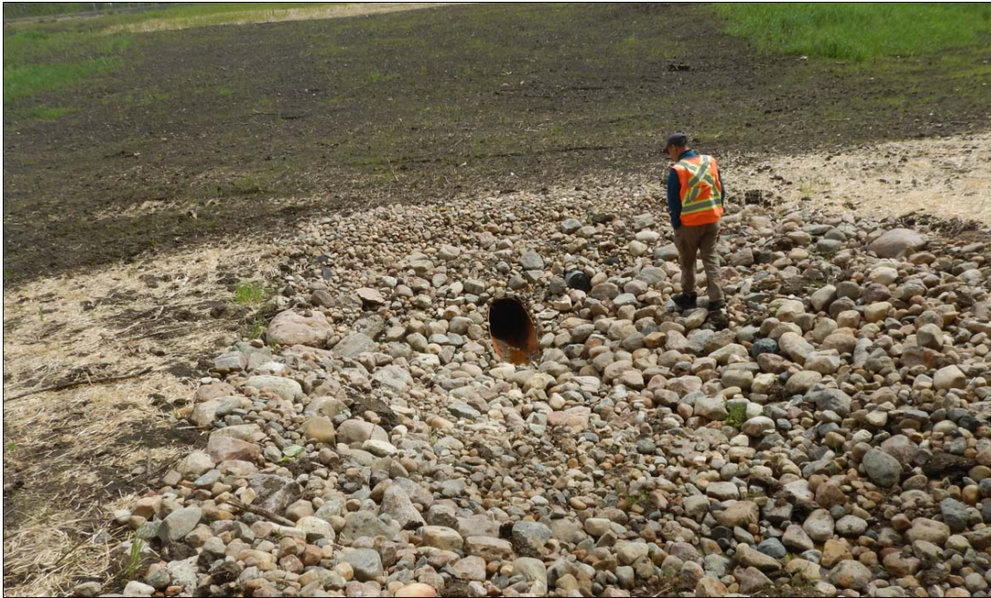
Photo No. 4 – Looking east at the new SWSP culvert outlet downslope of the pile wall location
