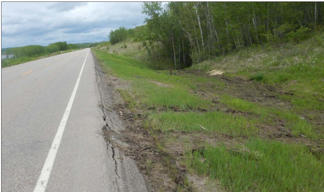
Photo No. 2 – Looking at the highway southeast side slope upslope of the 600 mm CSP culvert inlet location. Note asphalt surface outside of the white line was damaged during construction
