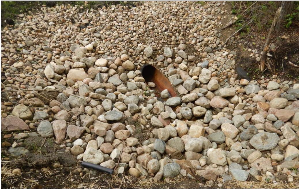
Photo No. 1 – Old 600 mm CSP Centre-Line Culvert was lined with 500 mm SWSP Culvert in the Spring of 2024
