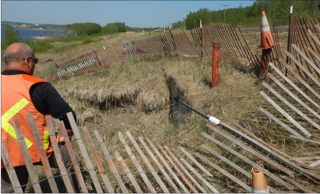
Photo No. 3 – Looking northeast at the slump downslope of the pile wall location
