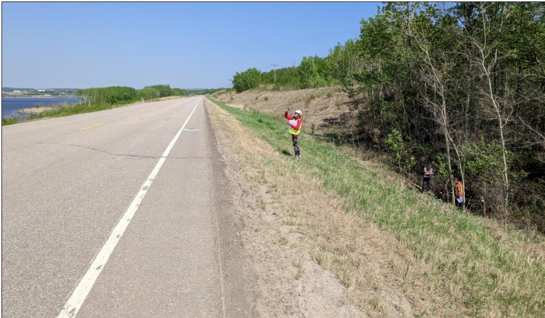
Photo No. 2 – Looking at the highway southeast side slope upslope of the 600 mm CSP culvert inlet location
