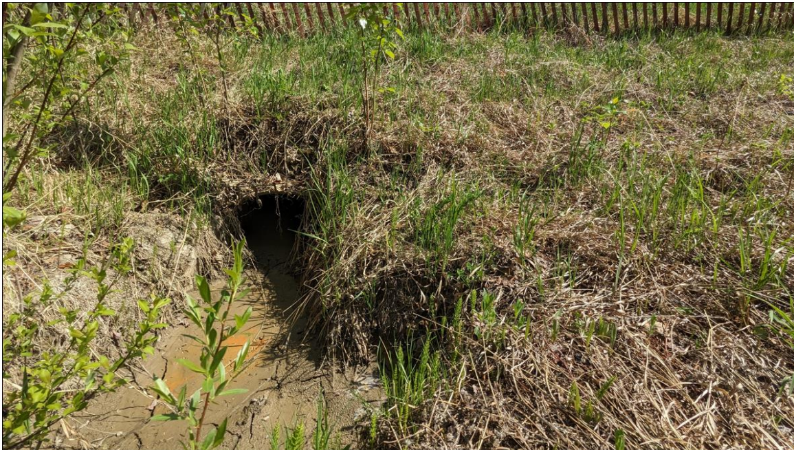
Photo No. 6 – Culvert outlet partially filled with sediment. No flow observed in 2023.
