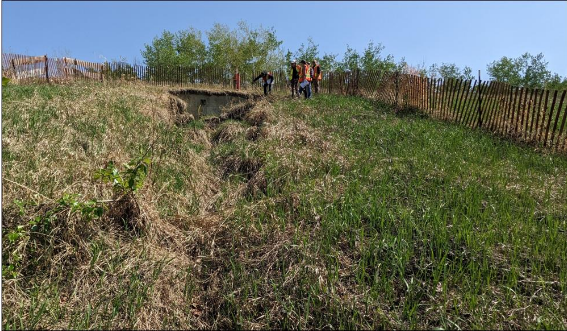
Photo No. 5 – Looking southeast at the head scarp crack of the slump; the slump exposed the waler and a couple of anchor caps.
