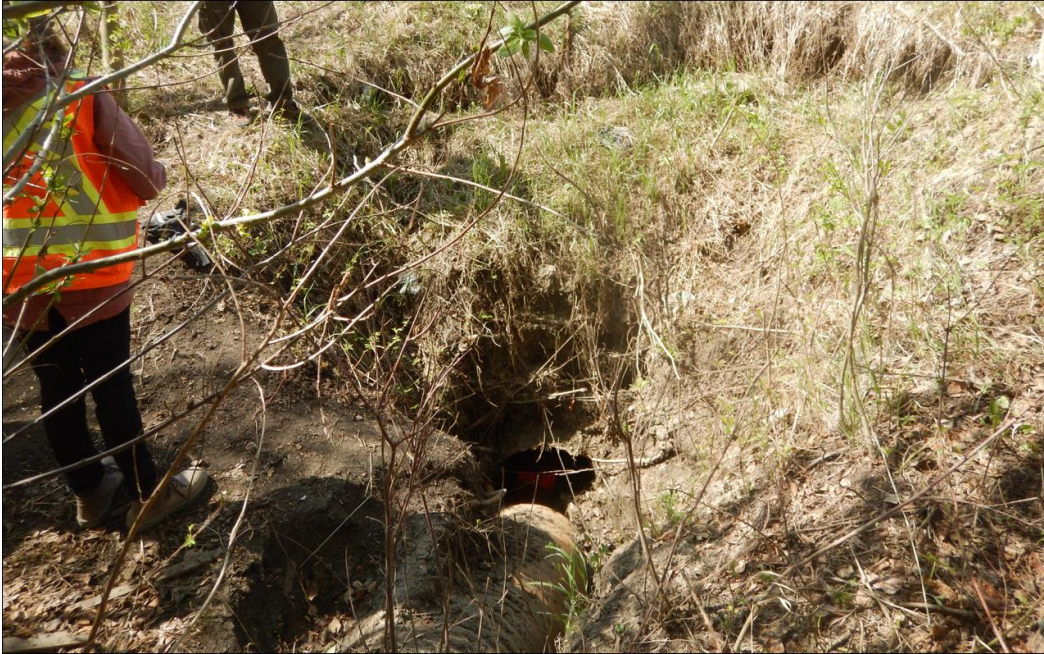
Photo No. 1 – 600 mm CSP culvert inlet got separated, resulting in a sinkhole and a slump at the bottom of the highway side slope.
